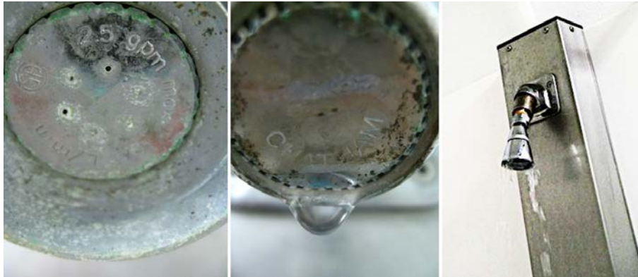
Figure 13. Examples of excessive mineral (calcium/lime) buildup in showerheads, showerhead leaks, and malfunctions.
