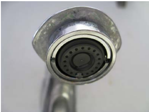
Figure 36. New 0.35 gpm aerator installed.
