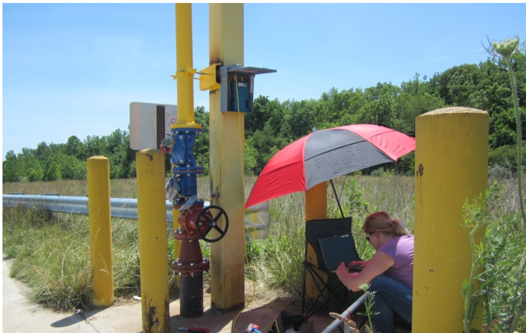
Figure 53. Flow recorder installed at bulk water station.
