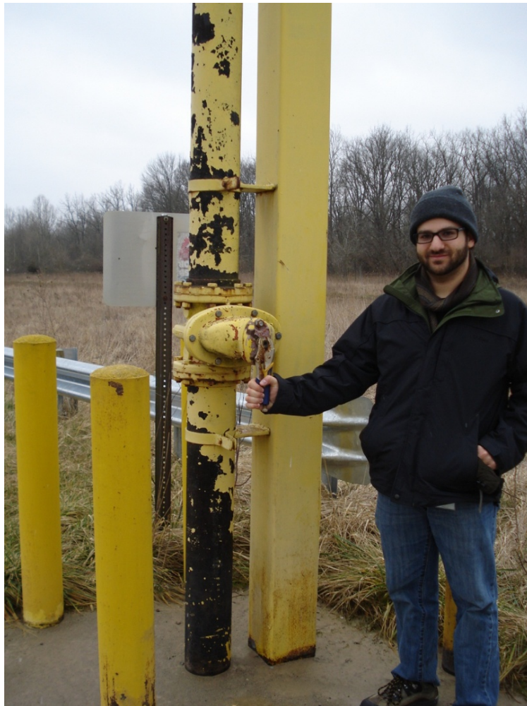
Figure 21. Bulk water station at Schoolhouse Road before retrofit.
