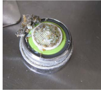
Figure 34. Corroded 0.5 gpm faucet aerator.
