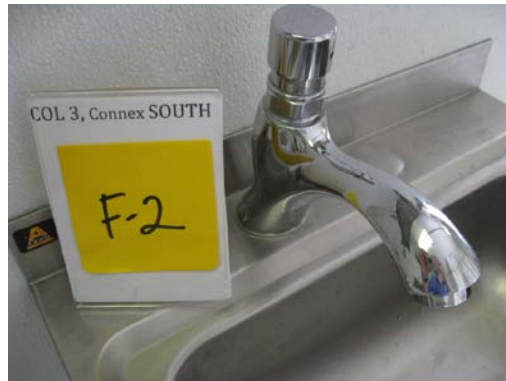
Figure 37. Retrofitted metering faucet.
