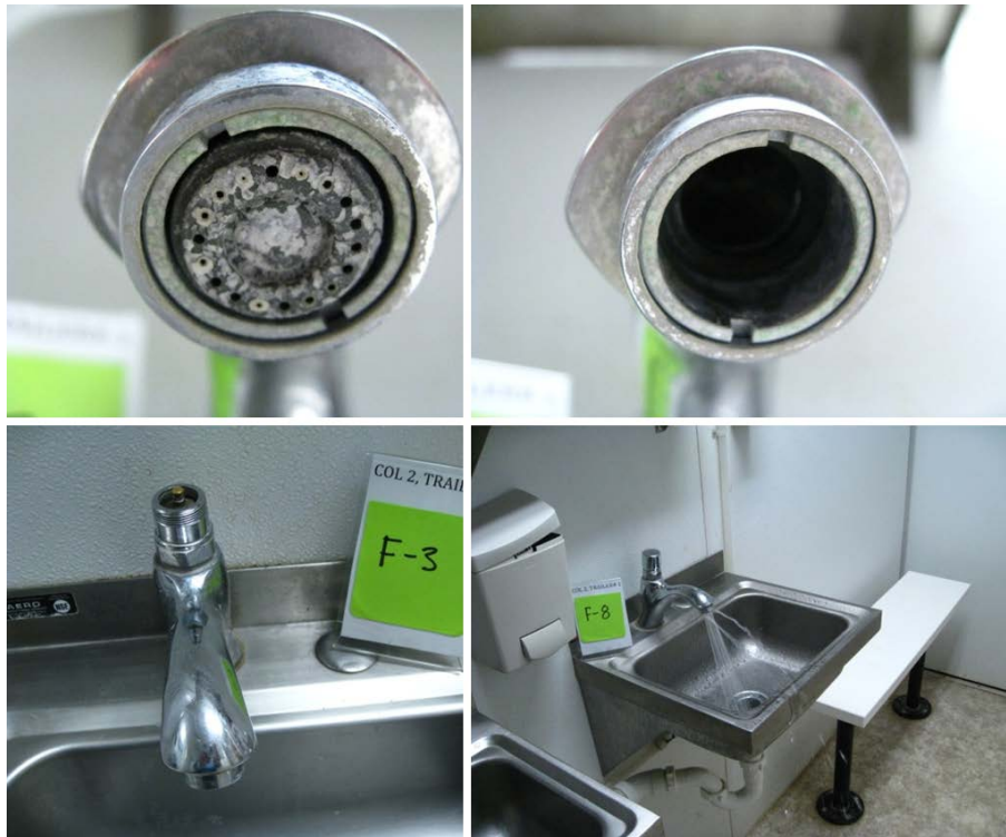
Figure 14. Examples of excessive mineral (calcium/lime) buildup in faucets, broken faucets, and sink overspray.
