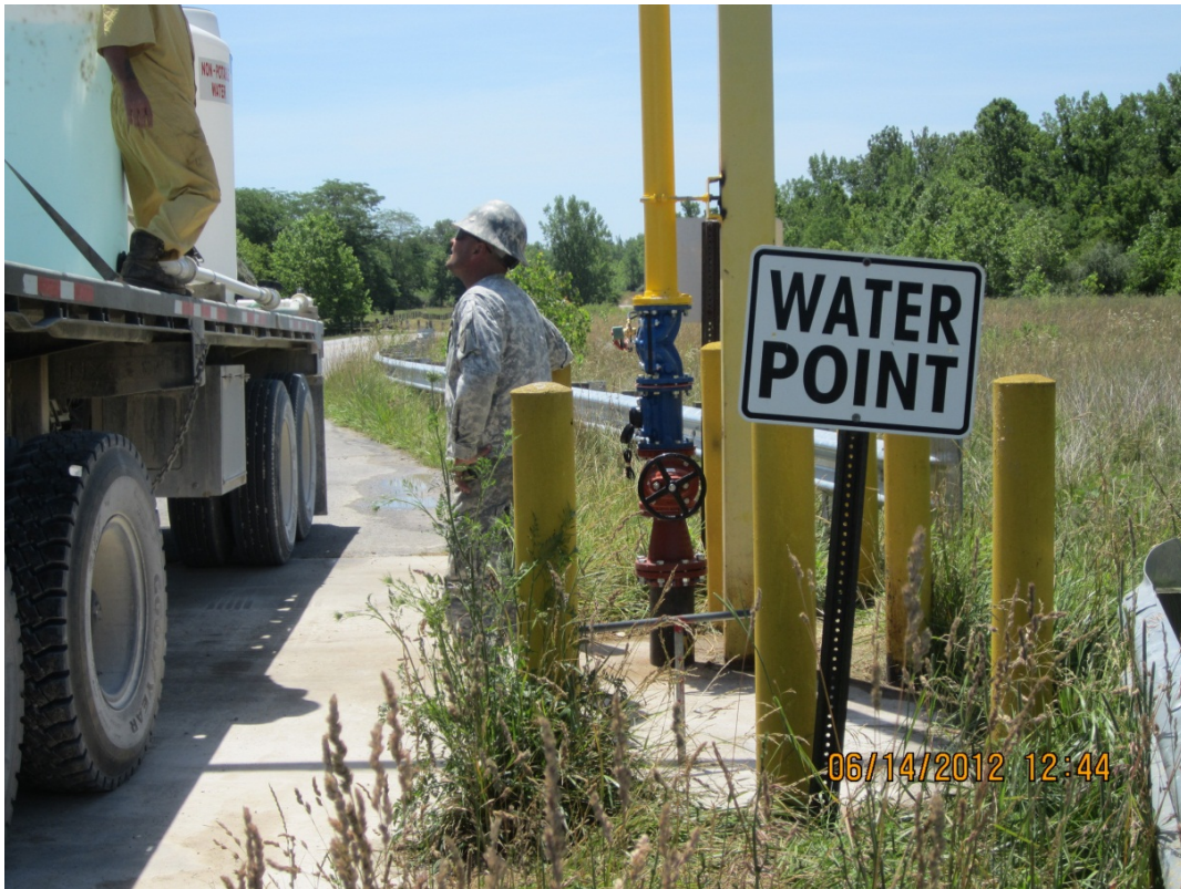
Figure 40. Bulk water station after first phase retrofit.
