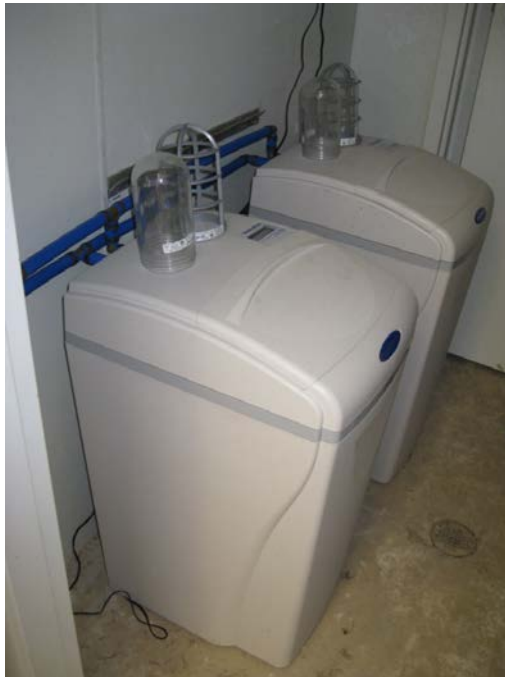
Figure 28. Water softener as seen in ReMS utility room.
