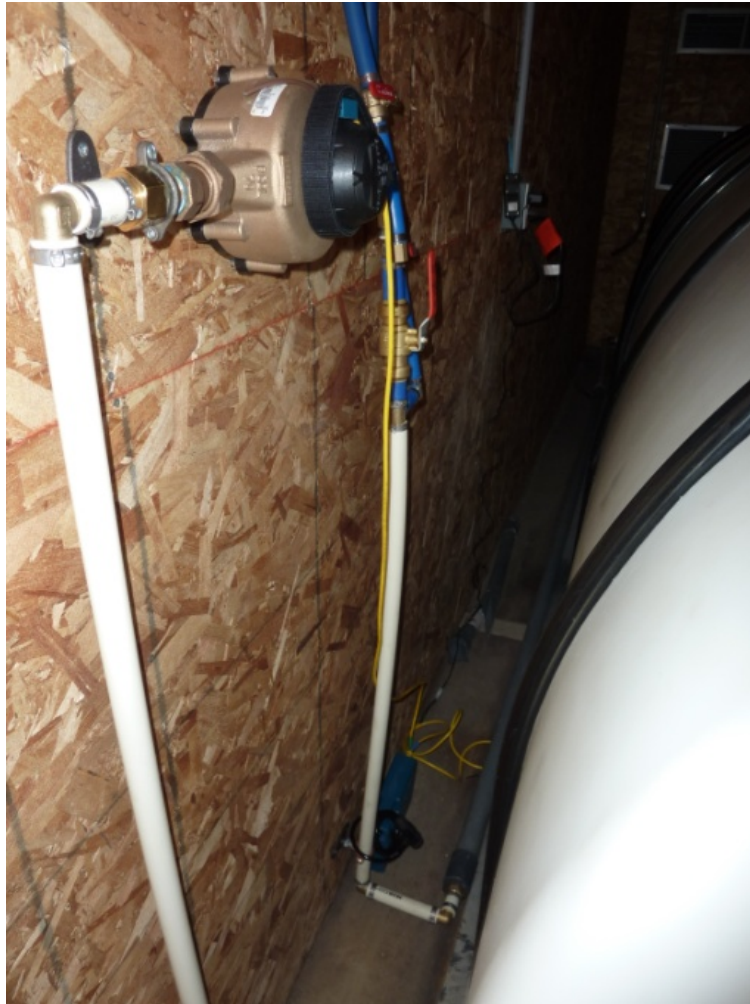
Figure 6. Bulk water tank in FOB 2 ReMS.
