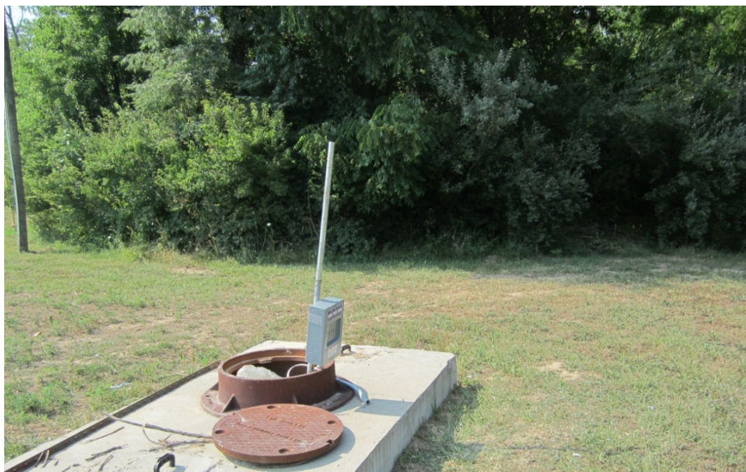
Figure 54. Flow recorder installed at the FOB 3 water meter.
