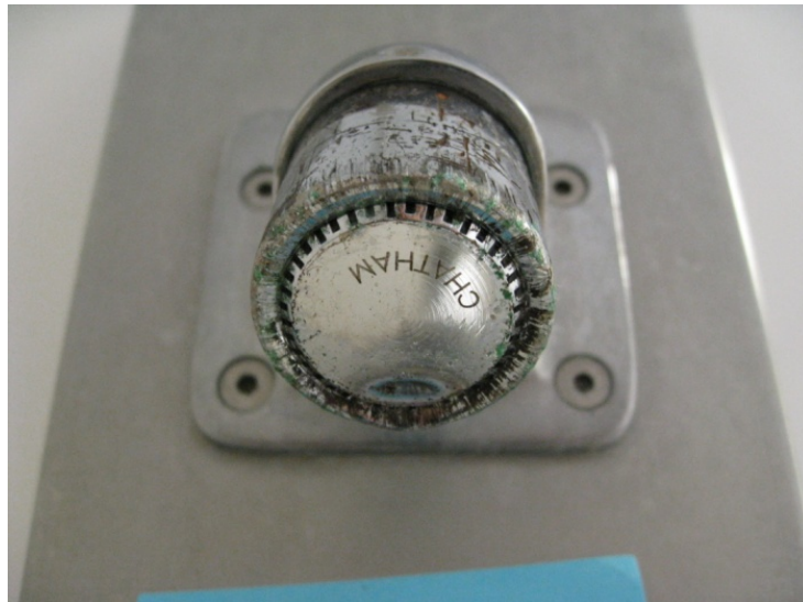
Figure 30. Showerhead after installation of water softener.
