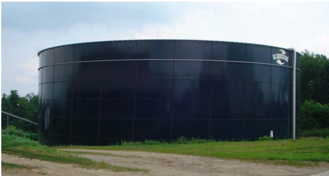
Figure A-7. View of the digestate feeding tank.
