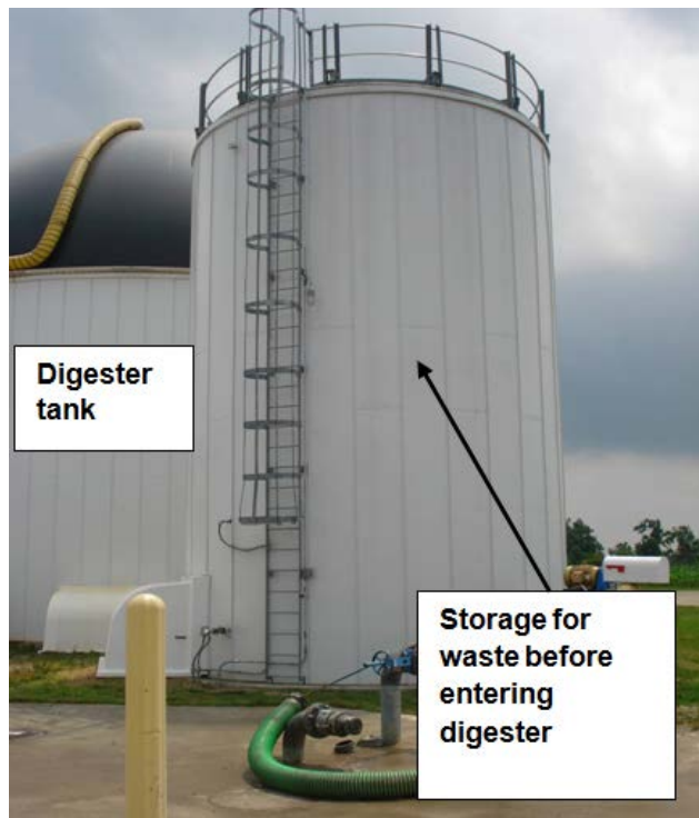
Figure A-3. View of the digester tank and storage tank.
