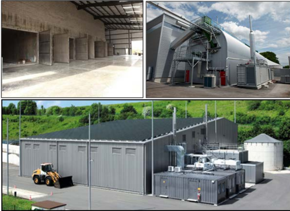
Figure 2-1. Top left, Interior of a food waste digester at the UWO Photo Gallery — Biodigester 2011). Top right, dry digester by Kompogas (German Biogas Industry 2013). Bottom, dry digester by BIOFerm (Ecopolis).
