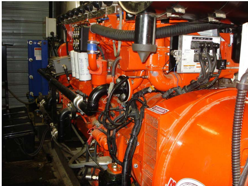
Figure A-11. The biogas was used to power a 300 kW generator. This generator was undersized and there were plans to replace it with a 500 kW generator. This generator was designed to run on biogas.
