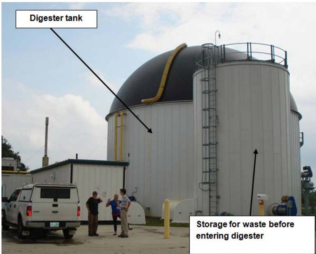
Figure A-6. View of the digester. The people in the foreground give a reference to the size of the system.
