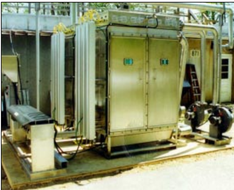
Figure 18. 650 SCFM PPCU equipment setup.
