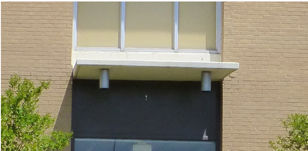
Figure 72. Ceiling-mounted light fixture placed on the underside of the flat concrete canopy, Building 29801, Nelson Hall (ERDC-CERL, 2015).
