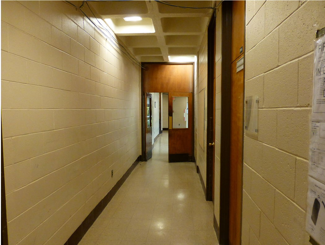
Figure 127. Example of painted exposed concrete block walls, painted exposed waffle ceiling, and vinyl composition tiled floor in classroom building hallways (ERDC-CERL, 2015).
