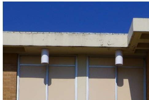
Ceiling-mounted light fixture under the waffle overhang on the east and west elevations.
