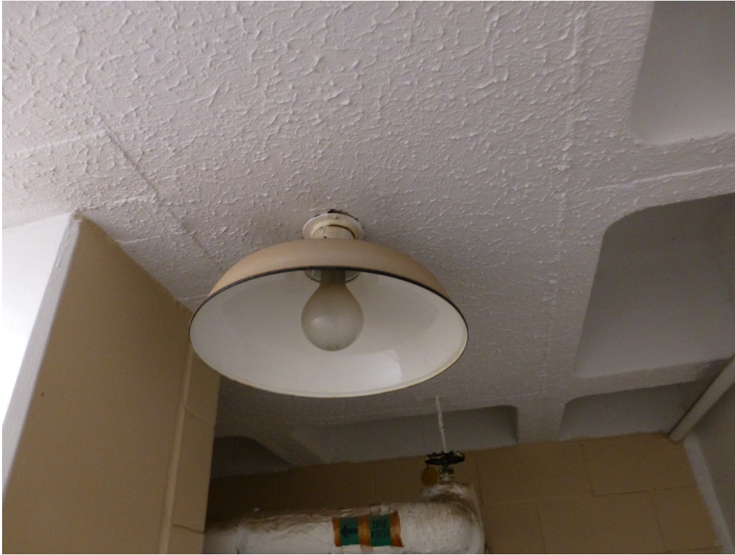
Figure 145. Typical original ceiling-mounted pendant light fixture (ERDC-CERL, 2015).
