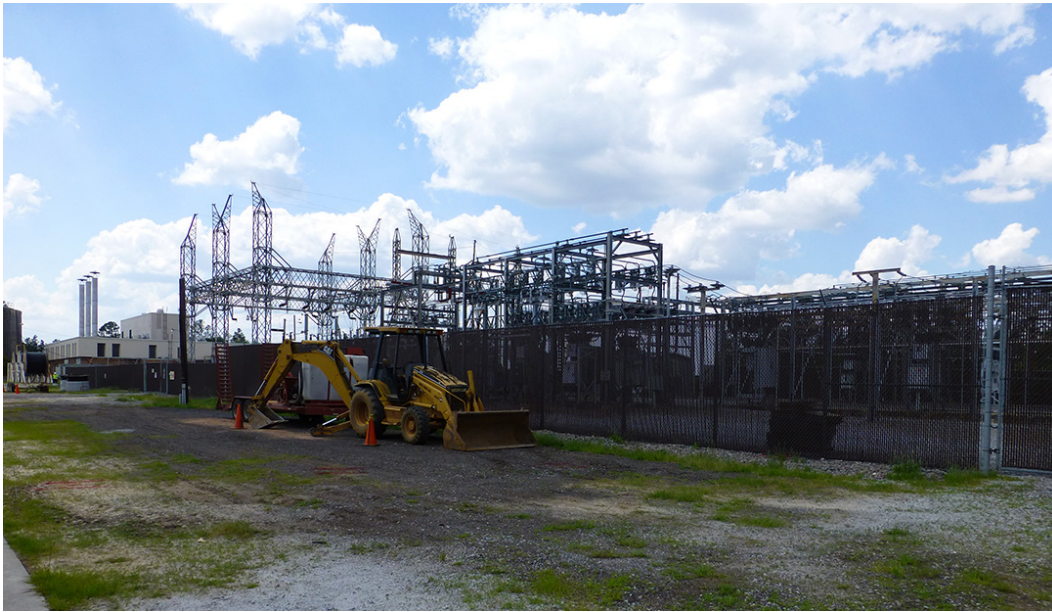
Figure 463. An electrical substation was added to the complex in 1975 (ERDC-CERL, 2015).
