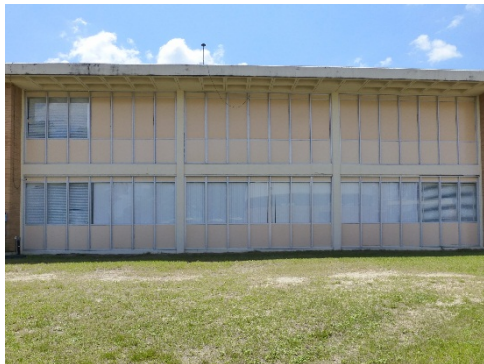
Groups of windows; bright-aluminum frame with fixed panes and insulated panels divided by concrete columns and beam. *Note: the removal of the second-floor windows replaced with new panel inserts.
