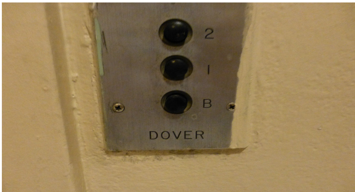
Figure 167. Close-up of the push-button mechanism to run the dumbwaiter (ERDC-CERL, 2015).
