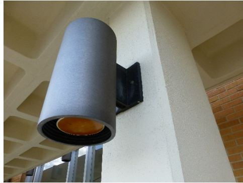
Wall-mounted bronze cylinder light fixtures near main entry.
