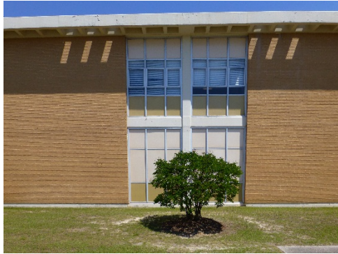
Window bays on the south elevation and "light pattern" cast from the perforated waffle roof overhang.
