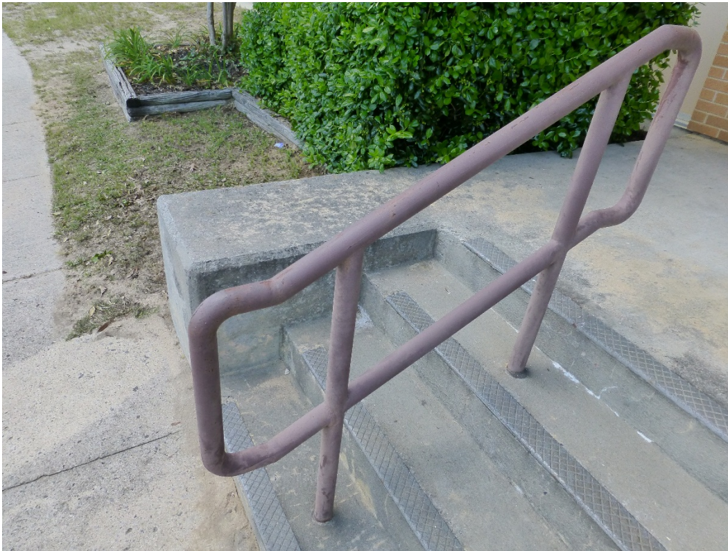
Figure 86. Example of the metal pipe handrail located near the entries for Building 25810, Brant Hall (ERDC-CERL, 2015).
