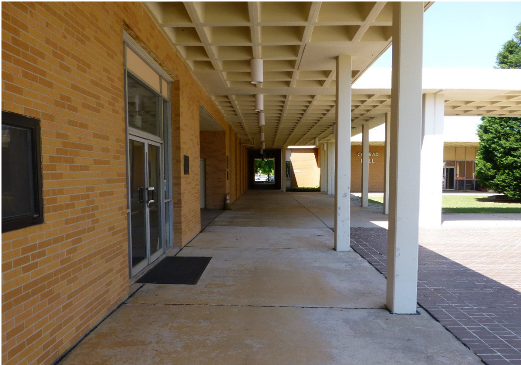
Figure 228. Concrete waffle canopy structure that encompasses Building 29805 and connects it to Buildings 29807 and 29808 (ERDC-CERL, 2015).
