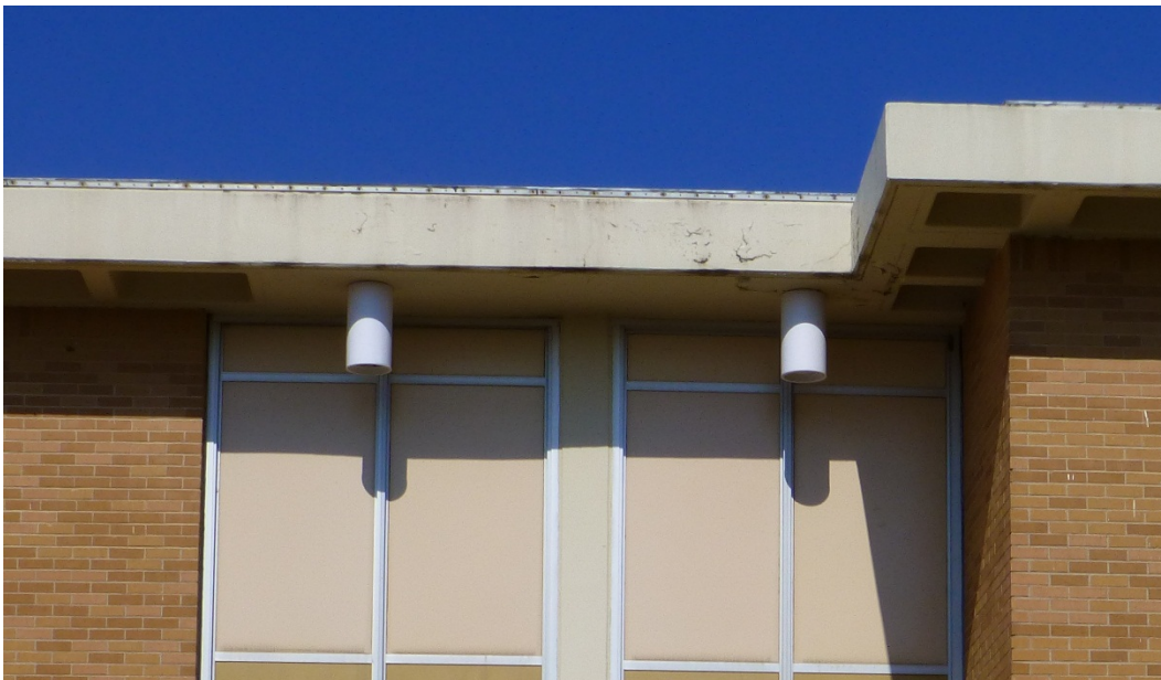
Figure 77. Ceiling-mounted light fixtures located under the concrete overhang at an entry bay on Building 29817, Allison Hall (ERDC-CERL, 2015).
