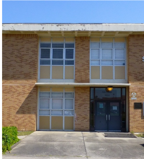
Main entry on the south elevation with groups of three windows, flat concrete canopy, and metal entry doors.
