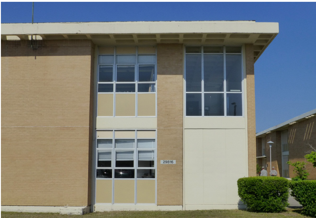
Figure 50. Example of three window systems: bright-aluminum framed awning windows with insulated panels, bright-aluminum framed fixed-pane windows, and concrete panel inserts, Building 29816, Fisher Hall (ERDC-CERL, 2015).
