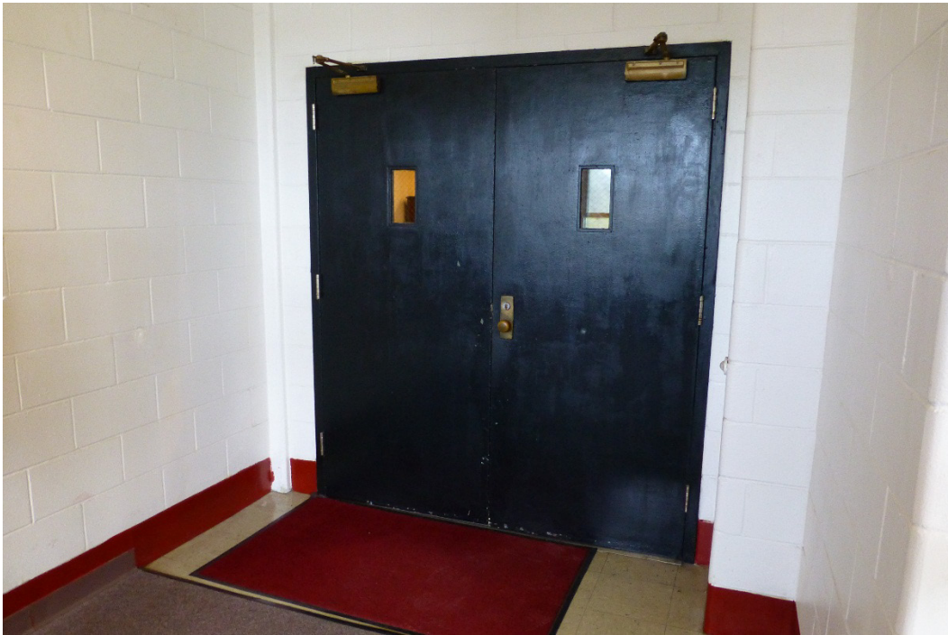
Figure 151. Typical metal security doors with one small pane, leading from the stairwell into the central hall (ERDC-CERL, 2015).
