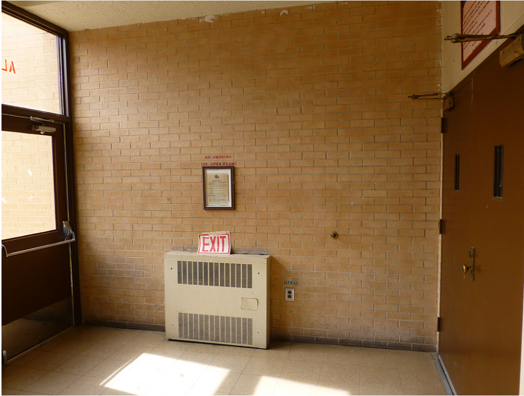
Figure 128. Example of unpainted, exposed brick in vestibules (ERDC-CERL, 2015).
