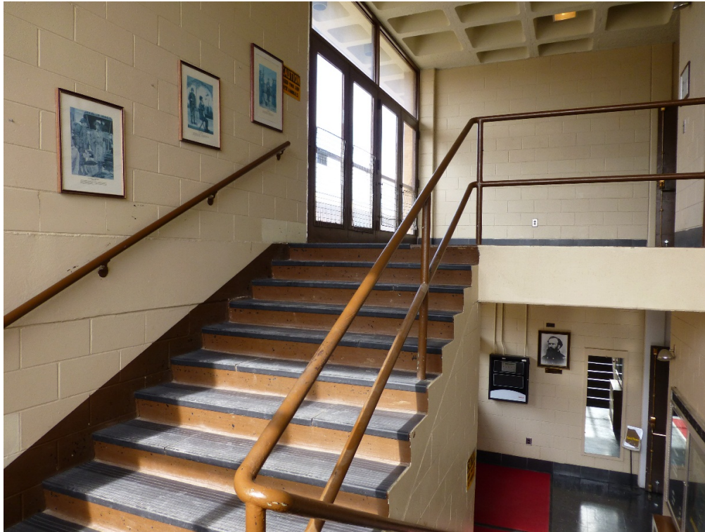
Figure 134. Interior view of typical stairwell with second-floor metal and plate-glass doors showing concrete switchback stairs, metal handrails, exposed concrete walls, and exposed concrete waffle ceiling (ERDC-CERL, 2015).
