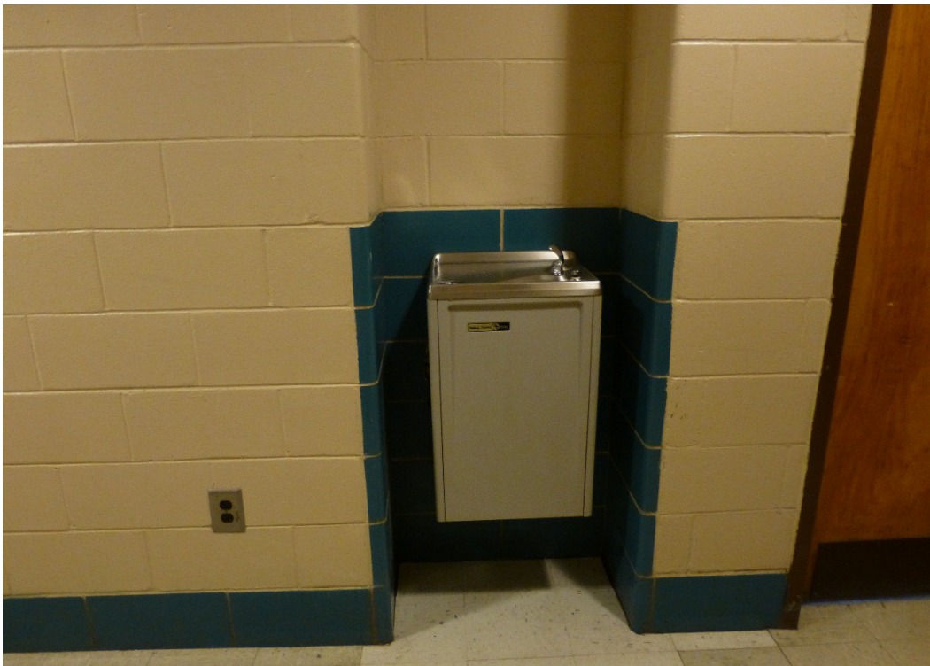
Figure 165. Typical water fountain alcove found in the Signal School classroom buildings (ERDC-CERL, 2015).
