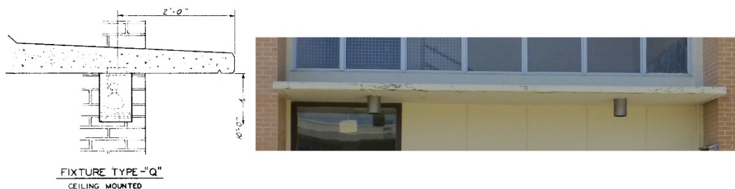
Figure 298. Ceiling-mounted light fixture under flat concrete canopy – comparison of the original design and material from 1966 [left] to the current condition of the ceiling-mounted light fixture [right] (ERDC-CERL, 2015).
