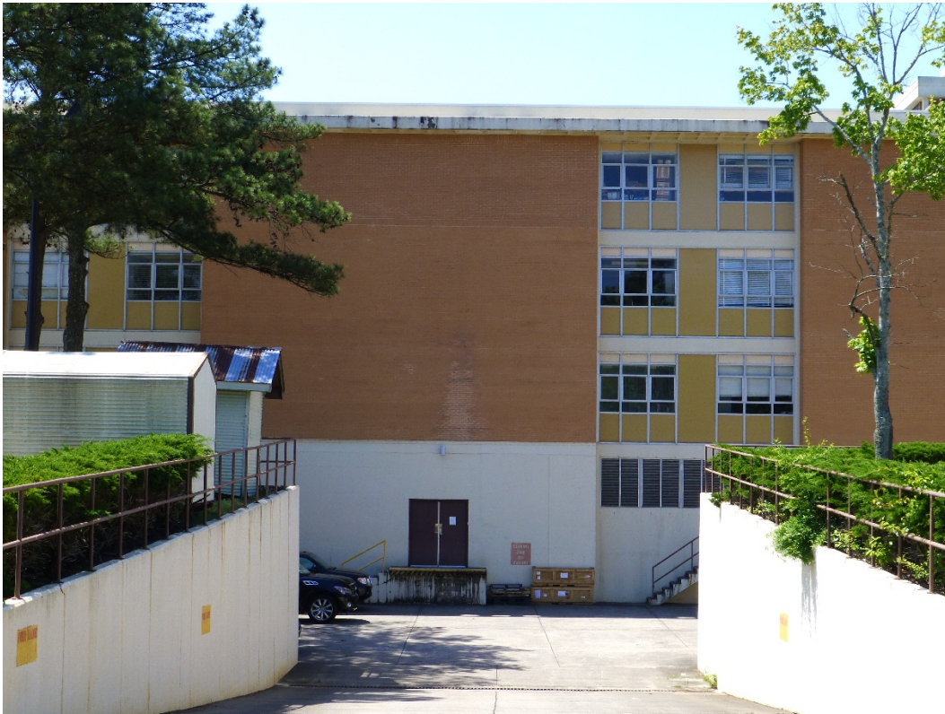
Figure 88. Poured-in-place concrete retaining walls framing driveway to walkout basement for Building 29810, Burkhardt Hall (ERDC-CERL, 2015).
