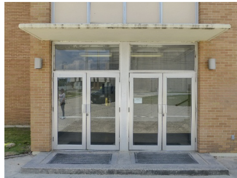
Bright-aluminum and plate-glass doors with transoms protected by a flat concrete canopy.
