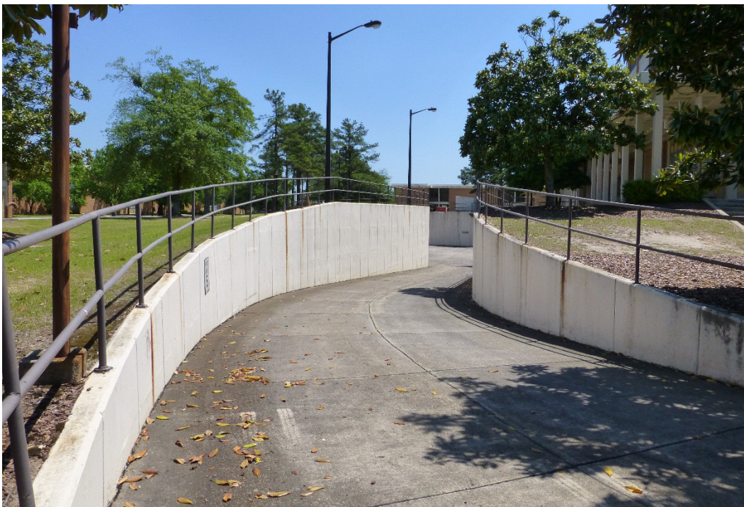
Figure 87. Curved poured-in-place concrete retaining wall system topped with metal pipe handrails, Building 29808, Signal Towers (ERDC-CERL, 2015).
