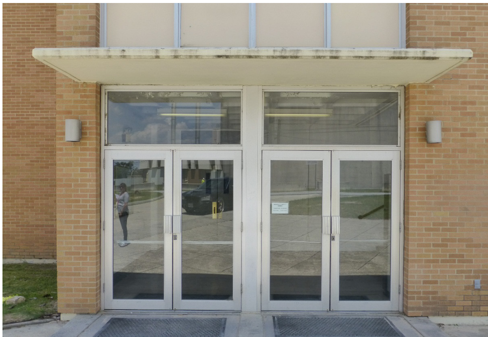
Figure 54. Paired bright-aluminum and plate-glass entry doors with transoms above, Building 25810, Brant Hall (ERDC-CERL, 2015).
