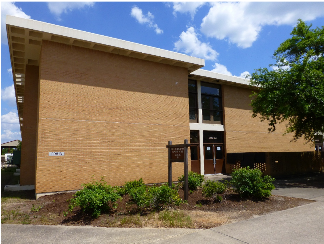
Figure 38. Typical concrete waffle overhang on the classroom buildings, Building 29813, Allen Hall (ERDC-CERL, 2015).
