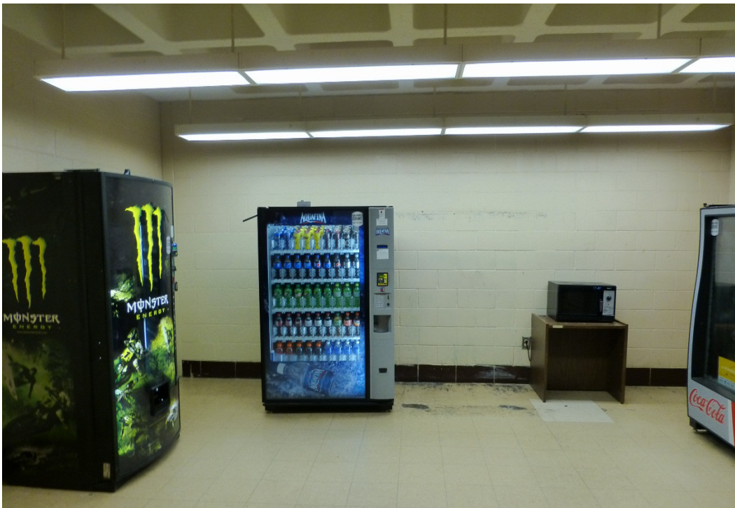
Figure 162. Example of a vending area with concrete block wall and exposed concrete waffle ceiling (ERDC-CERL, 2015).
