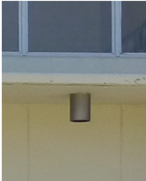
Ceiling-mounted light fixture under flat canopies.
