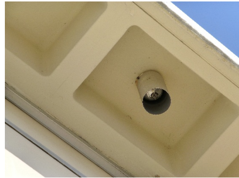
Ceiling-mounted light fixtures under the waffle overhang on the east and west elevations.
