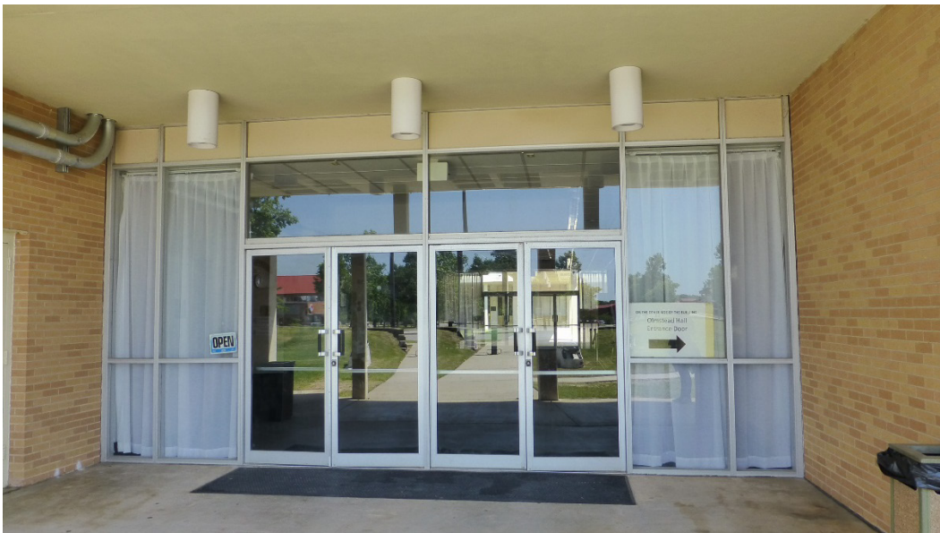
Figure 55. Bright-aluminum and plate-glass doors with sidelights and transom, Building 29805, Alexander/Olmsted Halls (ERDC-CERL, 2015).
