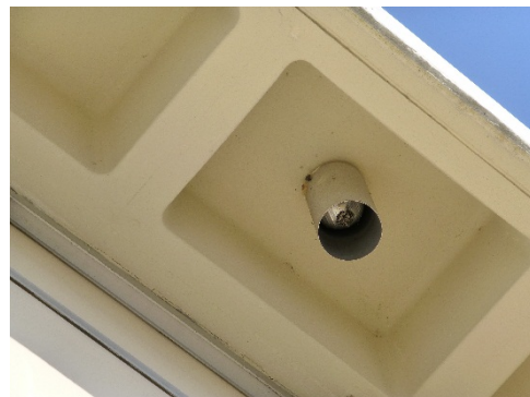
Ceiling-mounted light fixtures set within a waffle overhang.
