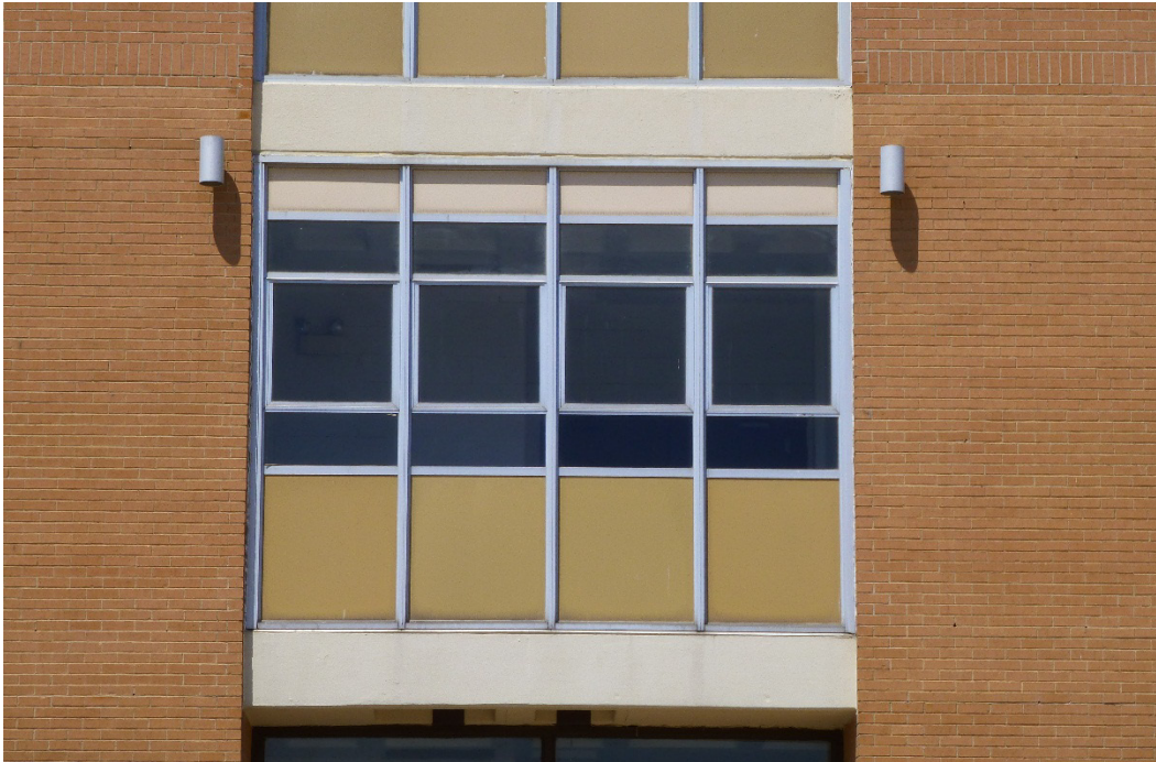
Figure 44. Typical four-bay window system designed with bright-aluminum frames, three-pane awning windows, and insulated panels, Building 29810, Burkhardt Hall (ERDC-CERL, 2015).
