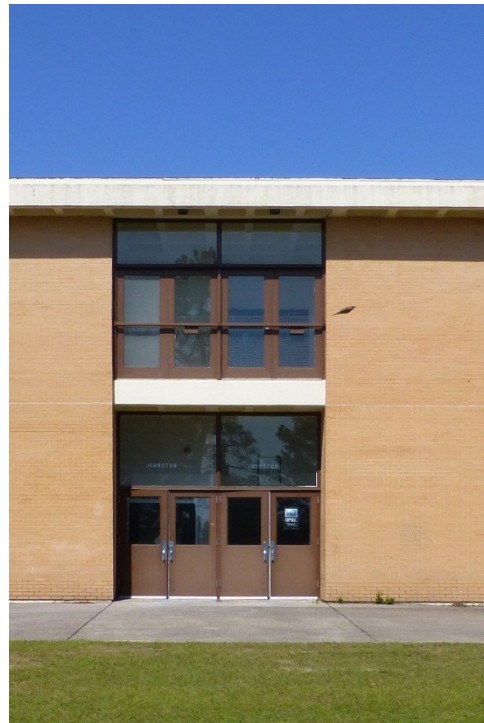
Metal doors with pane and transom on first floor and metal and plate-glass doors on second floor, separated by exposed concrete structural system.
