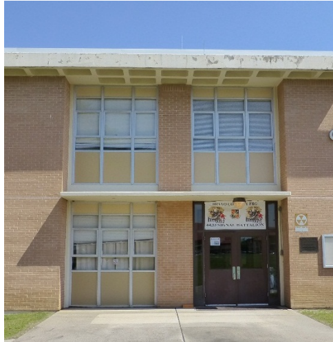
Entry bay with bright-aluminum framing three-pane awning-style windows sandwiched between insulated panels, flat concrete canopy, and metal doors with large pane.
