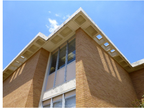
Overhanging eaves (waffle construction) with perforated waffles casting a "light pattern" on the second floor of the brick walls.
