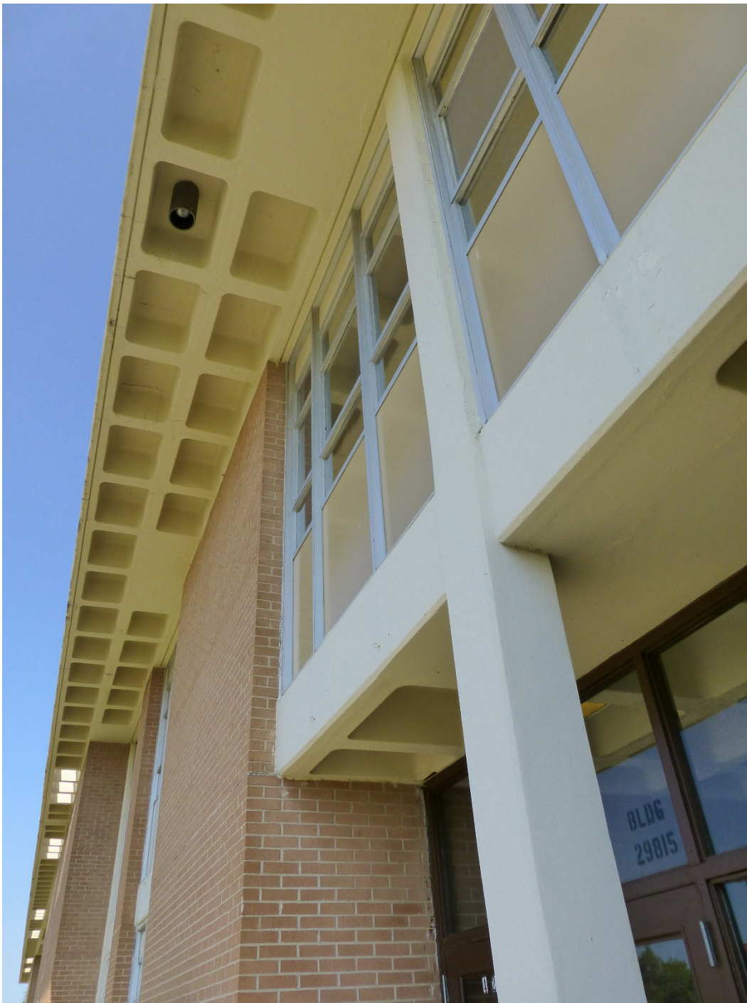
Figure 63. Close-up of the exposed concrete structural system framing the doors and window bays, Building 29815, Hazen Hall (ERDC-CERL, 2015).
