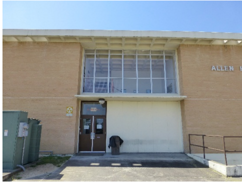
Entry bay on north elevation with concrete panels, metal doors, flat concrete canopy, and fixed windows framed with bright-aluminum sashes.
