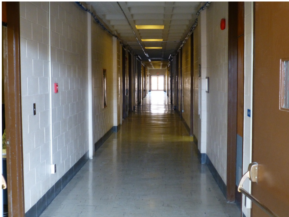
Figure 126. Example of an interior view looking down a central hallway with the exposed concrete waffle ceiling and concrete block walls (ERDC-CERL, 2015).
