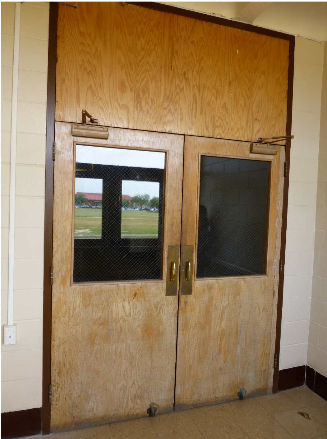
Figure 153. Typical wood doors with a large pane and wood transom, leading from stairwell into the central hallway (ERDC-CERL, 2015).
