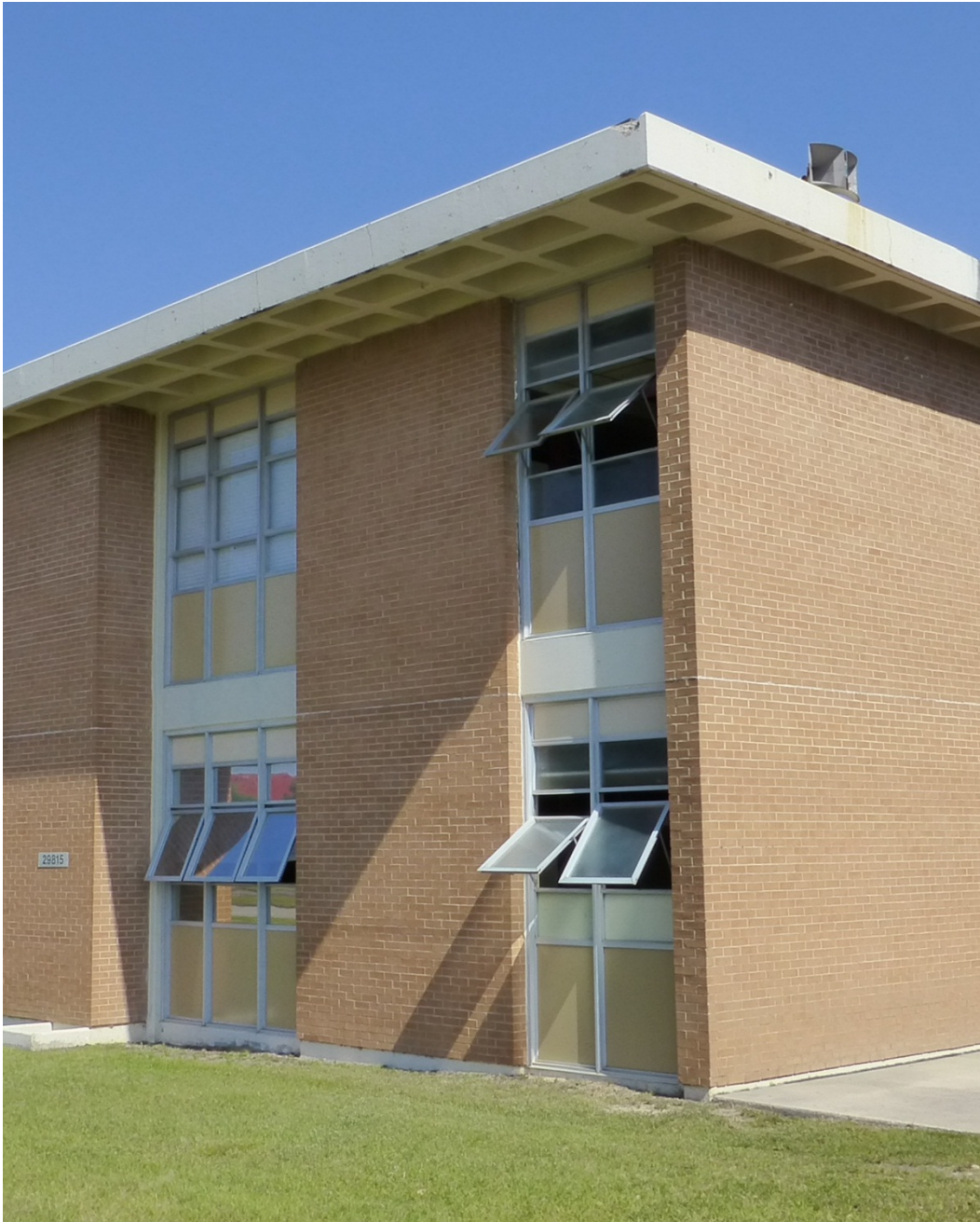
Figure 46. Typical window bay system with bright-aluminum frames, three-pane awning windows, and insulated panels, Building 29813, Allen Hall (ERDC-CERL, 2015).
