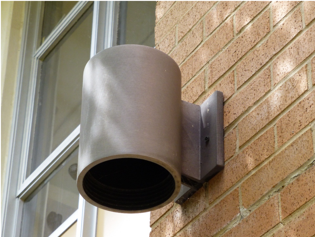
Figure 76. Example of a wall-mounted light fixture near an entry into a courtyard, Building 29817, Allison Hall (ERDC-CERL, 2015).
