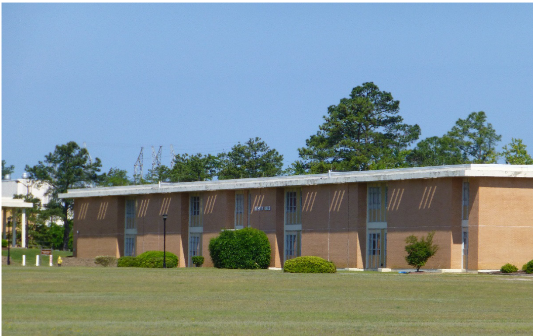
Figure 42. The “light pattern” displayed across the entire second floor of the south elevation, Building 29809, Greely Hall (ERDC-CERL, 2015).
