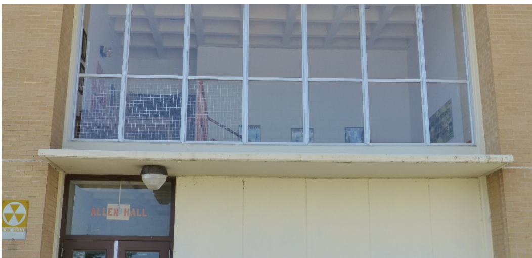
Figure 69. Flat concrete canopy extending over entry doors and a bay of concrete panels on Building 29813, Allen Hall (ERDC-CERL, 2015).
