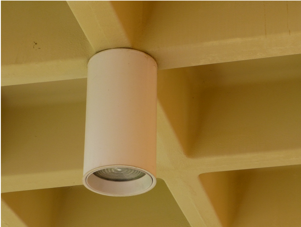
Figure 73. Ceiling-mounted light fixtures are placed on the underside of the concrete waffle canopy structure that connects Building 29805, Alexander/Olmsted Halls; 29807, Conrad Hall; and 29808, Signal Towers (ERDC-CERL, 2015).
