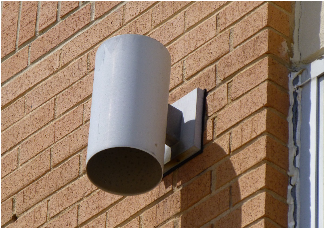
Figure 75. Example of a wall-mounted light fixture that flanks either side of a window bay, Building 29810, Burkhardt Hall (ERDC-CERL, 2015).
