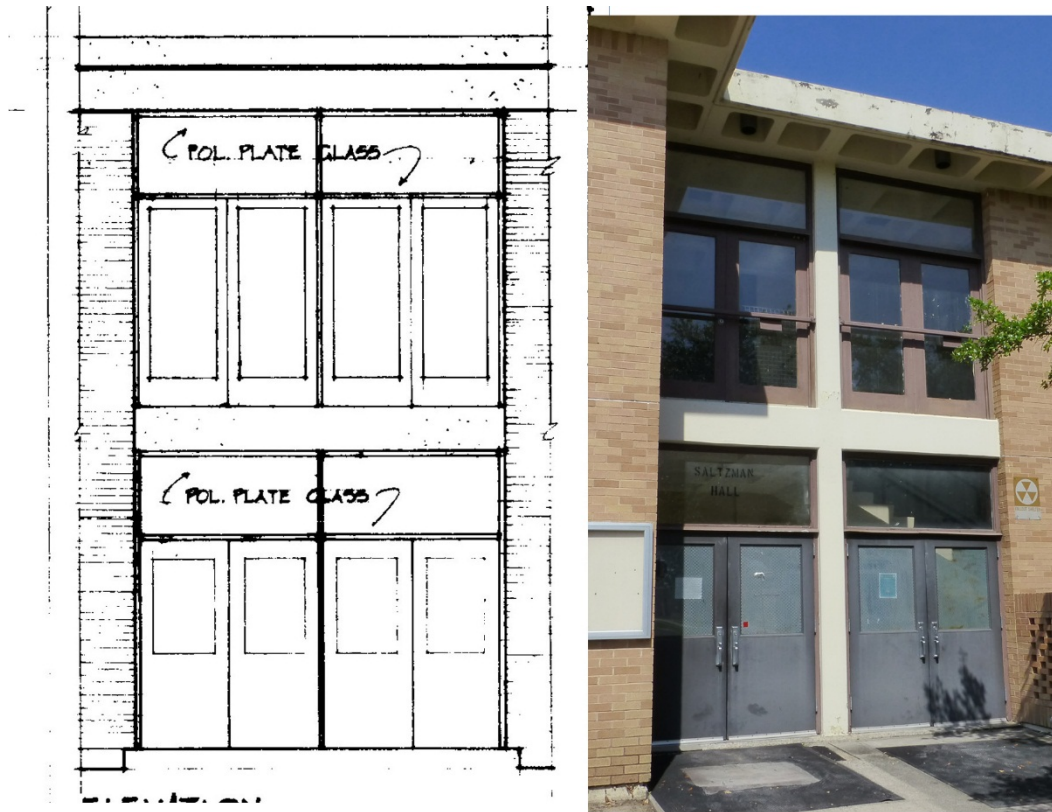
Figure 337. Doors on the east and west elevations – comparison of the original design and materials from 1964 [left] to the current condition of the metal doors with pane and transoms on the first floor and the metal and plate-glass doors with security bars on the second floor [right] (ERDC-CERL, 2015).
