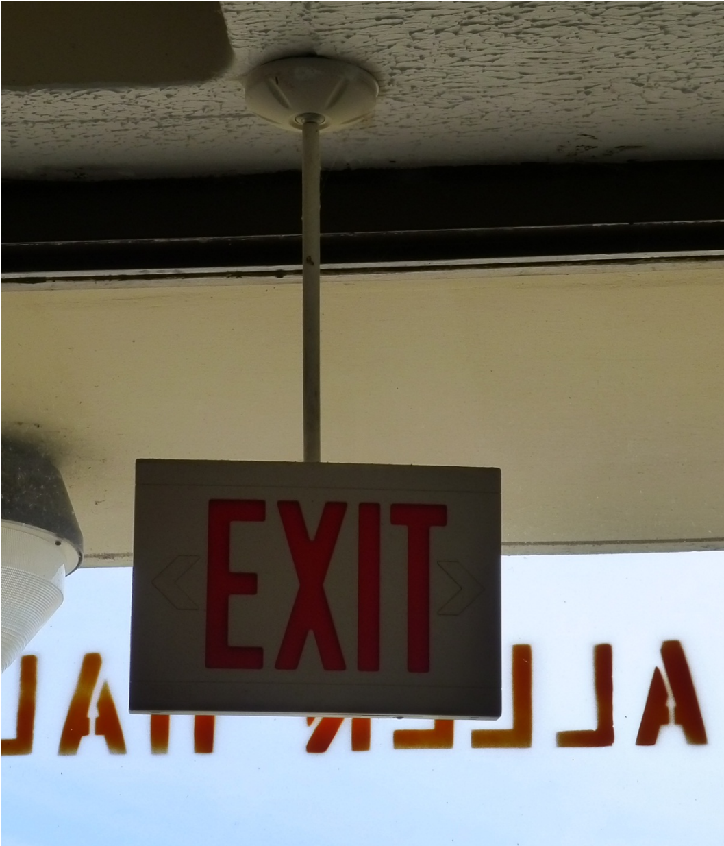
Figure 172. Typical suspended exit sign (ERDC-CERL 2015).
