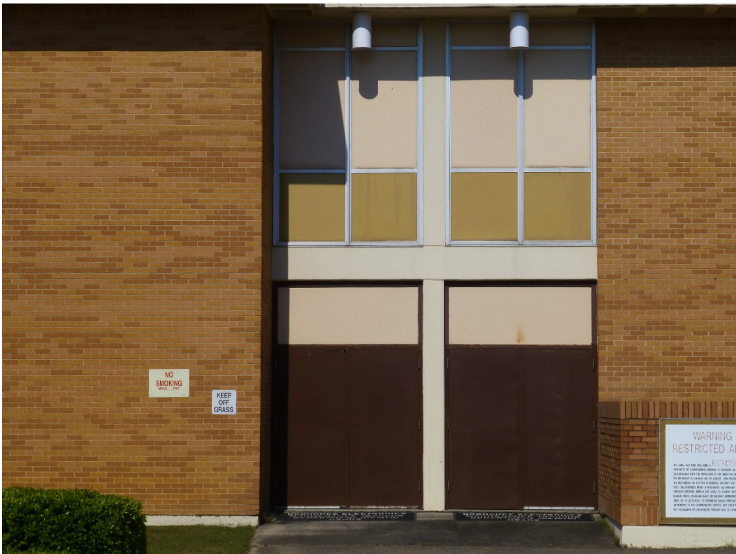
Figure 60. Metal doors with an insulated panel placed in the transom above, Building 29816, Fisher Hall (ERDC-CERL, 2015).
