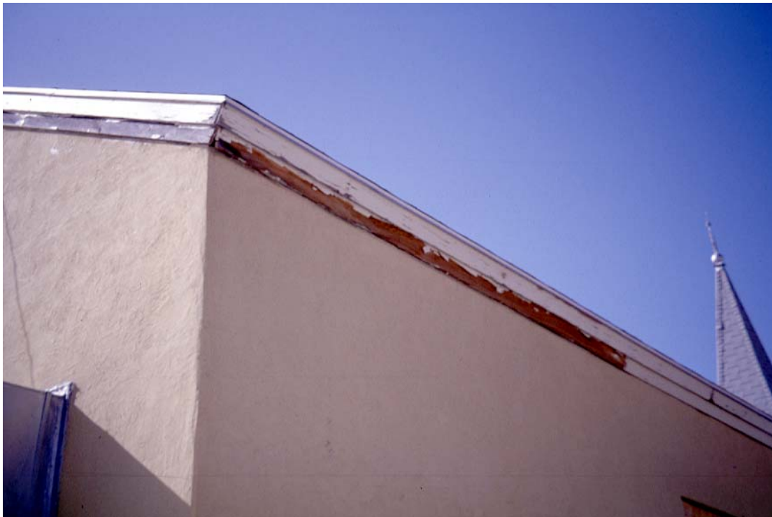
Photograph 10. Detail of paint failure on chapel trim.
