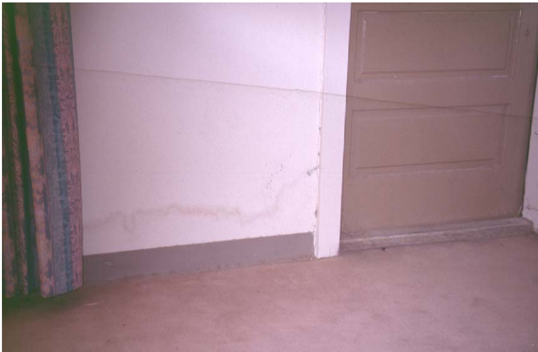
Photograph 67. Stains on BOQ wallboard indicate leaking exterior walls.
