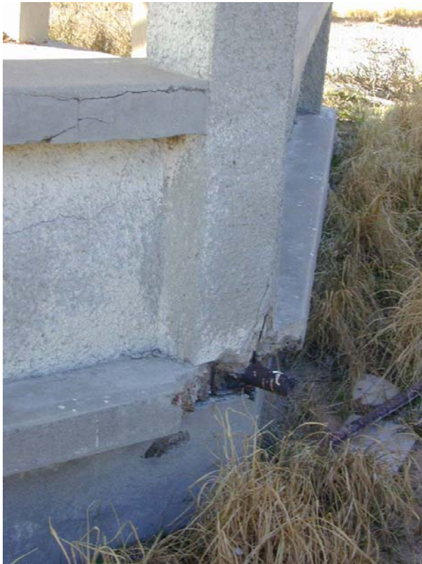
Photograph 3. Detail of exposed concrete reinforcement on bandstand.
