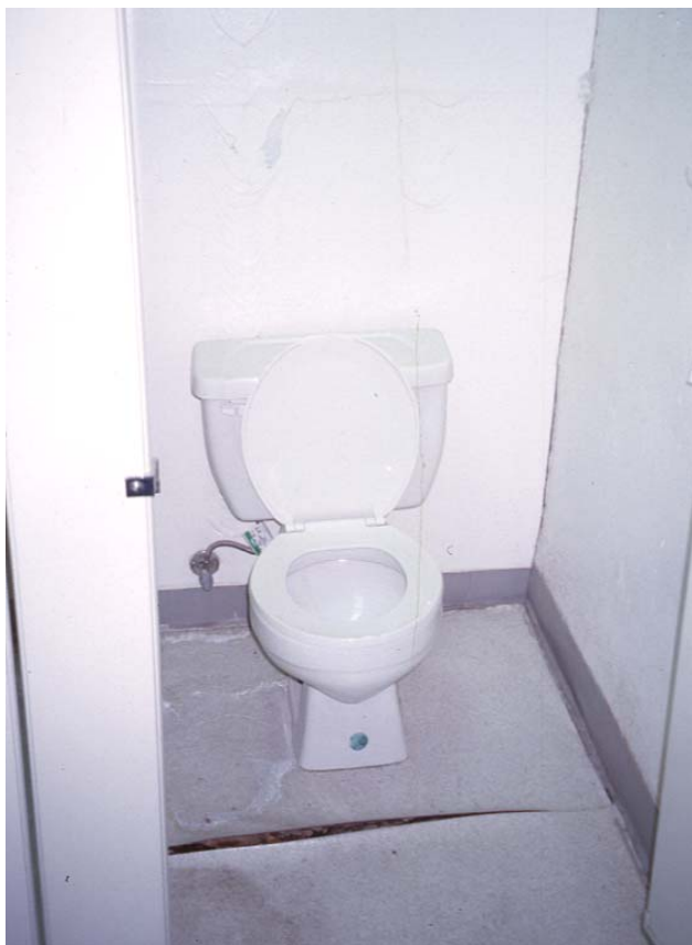
Photograph 53. Damaged vinyl flooring in Building 7158 washrooms.
