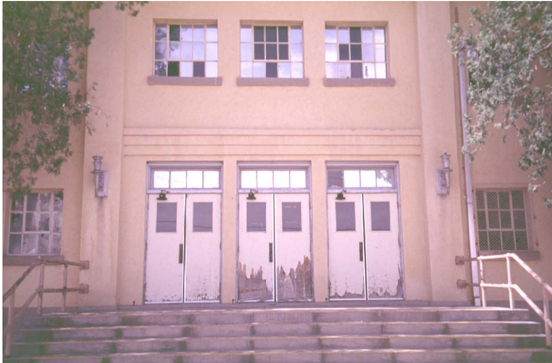
Photograph 26. Deteriorated gymnasium entry doors.
