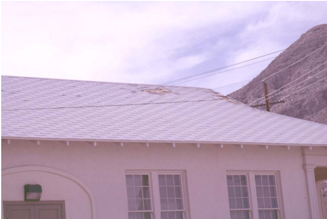
Photograph 81. Missing shingles on Conference Center.
