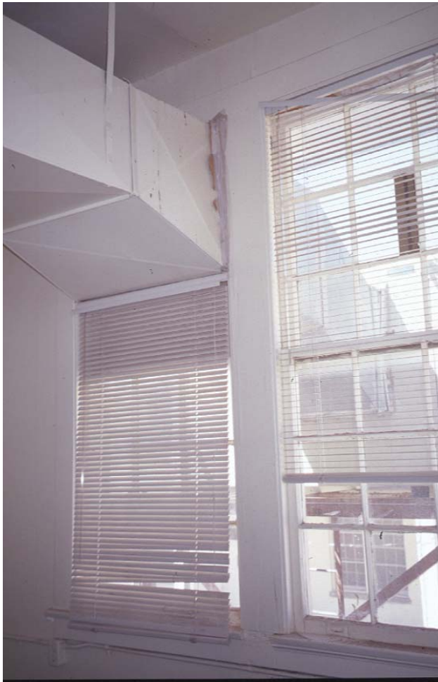
Photograph 59. Non-historic modification of window sashes in Building 7159.
