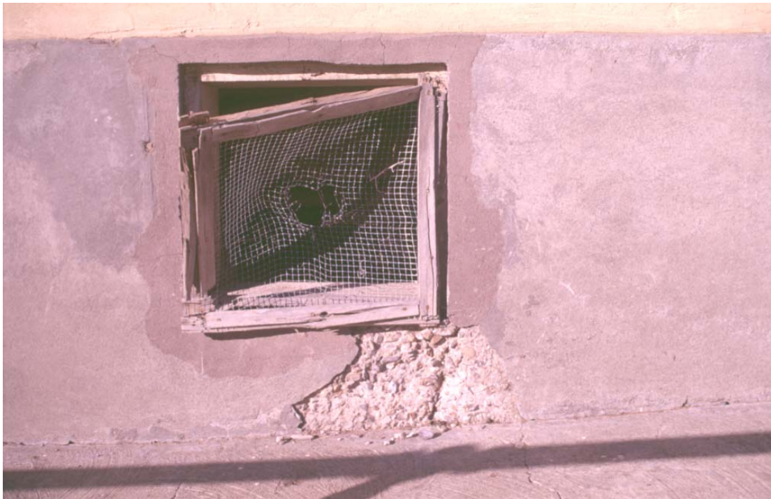
Photograph 20. Minor gymnasium foundation cracking.
