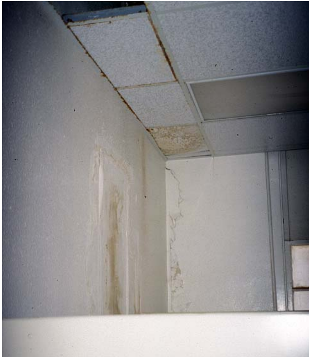
Photograph 52. Signs of water damage in Building 7158 washrooms.
