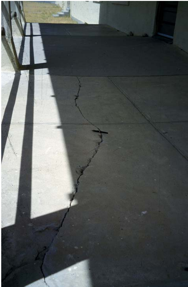
Photograph 73. Crack in west porch of Conference Center.
