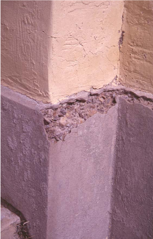
Photograph 21. Minor gymnasium pilaster cracking.
