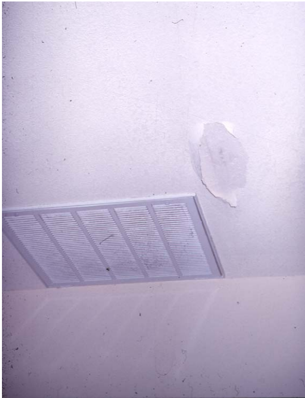
Photograph 66. Water stain on BOQ ceiling.
