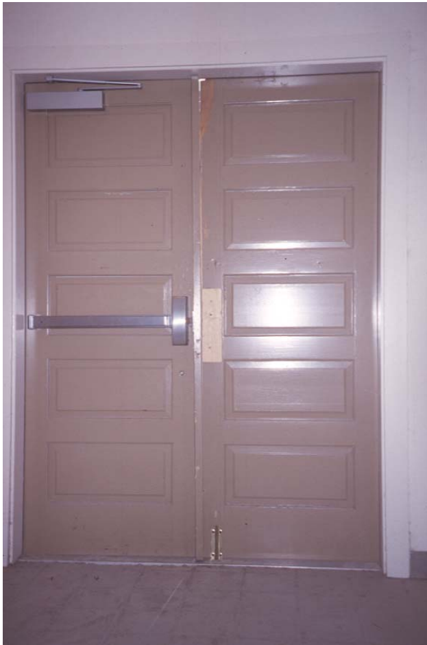
Photograph 63. Damage to BOQ entry door.
