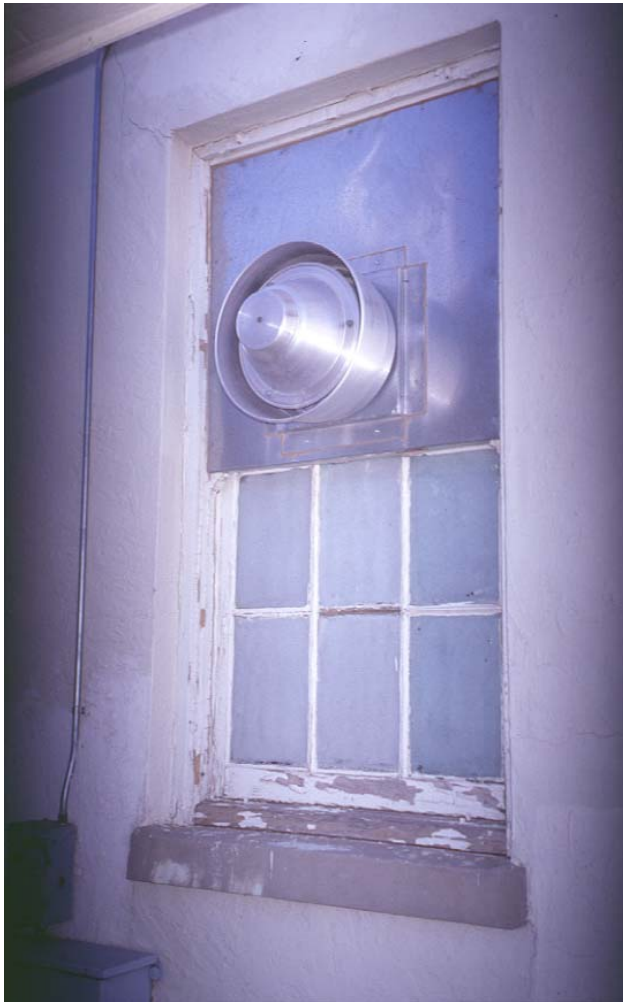
Photograph 43. Non-historic washroom window modification.
