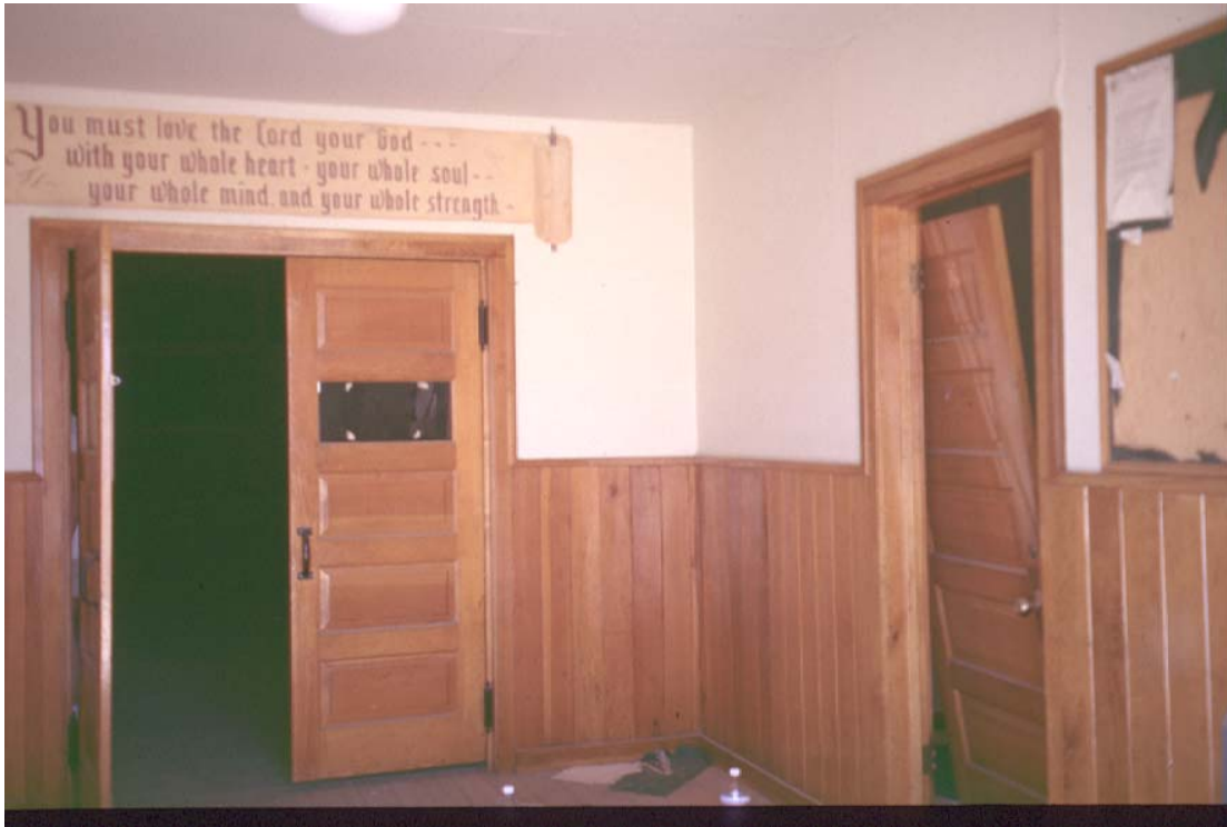
Photograph 12. Damaged chapel lobby door.
