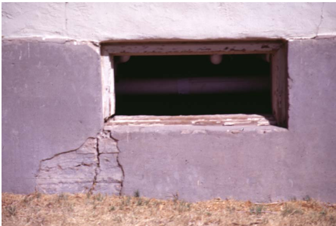
Photograph 33. Detail of minor barracks foundation damage.
