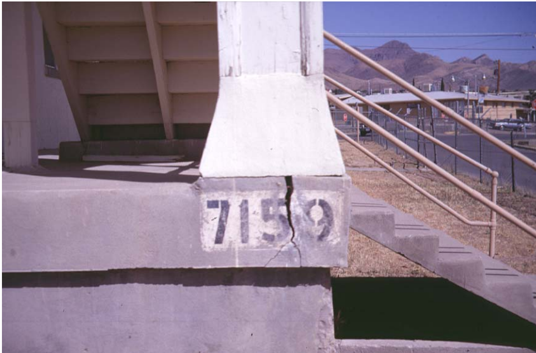
Photograph 34. Detail of barracks porch slab cracks.
