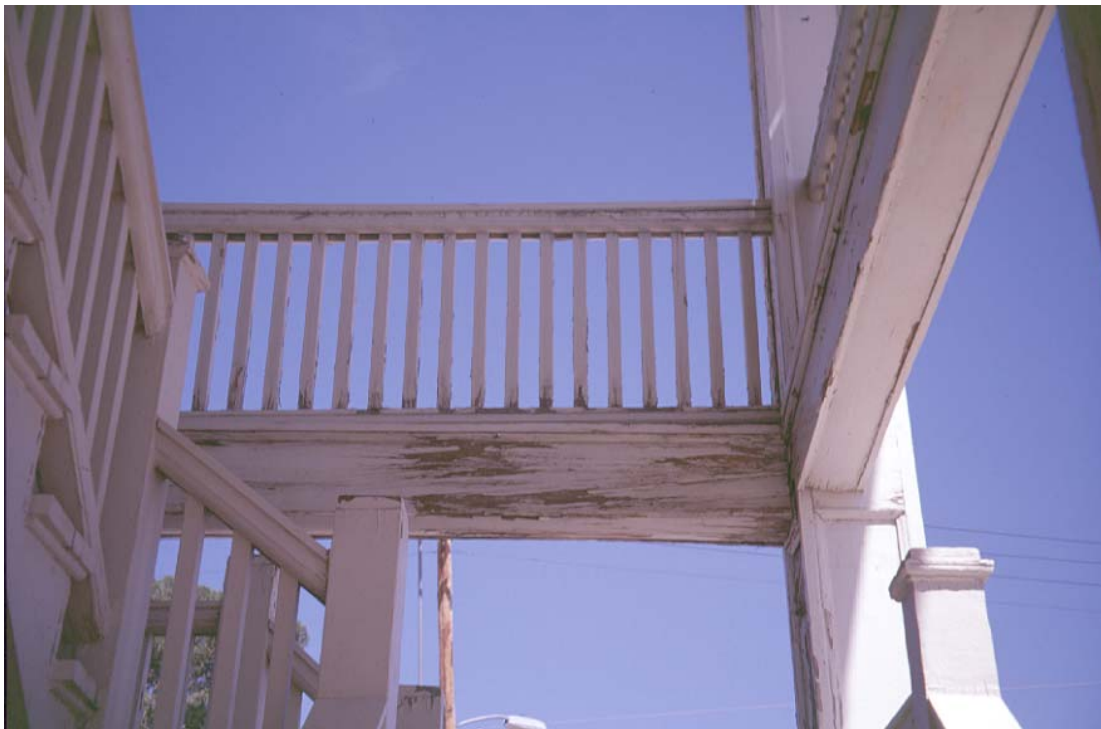
Photograph 40. Typical deteriorated exterior trim on barracks.
