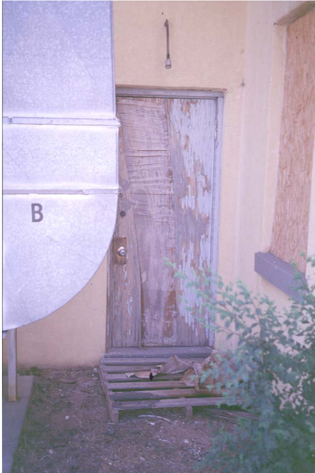
Photograph 9. Deteriorated sacristy door.
