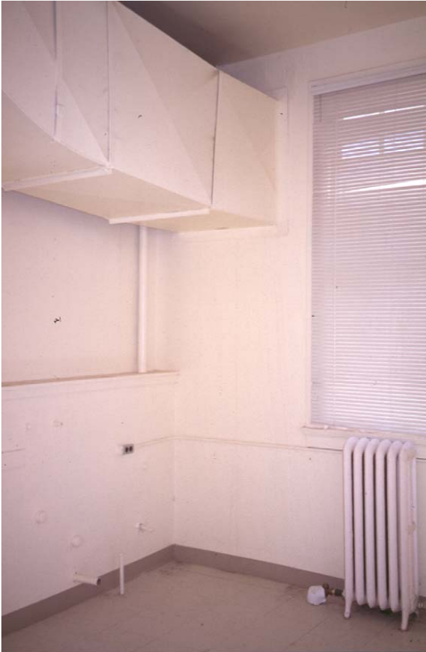
Photograph 50. Building 7157 cooling equipment.
