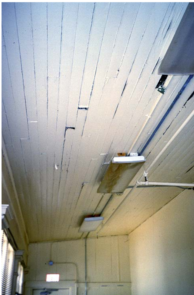
Photograph 51. Signs of porch roof leakage in Building 7158.
