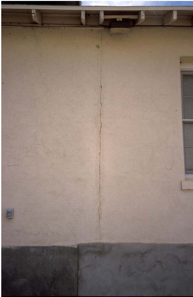
Photograph 61. BOQ foundation and wall crack.
