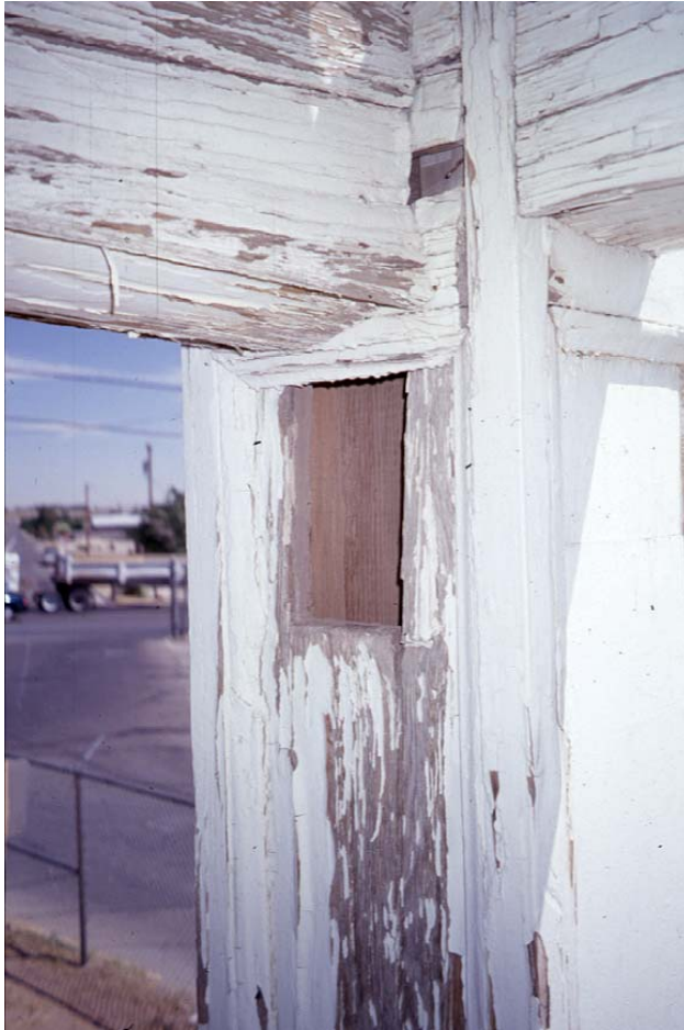
Photograph 57. Possible structural problem with barracks porch support beam.
