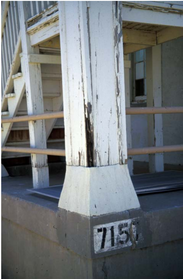
Photograph 37. Water-damaged stucco detail on barracks porch column.
