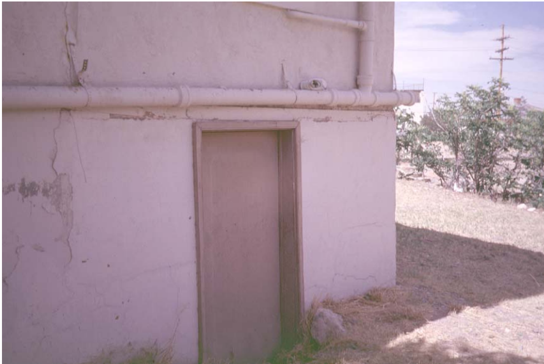
Photograph 64. Deteriorated BOQ basement door.
