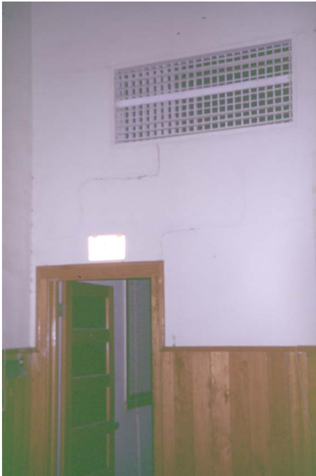
Photograph 11. Minor damage around chapel air conditioning duct.
