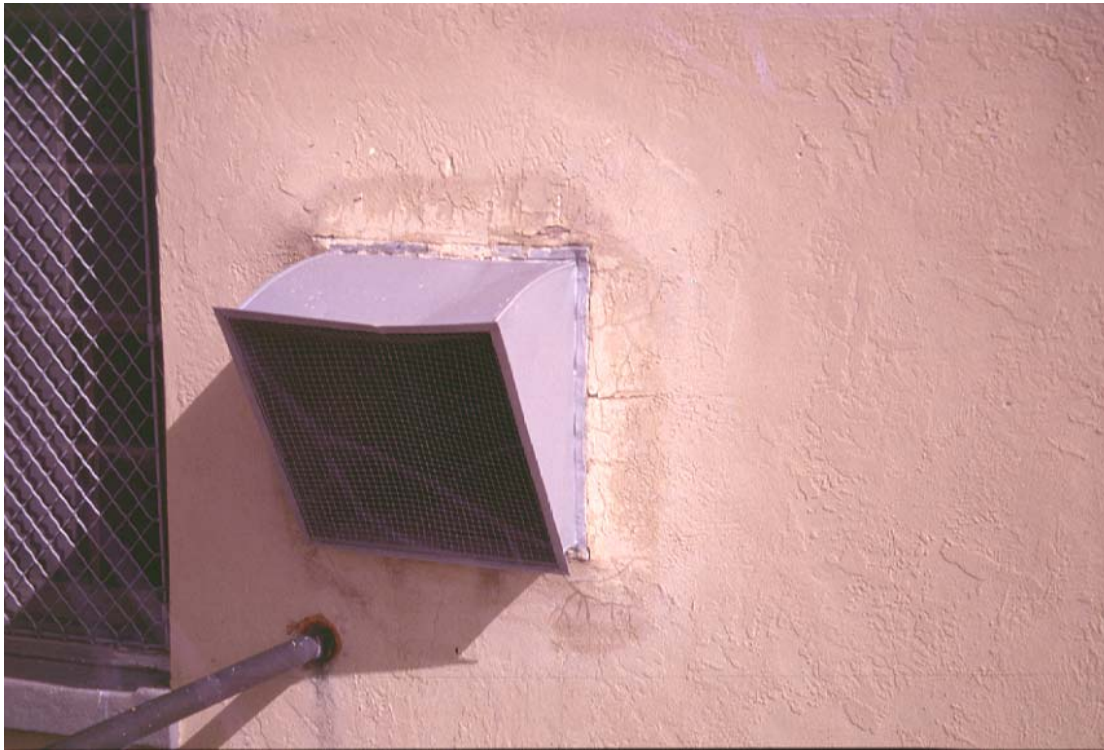
Photograph 16. Minor theater wall cracking around vent hood.
