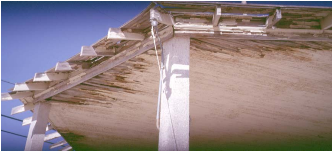
Photograph 5. Detail of bandstand roof structure deterioration.
