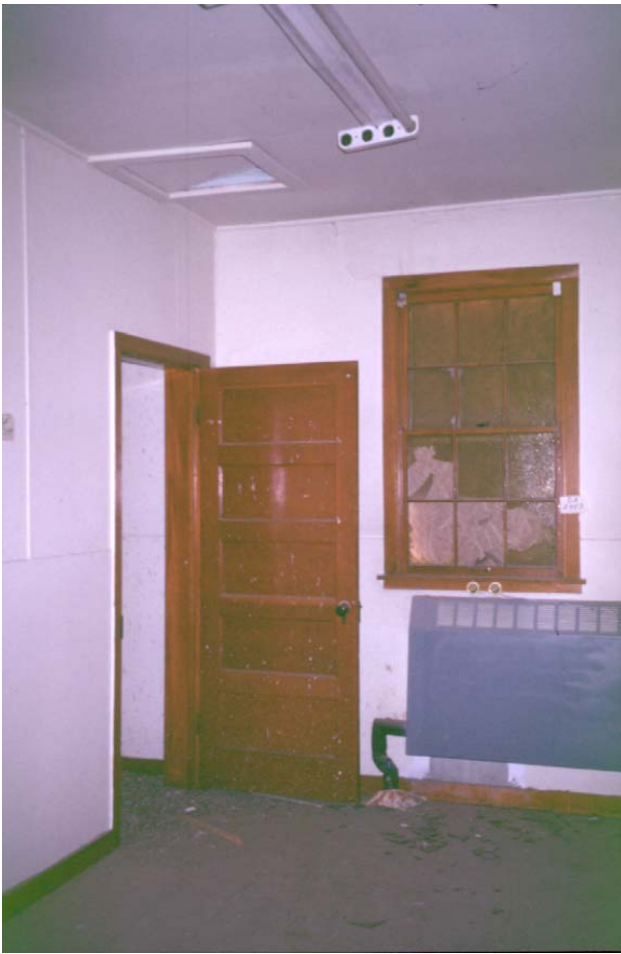
Photograph 8. Damaged sacristy window sashes.
