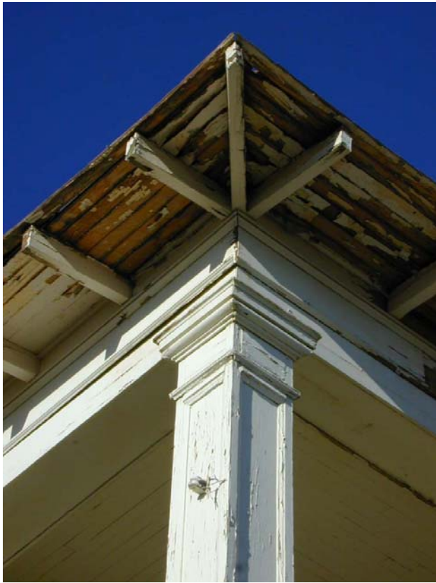
Photograph 46. Typical barracks porch roof damage.
