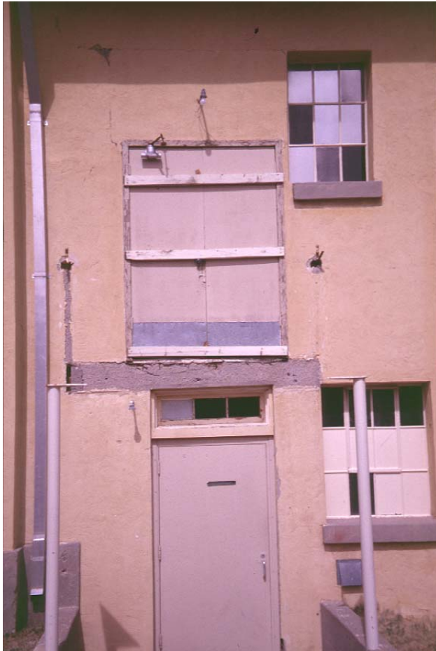
Photograph 24. Gymnasium wall damage where fire escape was removed.
