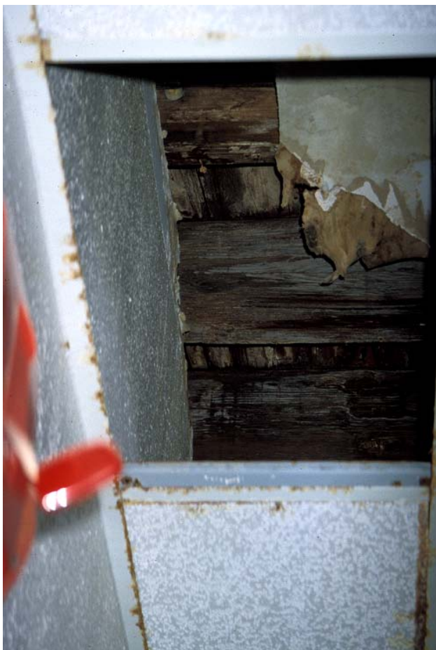
Photograph 45. Typical water-damaged barracks ceiling in first-floor washroom.
