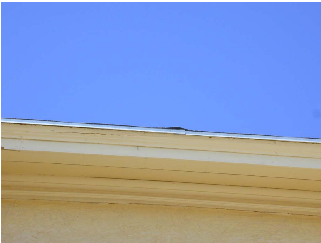
Photograph 28. 'Fish-mouth' shingle warpage on gymnasium gable.
