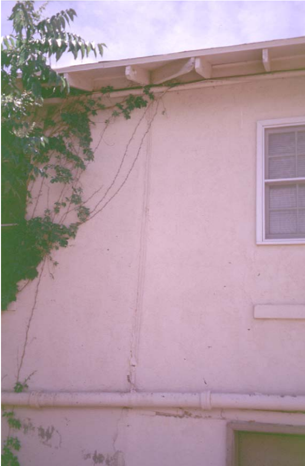
Photograph 62. Minor BOQ wall crack.
