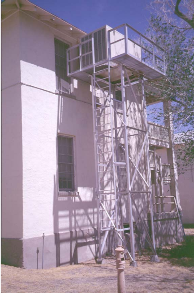
Photograph 47. Historically inappropriate barracks cooling equipment.
