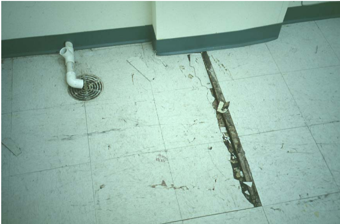
Photograph 76. Spongy floor area on Conference Center utility room.
