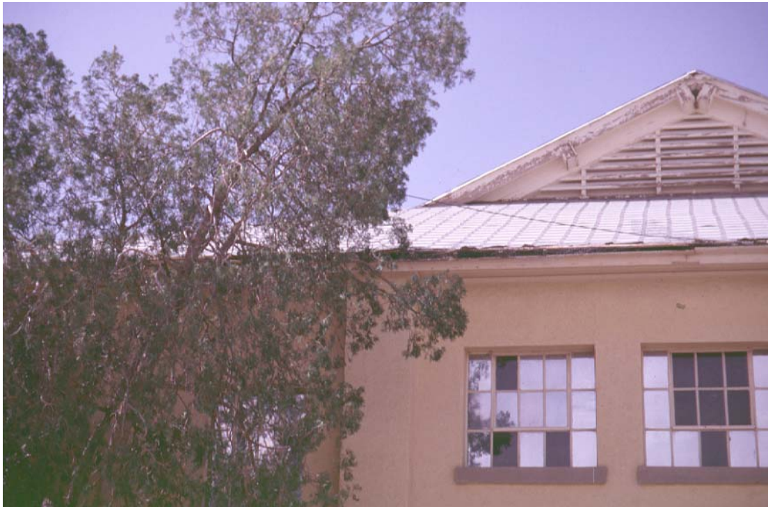
Photograph 27. Gymnasium roof abrasion.
