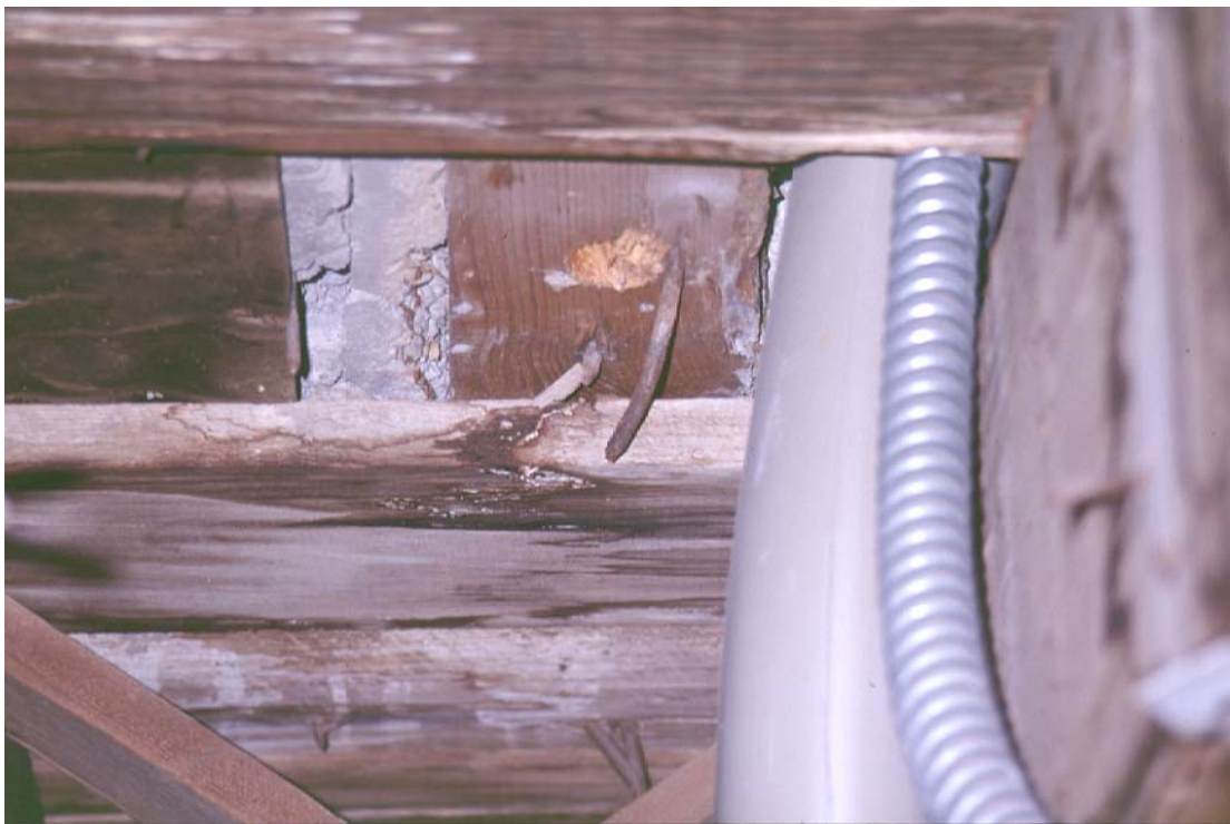
Photograph 77. Cut flooring joists under the spongy floor area.
