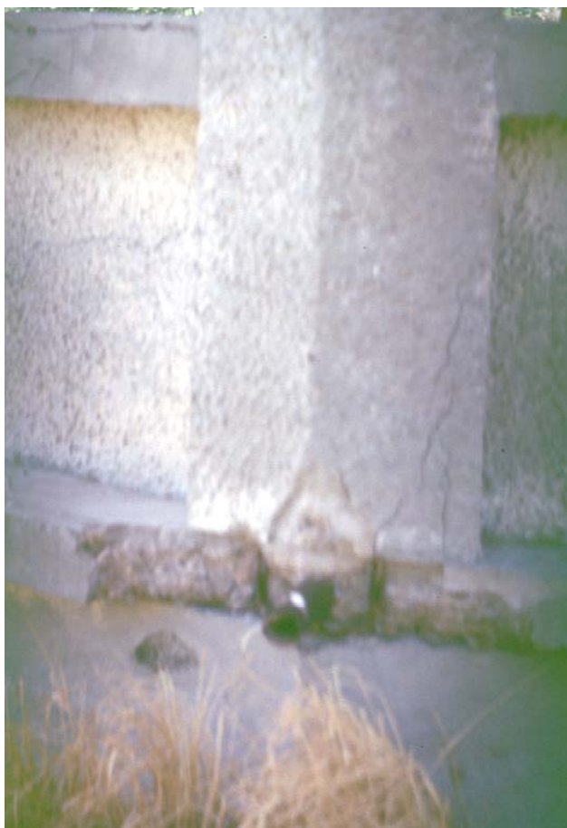
Photograph 2. Detail of spalled concrete on bandstand.
