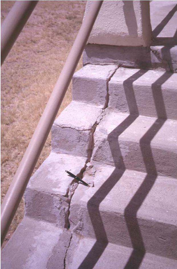
Photograph 74. Badly cracked Conference Center stairs.
