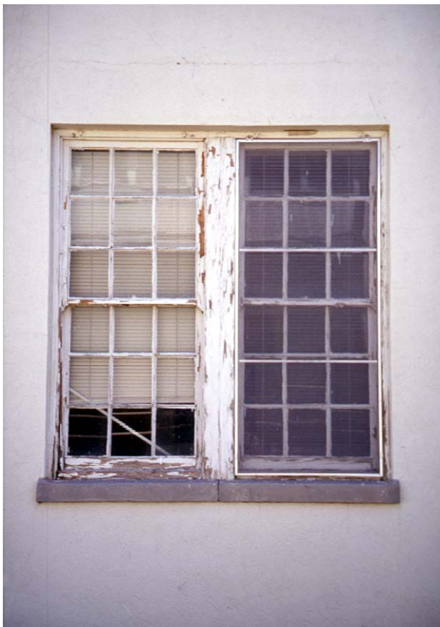
Photograph 36. Typical deteriorated wood trim on second-story barracks porches.
