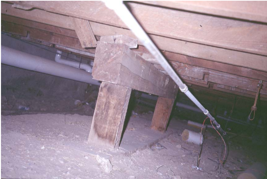
Photograph 56. Makeshift repair of floor framing under Building 7159.
