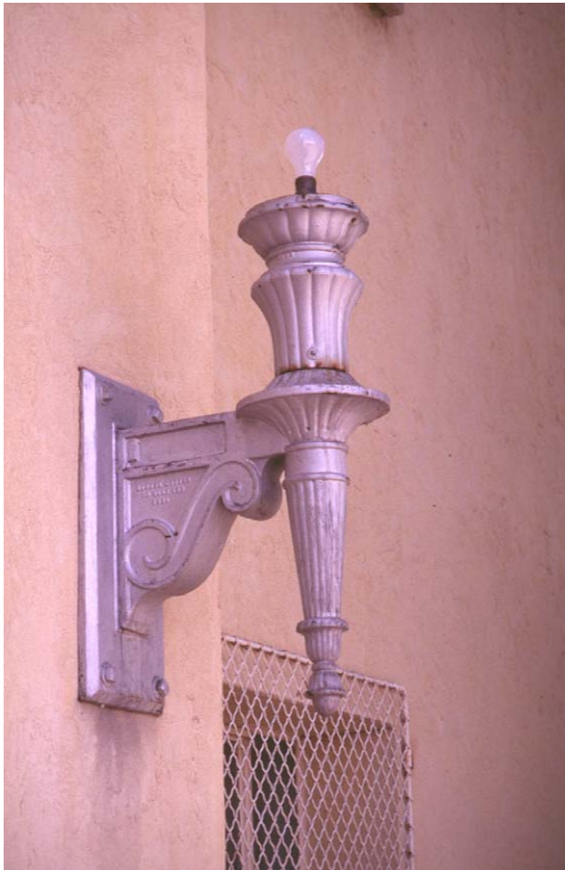
Photograph 31. Exterior gymnasium light fixtures with globes missing.
