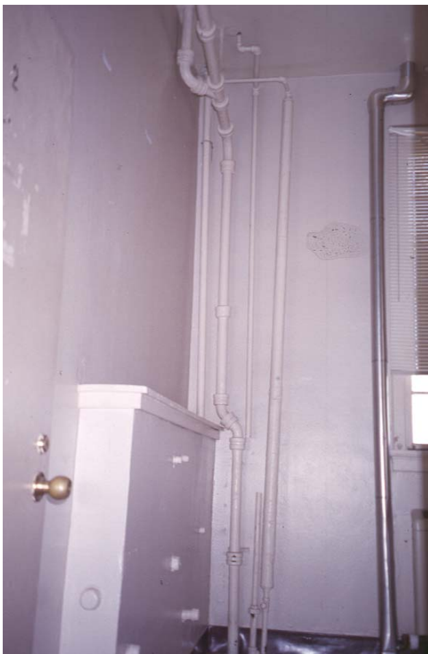
Photograph 49. Non-historic plumbing modifications in Building 7157.
