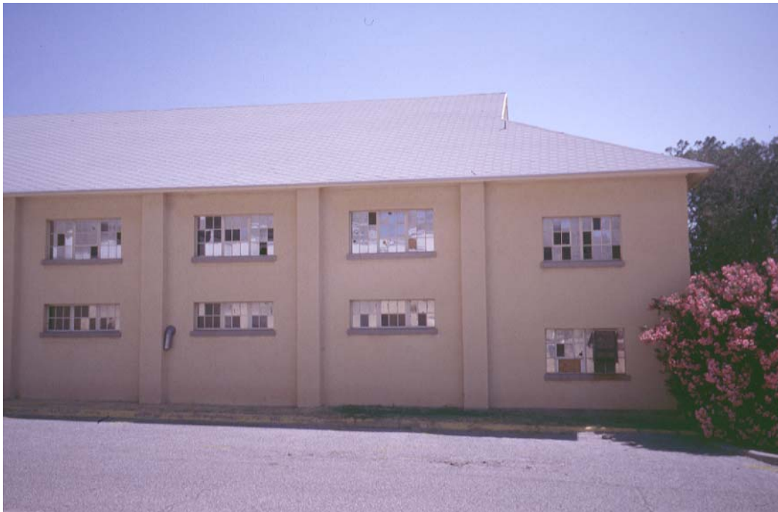
Photograph 25. Inconsistent use of film on gymnasium windows.
