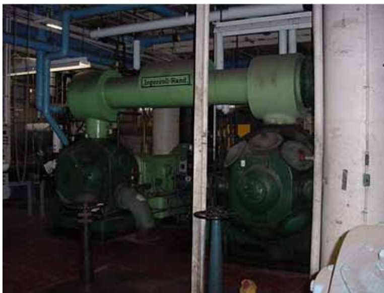
Figure 17. 4200 Ingersoll Rand reciprocating compressor.
