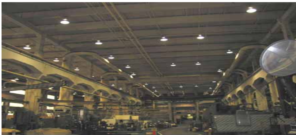
Figure 20. Building lighting with new high intensity discharge (HID) lamps.
