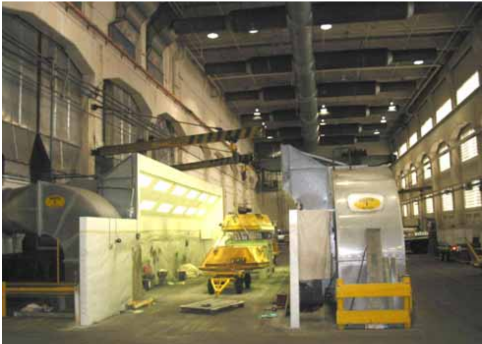
Figure 7. Open spray booth in the paint area.
