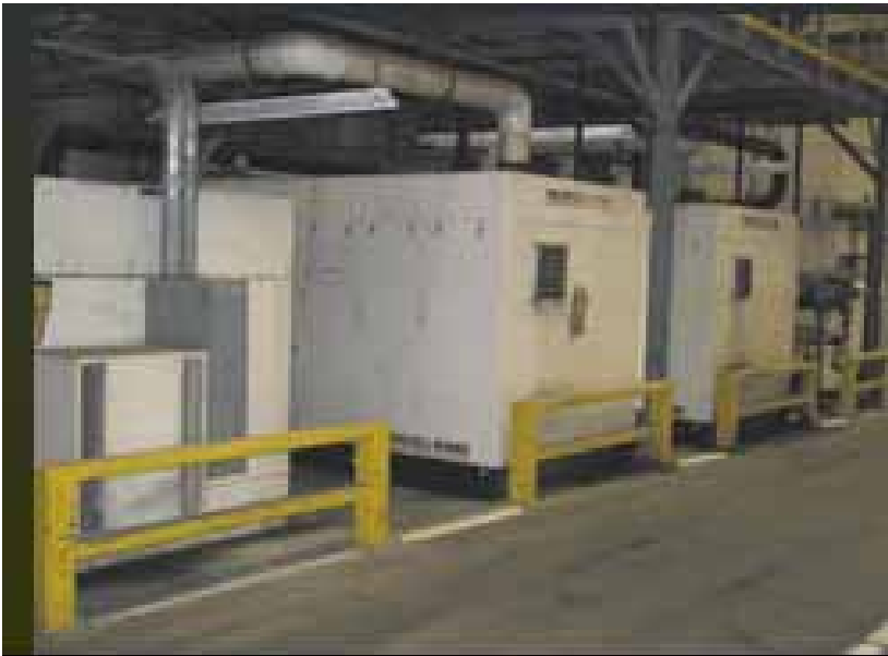
Figure 18. Photo of three air compressors in Building 222.
