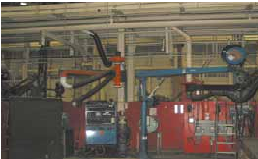
Figure 13. Welding booths with fume extraction arms.
