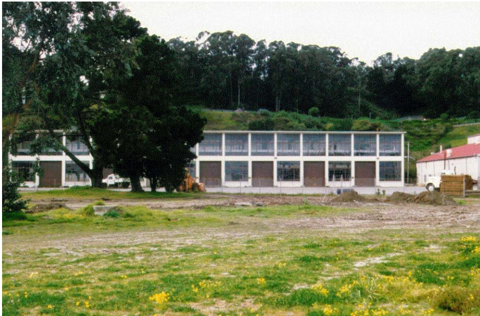
Figure 3. Site disturbance resulting from poorly planned staging of construction materials (source, R. Young).
