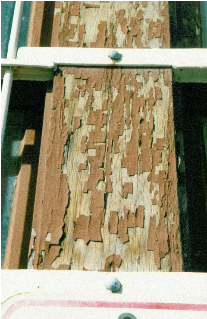
Figure 16. Construction activities in historic properties often disturb lead paint (source, R. Young).
