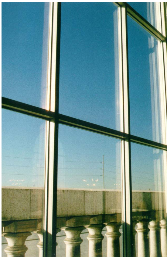
Figure 7. Windows and glazing can decrease the perceived need for natural light (source, R. Young).
