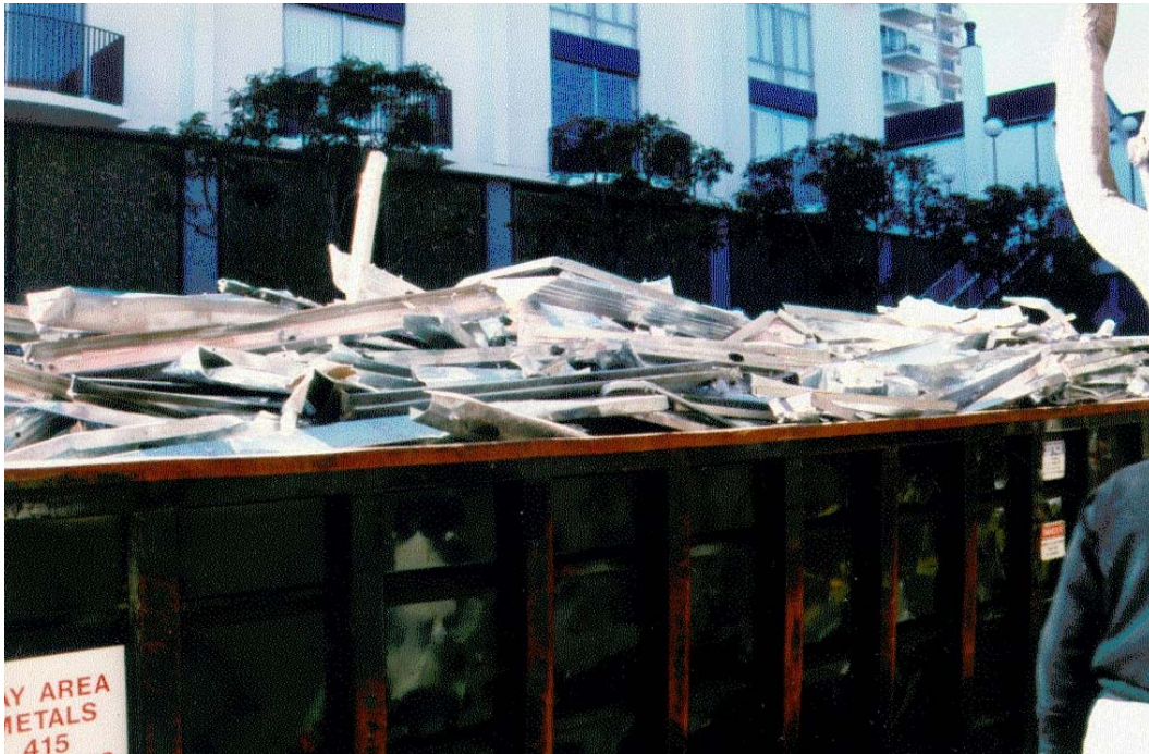
Figure 15. Toxic or hazardous building material should be carefully removed, stored, and disposed (source, CERL).
