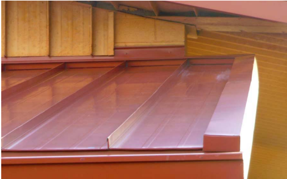
Figure 22. Finished edge detail and wall flashing. (Note that there are no exposed fasteners in these cleated eave details.)
