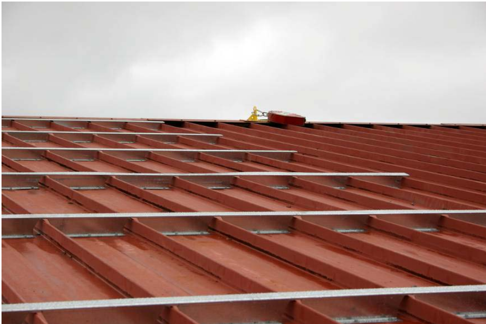
Figure 13. Installed custom manufactured sub-purlin system designed to bridge underlying metal roof panel ribs..
