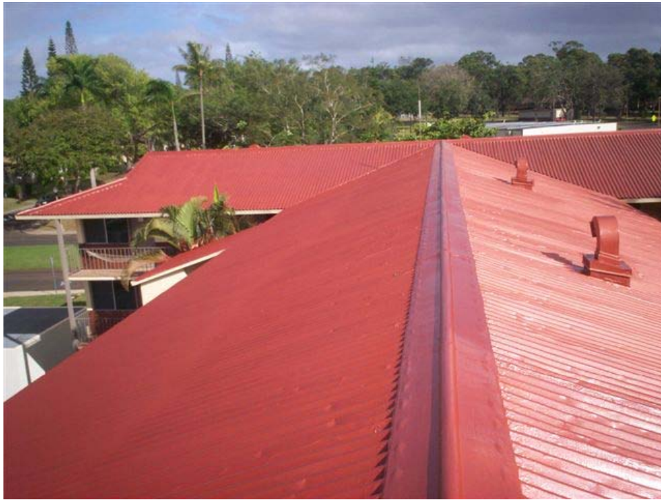
Figure 8. Top view of Building 118 roof after completion. An uneven high gloss was visible from the ground
