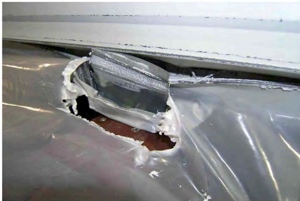
PHOTOGRAPH 22 FIXED CLIP FAILURE - 3
