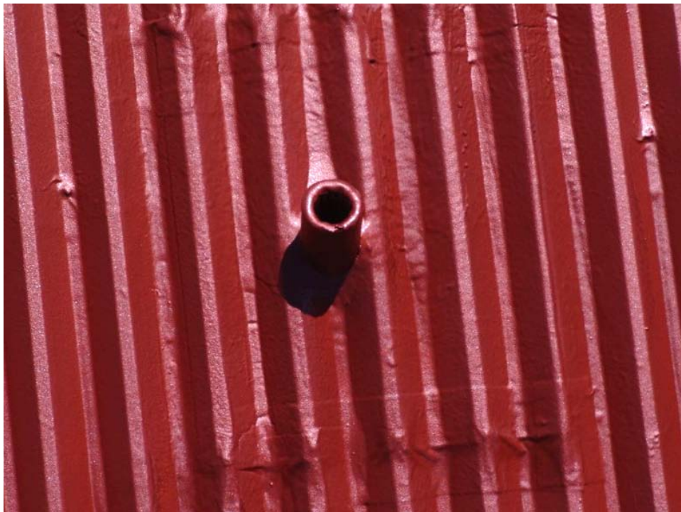
Figure 9. Finished appearance of vent stack. – Note the patch and thicker coating applied over the metal roof lap
