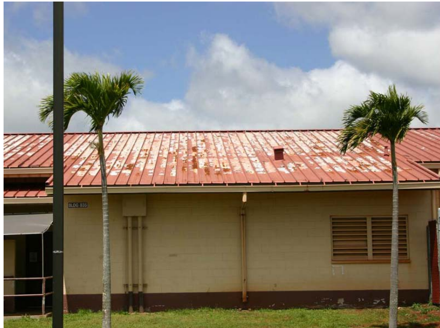
Figure 10. Roof of Building 835 before re-cover. Paint was peeling off in large sheets.
