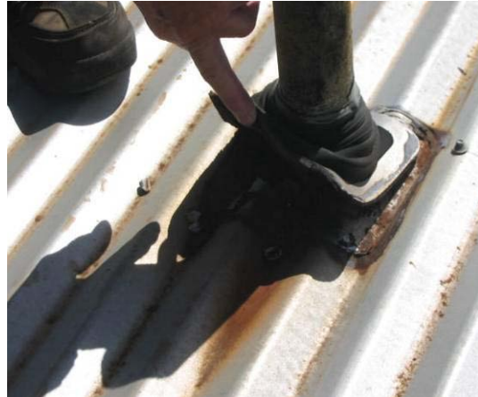
b. Badly corroded steel around exhaust stack
