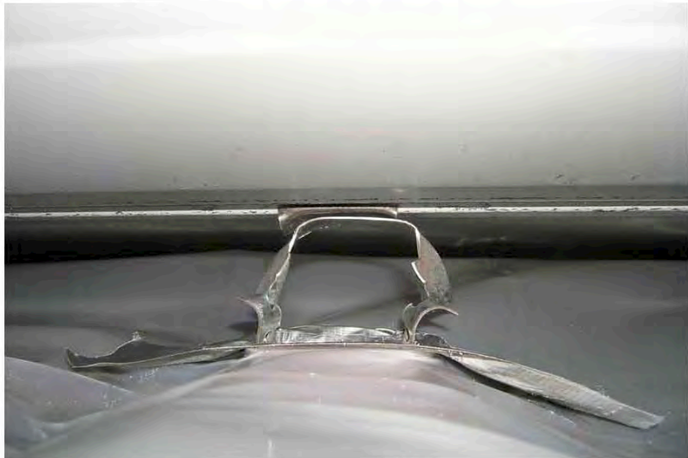
PHOTOGRAPH 12 EXPANSION CLIP FAILURE
