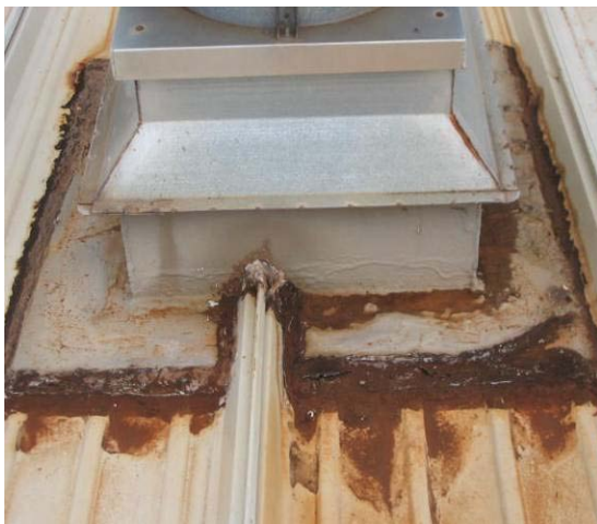
c. Severe corrosion around air vent.
