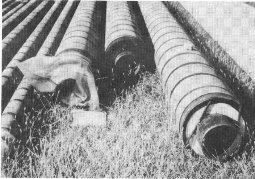
Figure 1. Conduit without protective covers.
