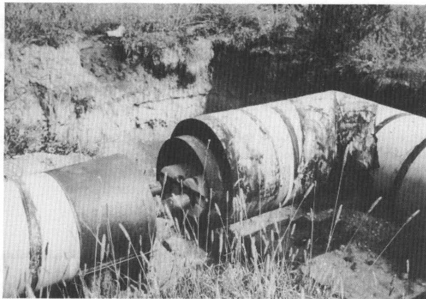
Figure 2. Thermal insulation exposed to rain and condensation.
