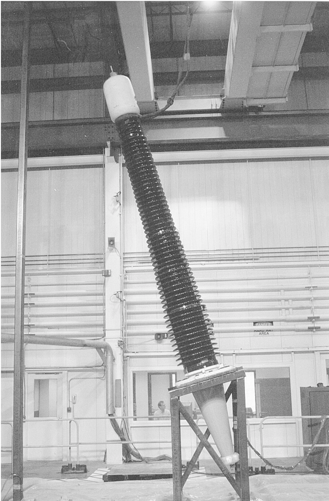
Figure 1. TVA power transformer bushing tested on the USACERL TESS.
