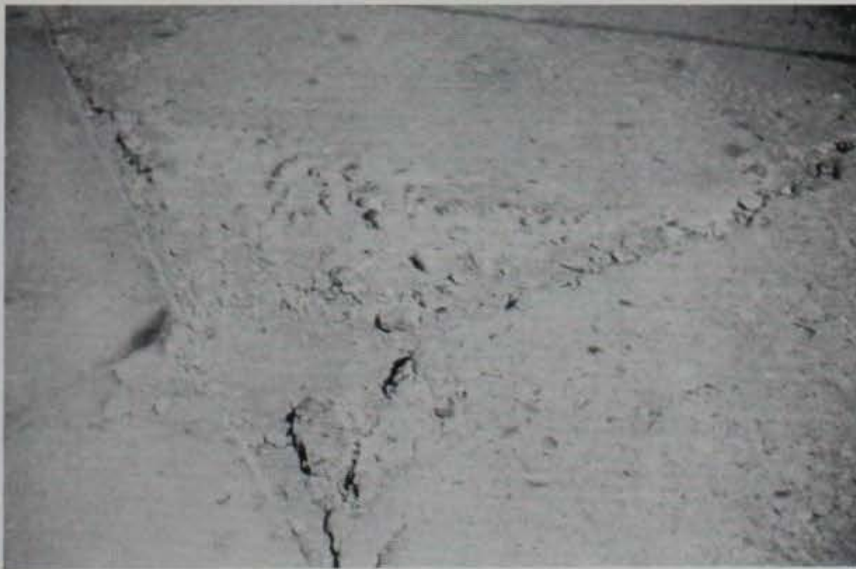
Figure 38c. High-Severity Spalling, Corner.
