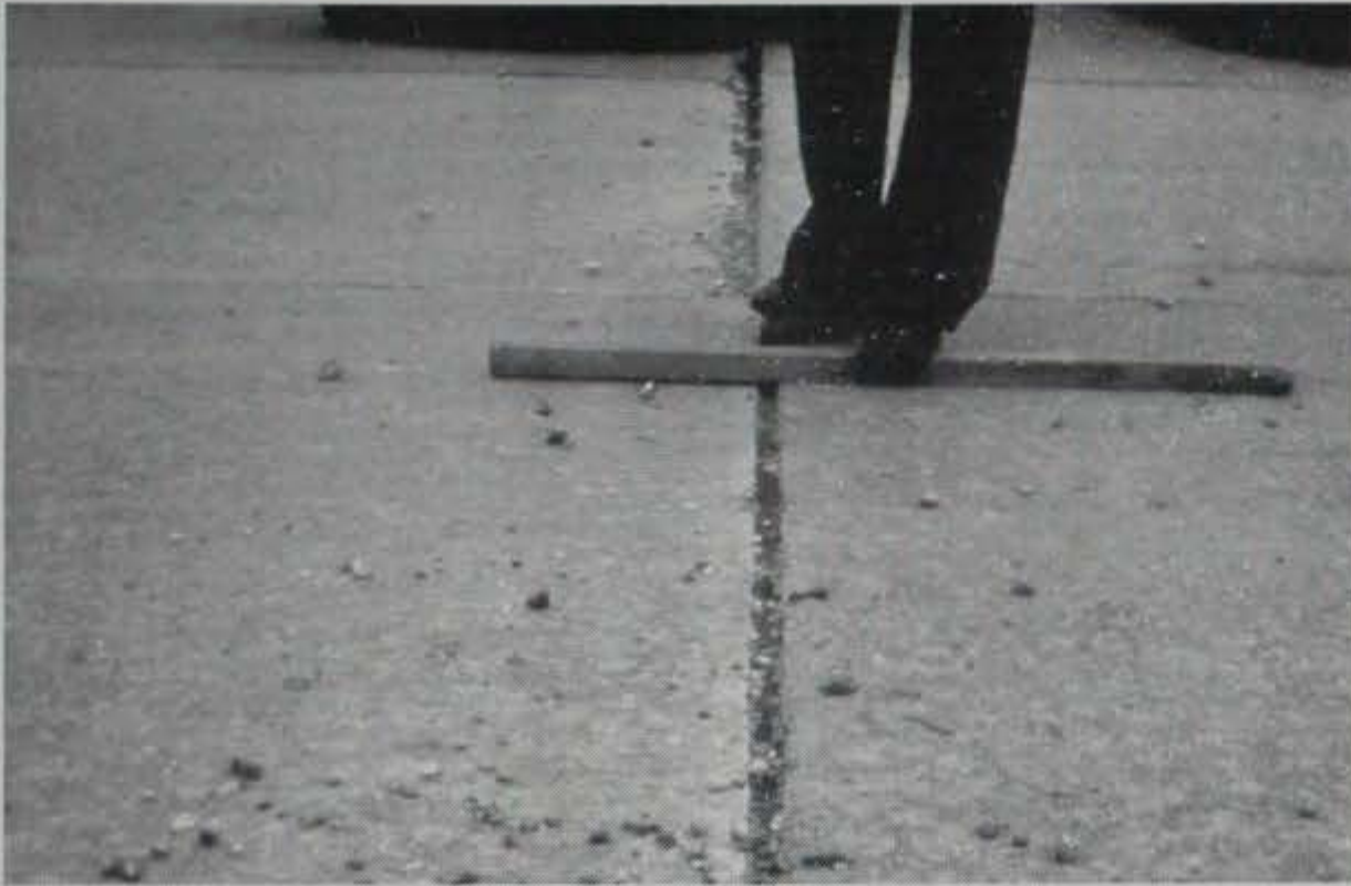
Figure 25a. Low-Severity Faulting.
