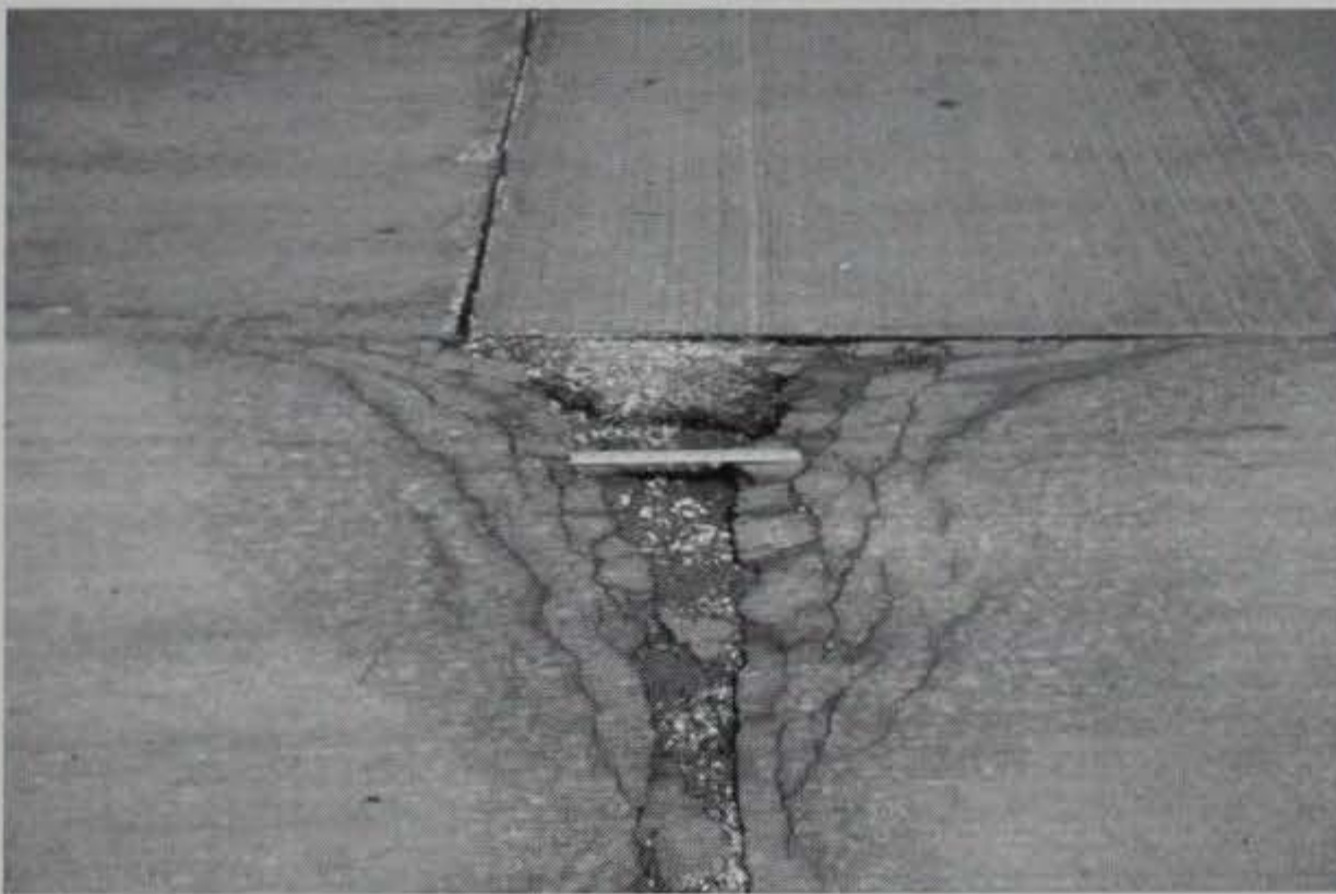
Figure 24b. Medium-Severity Durability Cracking.
