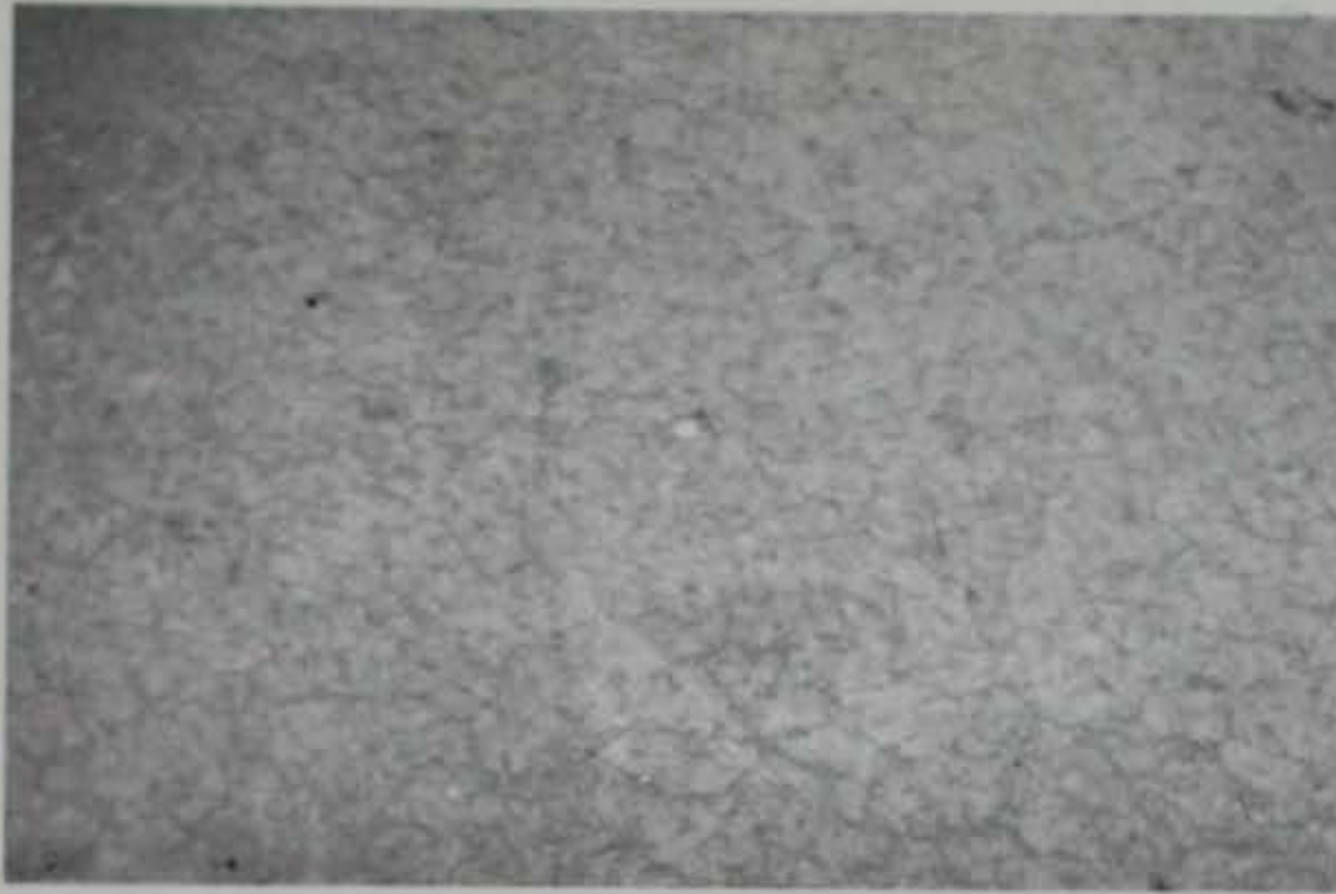
Figure 36a. Low-Severity Scaling, Map Cracking, and Crazing.
