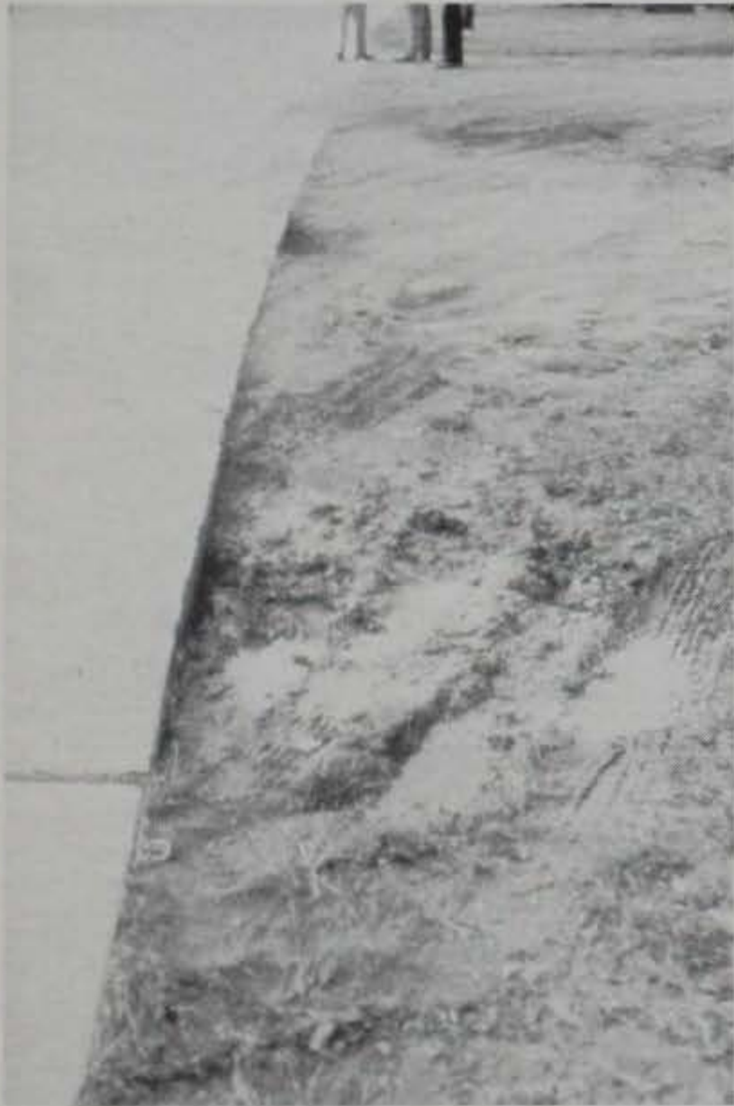
Figure 27b. Medium-Severity Lane/Shoulder Drop-Off.
