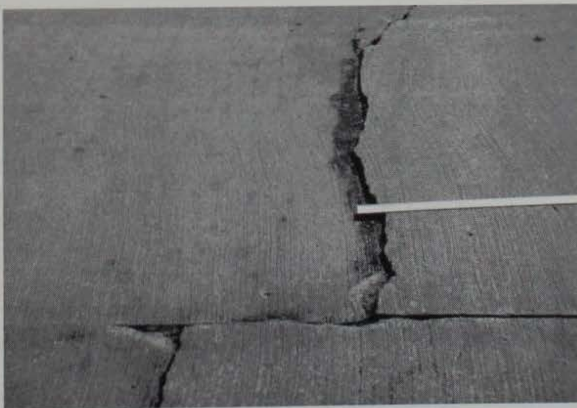
Figure 28c. High-Severity Linear Cracking.
