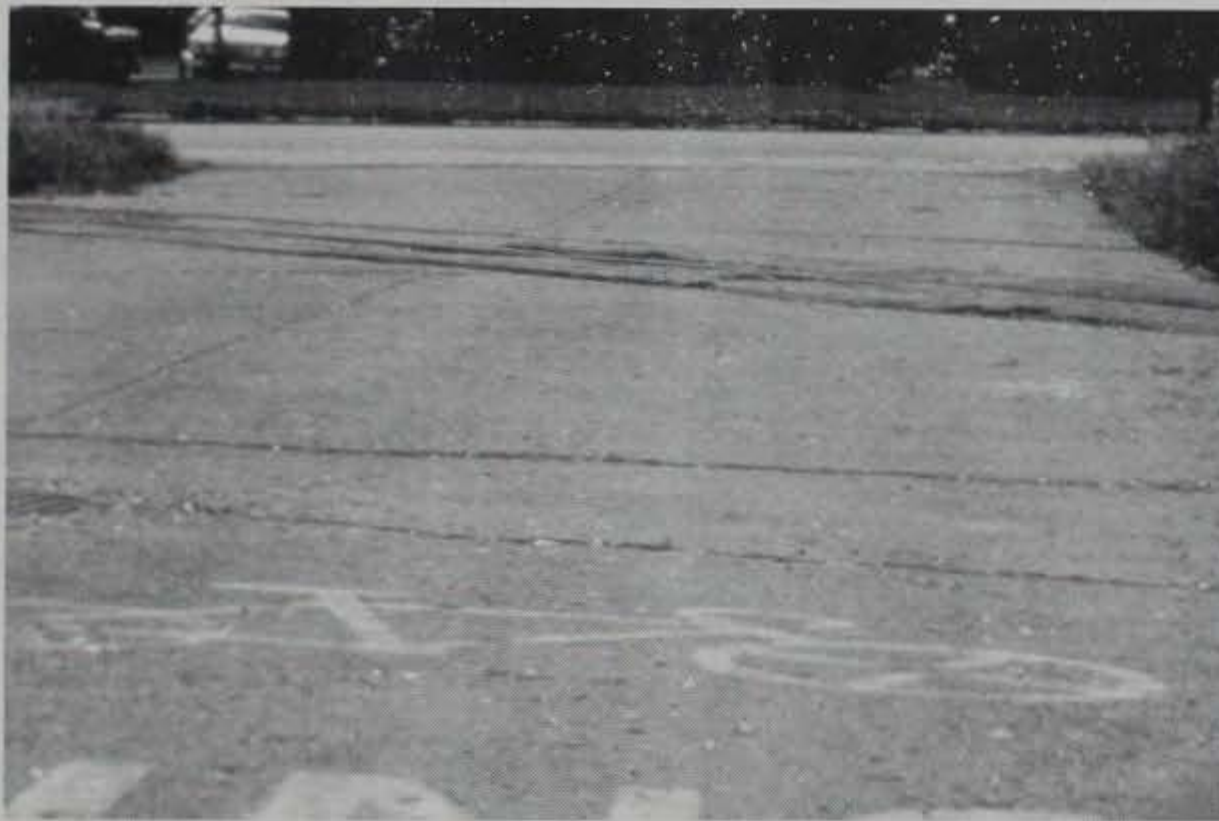
Figure 35b. Medium-Severity Railroad Crossing.
