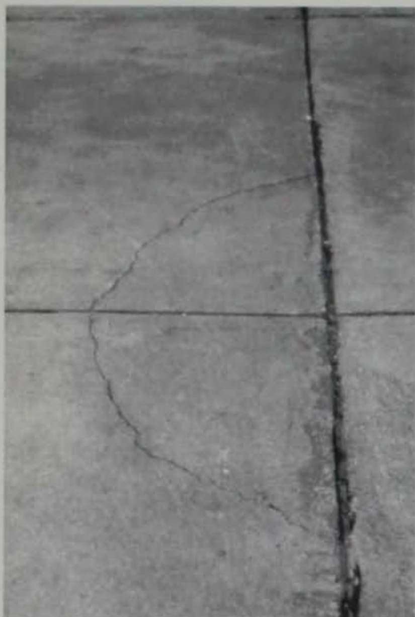
Figure 22a. Low-Severity Corner Break.
