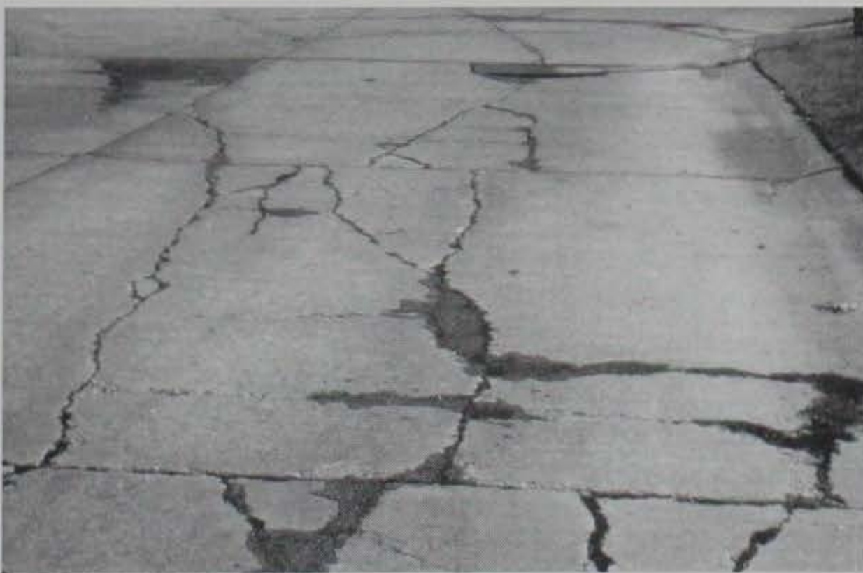
Figure 23c. High-Severity Divided Slab.
