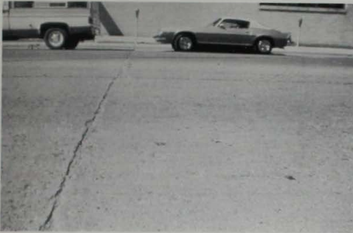
Figure 39a. Low-Severity Spalling, Joint.
