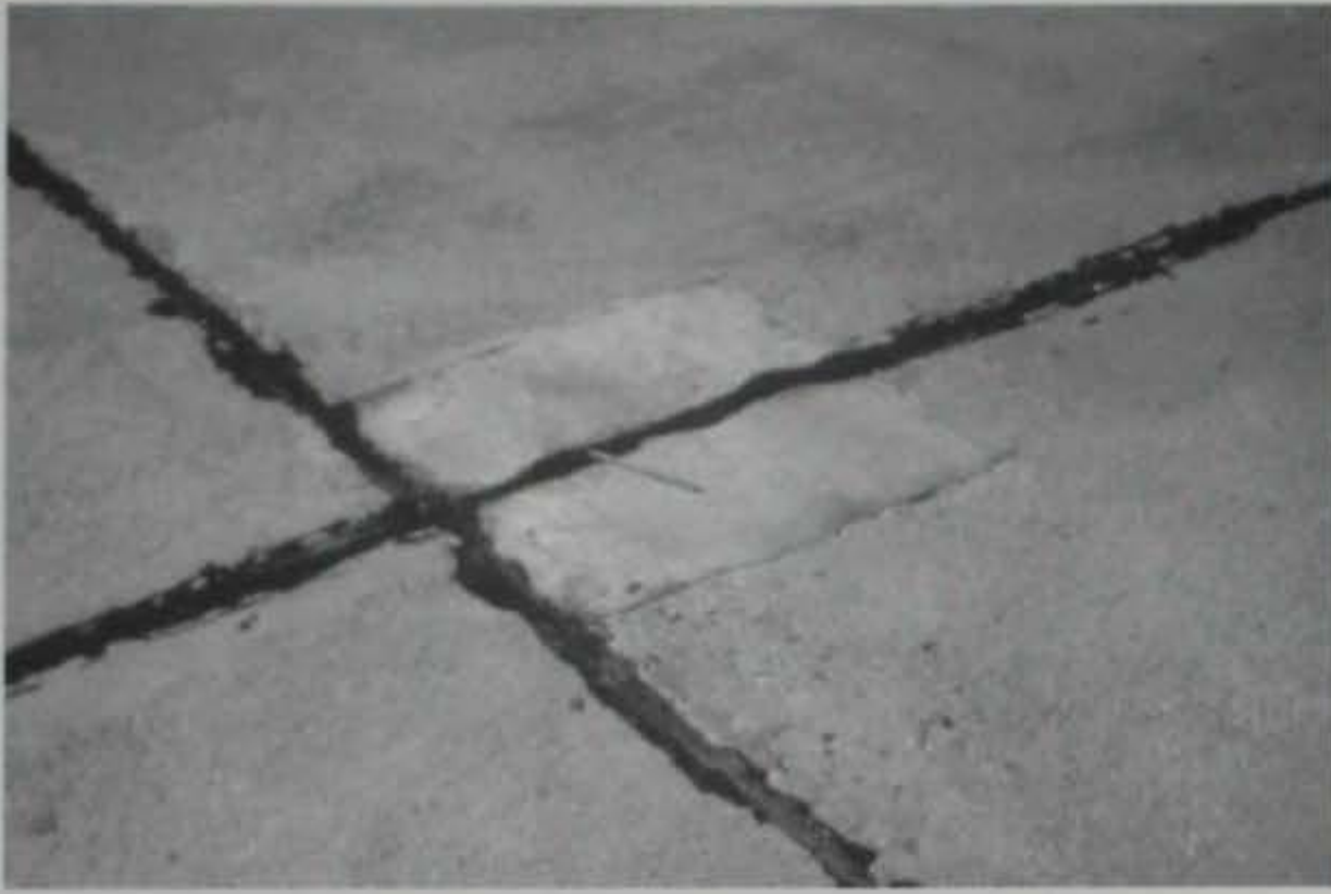
Figure 30a. Low-Severity Patching, Small.
