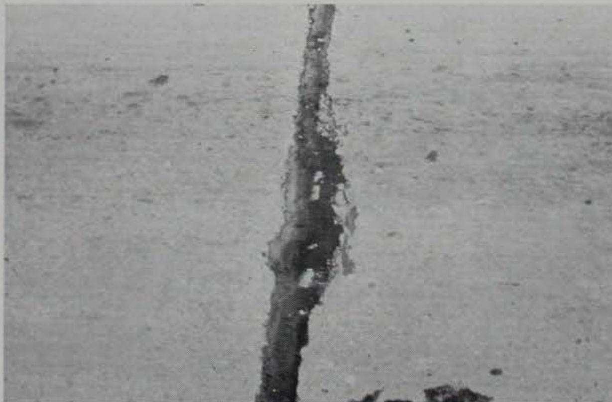
Figure 26b. Medium-Severity Joint Seal Damage.
