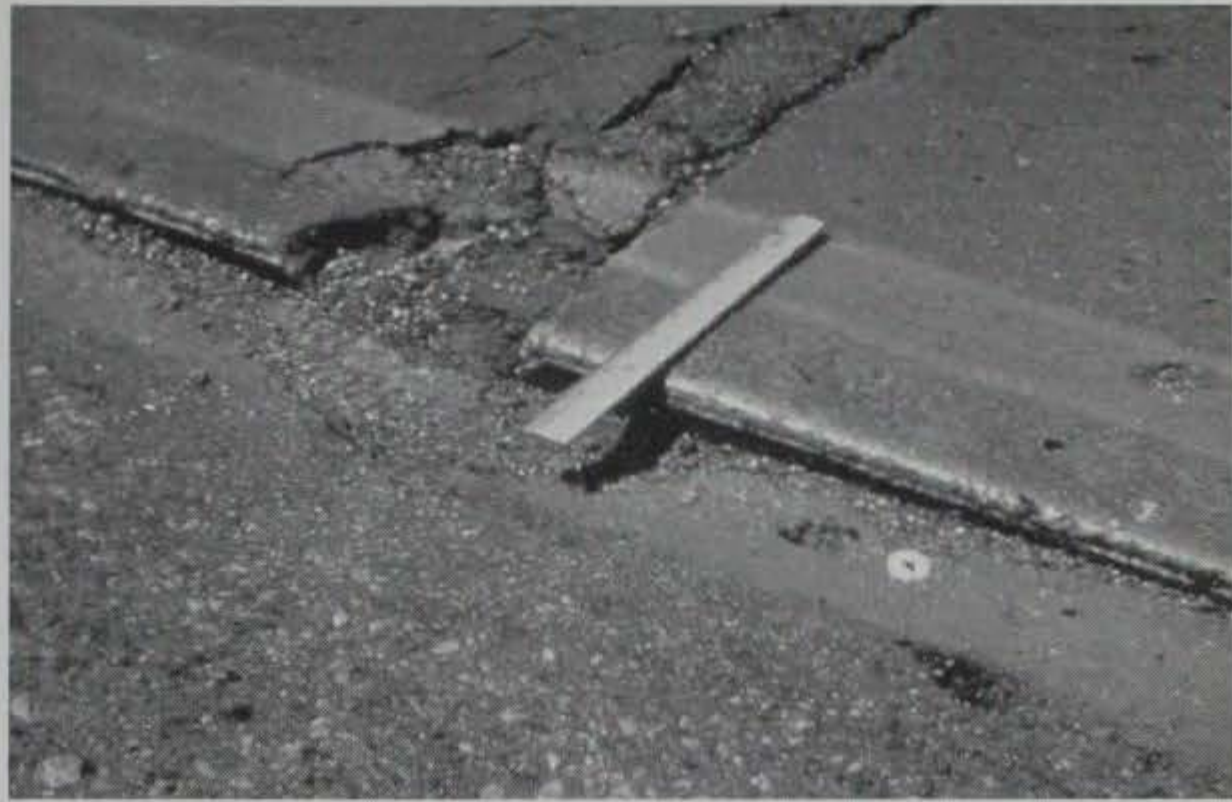
Figure 27a. Low-Severity Lane/Shoulder Drop-Off.
