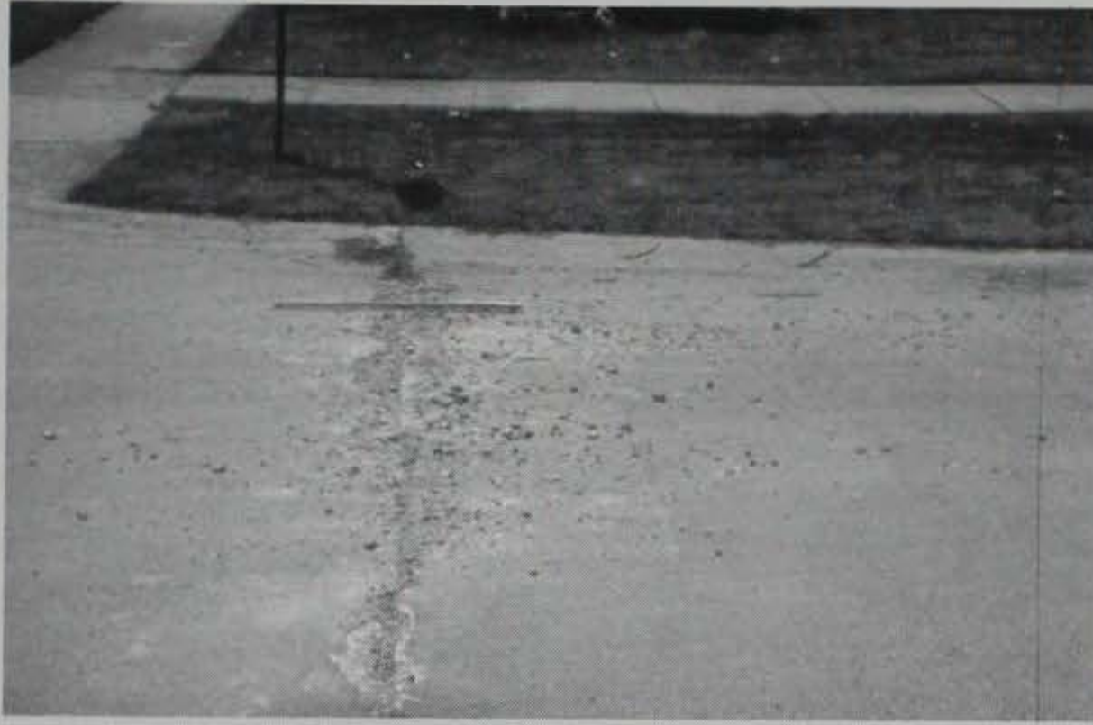
Figure 21a. Low-Severity Blowup/Buckling.
