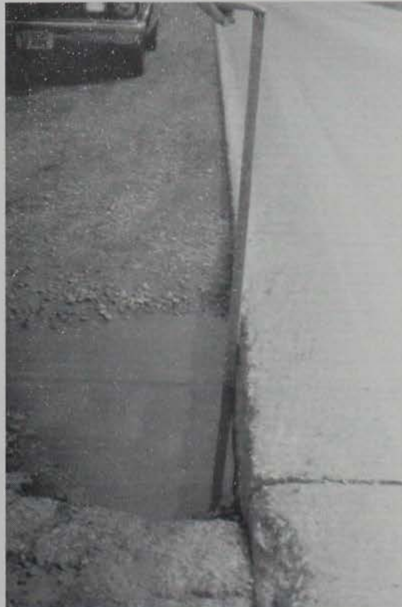
Figure 27c. High-Severity Lane/Shoulder Drop-Off.
