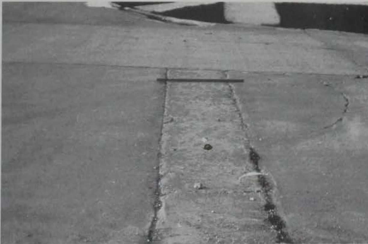
Figure 29b. Medium-Severity Patching, Large and Utility Cuts.
