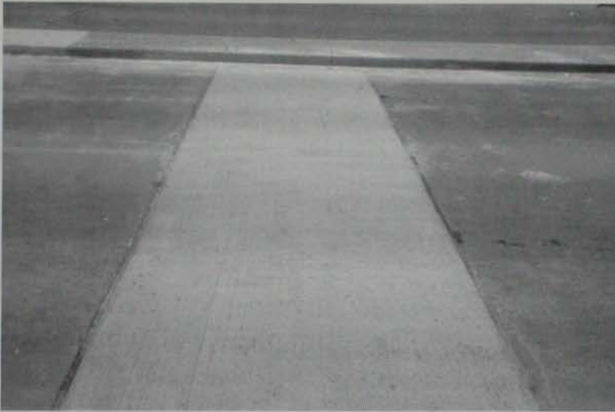
Figure 29a. Low-Severity Patching, Large and Utility Cuts.
