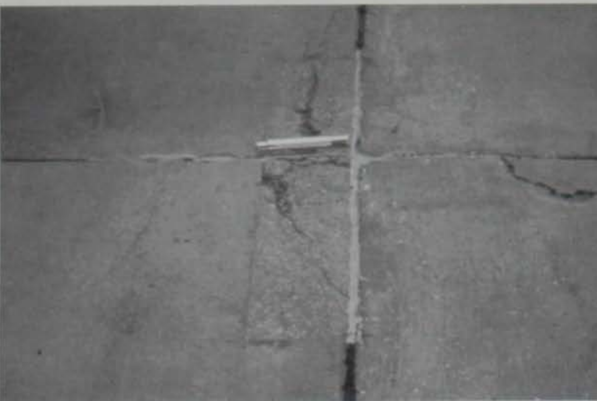
Figure 30c. High-Severity Patching, Small.
