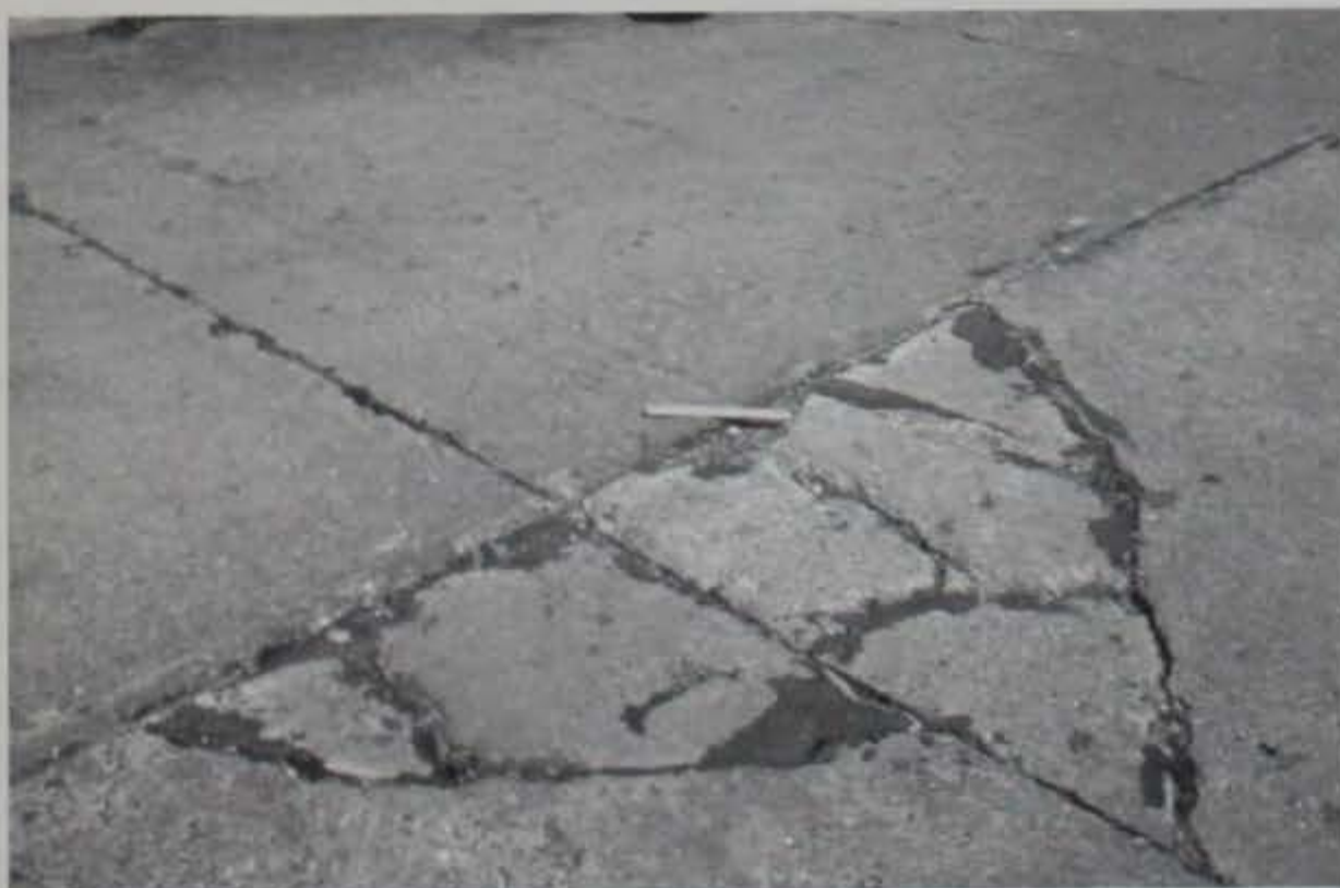
Figure 22c. High-Severity Corner Break.
