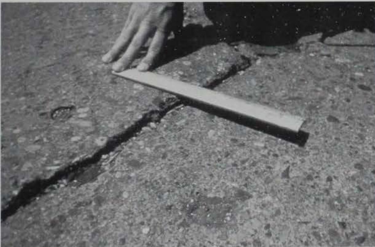
Figure 25b. Medium-Severity Faulting.
