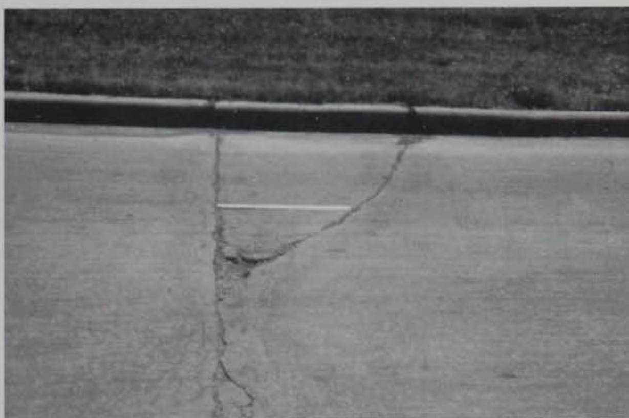
Figure 22b. Medium-Severity Corner Break.
