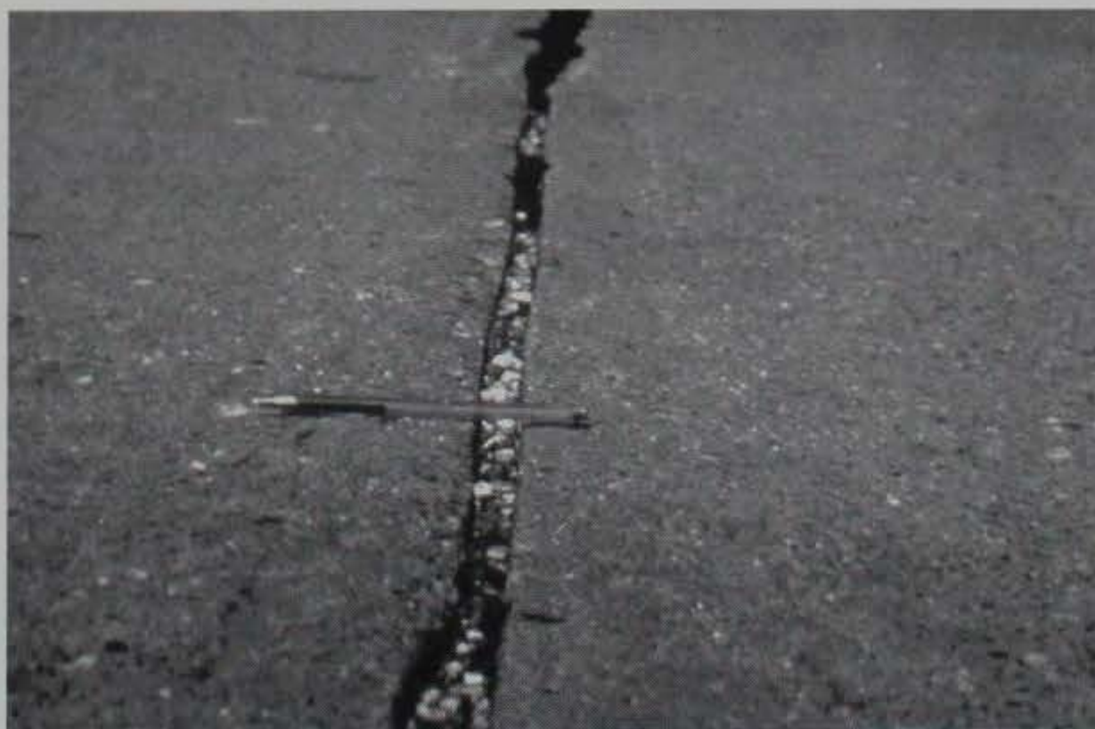
Figure 26c. High-Severity Joint Seal Damage.
