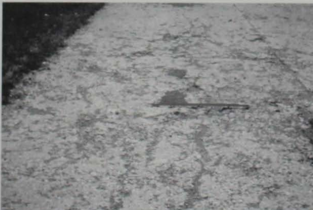
Figure 36c. High-Severity Scaling, Map Cracking, and Crazing.
