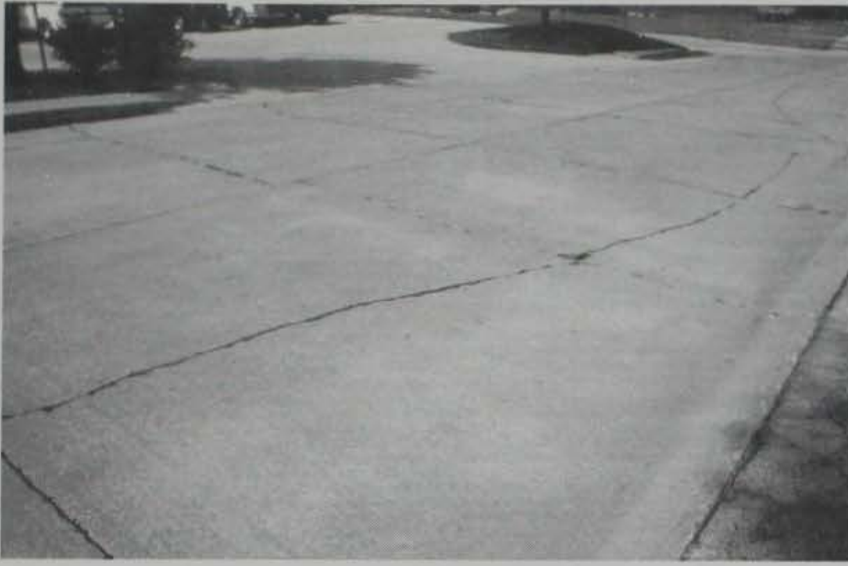
Figure 23a. Low-Severity Divided Slab.
