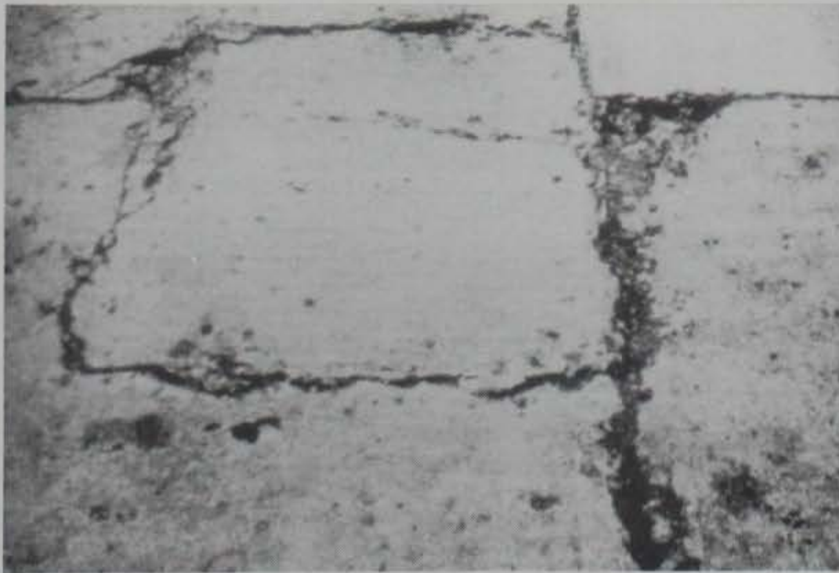
Figure 29c. High-Severity Patching, Large and Utility Cuts.
