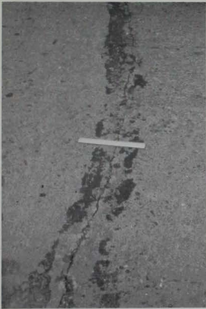
Figure 28a. Low-Severity Linear Cracking.
