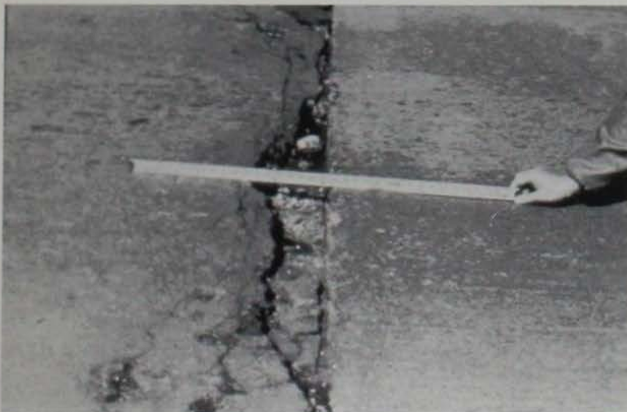
Figure 39c. High-Severity Spalling, Joint.
