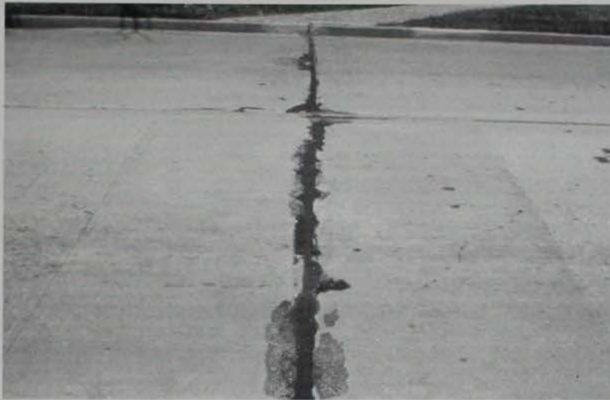
Figure 26a. Low-Severity Joint Seal Damage.
