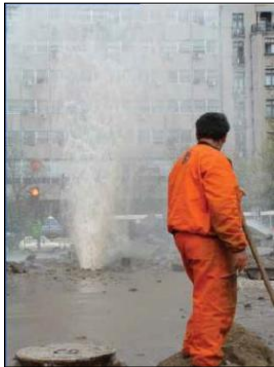
Figure 2. Leaks that are ignored can cause disruptive and costly failures.
