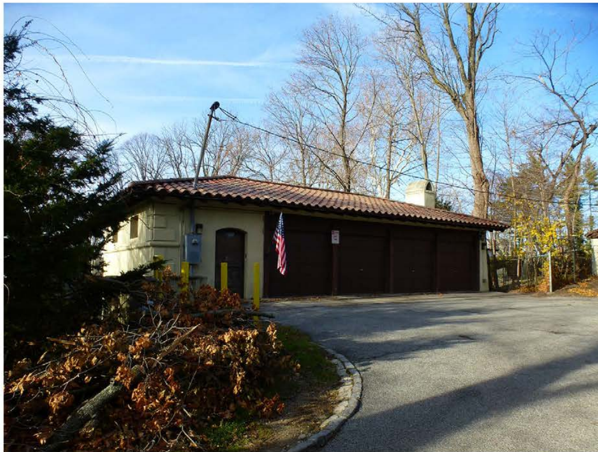
Photo 52. View to the northwest of the entrance door and garage doors on the east facade of the garage building.
