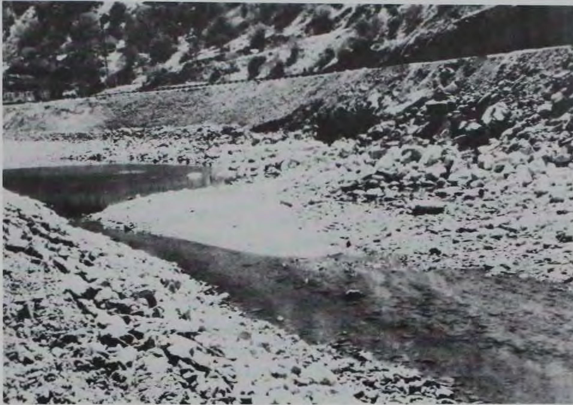
a. Closeup of failure of opposite bank
