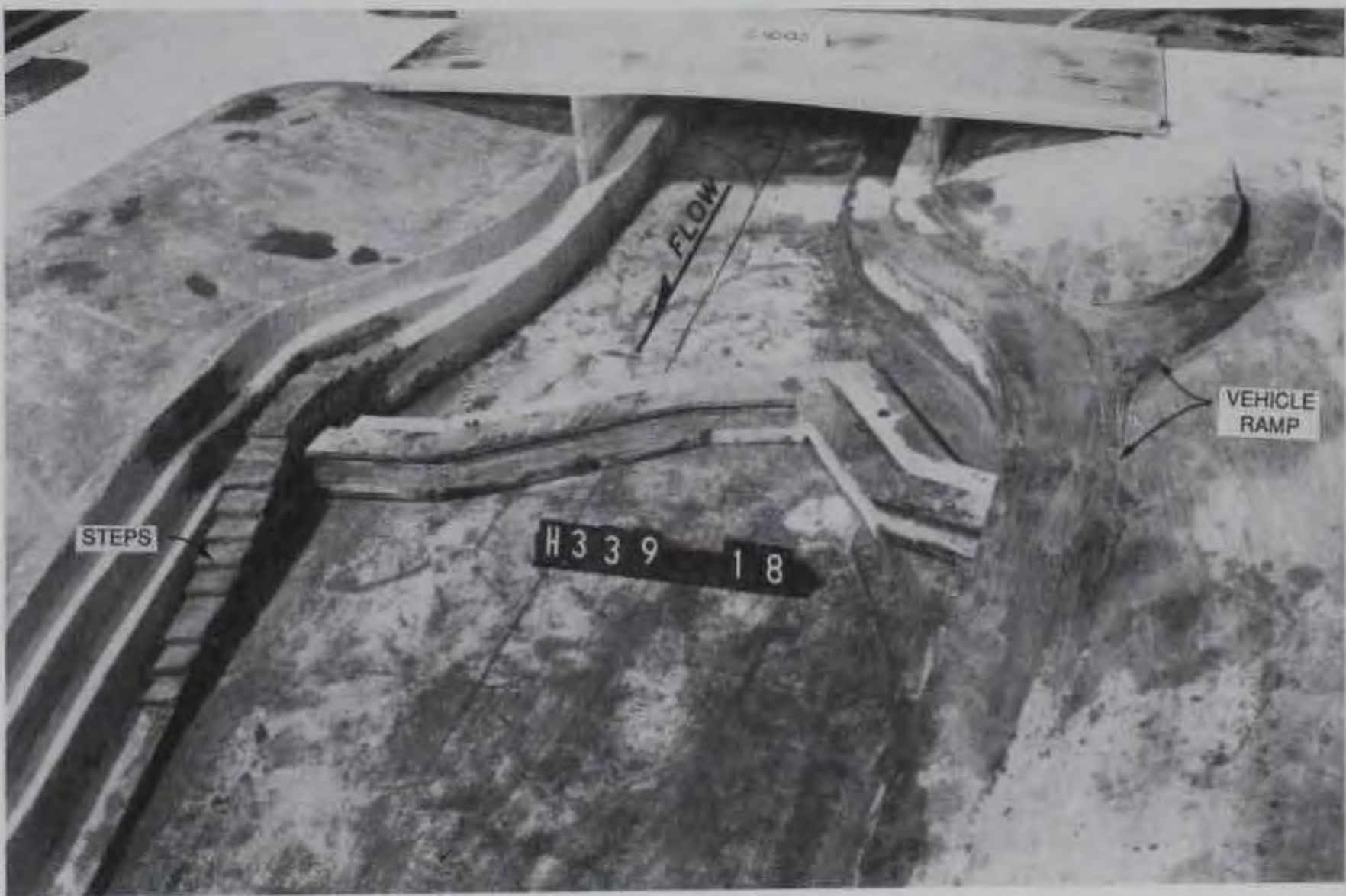
Photo 42. Irregular dam 1, sta 68+65
