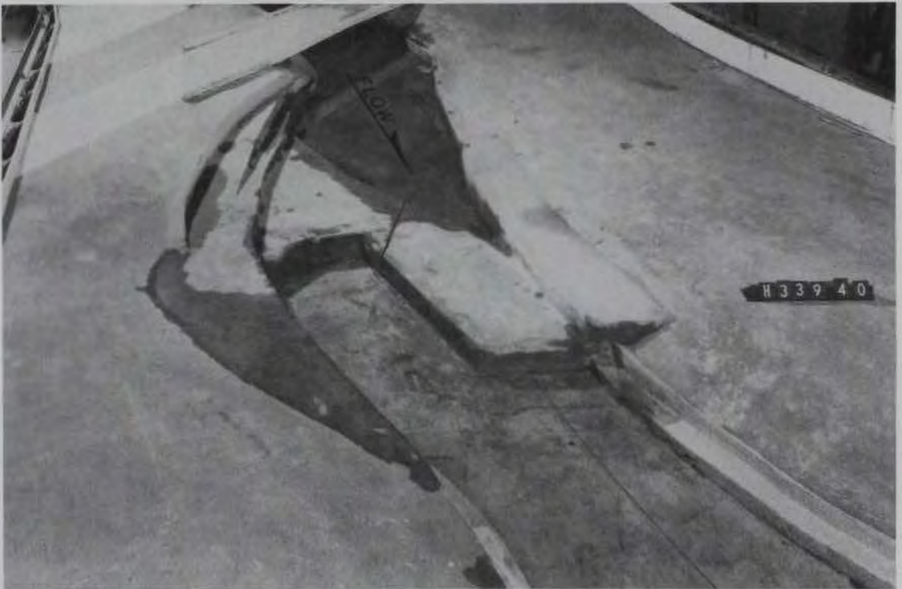
Photo 44. Irregular dam 1, sta 79+00
