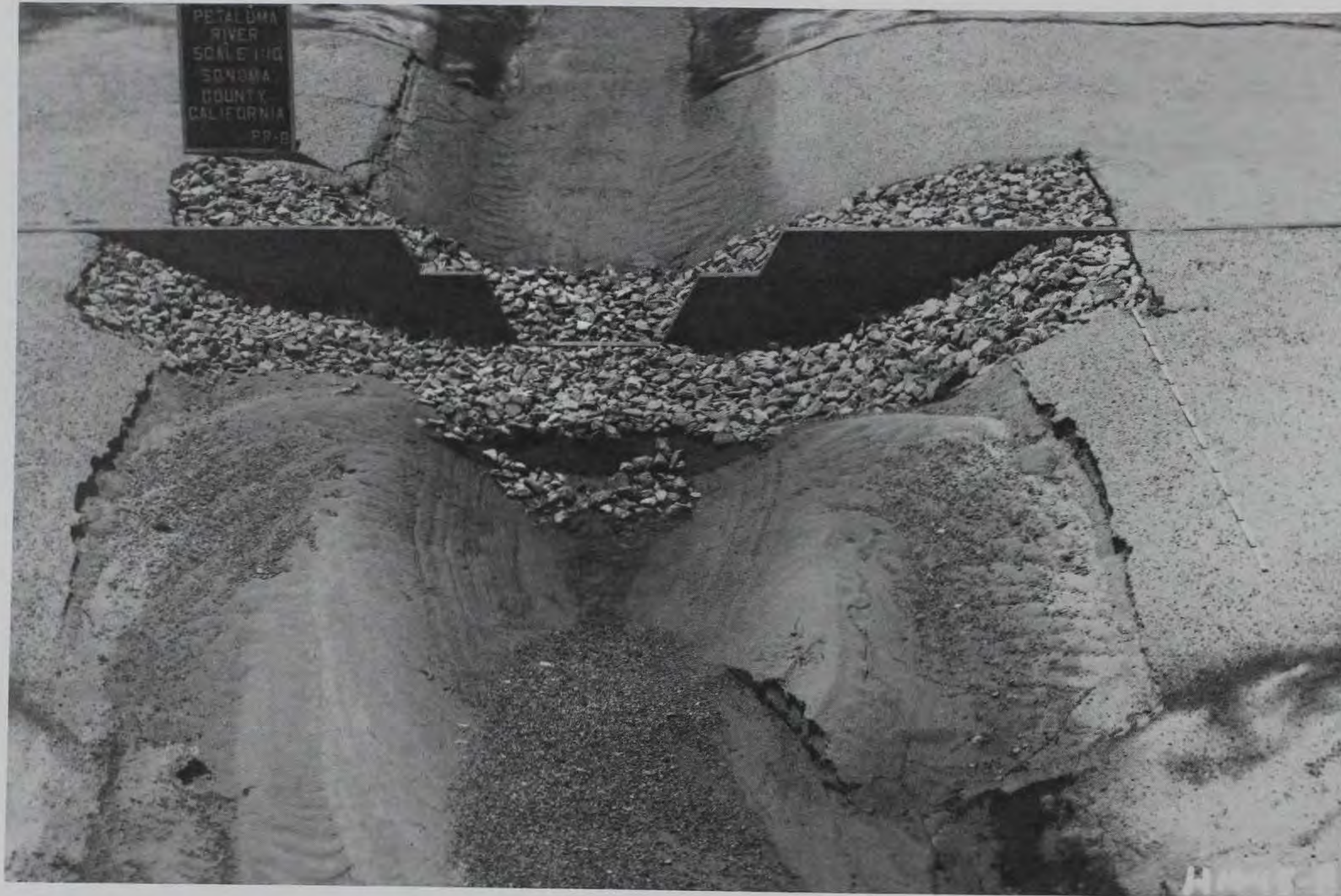
Photo 4. Riprap failure, upstream view; same flow conditions as shown in Photo 1
