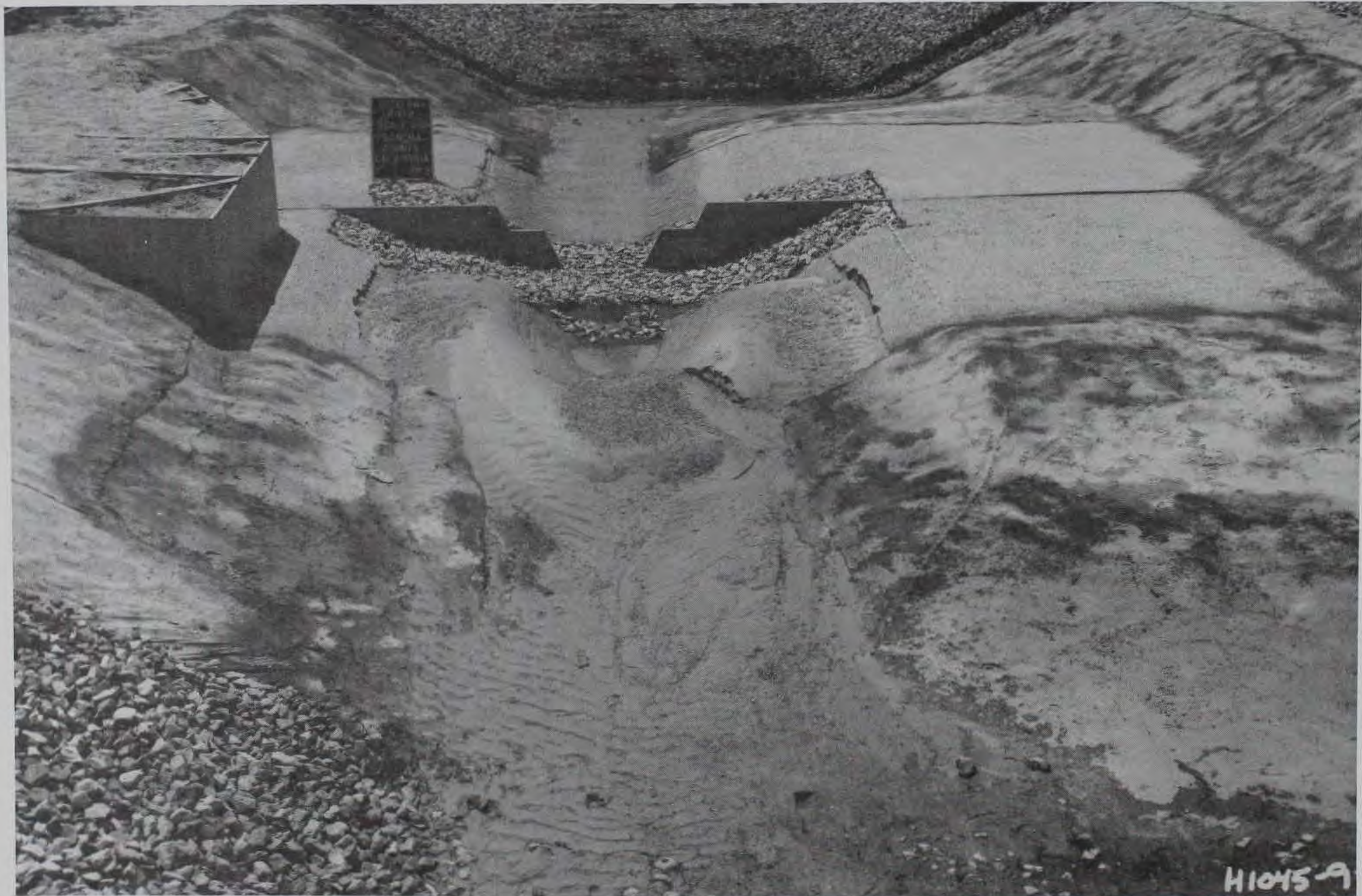
Photo 3. Riprap failure, upstream general view; same flow conditions as shown in Photo 1
