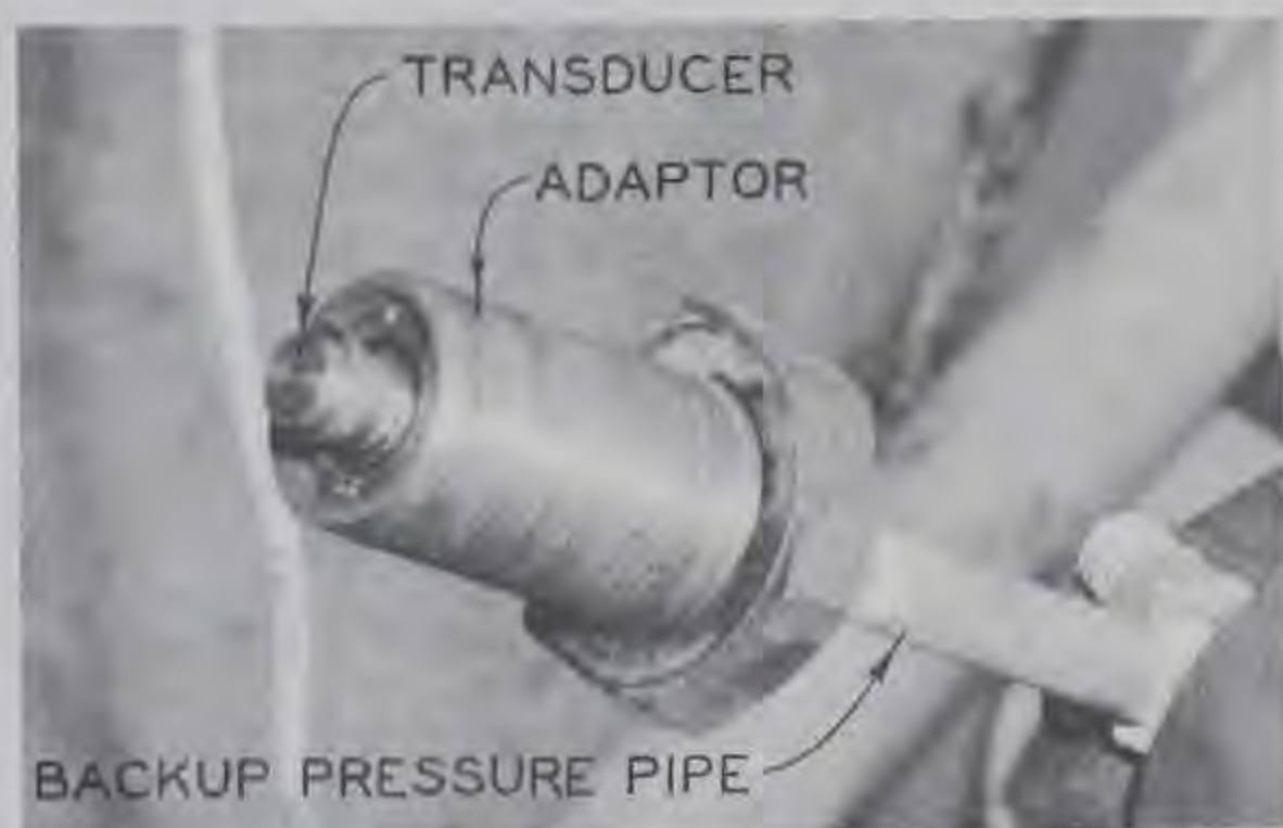
Fig. 7. Pressure transducer PS4 (flange not shown)
