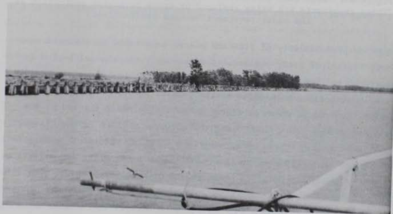
Figure 97. Older style pile revetment used for bank protection on the Missouri River
