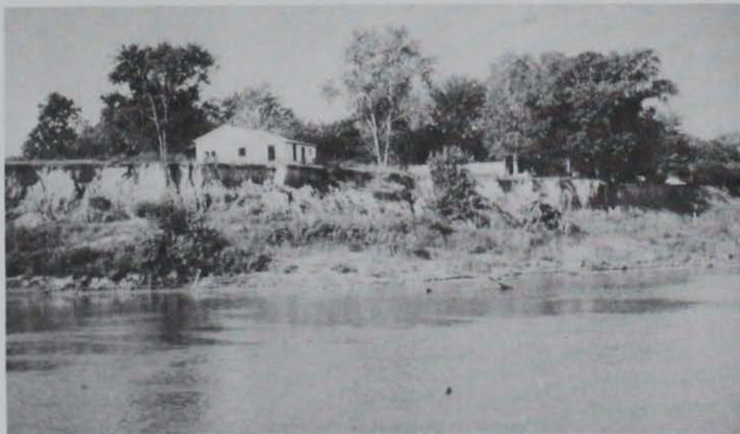
Figure 55. Section of the west bank at Des Arc, Ark., where active bank failure is occurring (The white frame house in the left center of the photograph can also be seen in the aerial photograph in Figure 46.)
