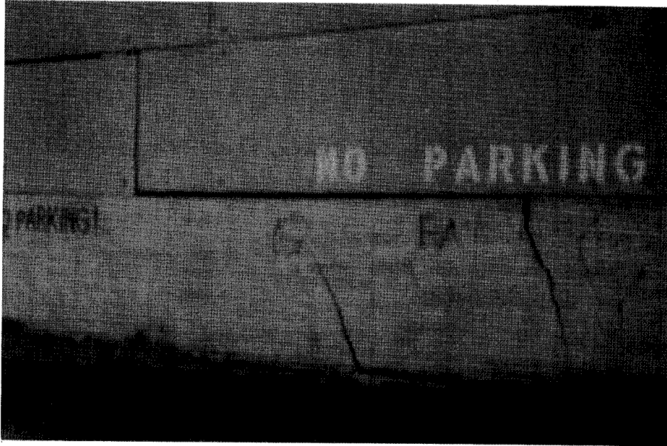
a. Settlement and cracking of structure on Pier 45
