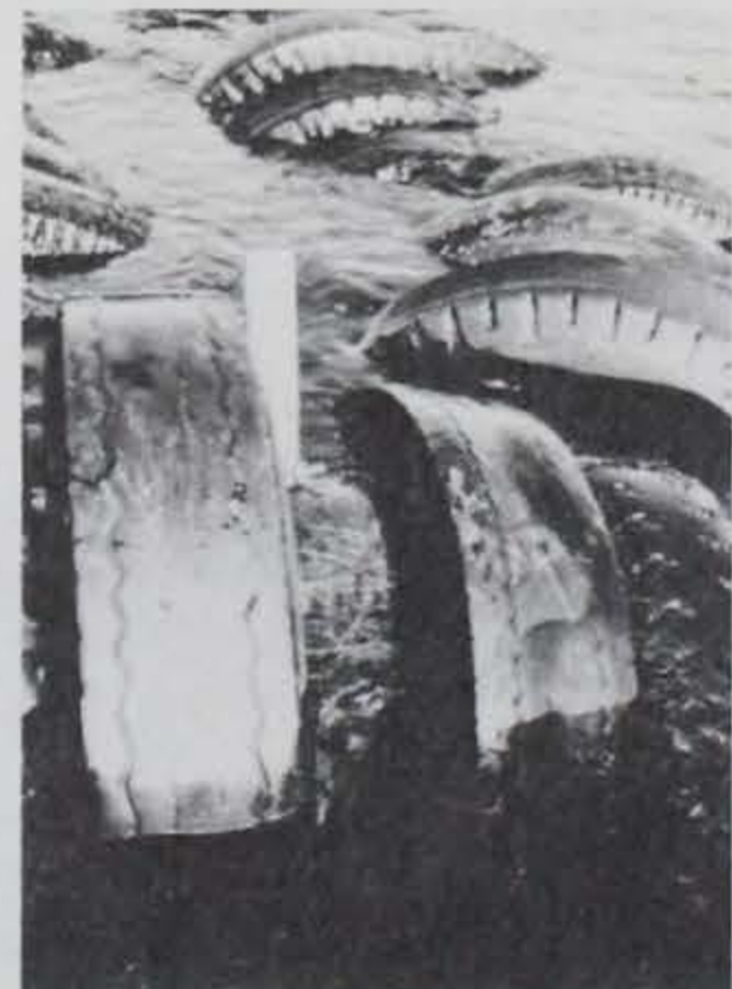
Photo B-30. Photo showing keeper pipe repair which prevented additional tires from falling off.
