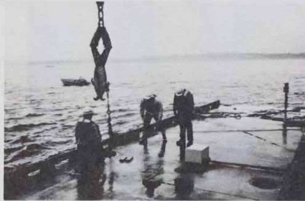
Photo C-28. Unanchoring the concrete breakwater for the second time (keeper plate on deck).
