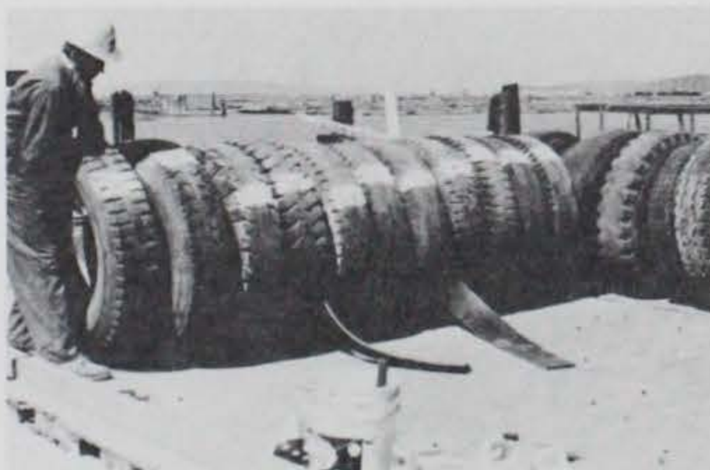
Photo B-5. Placing the first row of 11 tires (note belting around center 3 tires).
