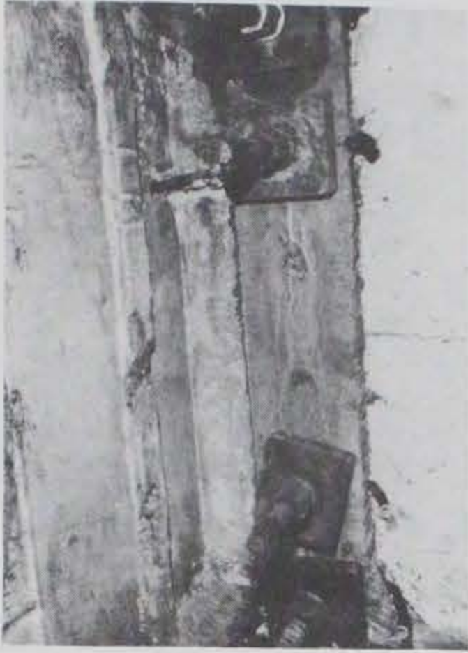
Photo D-19. Photo depicting inside of float with four tensioned bars near center line.
