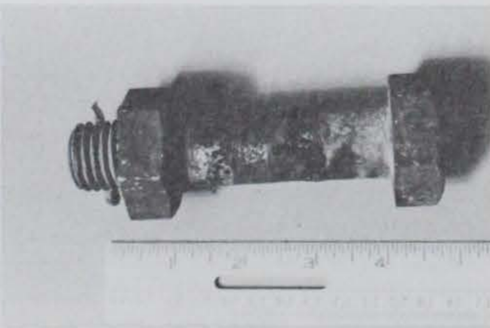
Photo C-23. Photo depicting corrosion of the mild steel cotter key in a shackle bolt.
