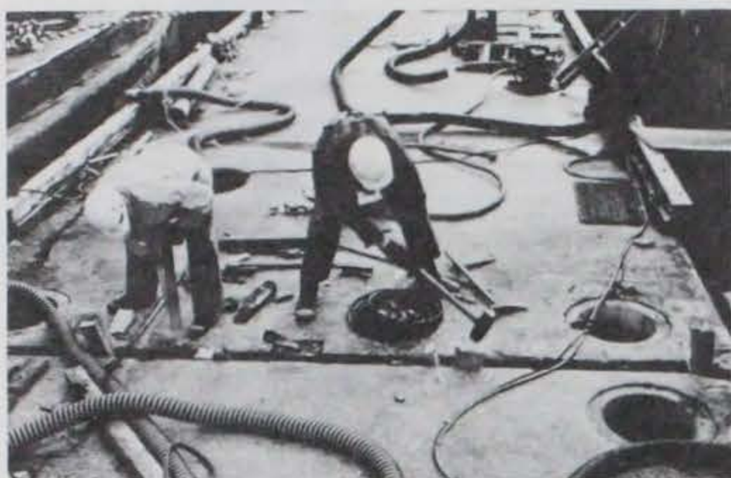
Photo D-25. Floats being parted after rigid connection bars have been detensioned.
