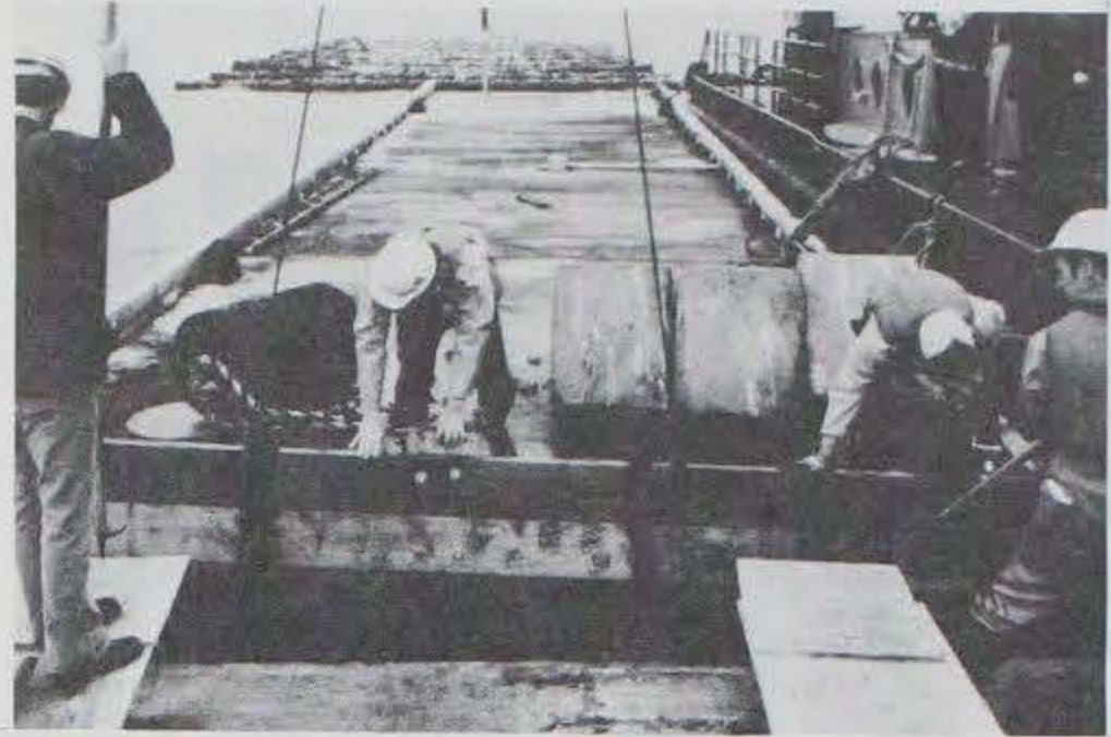
Photo D-8. Two 3- by 12-in. timbers being bolted between the bumper plates.
