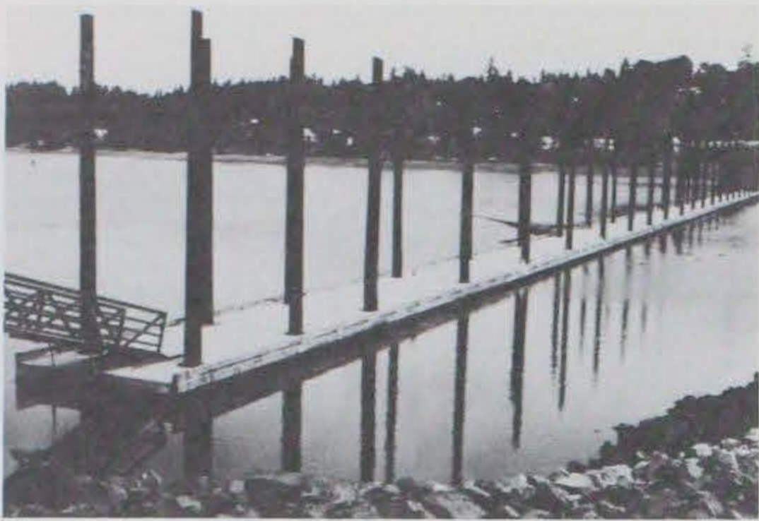
Photo 25. Photo showing the 16-ft-wide by 600-ft-long piling moored breakwater at East Bay, Washington.
