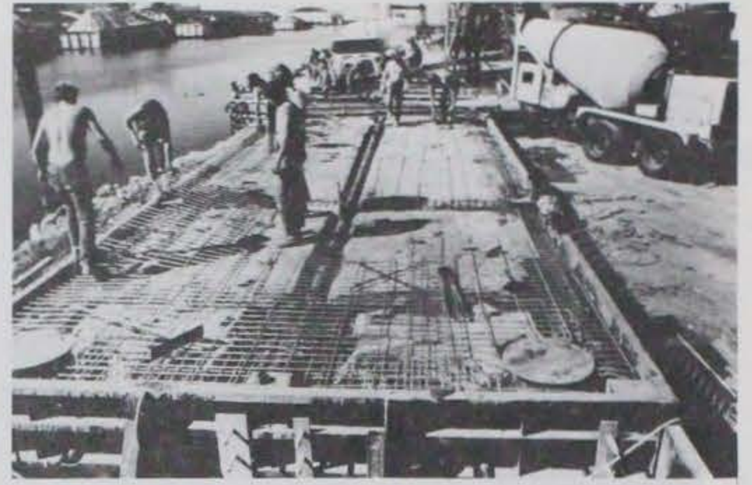
Photo A-8. Fabric being placed carefully in corner areas (crossed rebar strain gages near center of photo).
