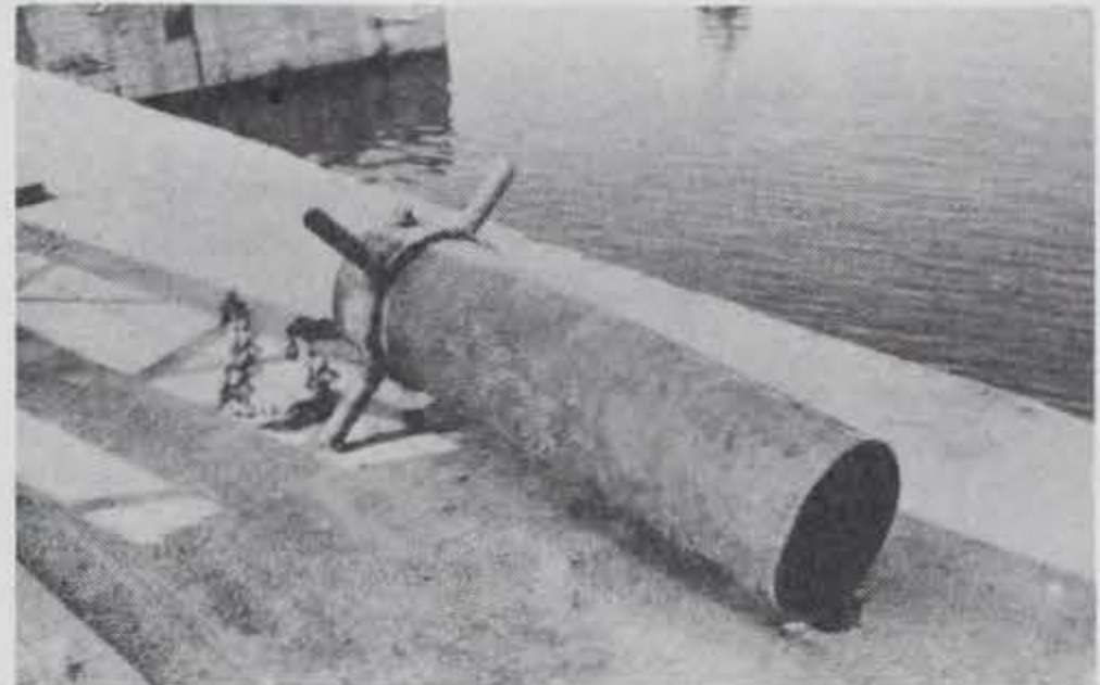
Photo B-34. Photo showing a clearly broken 5-ft section of pipe indicating an incomplete weld.
