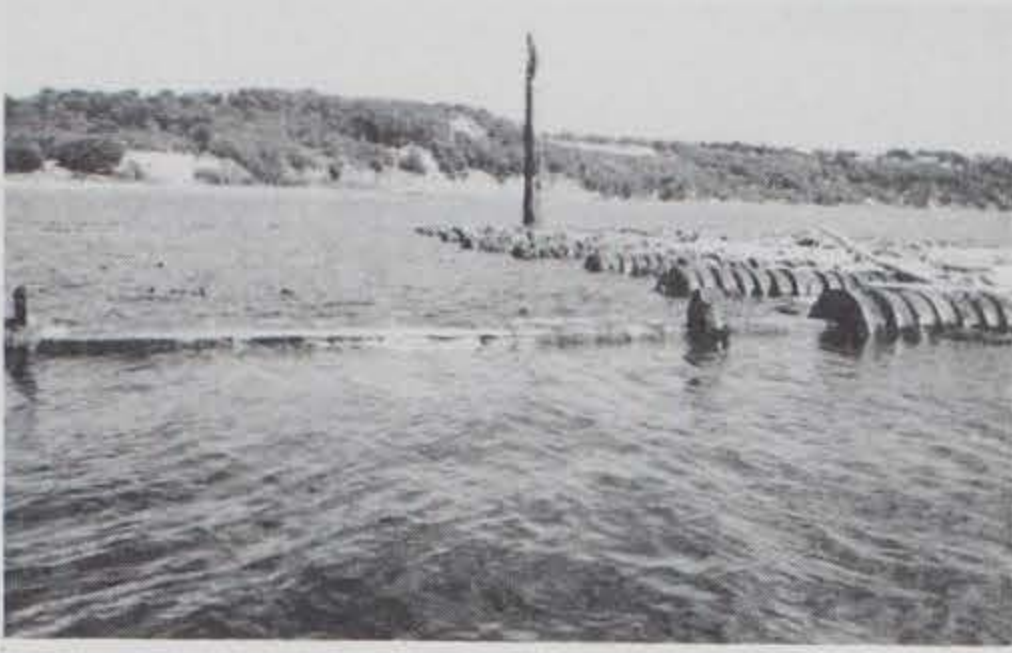
Photo B-31. A 45-ft pipe pulling out after breaking at a welded joint.
