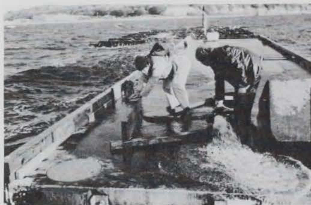
Photo A-22. About 3,000 gallons being pumped from an end compartment after a storm.
