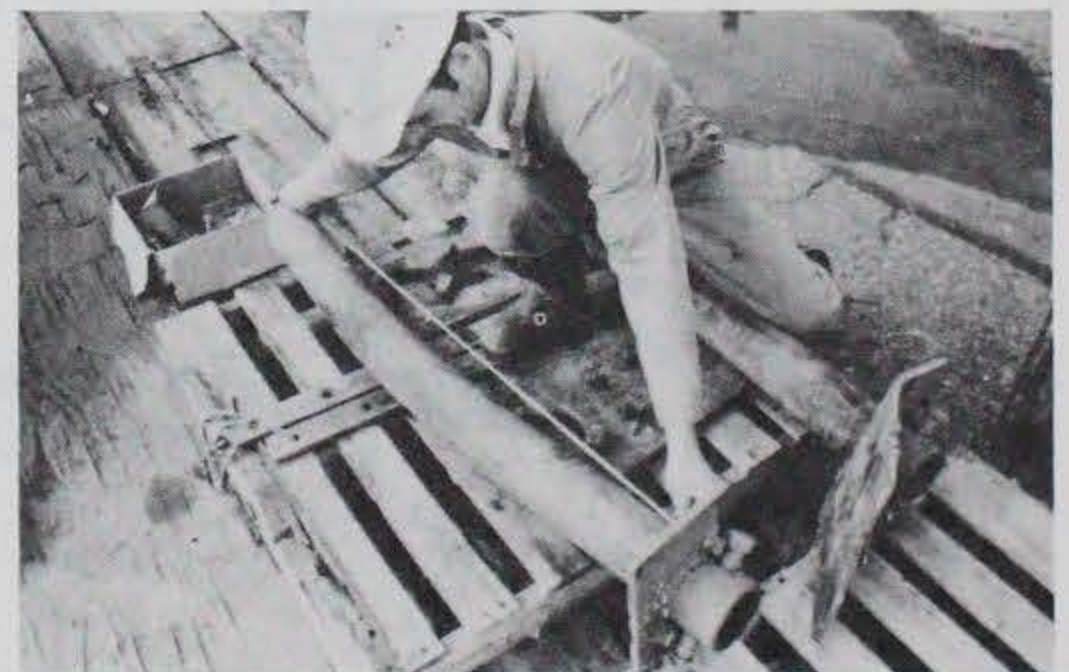
Photo D-6. Photo depicting failure of U-shaped brackets after 7 weeks.
