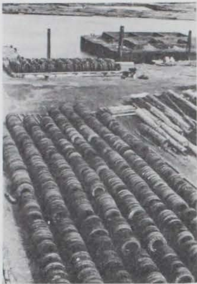
Photo B1. Truck tires (1,650) being prepared for assembly of the pipe-tire breakwater.
