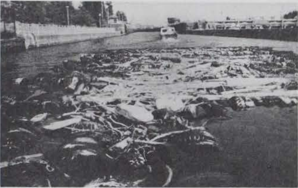
Photo B-33. The tire breakwater being removed from the test site on 5 August 1983.
