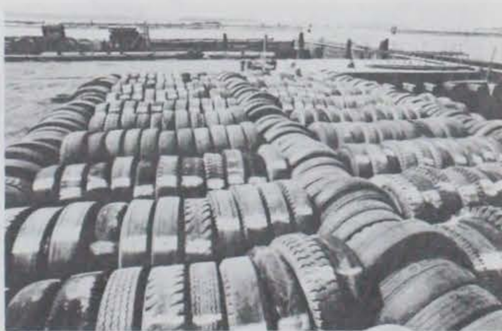
Photo B-17. Photo showing two bays of tires after being assembled on the platform.
