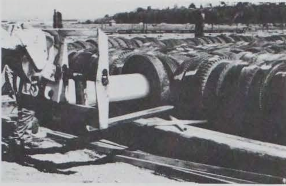
Photo B-19. Styrofoam-filled pipe being shoved through a beamwise row of tires.
