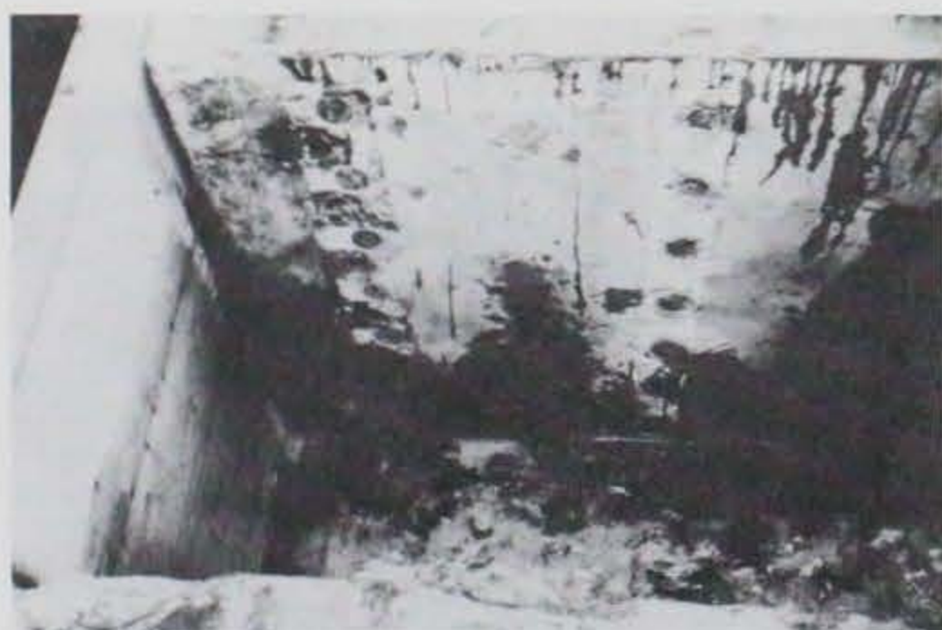
Photo D-17. Photo showing the end of the float after being cleaned and ground smooth.
