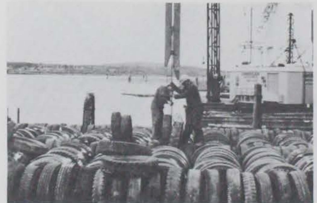
Photo B-18. Free tires being shoved into the beamwise row prior to insertion of the pipe.
