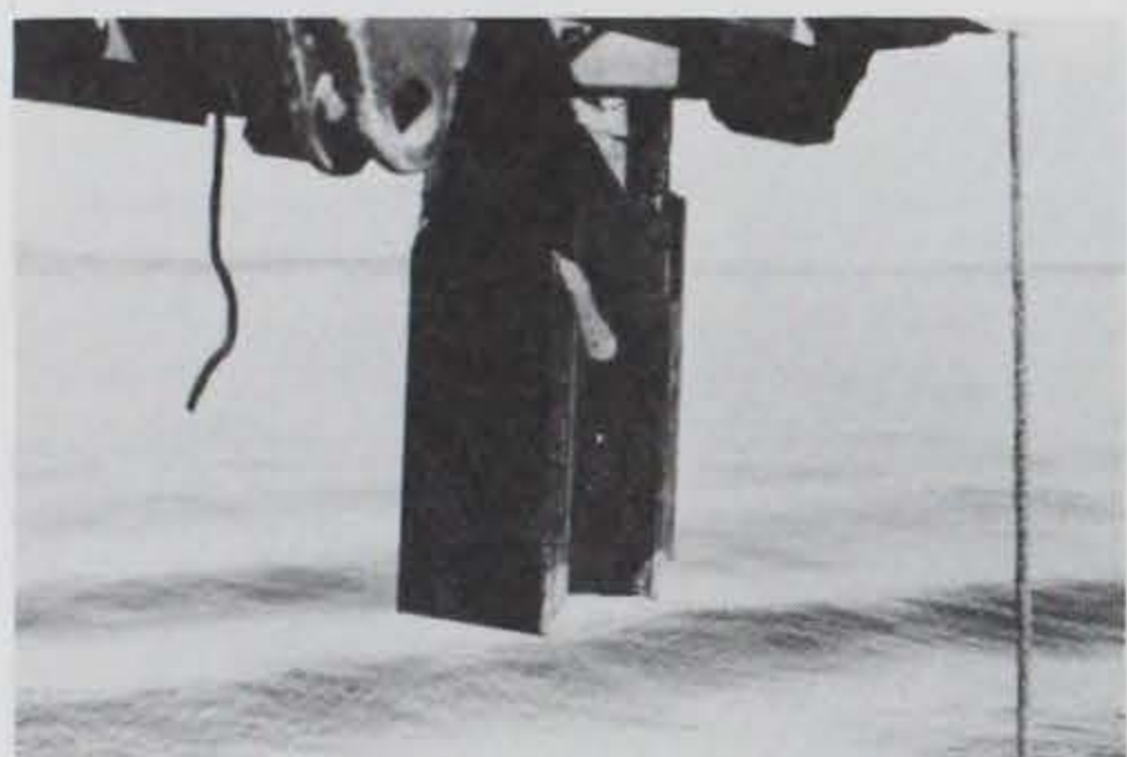
Photo C-9. Photo showing special fitting used to hold H-piles in proper alignment for driving.
