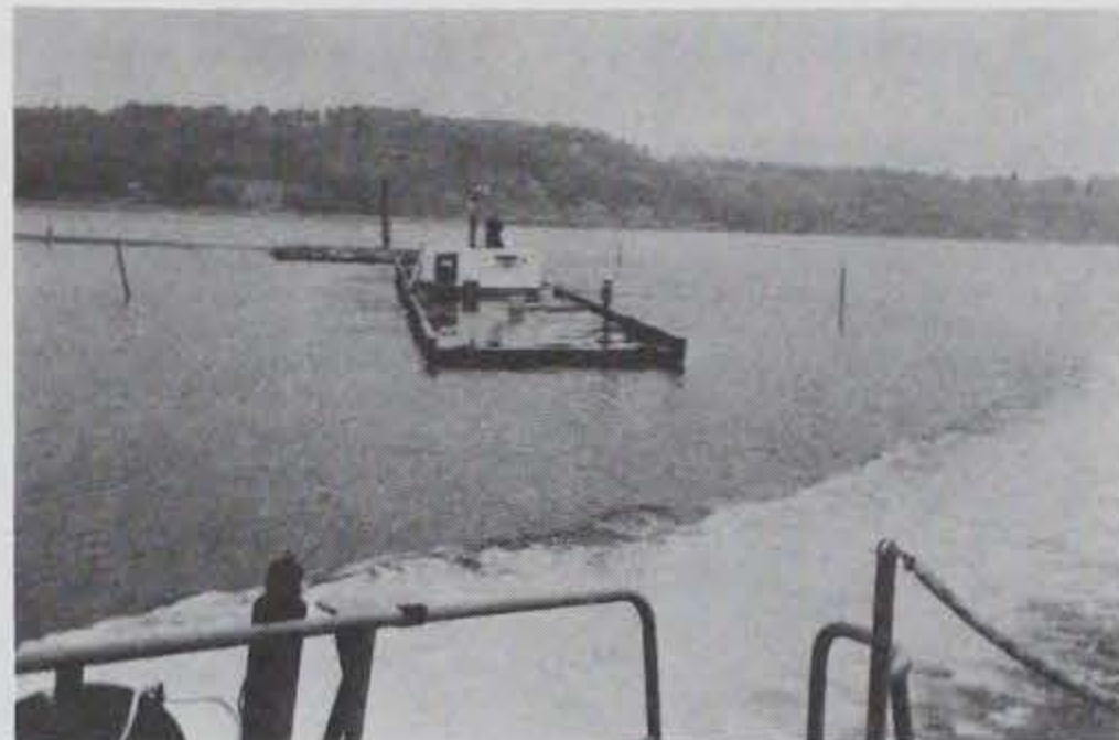
Photo E-4. The cutter traveling on a line at a 45-deg angle with respect to the breakwater.
