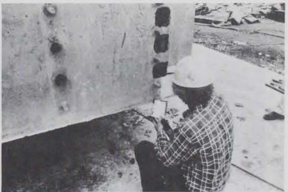
Photo A-18. Rubber patches being glued over the bolt holes (later covered by steel angles).
