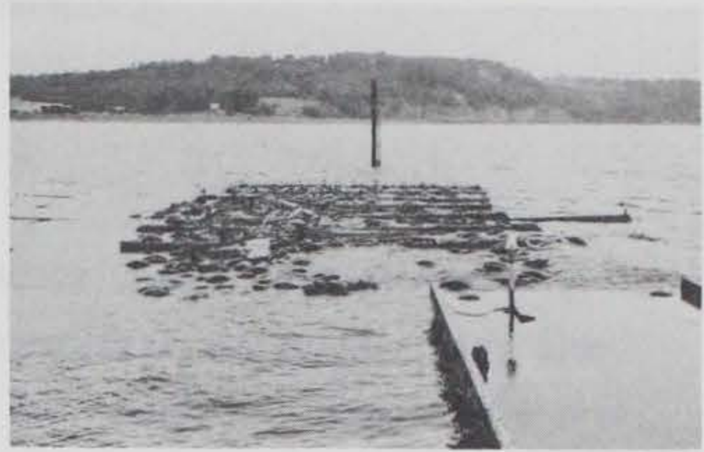
Photo B-32. The center pipe protruding from the breakwater after failure of keeper pipes.
