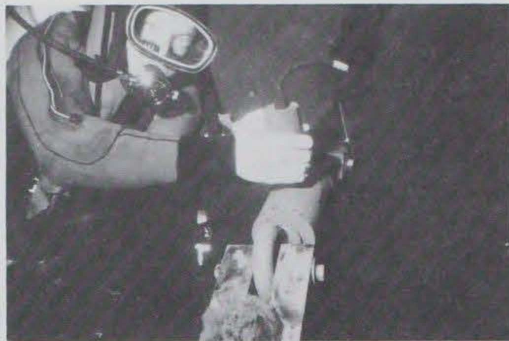
Photo F-20. A diver installing a new electrical lead to an anchor force load cell.
