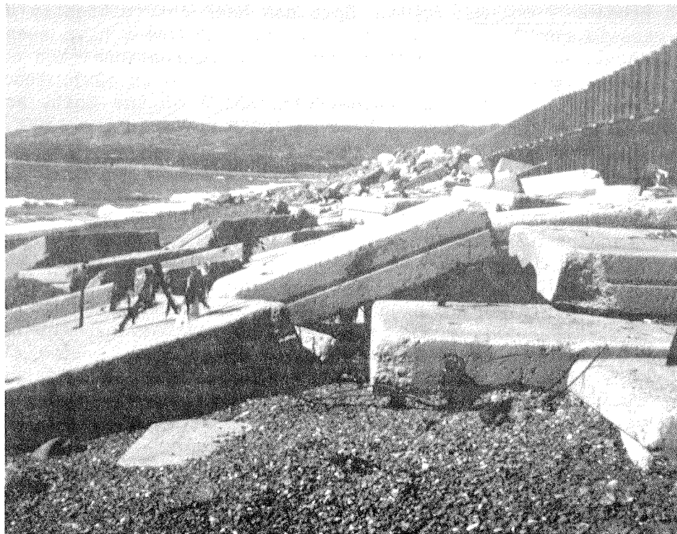
Figure 5 - August 1984 photo of sheet-pile wall, failed concrete slab toe protection, and rock revetment beyond
