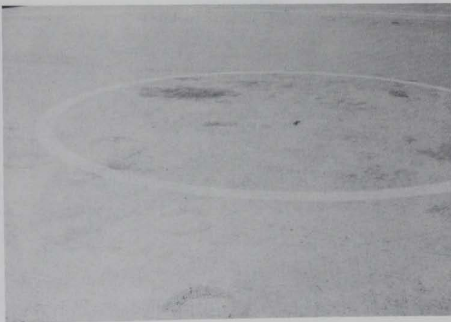
Photo 22. Typical condition of Salviacim pavement
