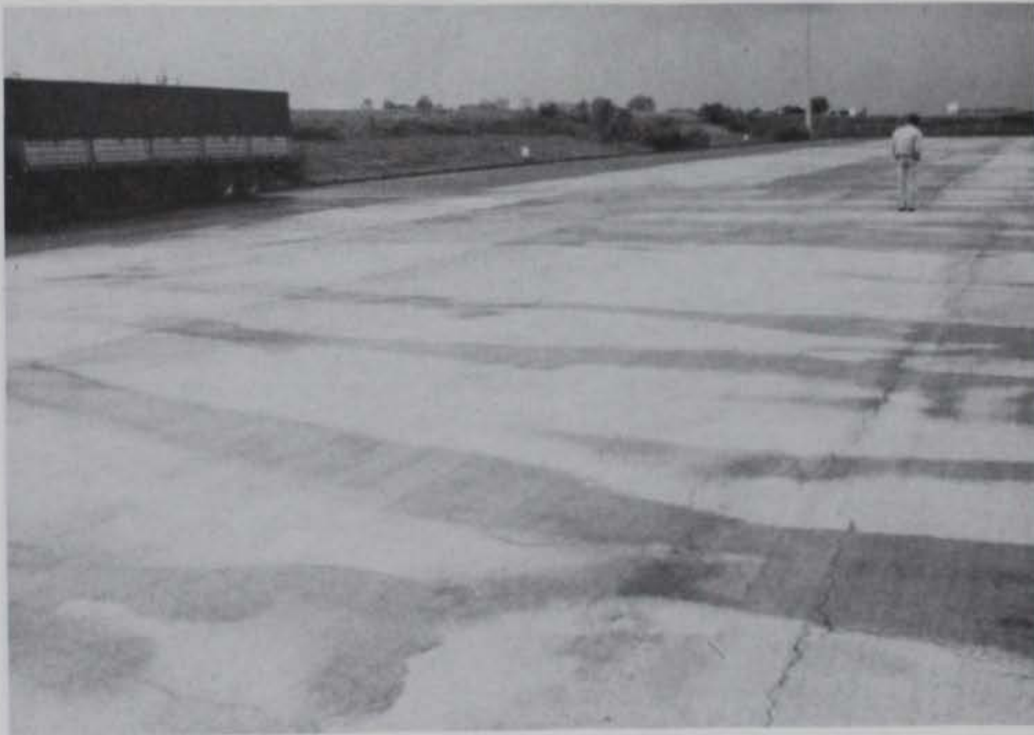
Photo 2. Typical crack pattern
