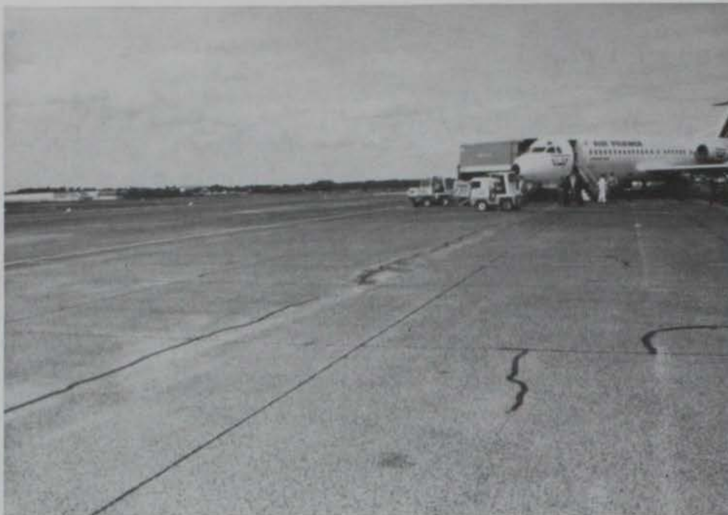
Photo 7. Minor random cracking in 1979 Salviacim pavement
