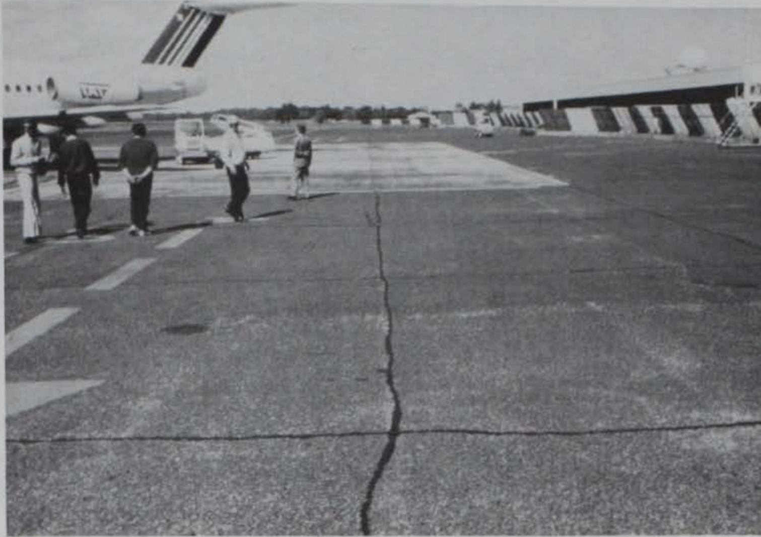
Photo 5. Reflective joints in 1976 Salviacim pavement
