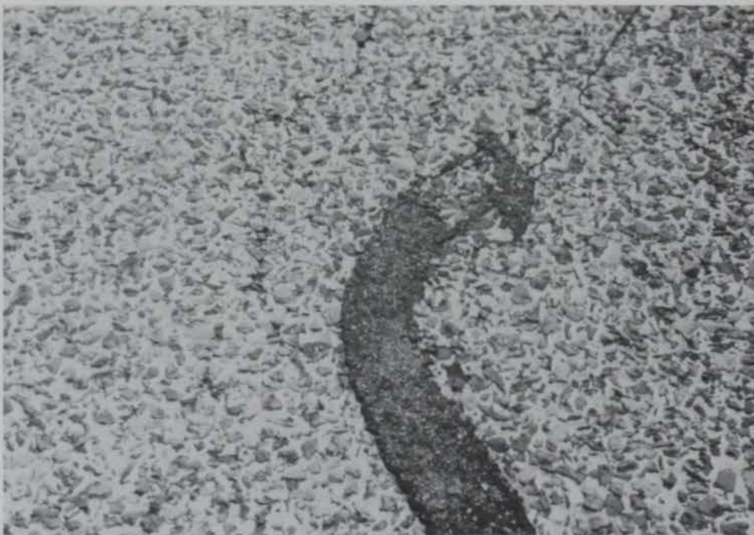
Photo 8. Typical bandaid seal of small crack
