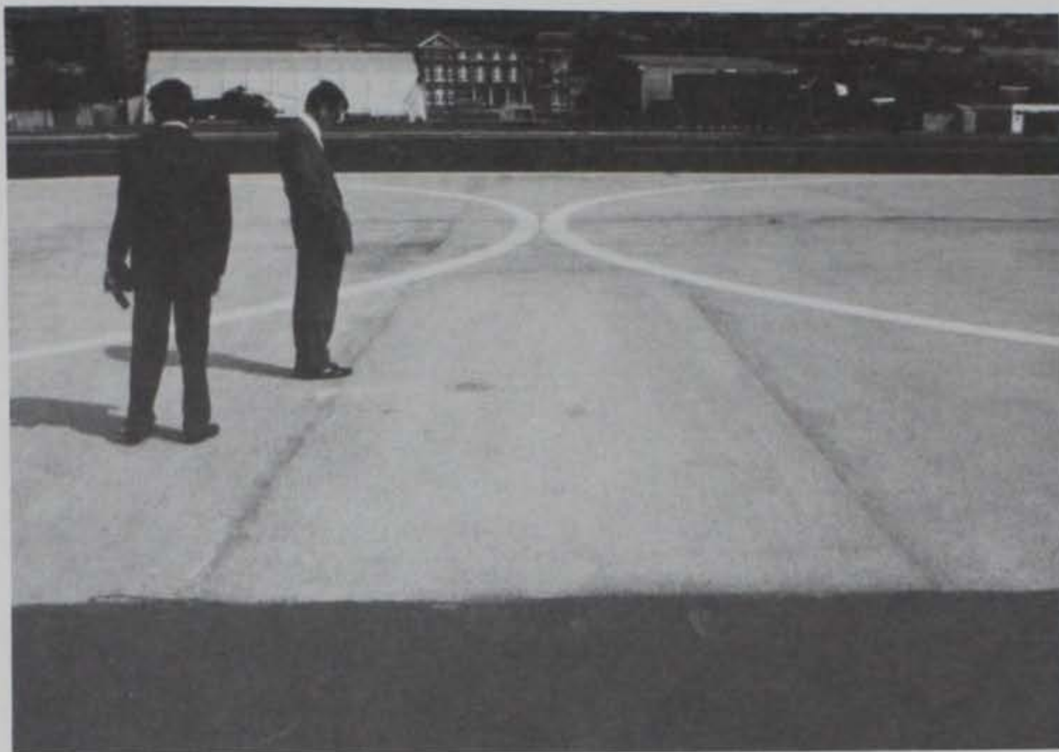
Photo 25. Patched area of Salviacim pavement
