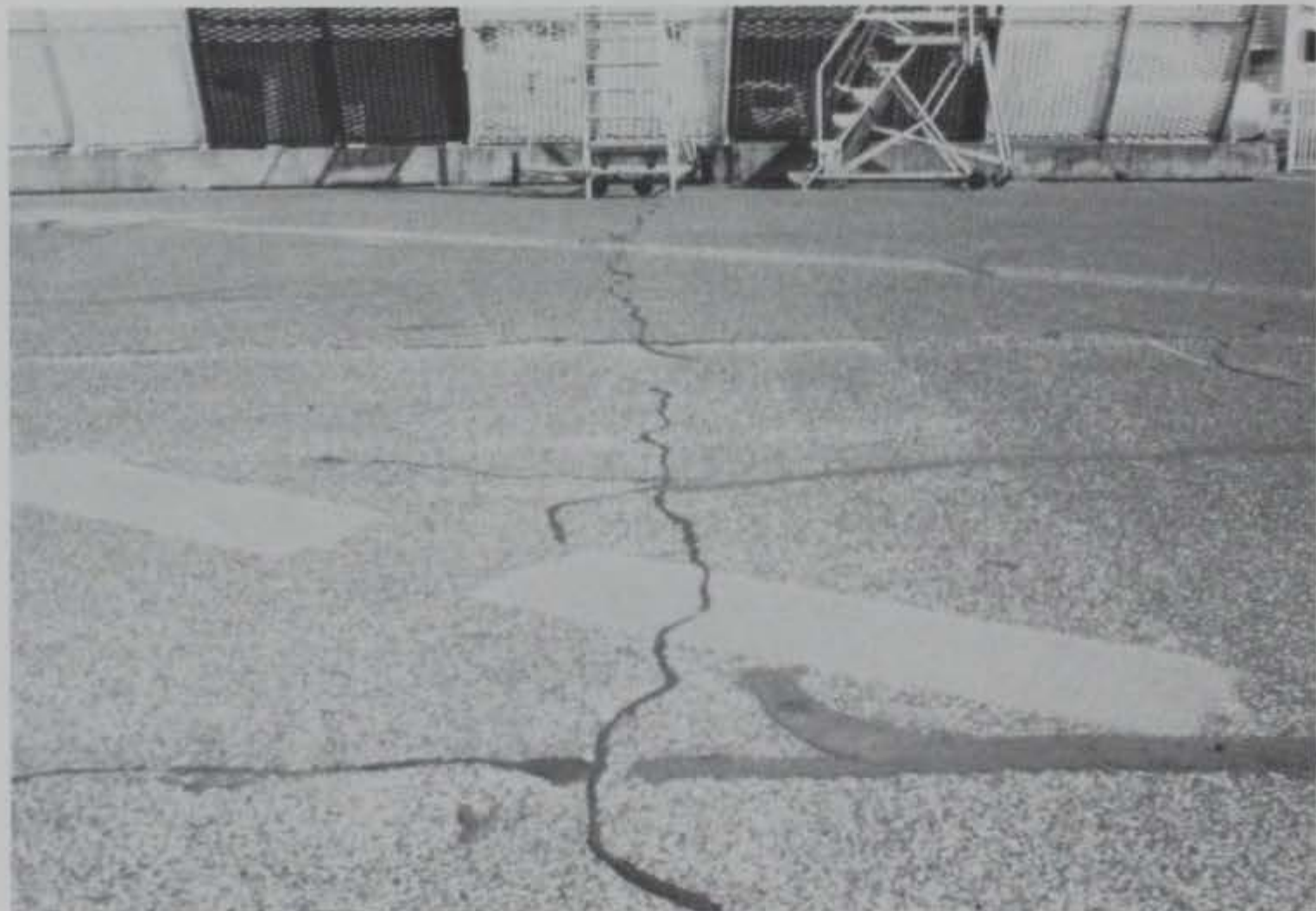
Photo 4. Random reflective cracks in 1976 Salviacim pavement
