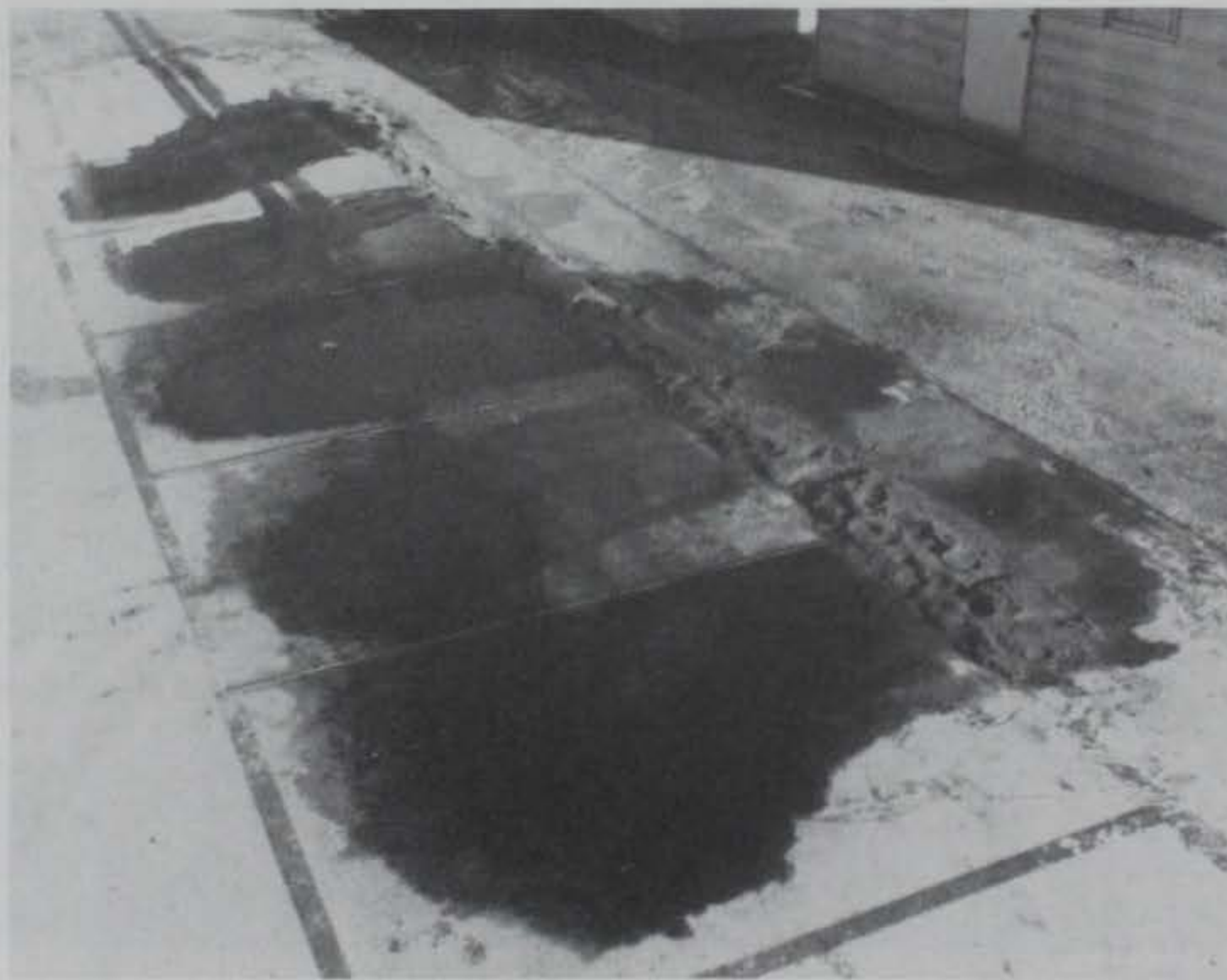
Figure 22. Fuel and oil spillage areas
