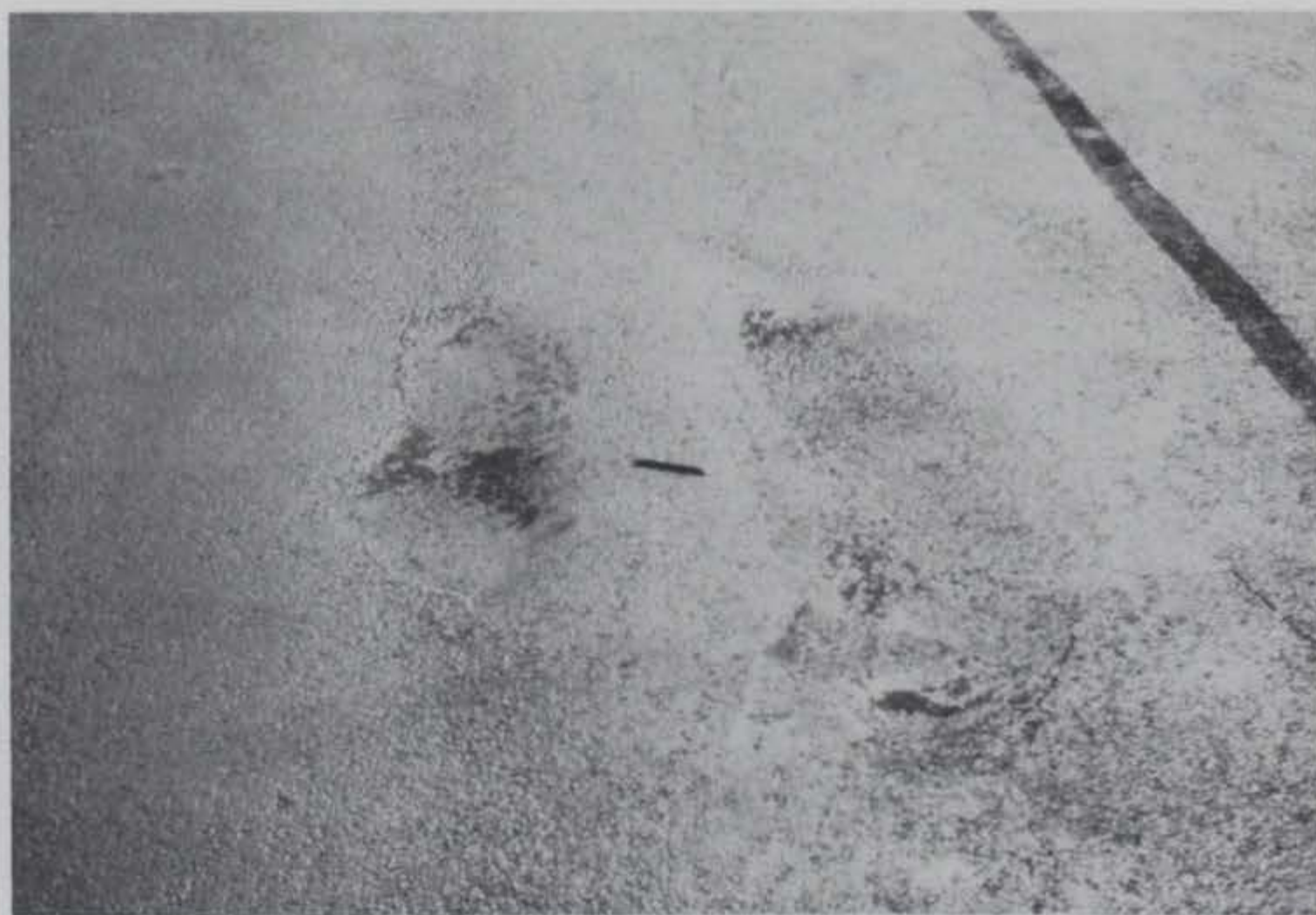
Photo 12. Depression in asphalt concrete caused by fuel spillage and heavy aircraft loads
