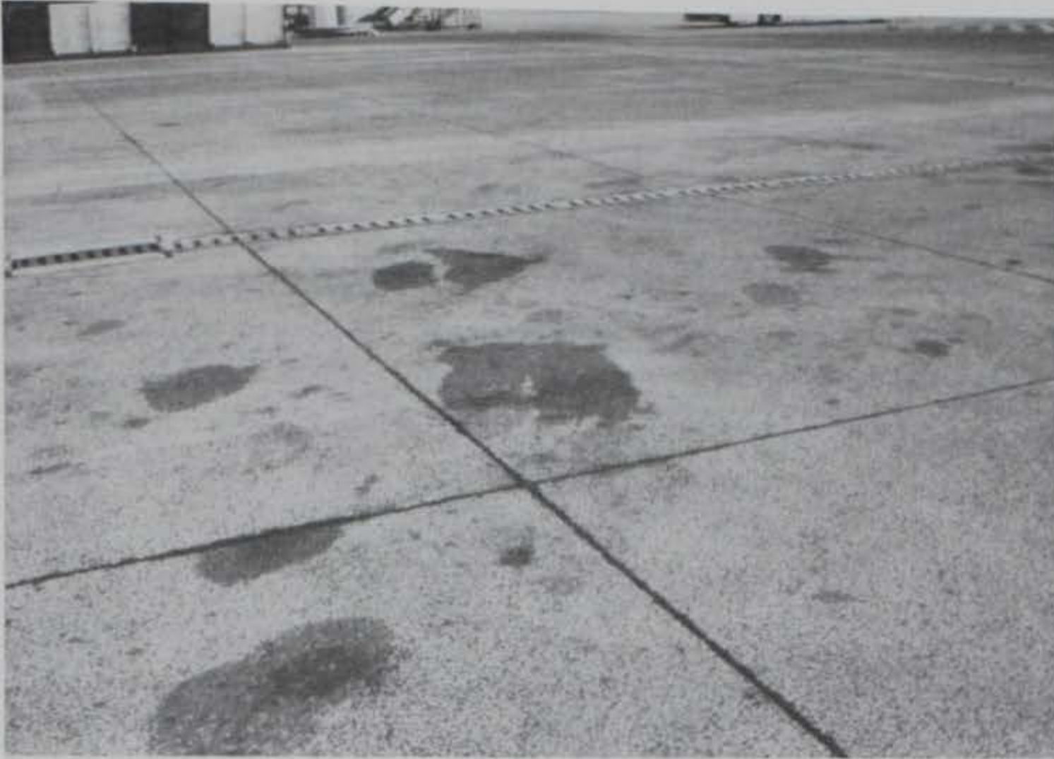
Photo 9. Jet fuel spillage on parking apron
