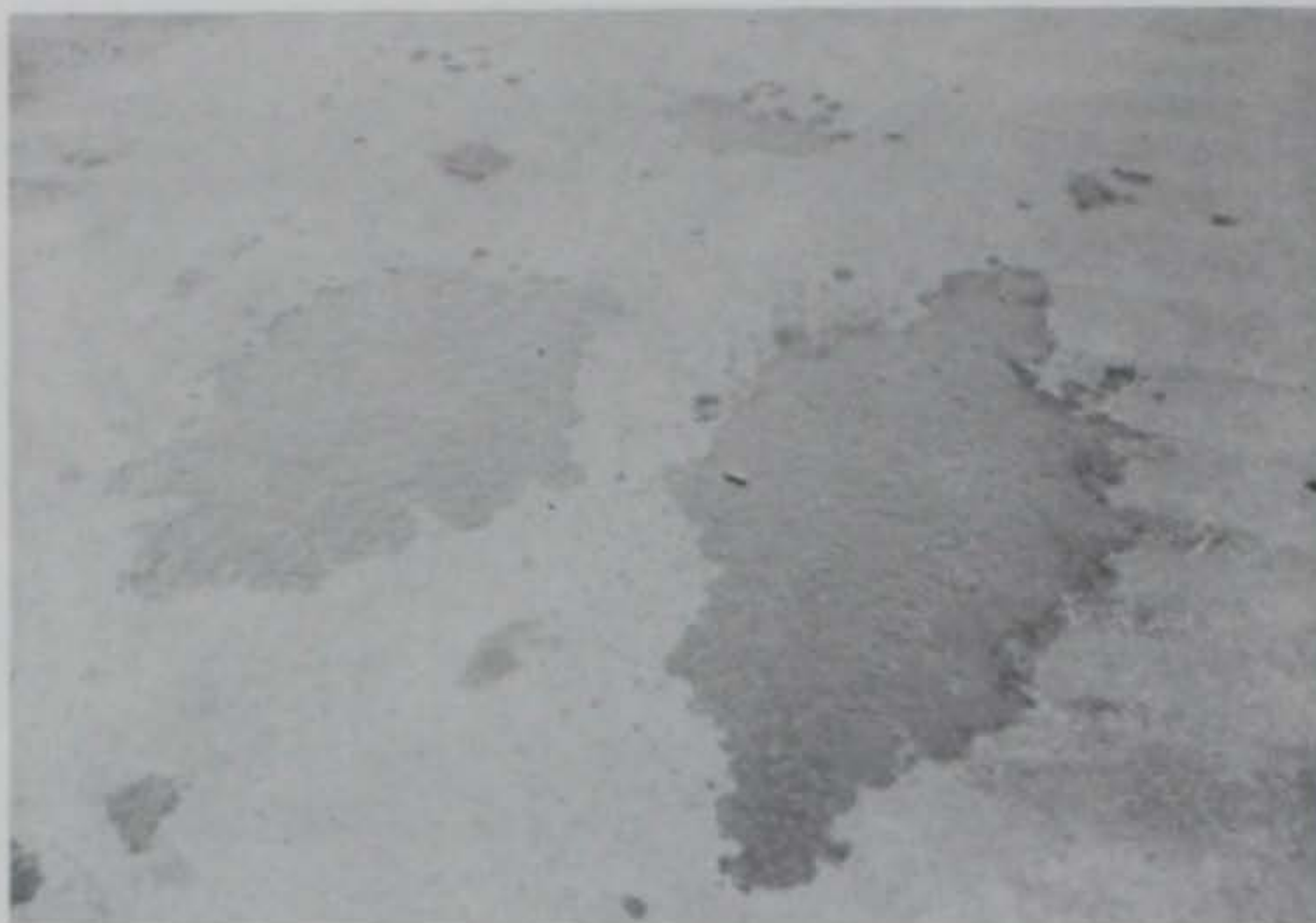
Photo 27. Tank fuel spillage on Salvicim pavement
