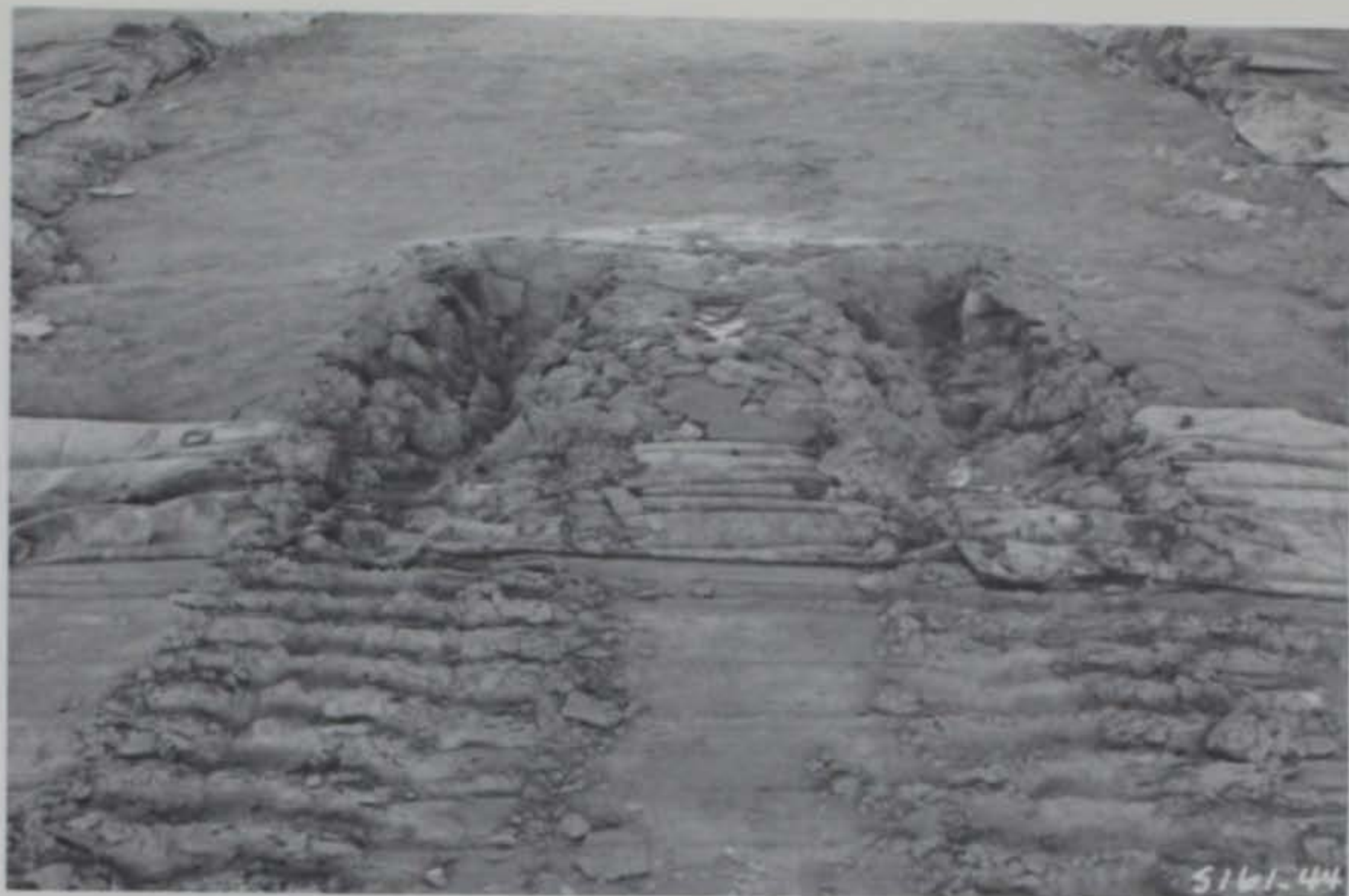
Photo 37. Closeup showing rutting and damaged grid from D-4 tractor
