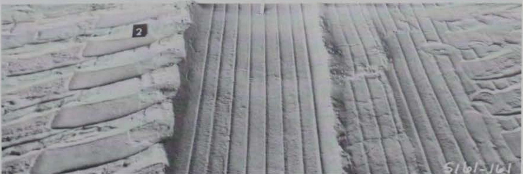
Photo 90. Two- and one-half-inch rut in Test Section No. 5, item 2, under C-130 traffic
