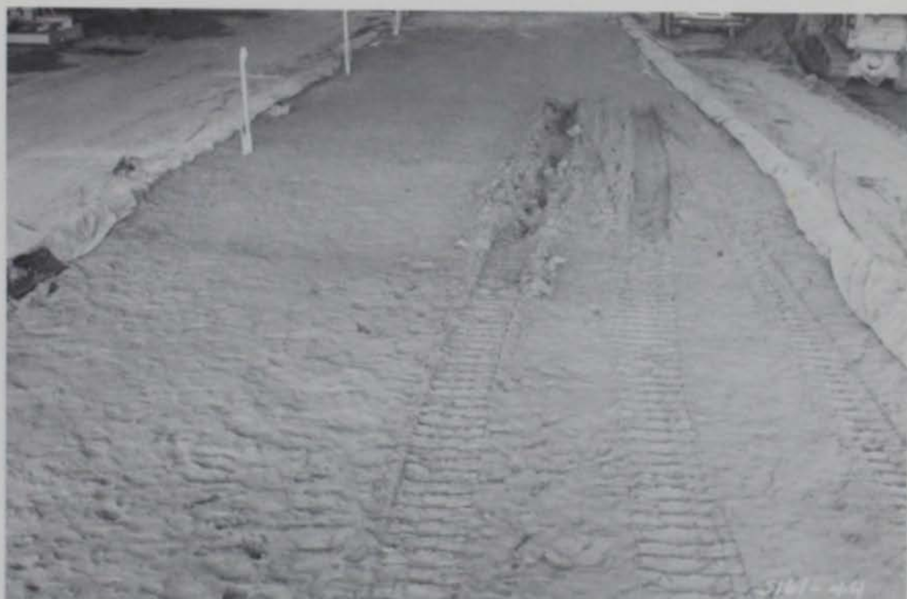
Photo 38. Two passes of D-4 tractor, Test Section No. 3, items 1 and 2, water level 23 in. below surface
