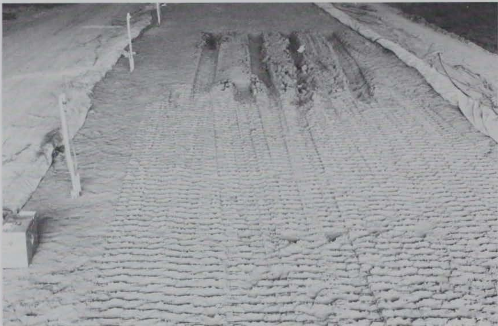
Photo 39. Two coverages of D-4 over item 1 (foreground) and two passes of D4 over item 2 (background), Test Section No. 3
