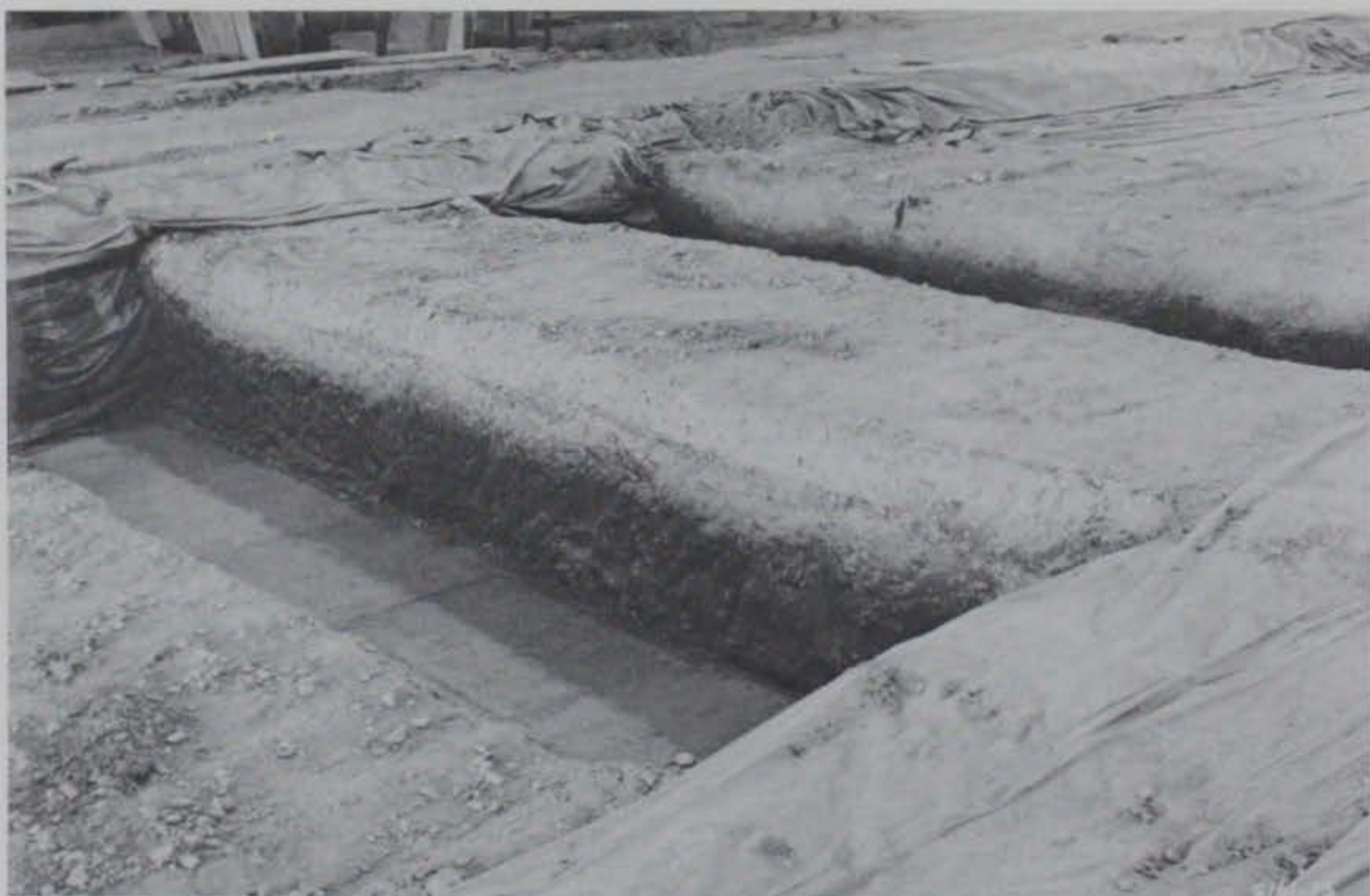
Photo 24. Eight-foot-wide trenches excavated in Test Section No. 3, item 4, to be backfilled with loose sand
