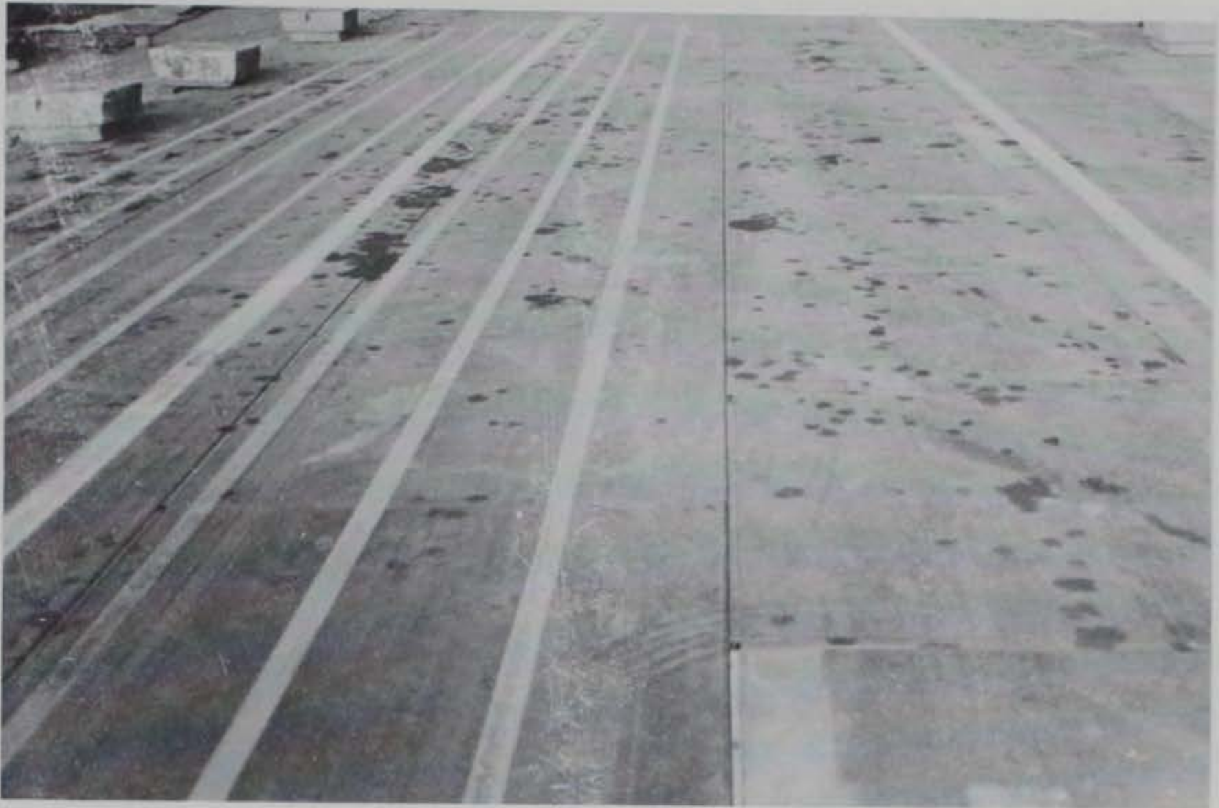
Photo 5. General view of XML9 landing mat, Test Section No. 1, item 1, prior to traffic
