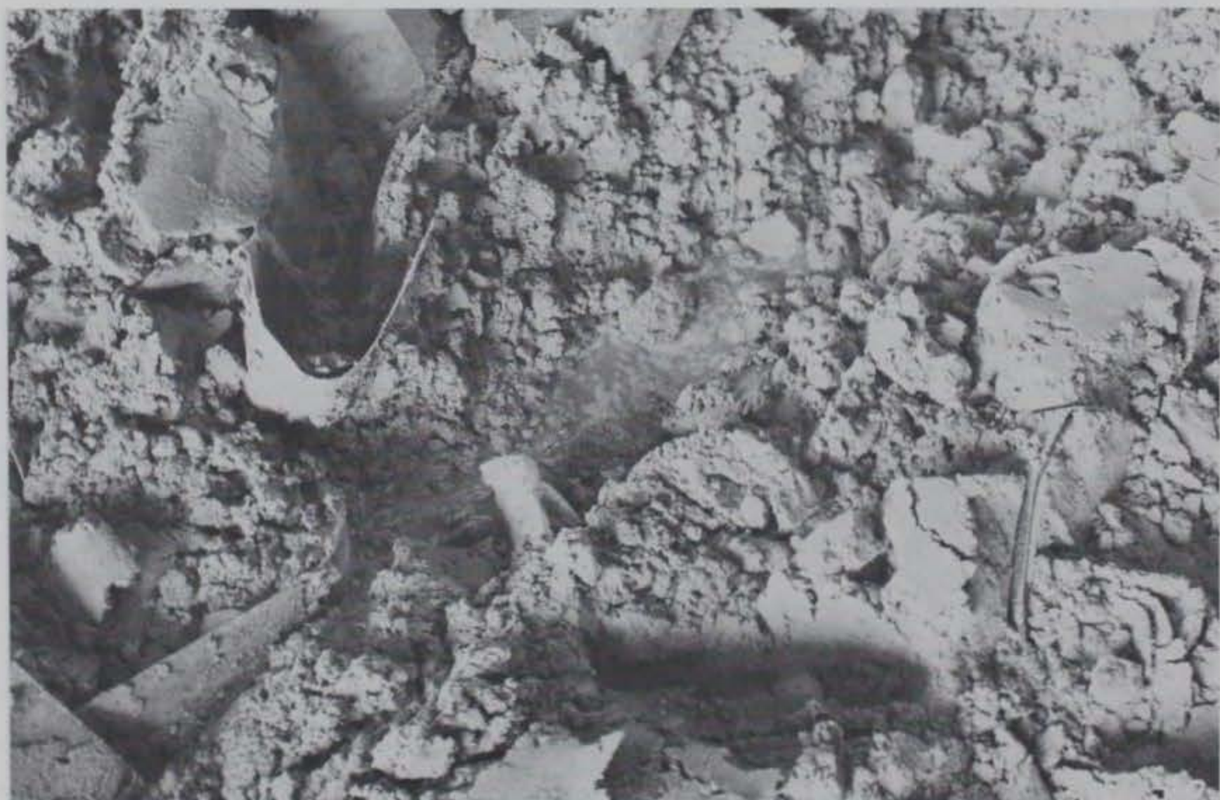
Photo 40. Closeup of damaged grid and water in ruts of Test Section No. 3, item 2
