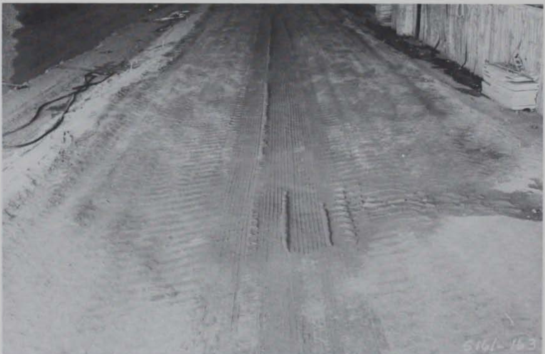
Photo 92. Overall view of Test Section No. 5 after wetting and C-130 traffic
