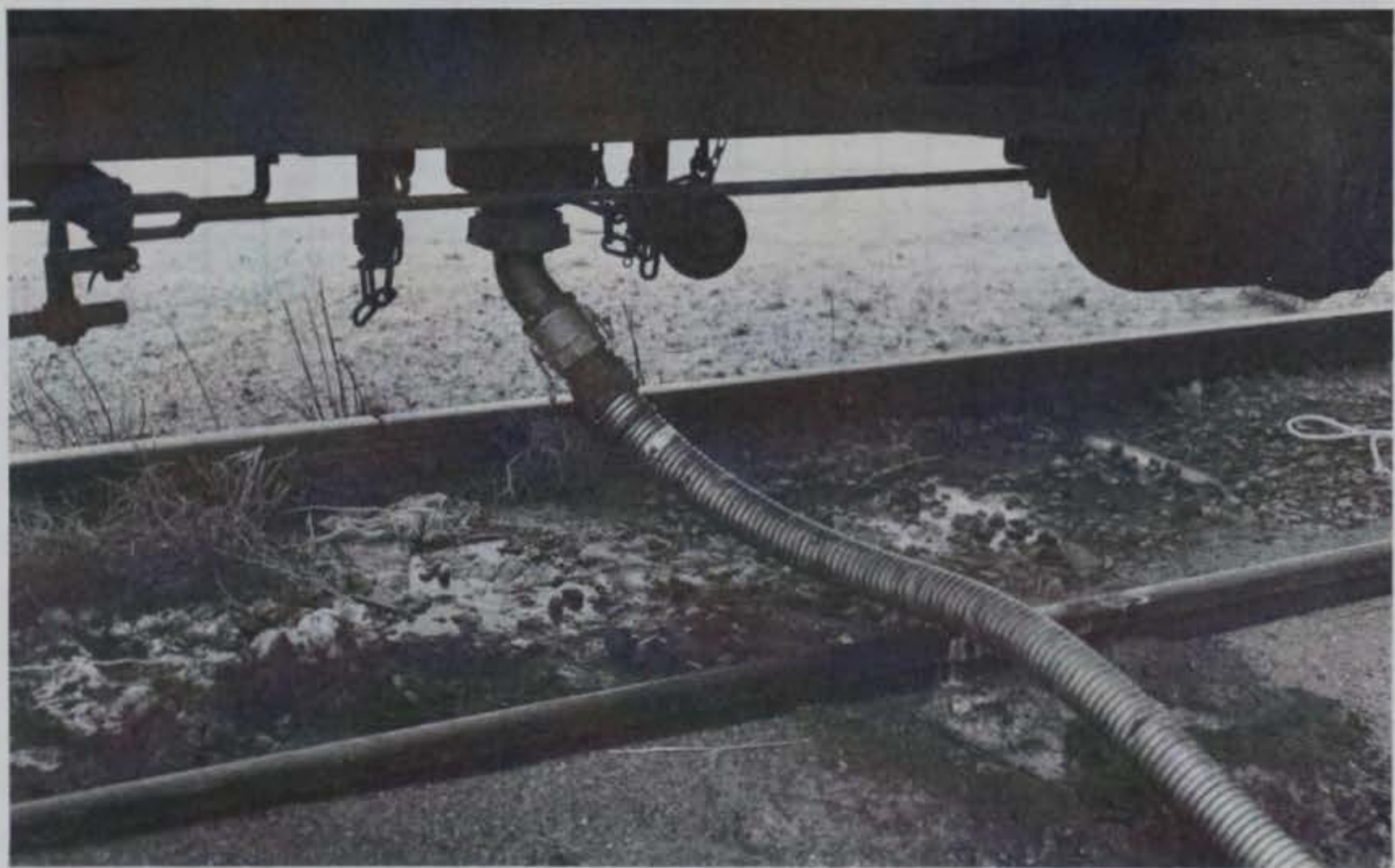
Figure 10. Collar device required for tank access
