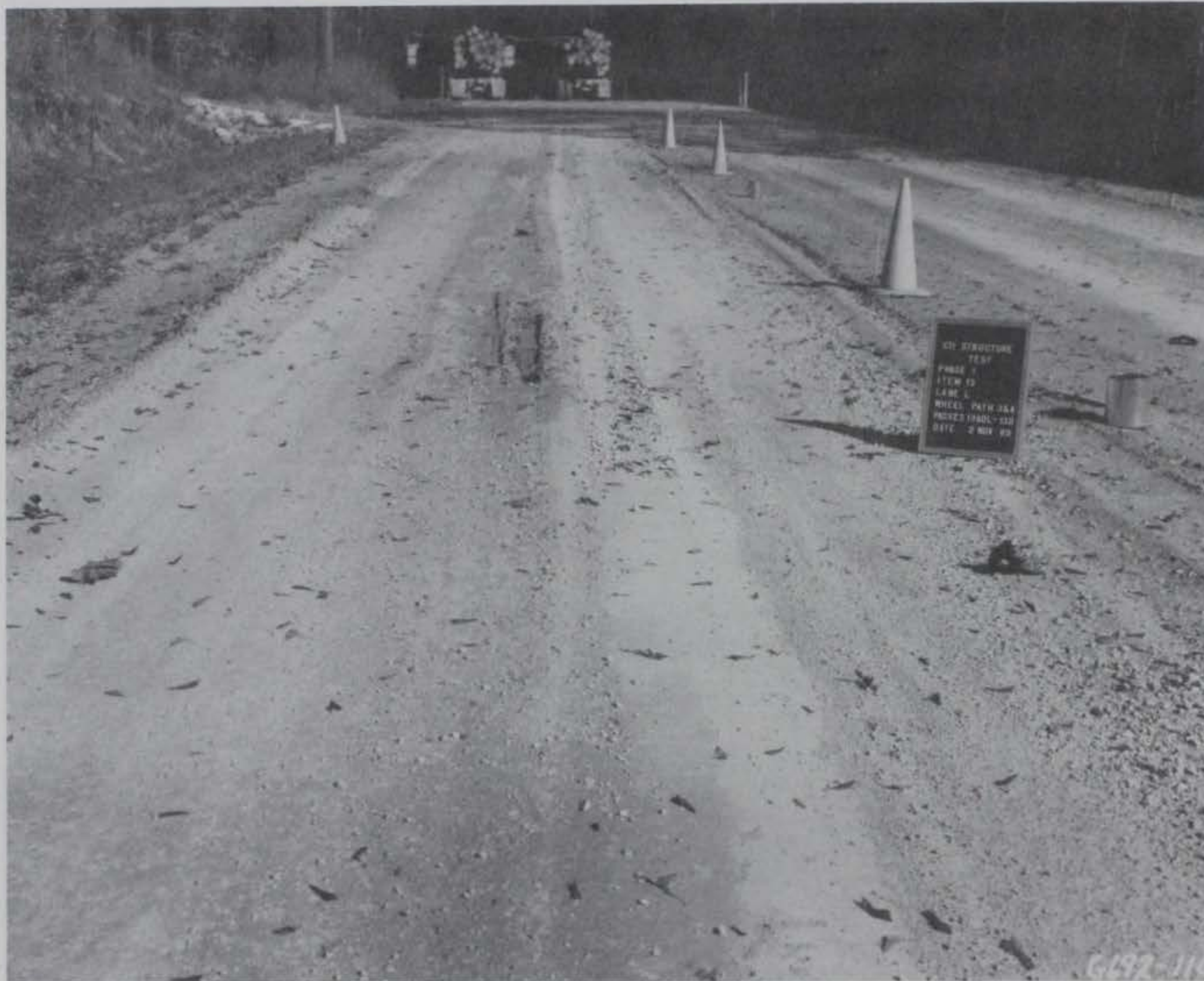
Photo 56. Item 13, low-pressure tire lane, general view after 130 passes during the induced failure plan
