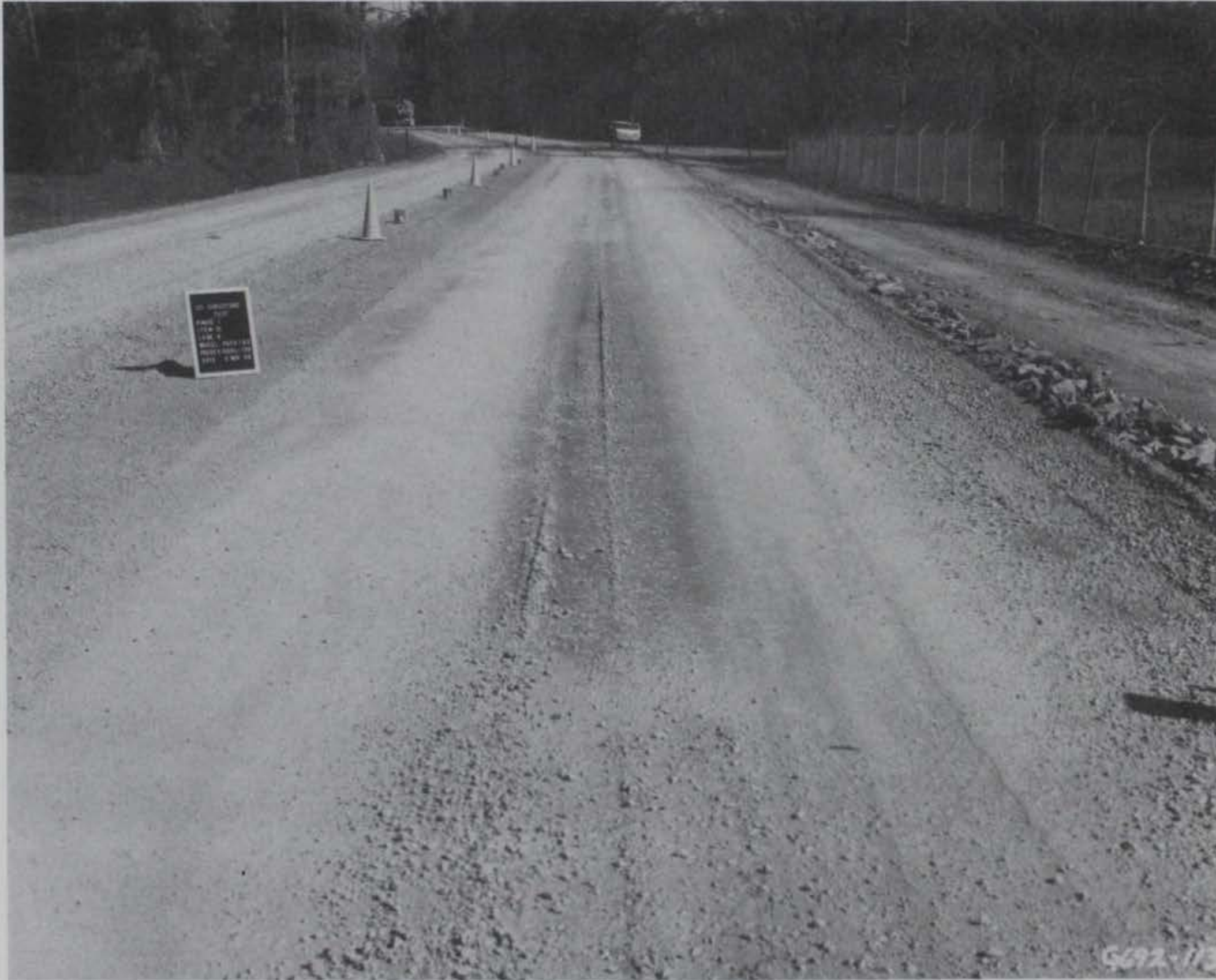
Photo 61. Item 15, high-pressure tire lane, general view after 139 passes during the induced failure plan
