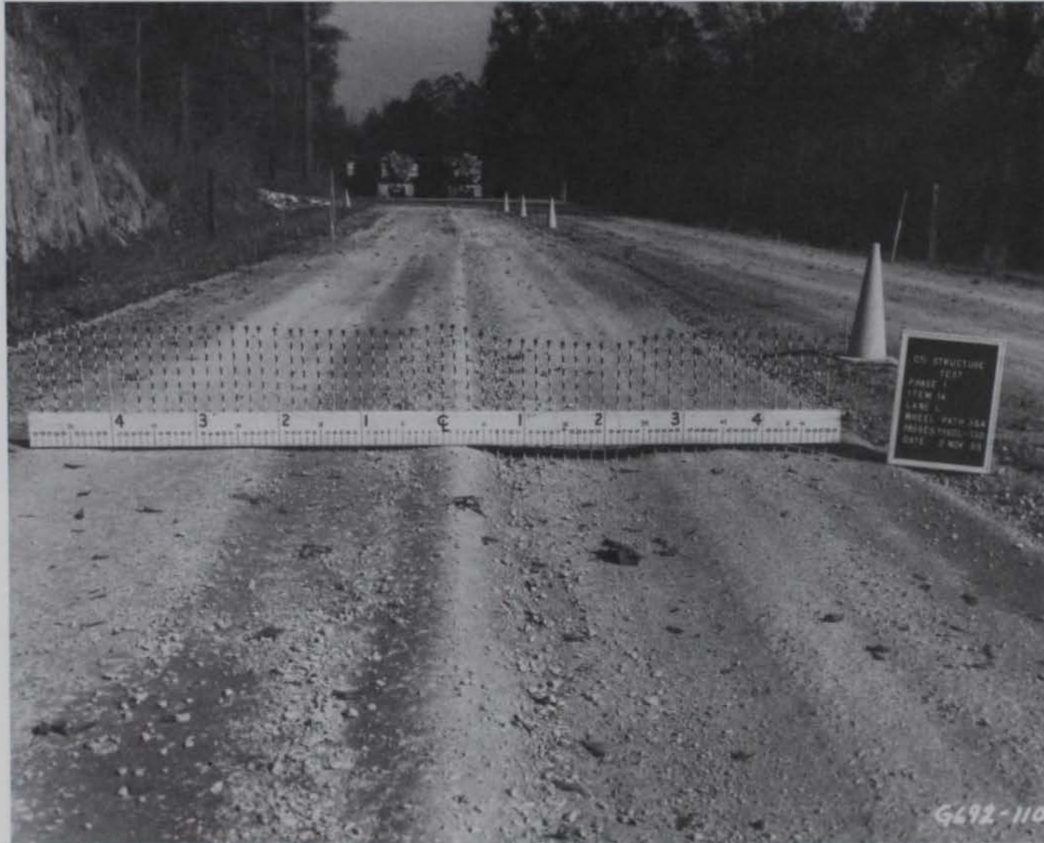
Photo 55. Item 14, low-pressure tire lane, high-severity rutting after 130 passes during induced failure plan
