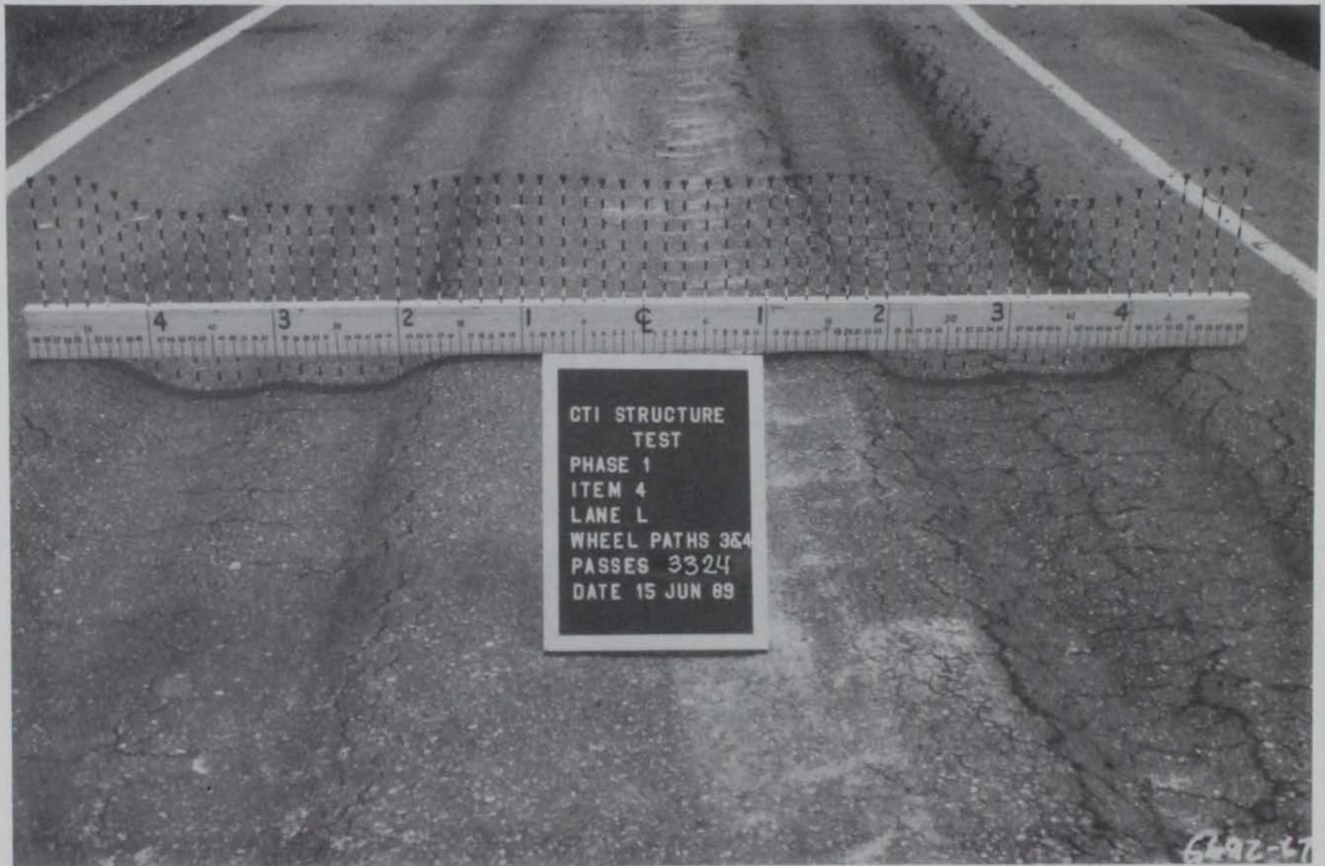
Photo 23. Item 4, low-tire pressure lane, general view of failure after 3,324 passes
