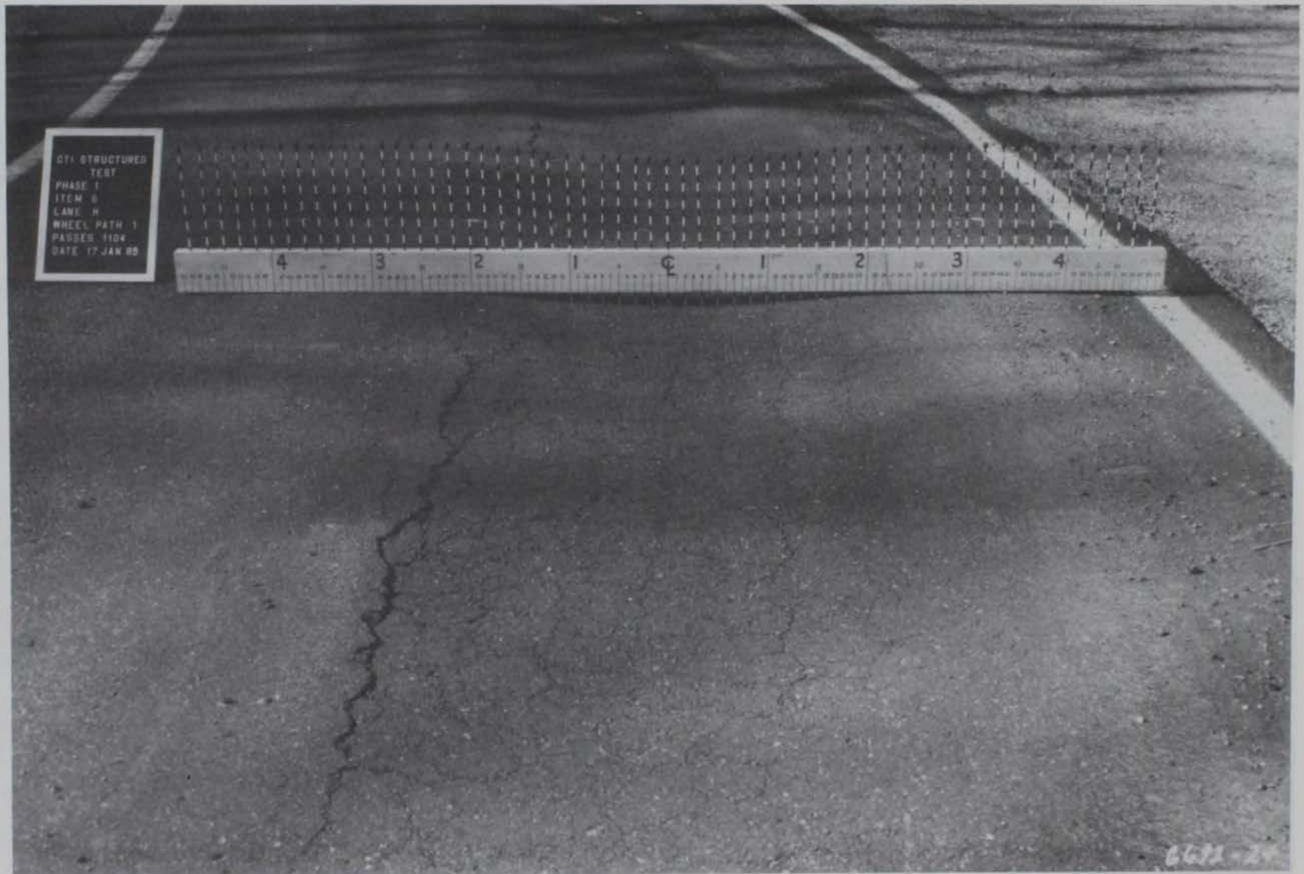
Photo 19. Item 6, high-tire pressure lane general view of failed area after 1,104 passes
