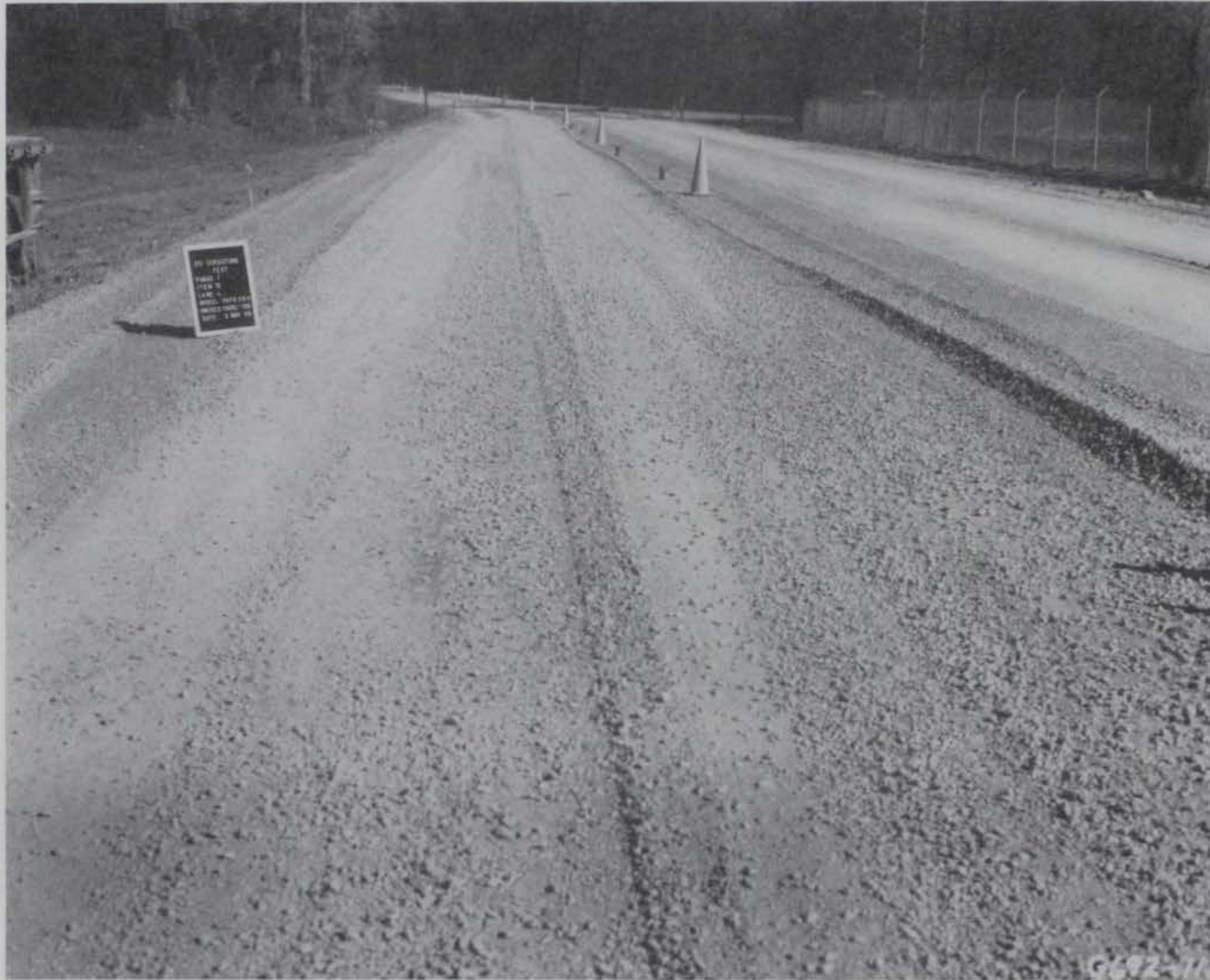
Photo 58. Item 15, low-pressure tire lane, general view after 130 passes during the failure induced plan
