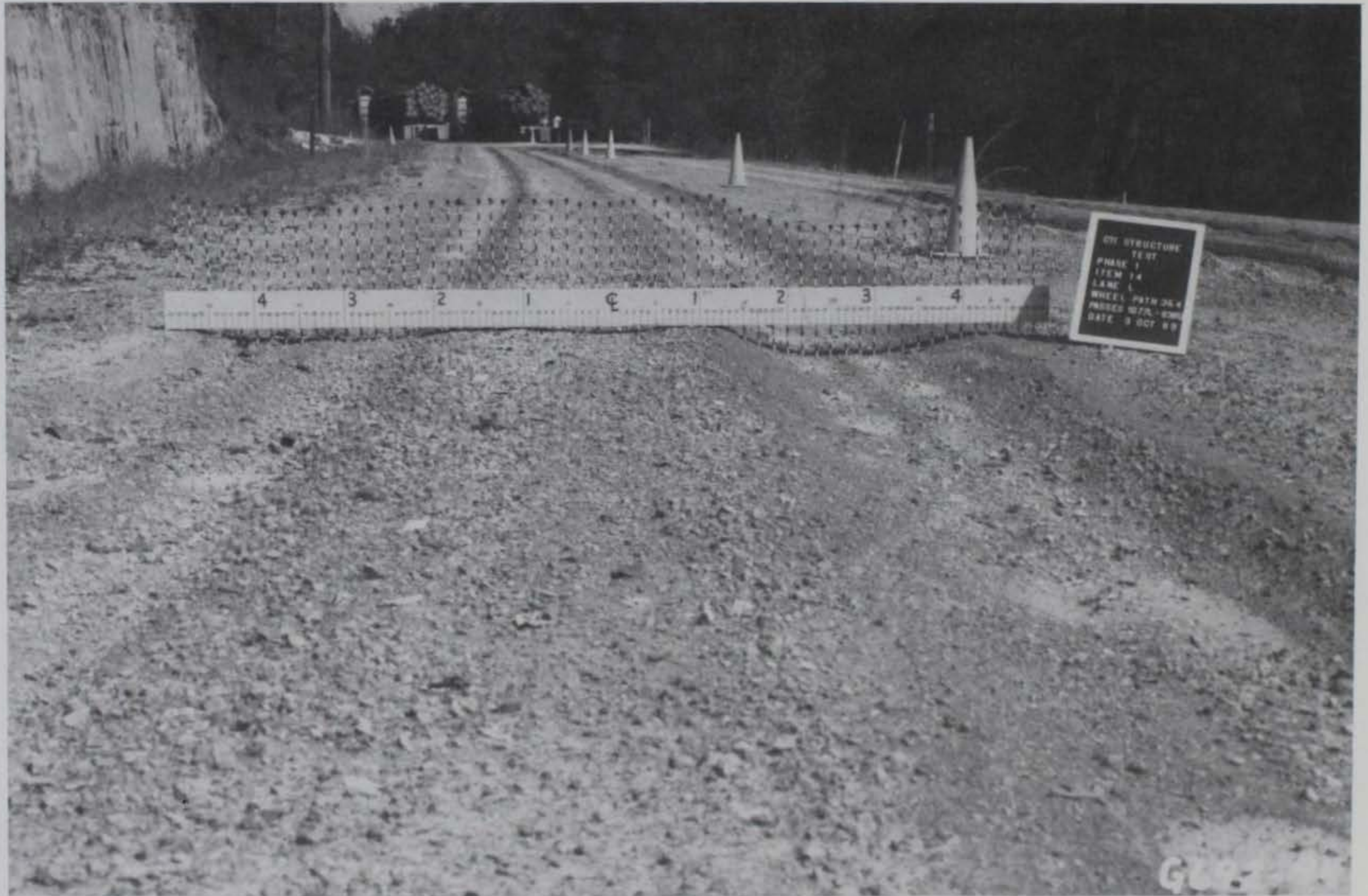
Photo 53. Item 14, low-pressure tire lane, high-severity rutting after 90 passes over a wet subgrade
