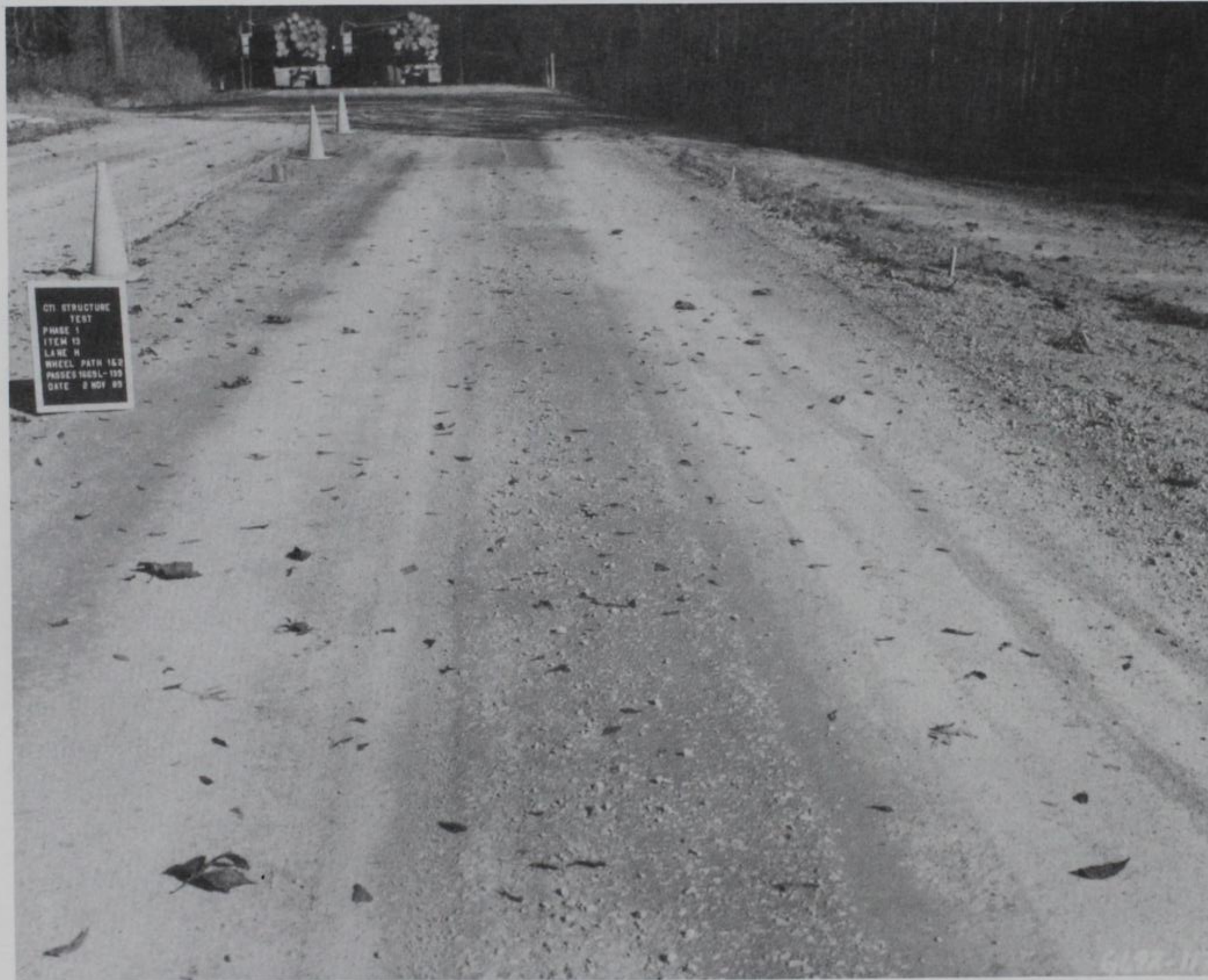
Photo 59. Item 13, high-pressure tire lane, general view after 139 passes during the induced failure plan
