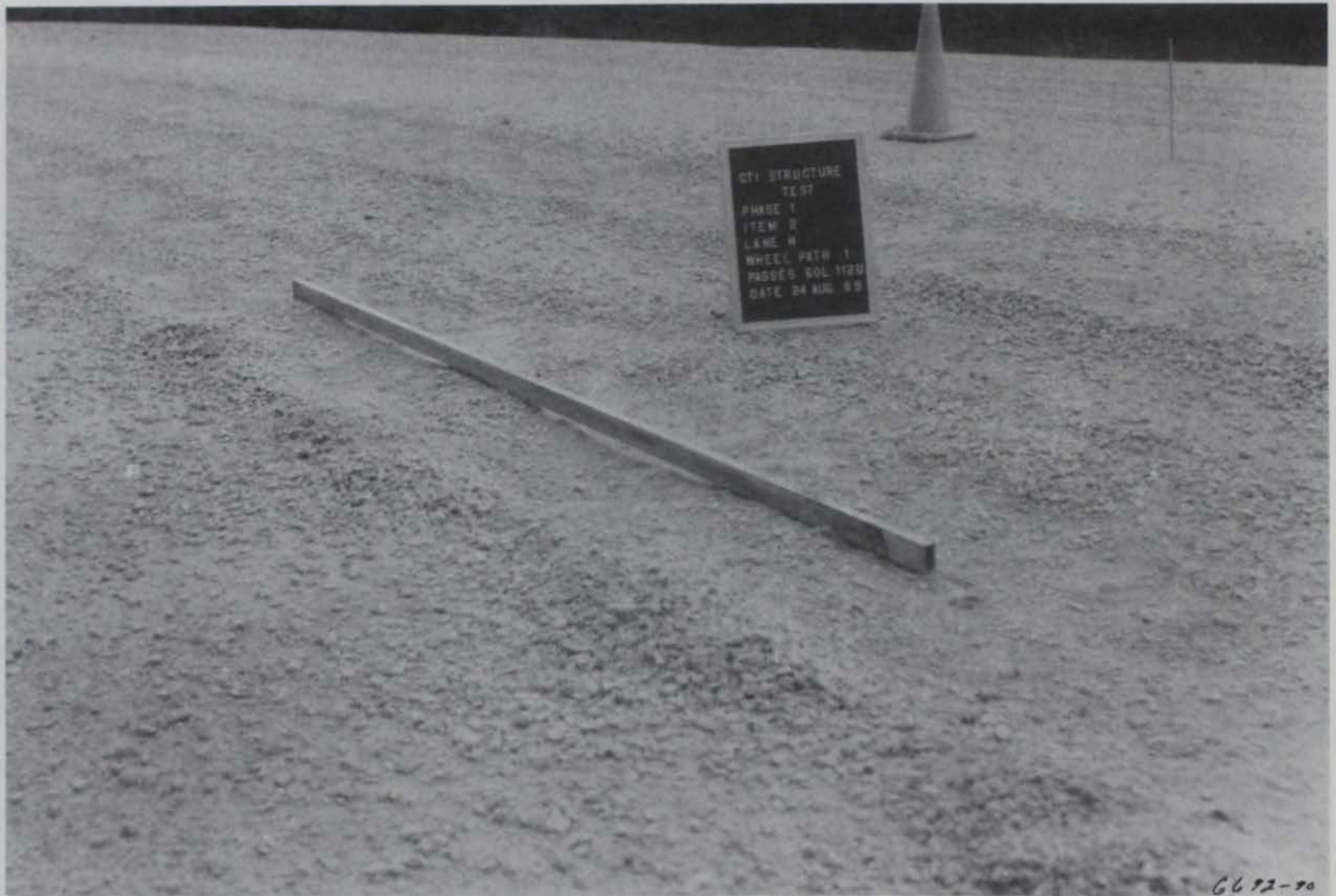
Photo 48. Item 2, high-pressure tire lane, close-up of high-severity washboarding after 112 unloaded passes
