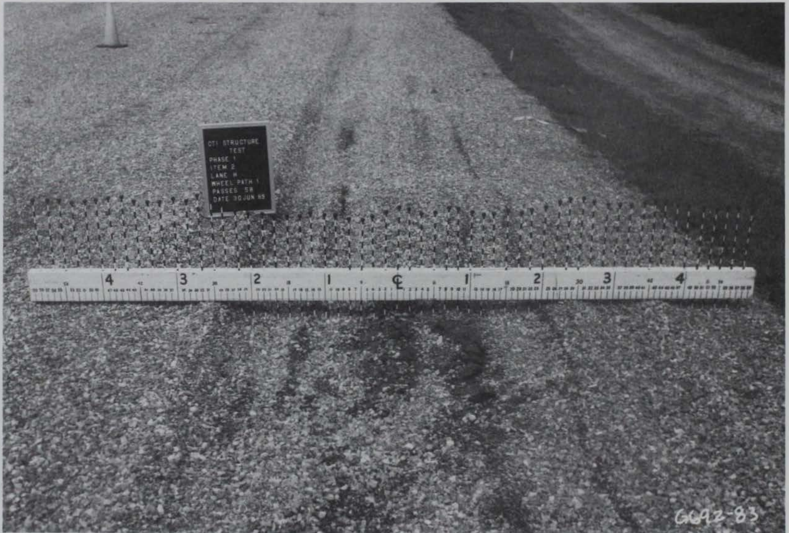
Photo 44. Item 2, high-pressure tire lane, failure after 58 passes
