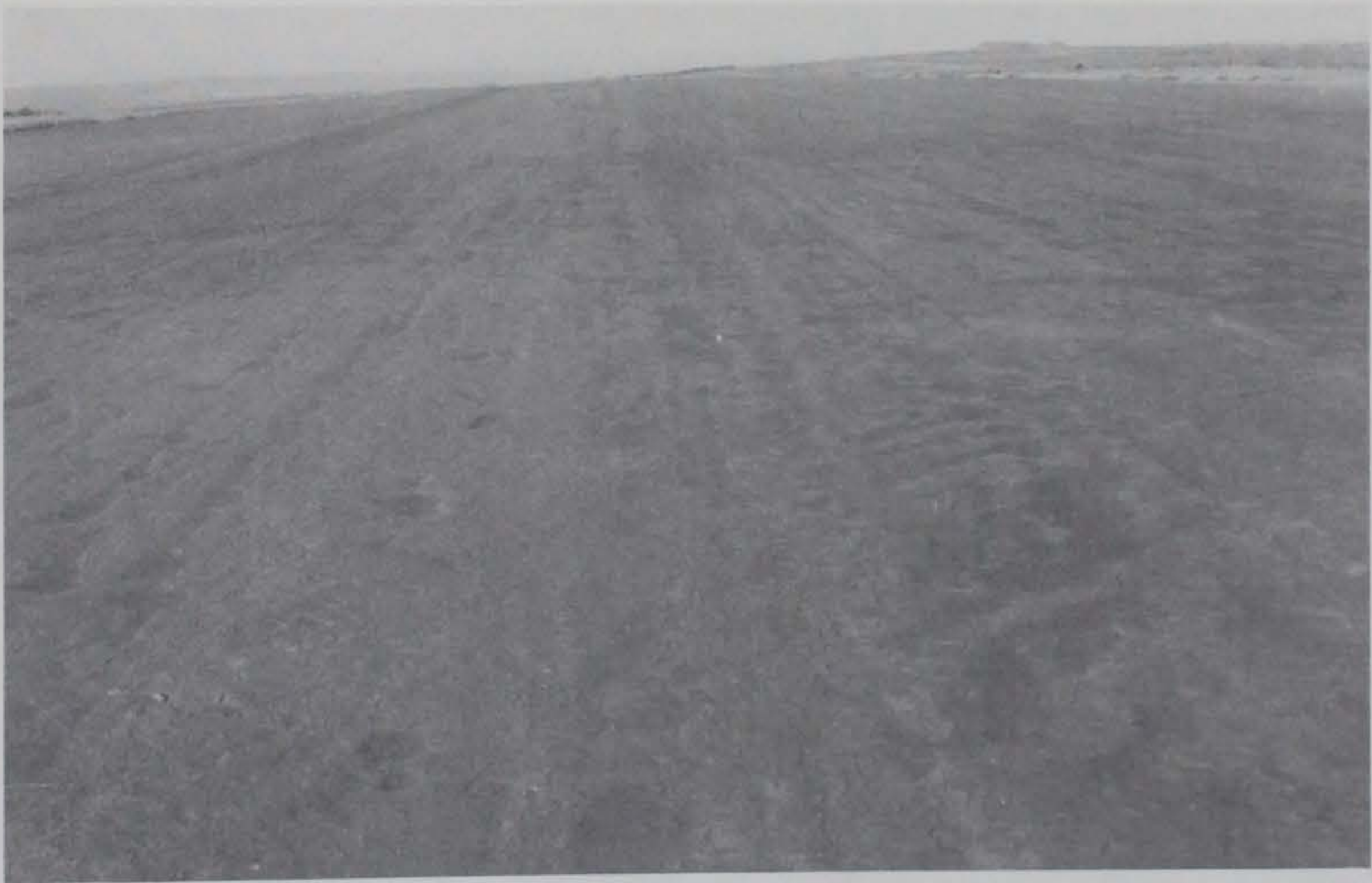
Figure 28. Airstrip surface showing some shrinkage cracks beginning to form
