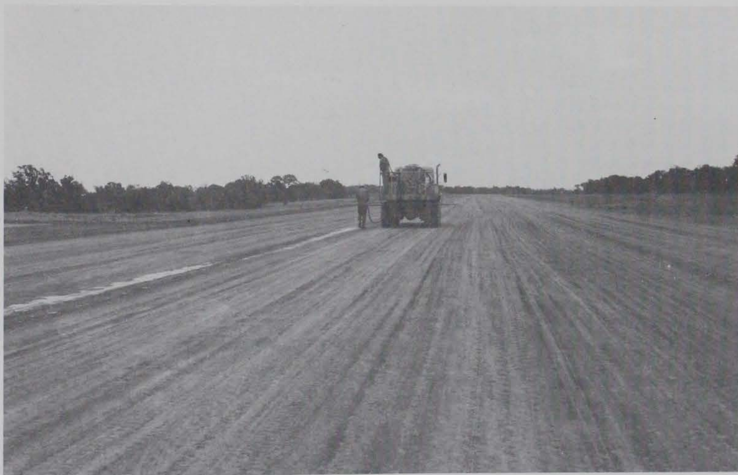
Figure 36. Wetting a damaged area by applying a light coat of water and allowing the treated material to melt back together
