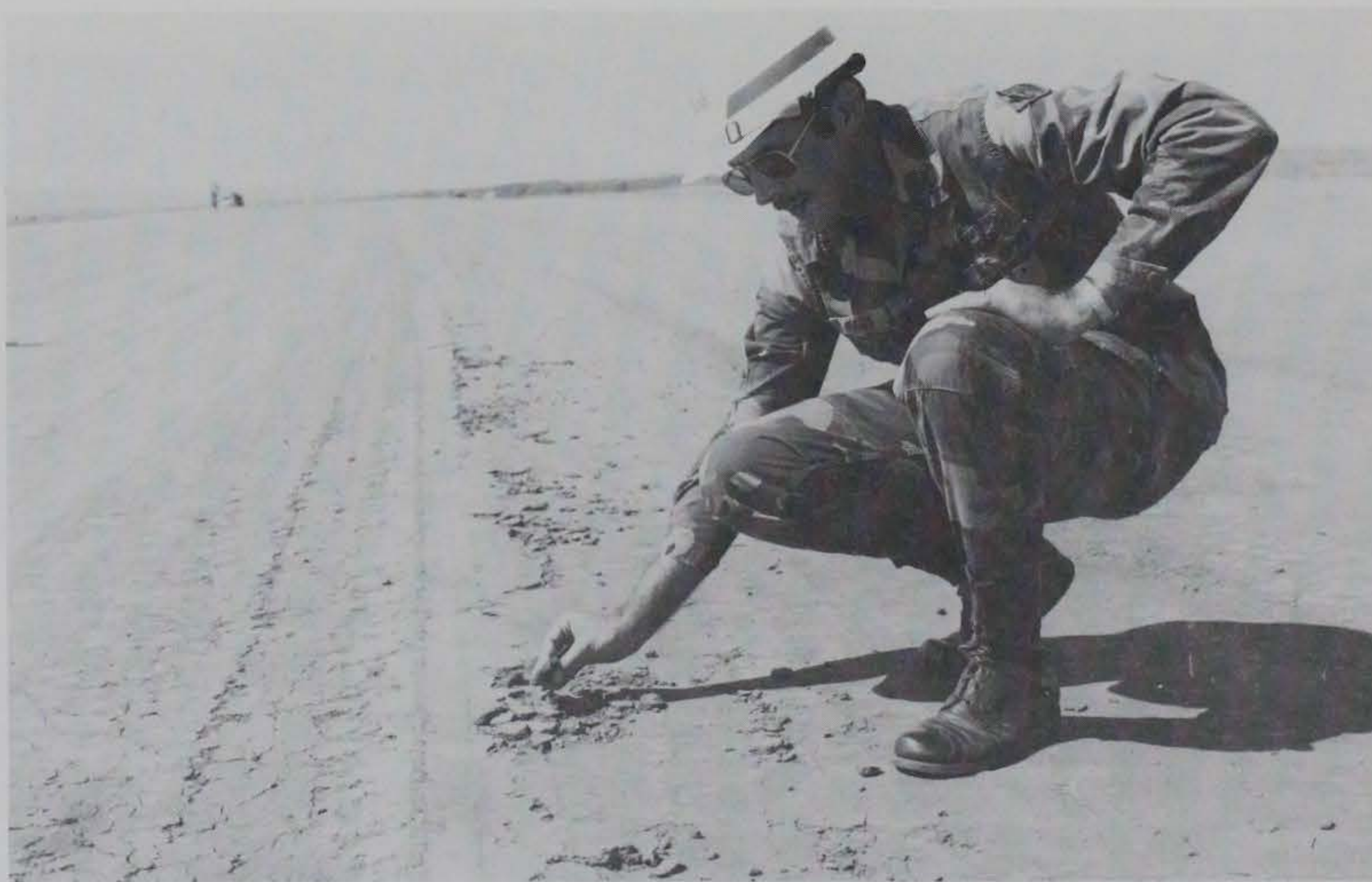
Figure 34. Minor rutting of airstrip surface where a C-130 aircraft bounced during a hot landing
