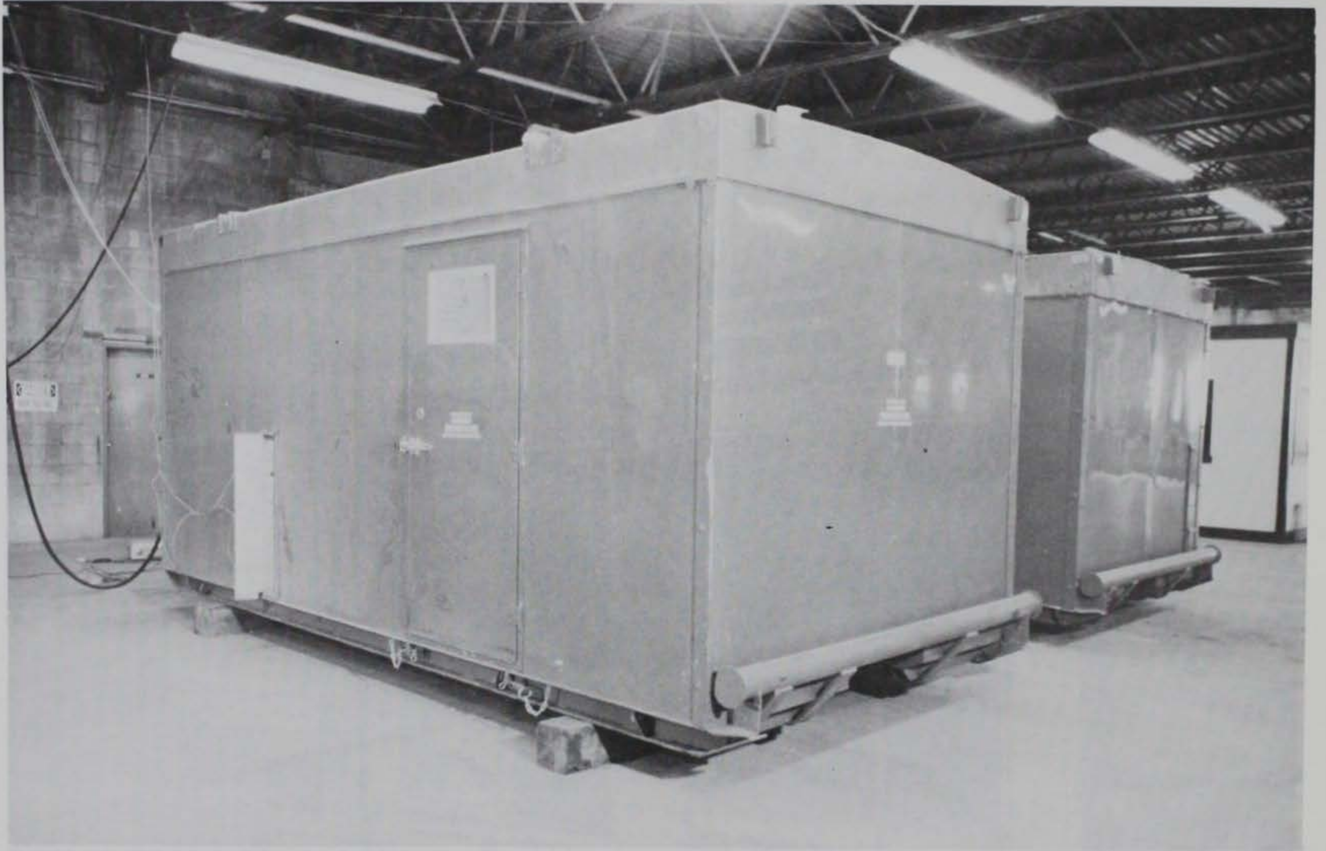
Figure 9. Metal cabs housing MSHA seismic system
