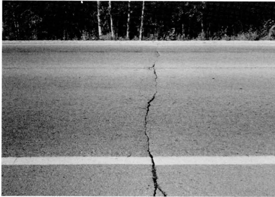
Figure 37. Typical low temperature cracking on Route 115, outside Cadillac, Michigan.
