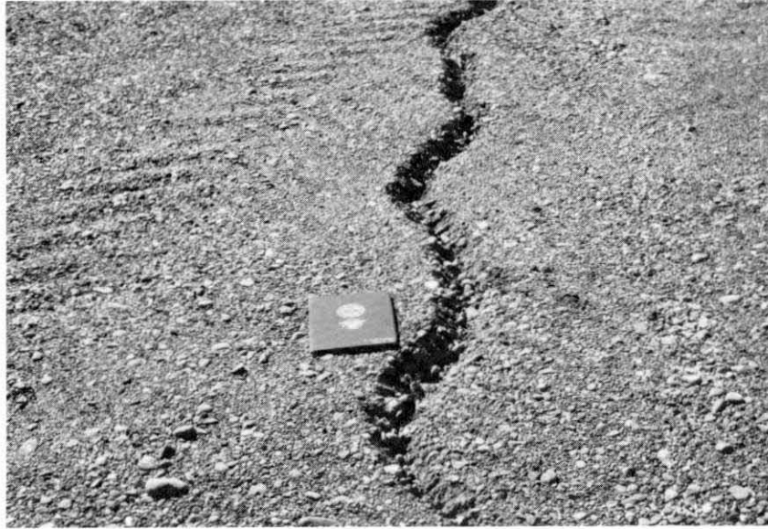
Figure 23. Severe earth-related cracking in granular fill at Deadhorse (Carpenter and VanDam 1985).
