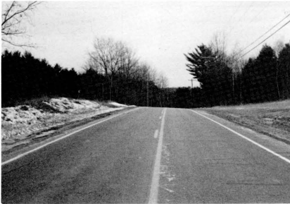
Figure 41. Low temperature cracks on Route 5N outside Norwich, Vermont.
