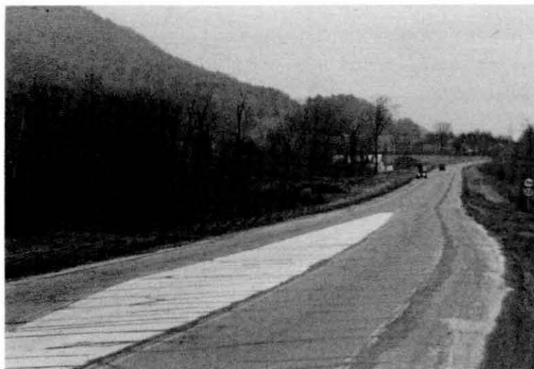
Figure 30. Typical low temperature cracking on Route 9N, New York.
