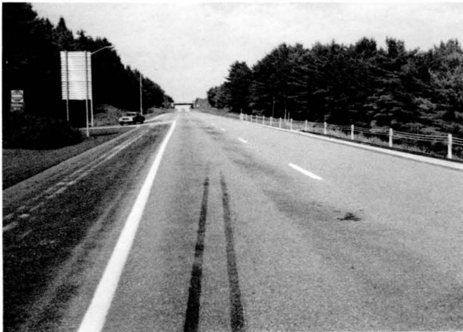
Figure 42. Rutting on Interstate 91 near Fairlee, Vermont.
