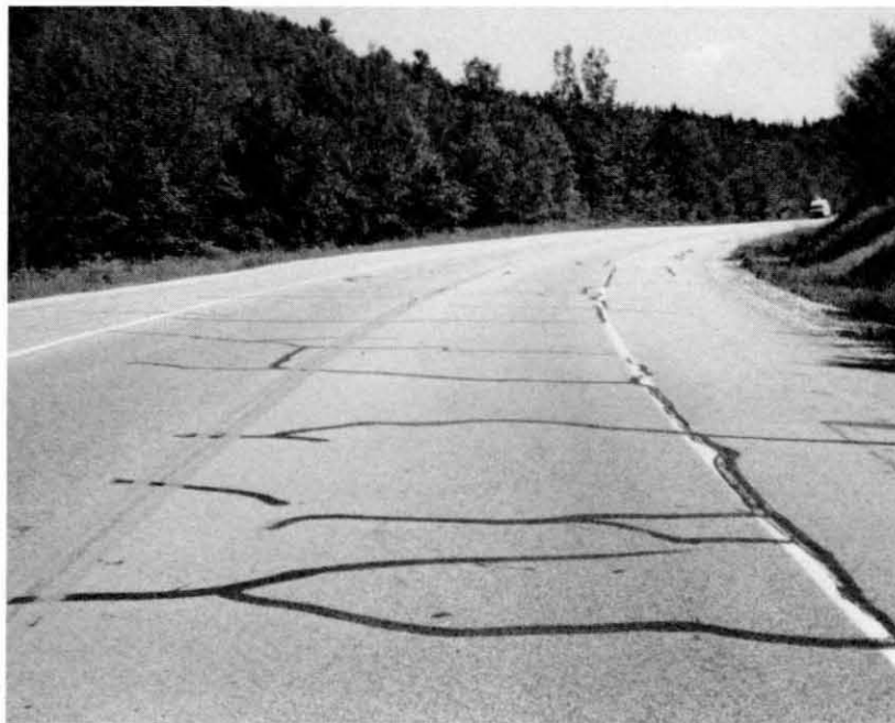
Figure 40. Low temperature cracks on Route 302 outside Montpelier, Vermont.
