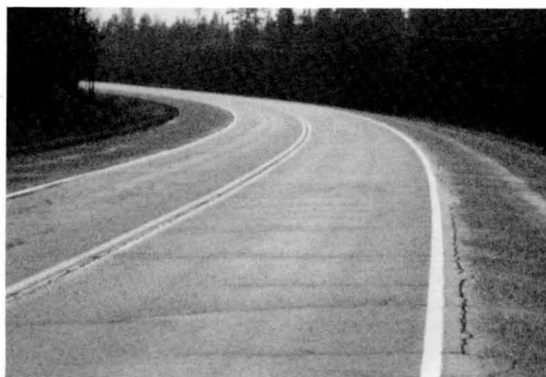
Figure 31. Typical low temperature cracking on Route 3, New York.
