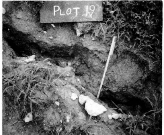
Figure 15. Closeup of damage showing extent of erosion.
