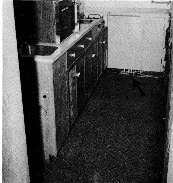
Figure 4.4.3. Water system drain valves. (Other drain valves are in the water compartment and adjacent to the wastewater holding tank.)
