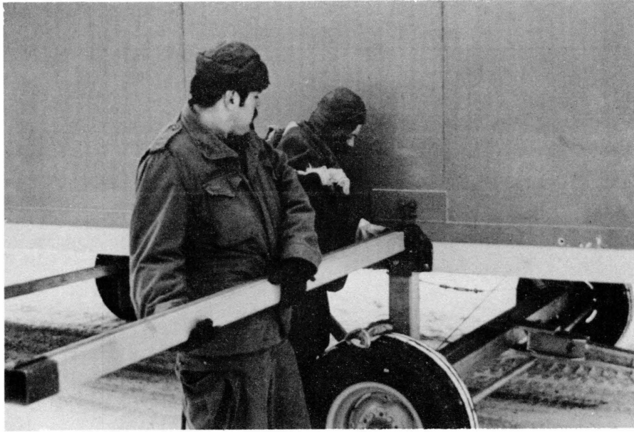
Figure 3.4.2. Installing the deployment beams. One person should hold up the free end while the other tightens bolts with an expansion wrench.
