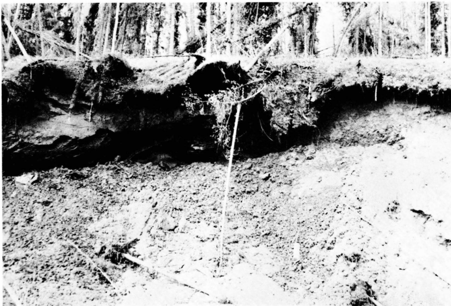
Plate 24. Ice cut at south abutment of Yukon Bridge. Large ice lenses in silt exposed by road cut. Trees left in place on vegetative mat are tearing the mat as they are undercut by thaw.
