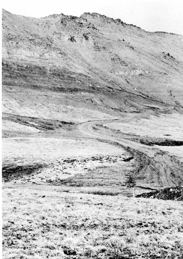
Plate 4. A.S. 119.1: Trail near Slope Mountain material site, hydroseeded and mulched with little growth.
