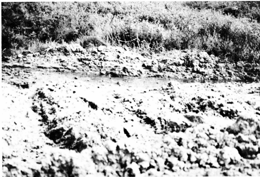
Plate 28. A.S. 66: MP 418 hydroseeded cut. Workpad was soft; several seeps appeared on work pad surface. Potential problems with icings and groundwater flow down trench.
