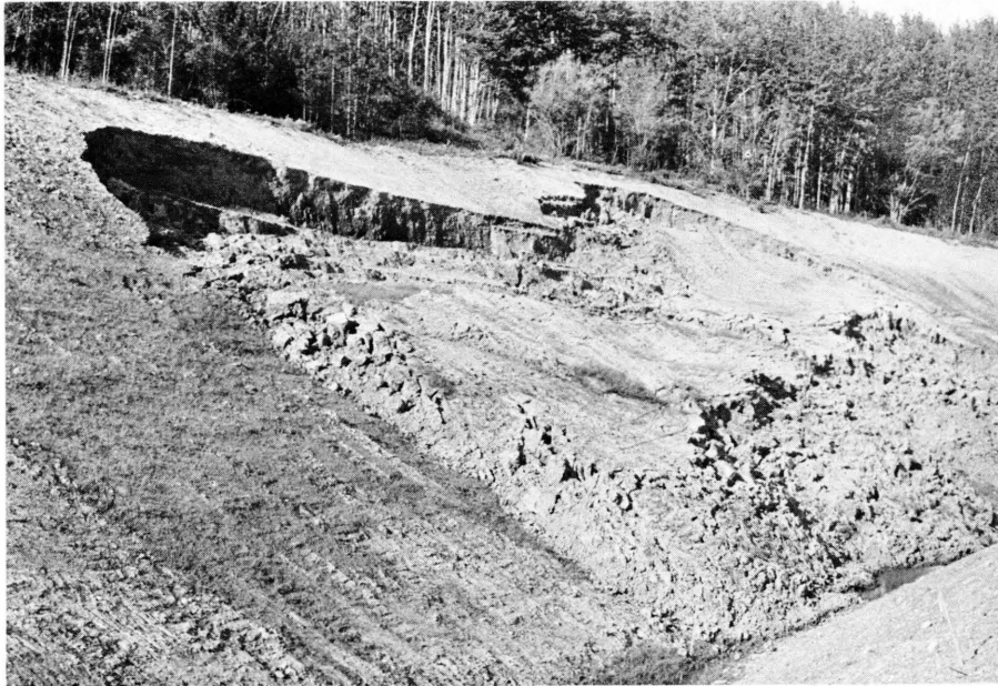
Plate 33. Pump Station 11: Massive deep seated slope failure. Failure began about mid-June after a period of heavy rainfall. Some additional sliding occurred about mid-July. Seeded latter part of June.
