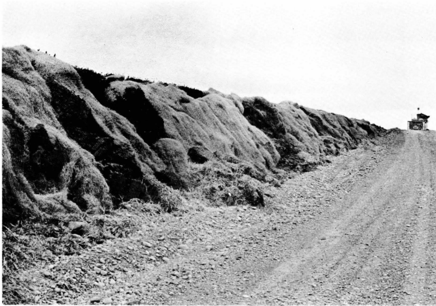
Plate 1. A.S. 131.3: Road cut near Franklin Bluffs airport slumping despite excelsior netting.
