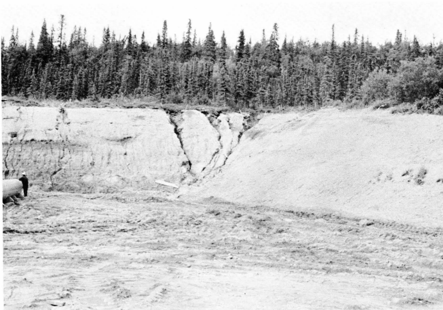
Plate 32. A.S. 28: Large pipe storage yard 2-1R north of Hogan Hill. Some erosion gullies despite hydroseeded slopes. Considerable amount of waste silt had flowed toward Haggard Creek in spring. Dikes used to contain waste silt.
