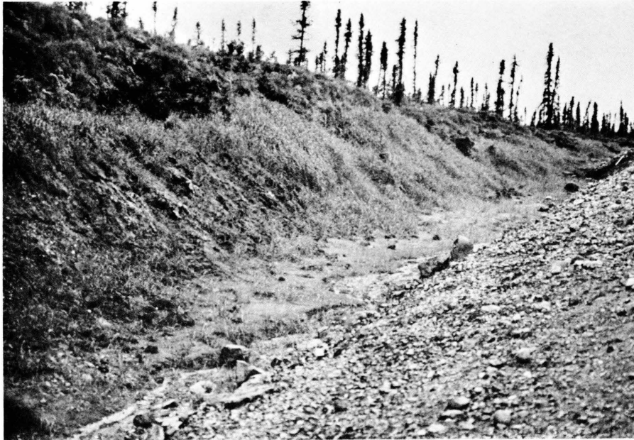
Plate 17: A.S. 91: Hydroseeded road cut with overhanging mat and some tussocks and black spruce.
