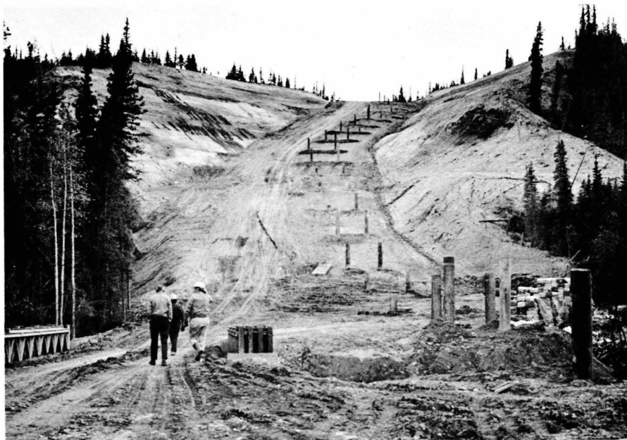
Plate 36. A.S. 16: Steep slope on south side of Squirrel Creek. Some erosion still evident. Wood fiber mulched at 2000 to 2500 lbs/acre. Additional erosion control efforts were planned in 1975.
