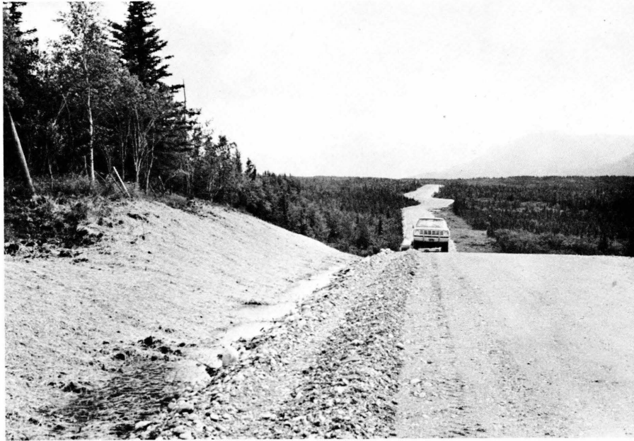
Plate 31. A.S. 42 and 41: Numerous cuts on sides of workpad hydroseeded in alpine area near Donnelly Dome.
