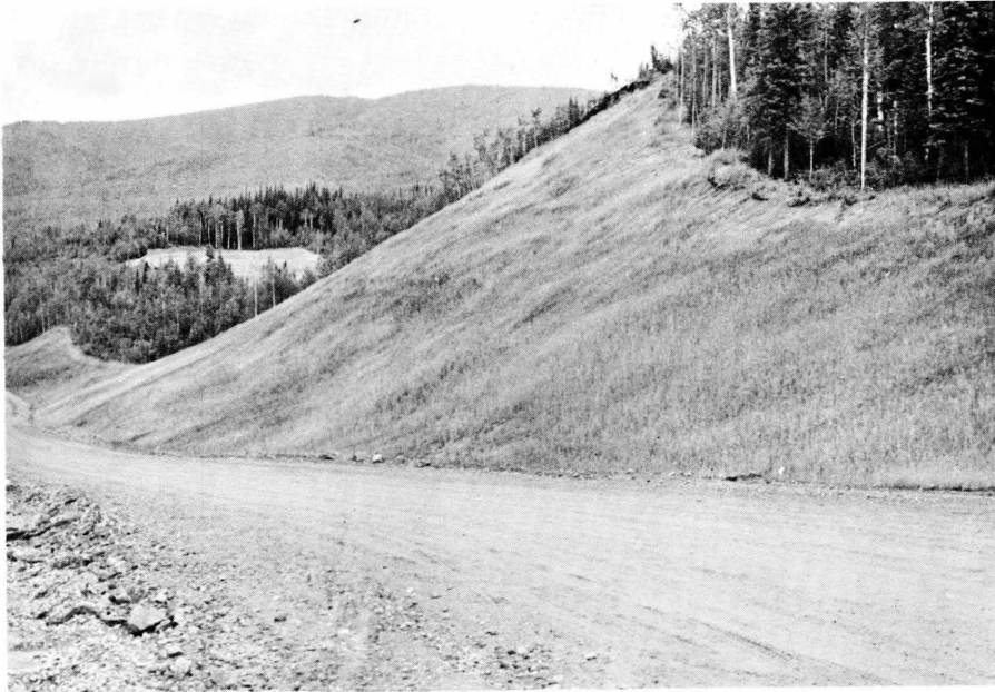
Plate 29. A.S. 51: Massive sandy slopes in vicinity of Rosa Creek. Hay and netting used to stabilize slopes as well as hydroseeded slopes in pipe storage yard and along access road.
