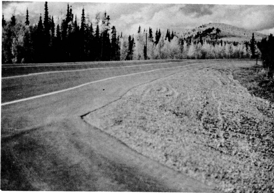
Figure 16. Undulation of pavement on Richardson Highway.
