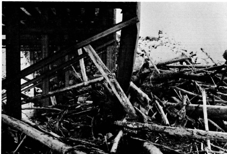
Figure 37. Closeup of damage to Hess Creek bridge.
