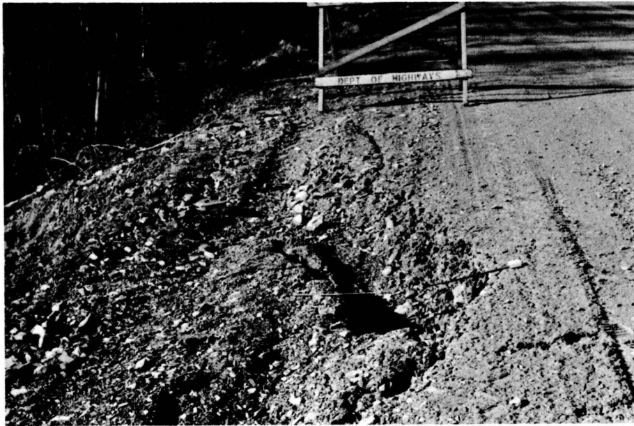
Figure 21. Slope failure along the Elliott Highway
