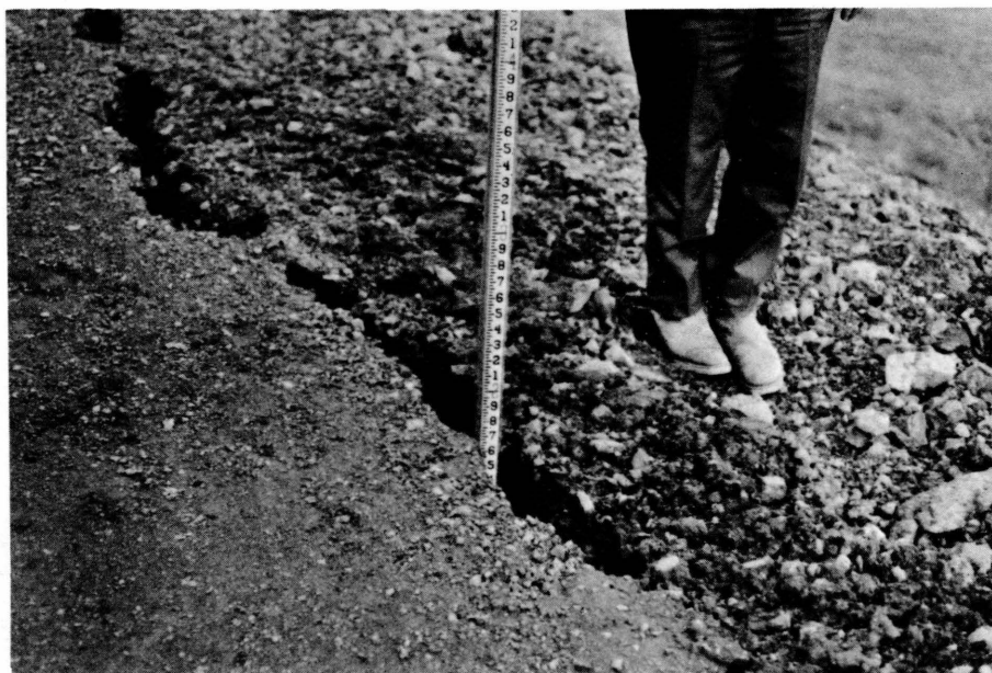
Figure 23. Longitudinal crack caused by settlement of embankment toe (TAPS road, mile 54.9).
