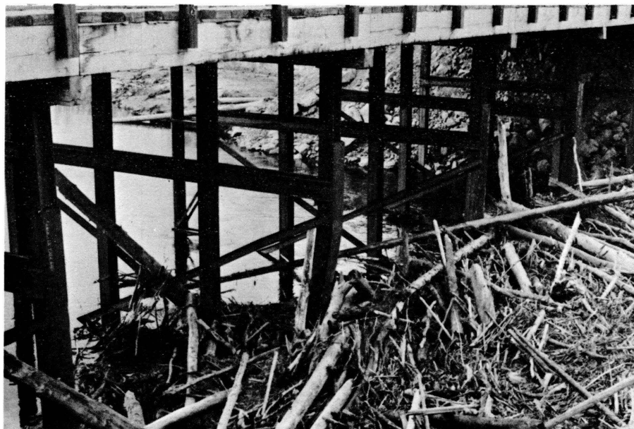
Figure 36. Damage to Hess Creek bridge from ice and debris during high water and ice breakup.
