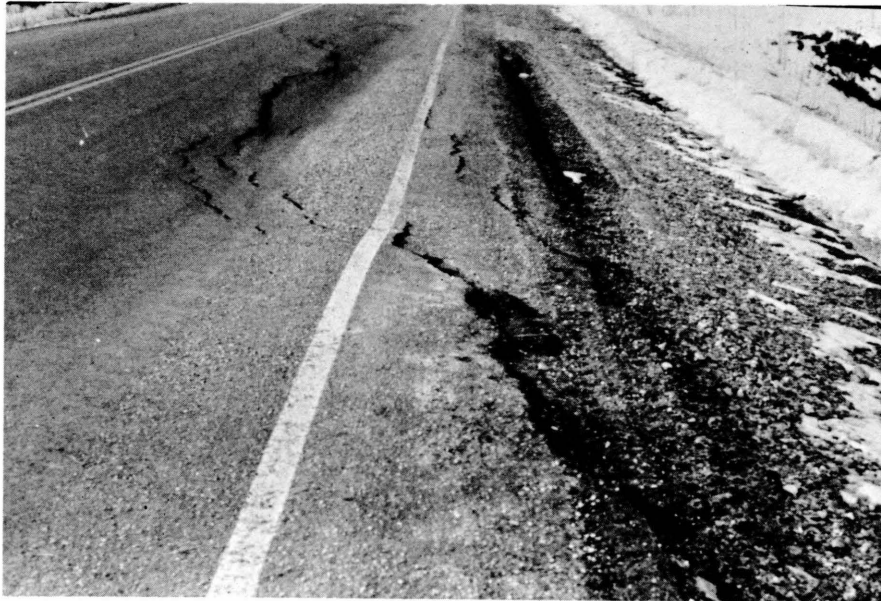
Figure 17. Embankment failure at road shoulder.
