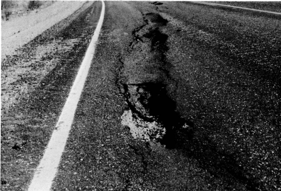
Figure 15. Pavement failure on Chena Hot Springs Road.
