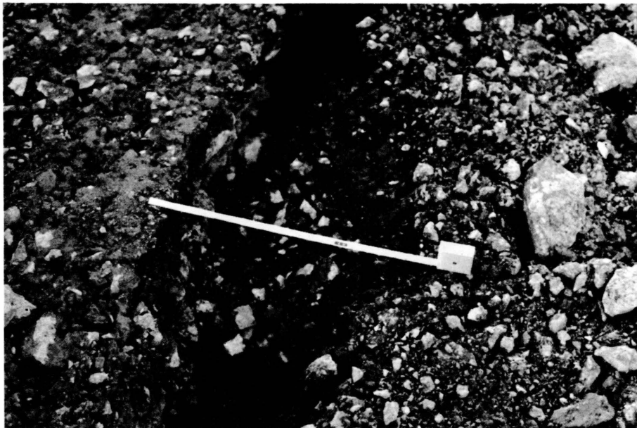
Figure 22. Shoulder failure along TAPS road
