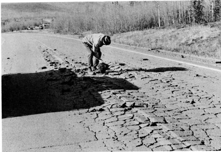
Figure 19. Pavement failure on the Elliott Highway.
