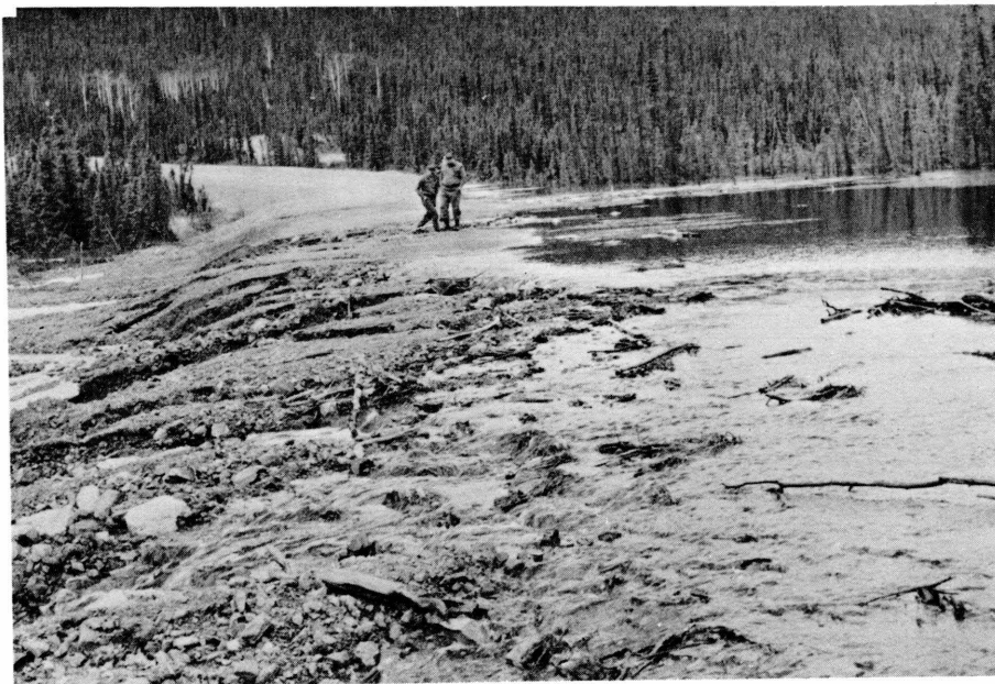
Figure 33. Washout along TAPS road (mile 5.6).
