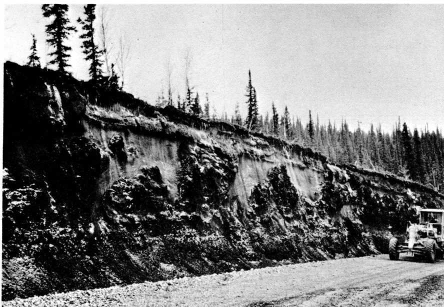
Figure 28. Vertical sidehill cut on TAPS road, 23 April 1970 (Smith and Berg 1973).
