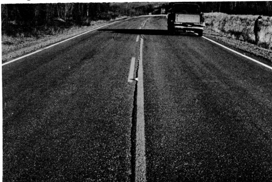
Figure 18. Longitudinal crack along center line.
