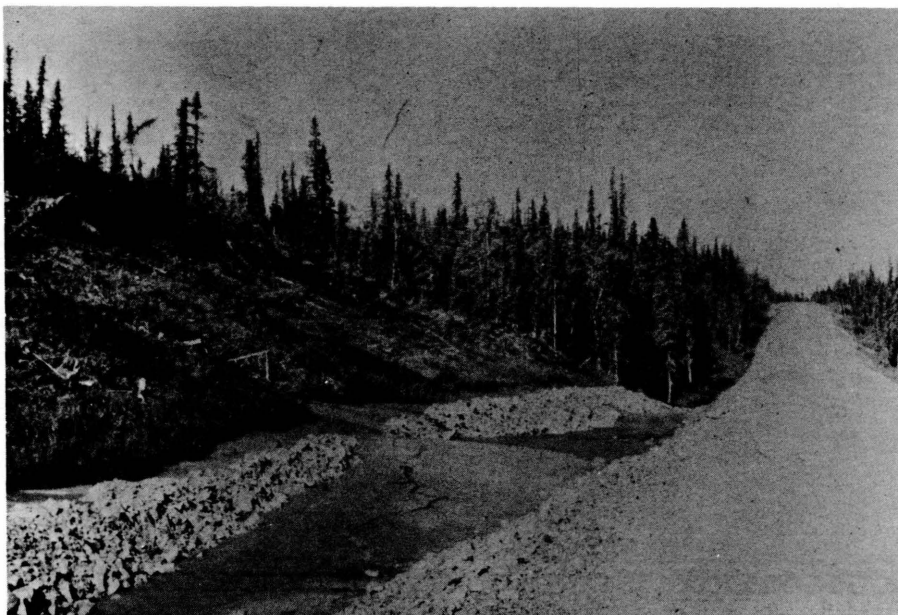
Figure 26. Slope instability on TAPS road (from Smith and Berg 1973).
