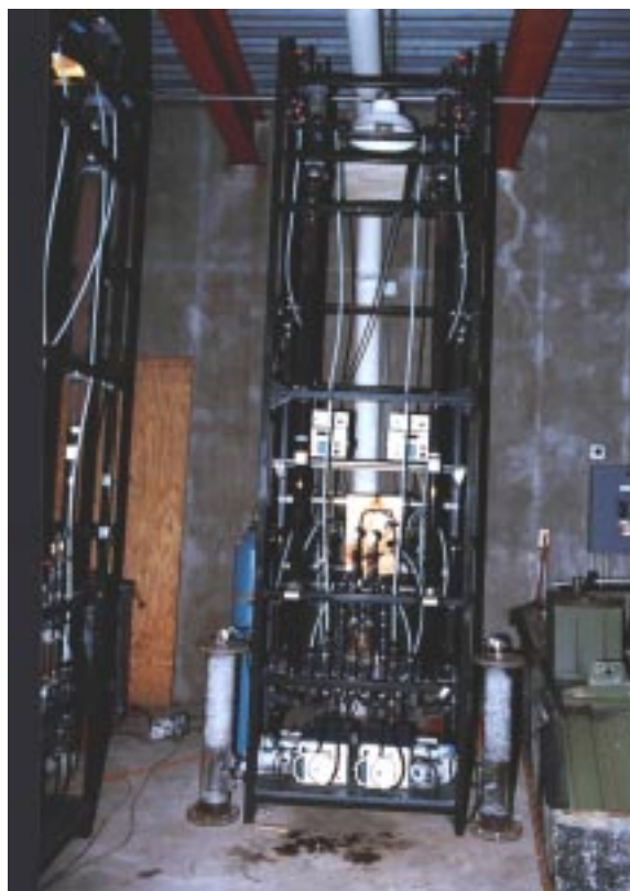
Figure 3. Skid 1 of the pilot scale fluidized-bed adsorption bioreactor system.
