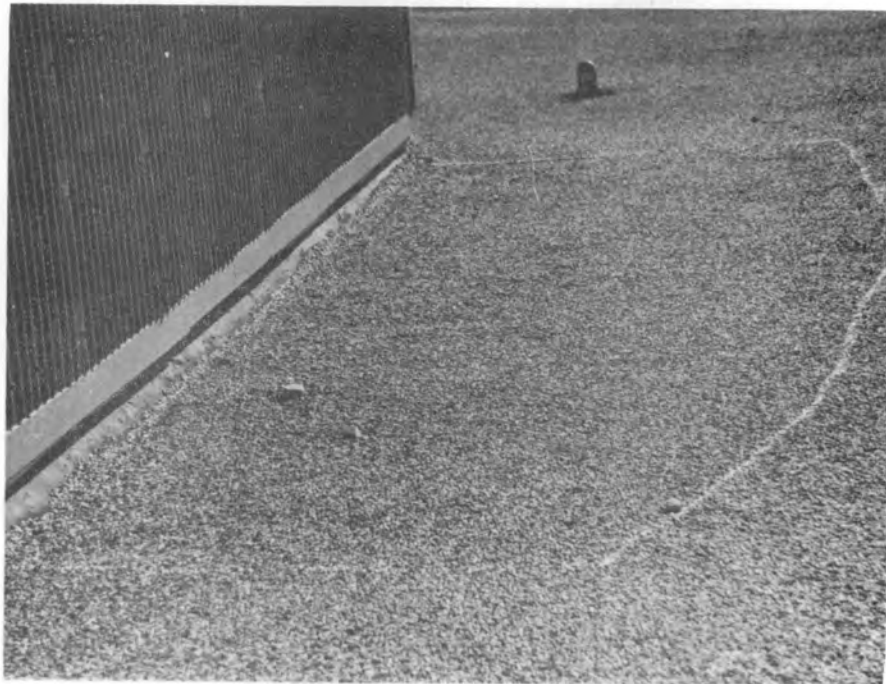
Figure 16. 1977 thermogram and photograph of wet area abutting parachute flue, Building 112.
