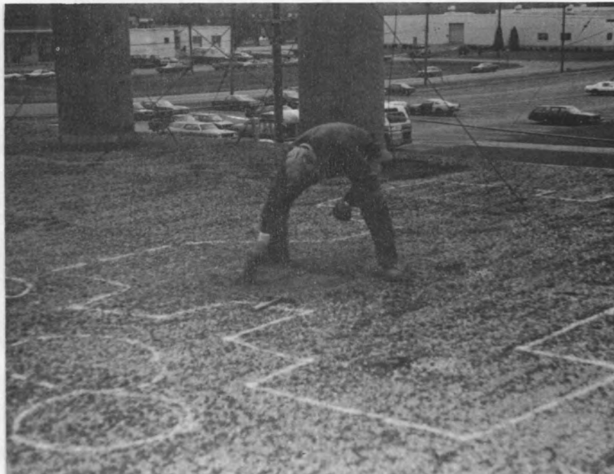
Figure 7. 1975 thermogram and 1977 photograph showing extent of wet area surrounding bolt, Building 120.
