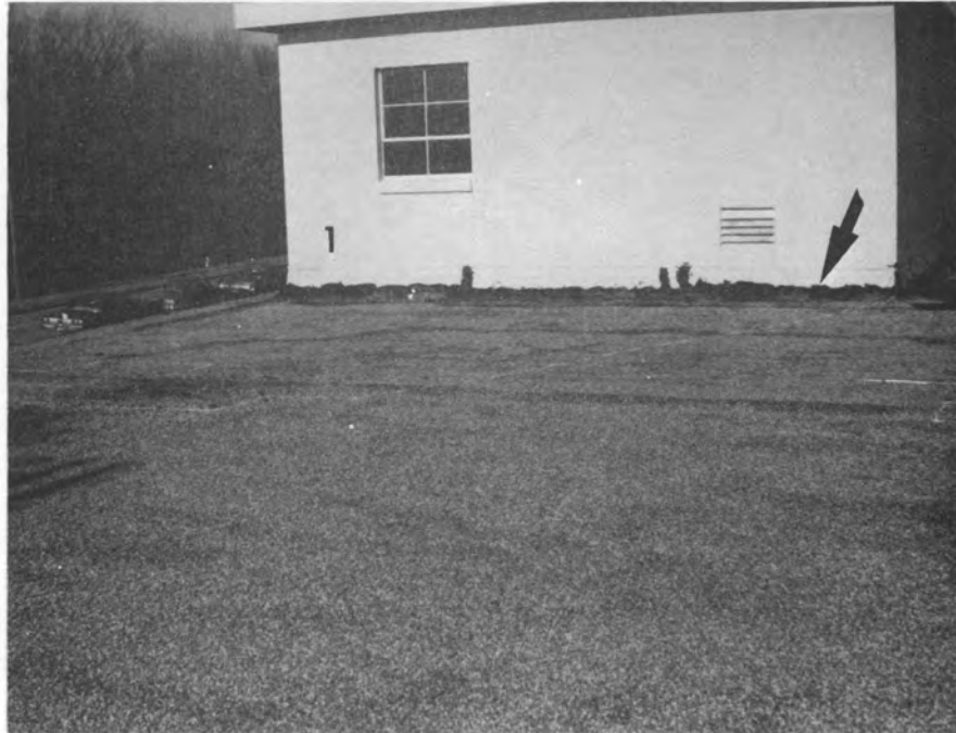
Figure 2. Thermogram and photograph of wet area abutting the penthouse on Building 113 (arrow points to patched flashing).
