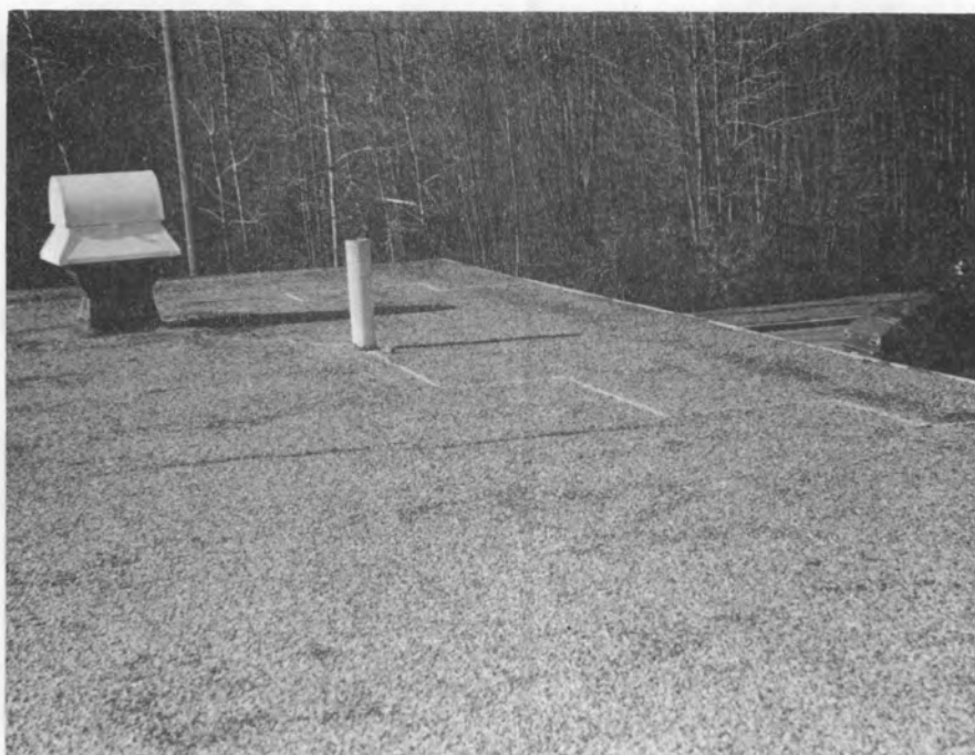
Figure 3. Thermogram and photograph of wet area that appears to be emanating from the base of a roof fan, Building 113.
