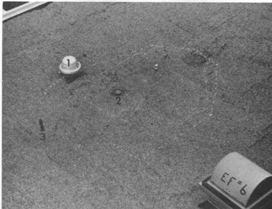
Figure 22. 1977 thermogram and photograph of wet area in Figure 19.
