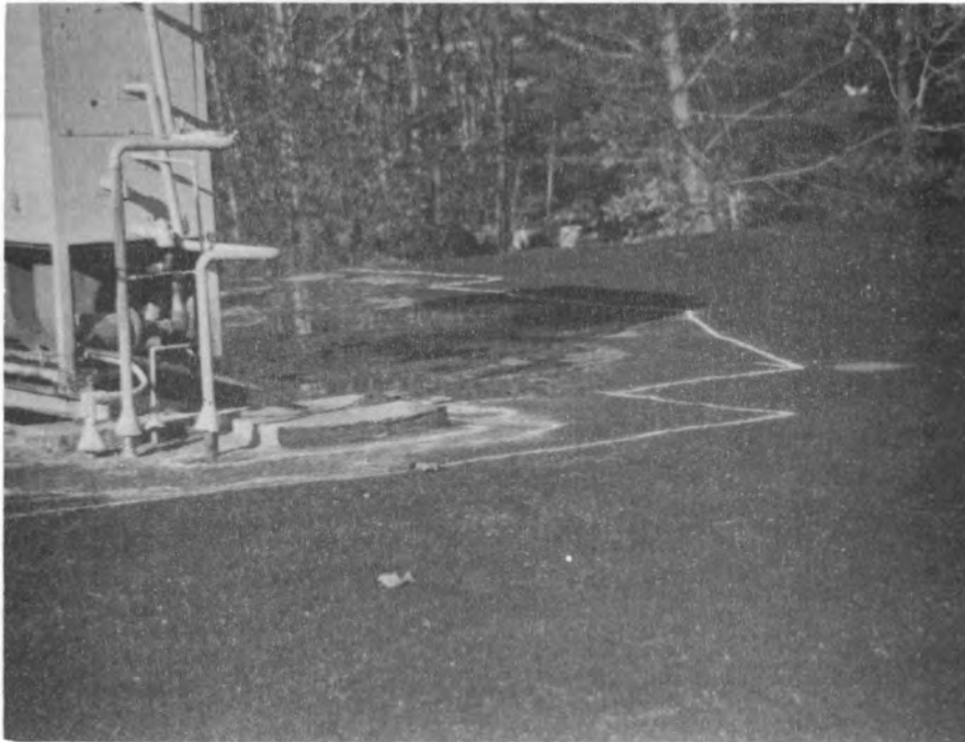
Figure 12. Thermogram and photograph of a wet area on Building 35.
