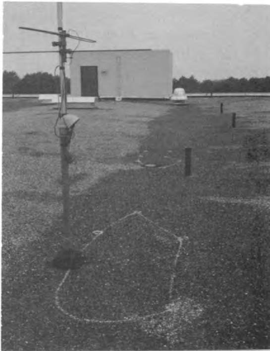
Figure 20. Painted boundaries of two 1976 thermal anomalies on the upper roof. Both anomalies are associated with roof penetrations (i.e., an antenna and a drain).
