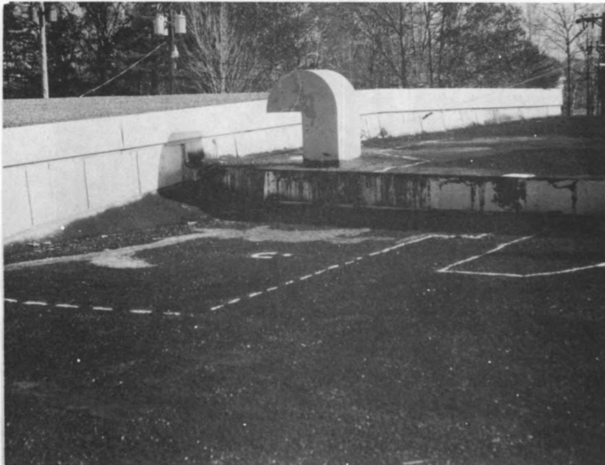
Figure 13. Wet areas on roof of Building 35 (arrow points to a split in the roof membrane).
