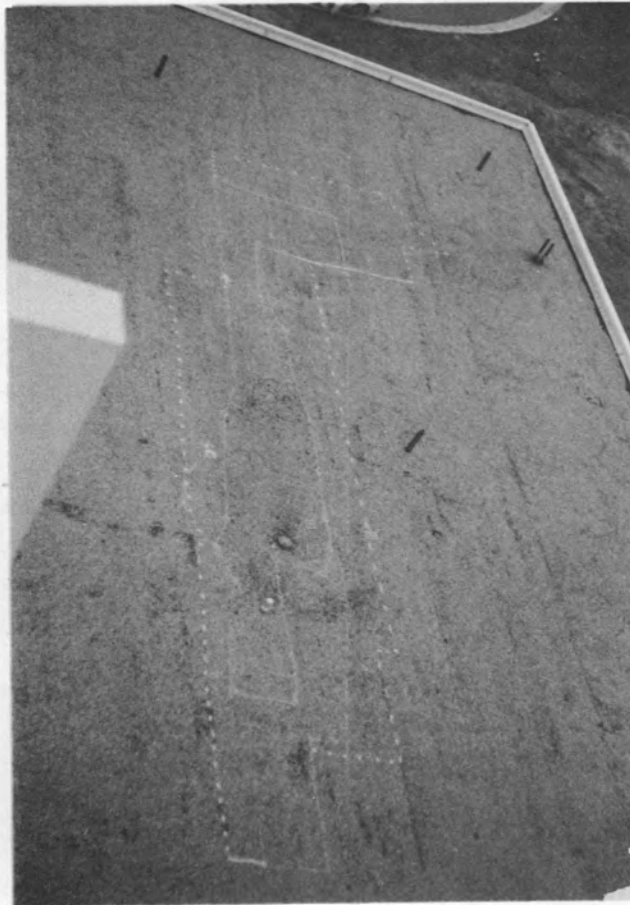
Figure 23. Thermogram and photograph of wet area on Building 93 (solid line shows extent of wet area in 1976, dotted line shows extent of wet area in 1977).
