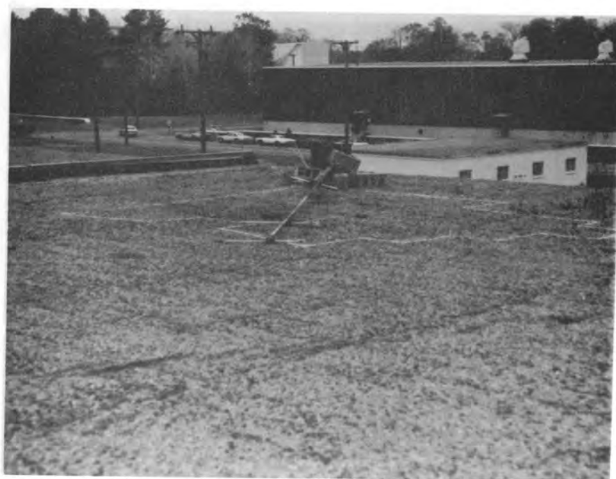
Figure 10. 1975 (top) and 1977 photographs of wet area in bay 2, Building 120. Notice increase in extent of outlined area.
