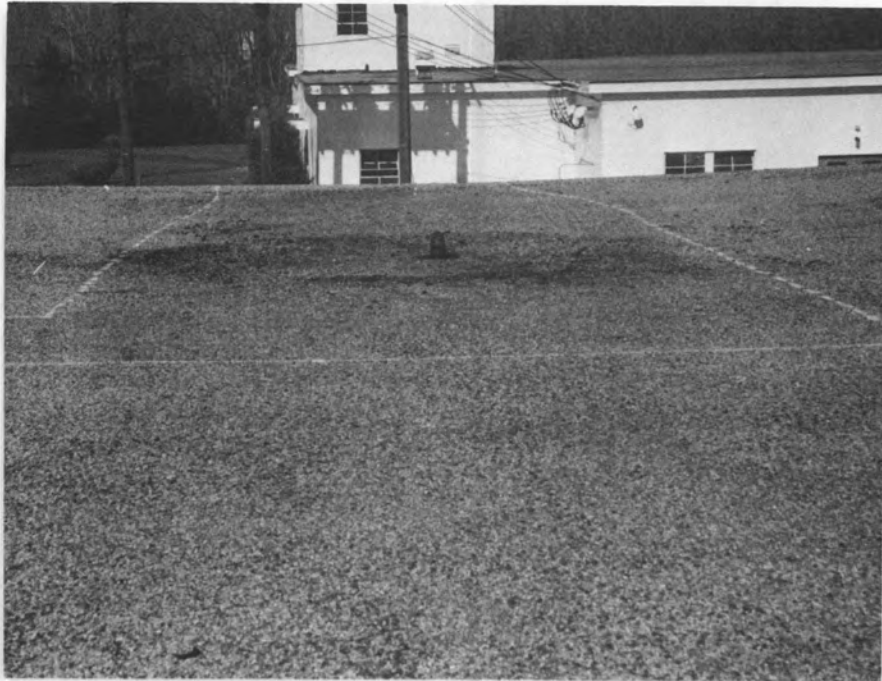
Figure 15. 1977 thermogram and photograph of wet area, Building 112.
