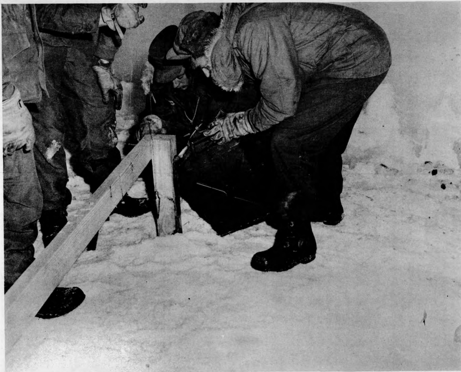
Figure 7. Aligning and freezing post into place using ice cuttings and water to saturate.
