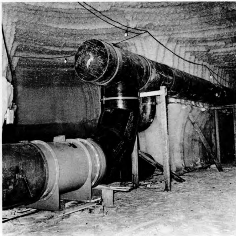
Figure 10. Single 15 hp 10,000 cfm ventilation fan installed during construction to provide ventilation in tunnel.
