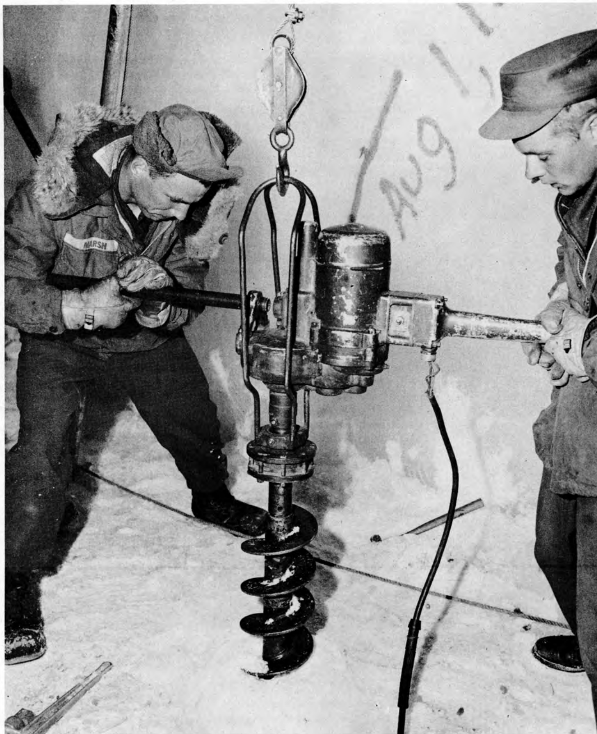
Figure 6. Augering hole in ice floor preliminary to installation of 4 x 4 underpinning post.
