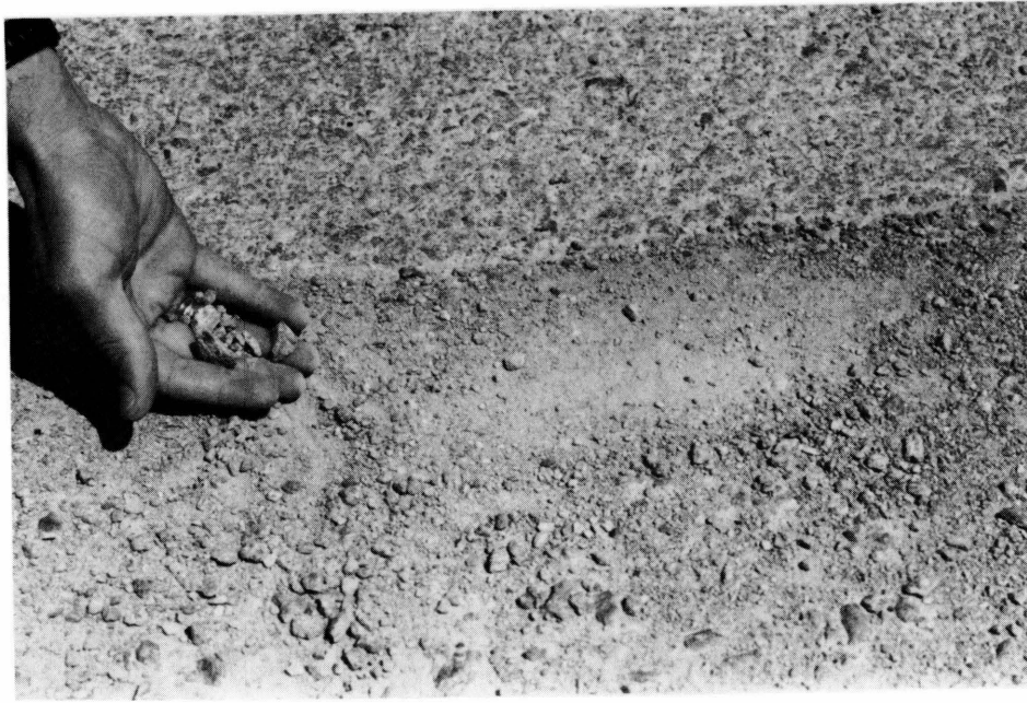
Figure 5. Loose pavement material at the vicinity of cold joints when opened to traffic.
