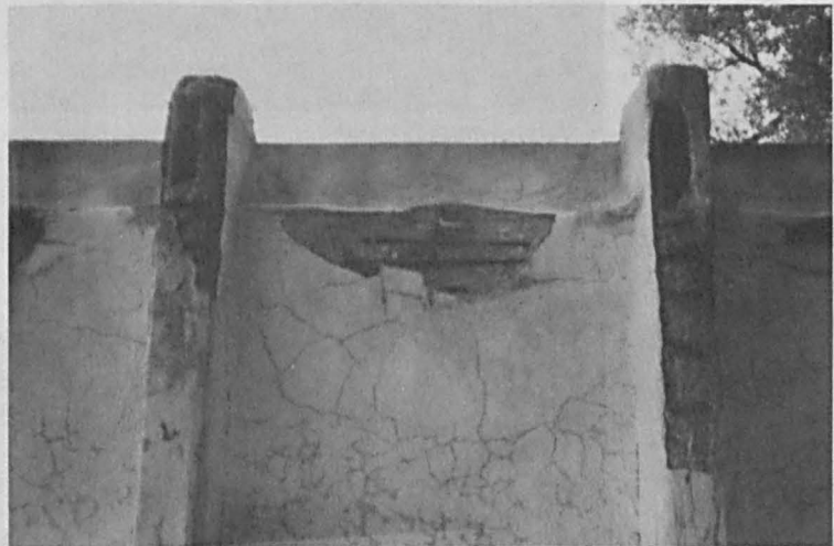
b. Exposure of rebar and steel elements
