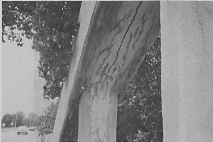
a. Cracks running parallel with arch
