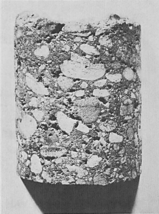
CONCRETE WITH NUMEROUS LARGE VOIDS, DEPTH ABOUT 33 FT., CORE 5-1. THE SURFACE IS TYPICAL OF THE CORE FROM 14.5 FT. TO 39.6 FT. DIRECTION OF PLACEMENT TOWARDS BOTTOM OF PHOTOGRAPH. THE VOIDS ARE MORE FREQUENT ADJACENT TO COARSE AGGREGATE PARTICLES.
