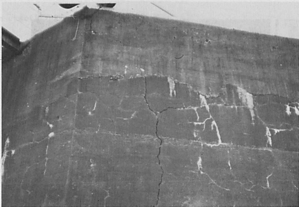
Fig. 78. Portions of Monolith No. 51 repair after approximately 20 years.
