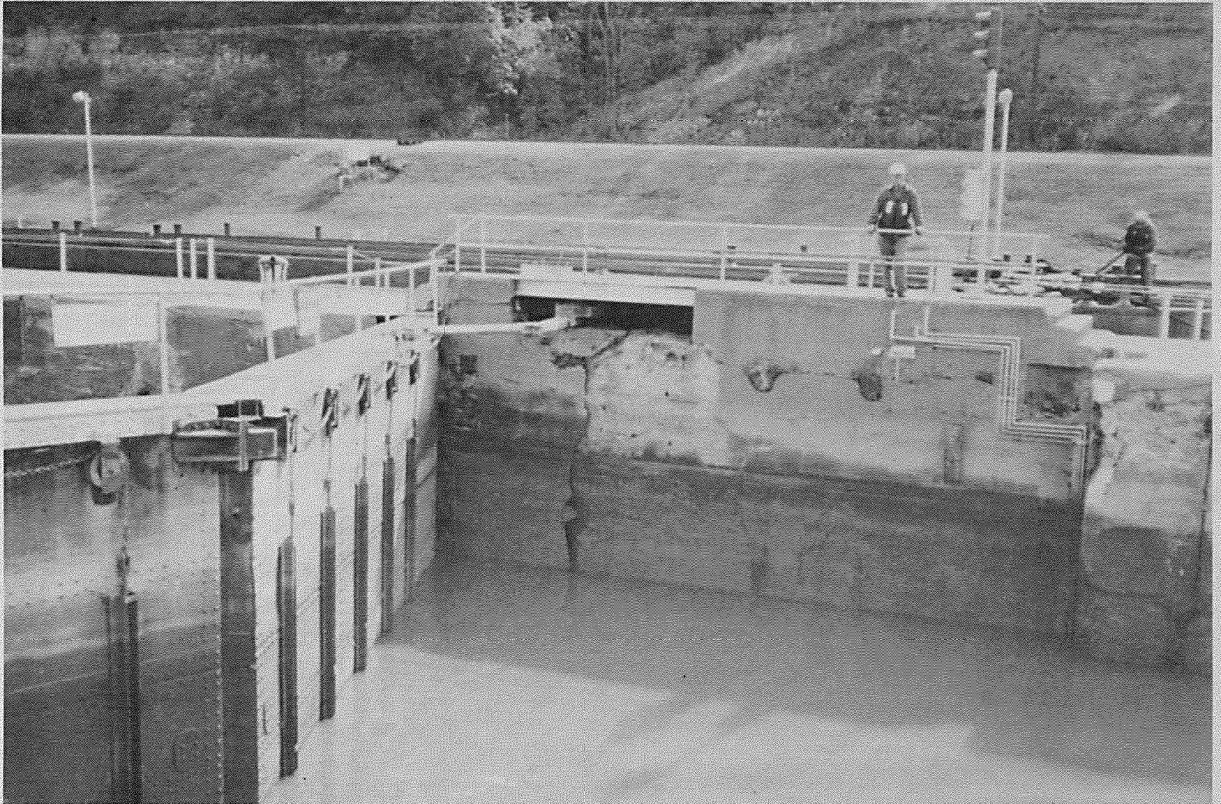
Figure 7.2. Deteriorated Locations at Gate Anchorages
