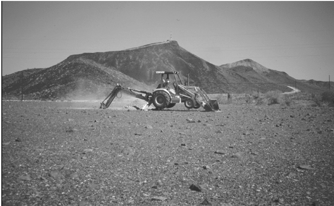
Figure 3. Soil pit excavation on the Qf1b Pleistocene geomorphic surface. The volcanic cone in the background is outside (north of) the study area boundary.
