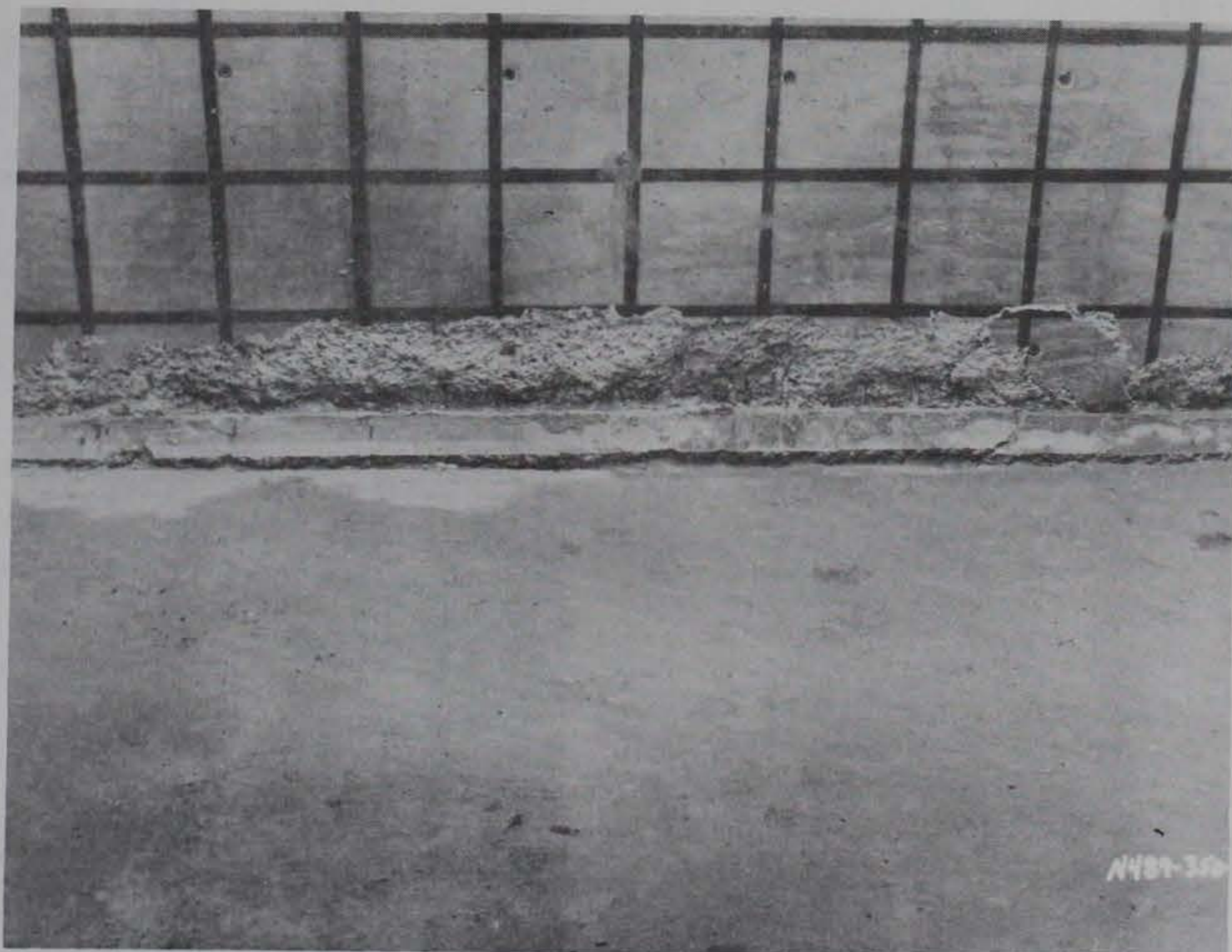
b. Damage to lower edge.
