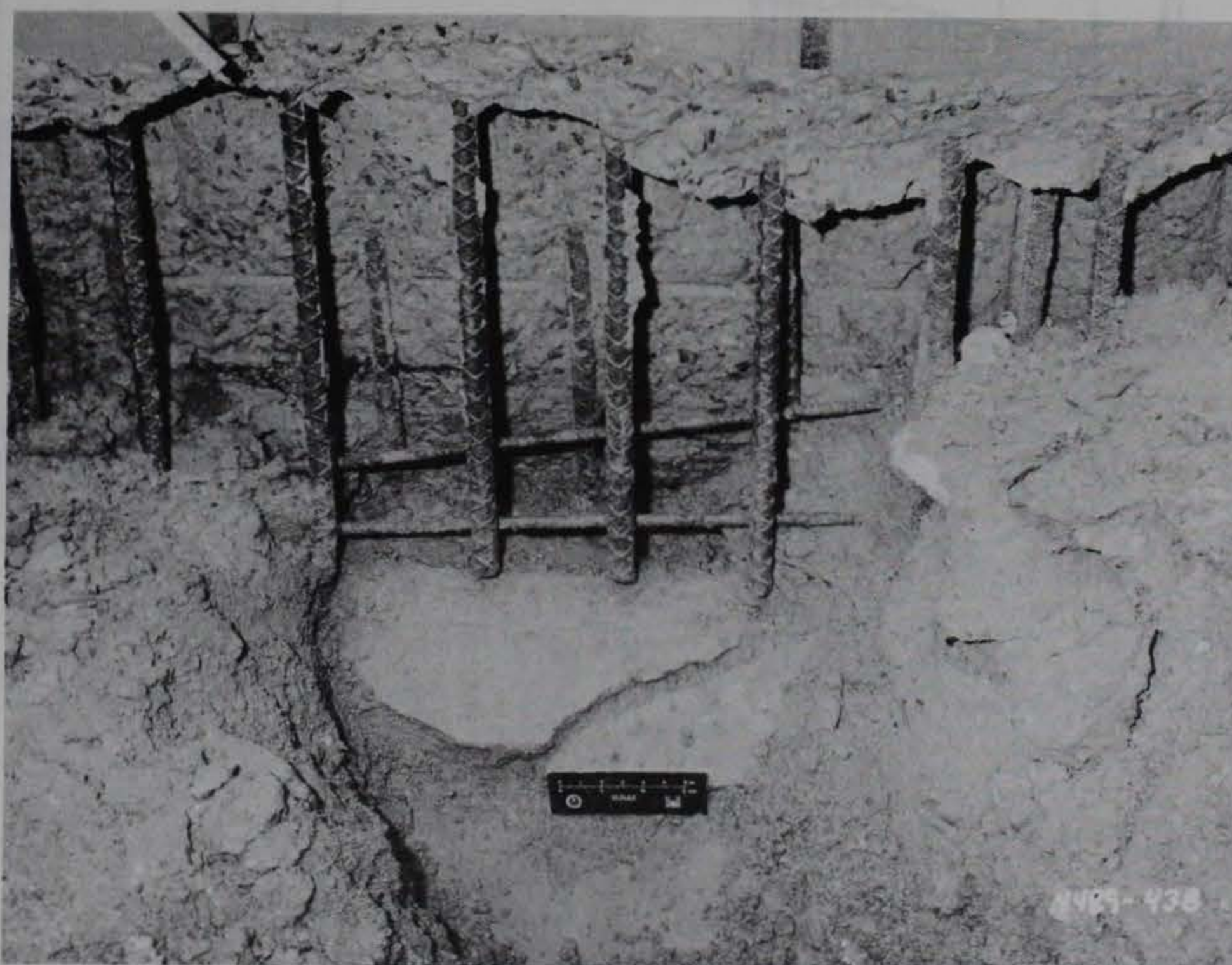
b. Reinforcement separation at base of wall.
