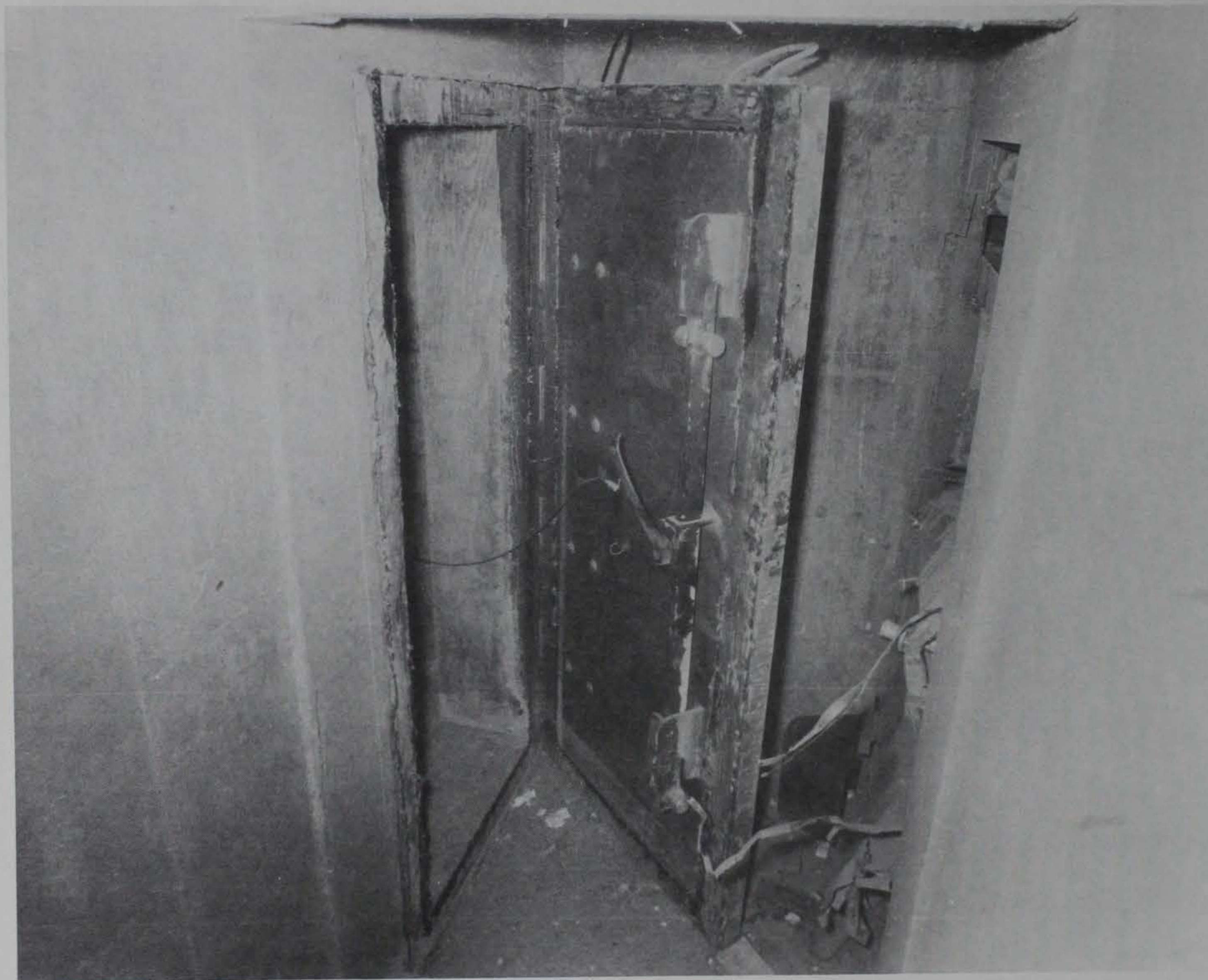
Figure 4.4. Closures, reinforced concrete blast door on left, open, commercial door on right.
