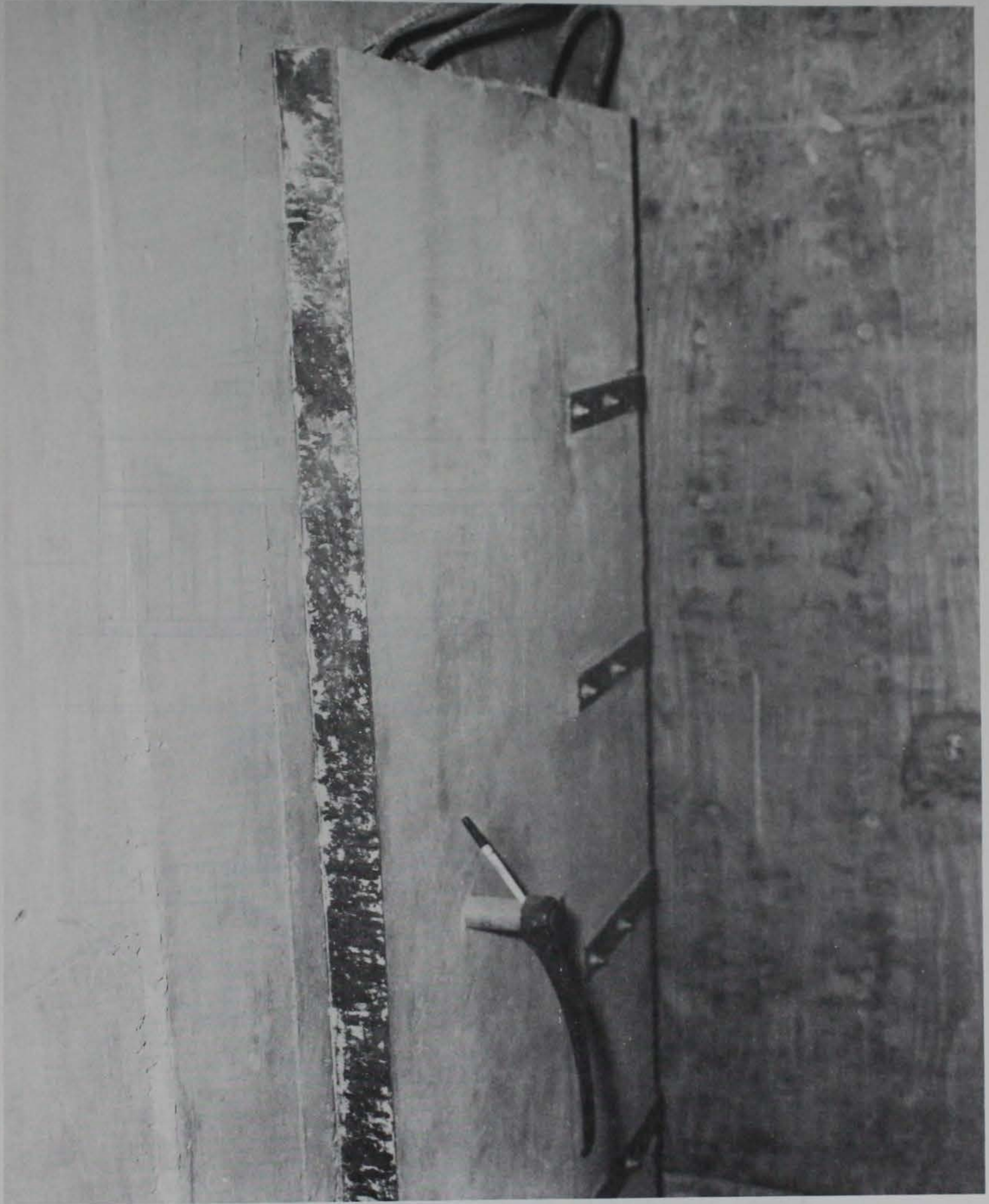
Figure 3.4. Reinforced concrete blast door in place.
