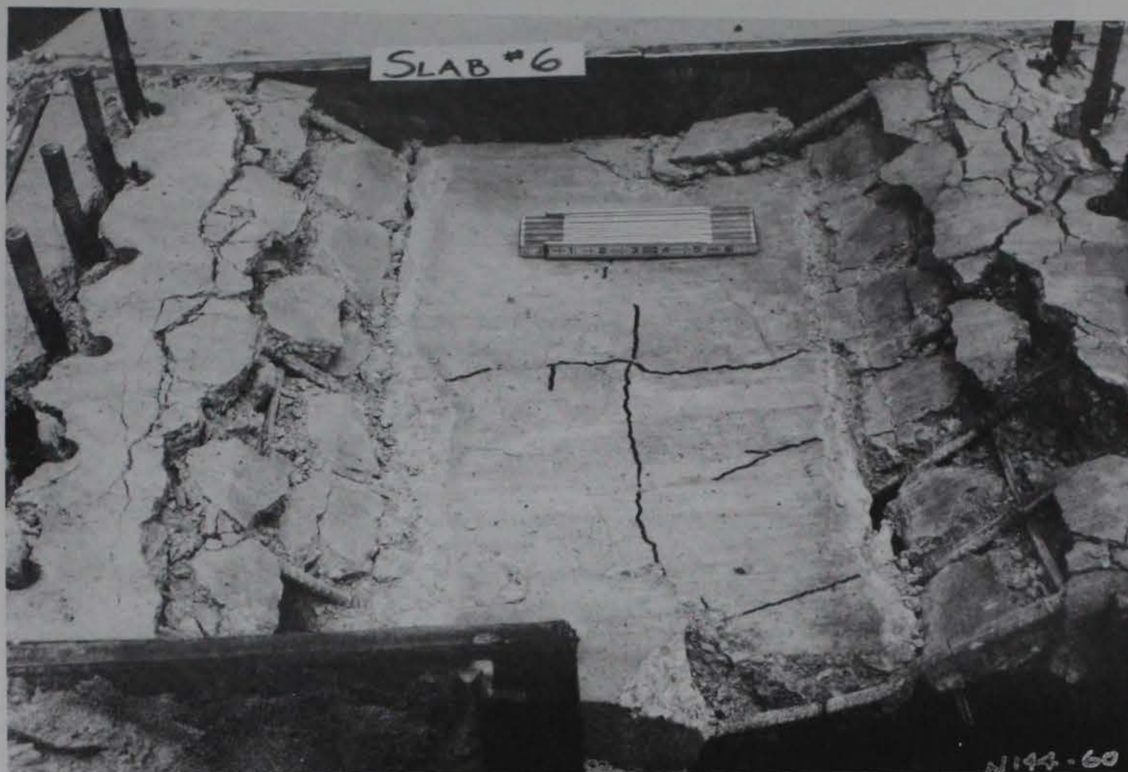
Figure 4.16. Closeup view of Slab 6 following retest.
