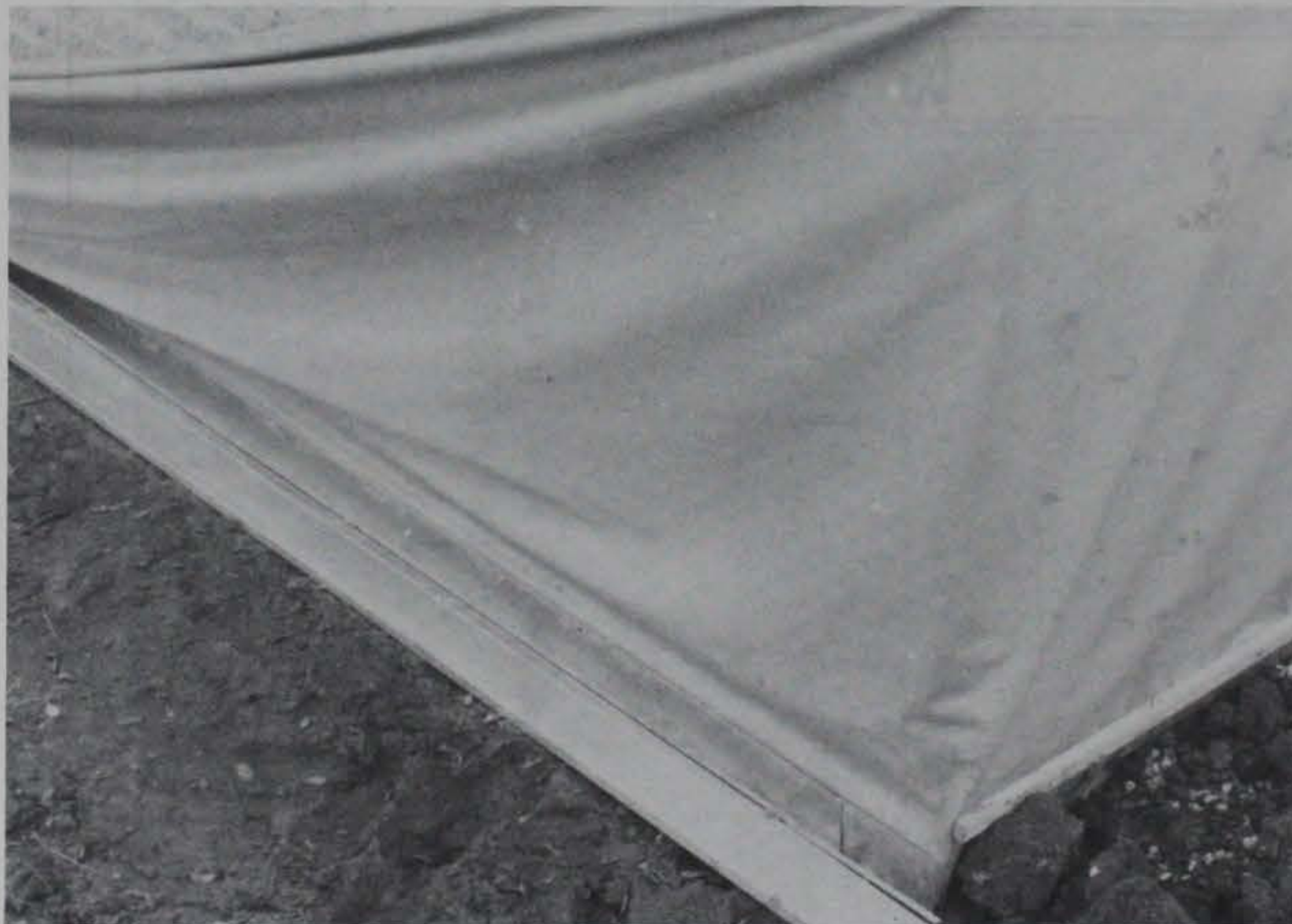
Figure 58. Protective fabric being removed from storage container and attached to the house at the desired elevation
