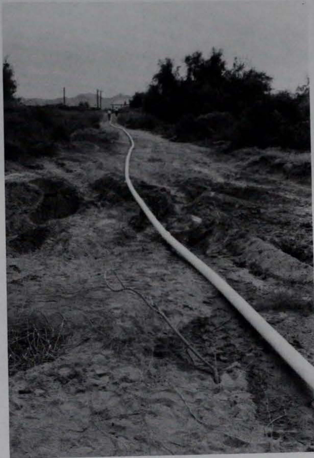
Figure 48. Pipe through which water was pumped to test house
