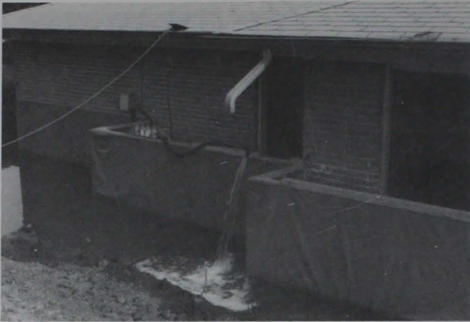
Figure 61. Water being pumped outside the protected area
