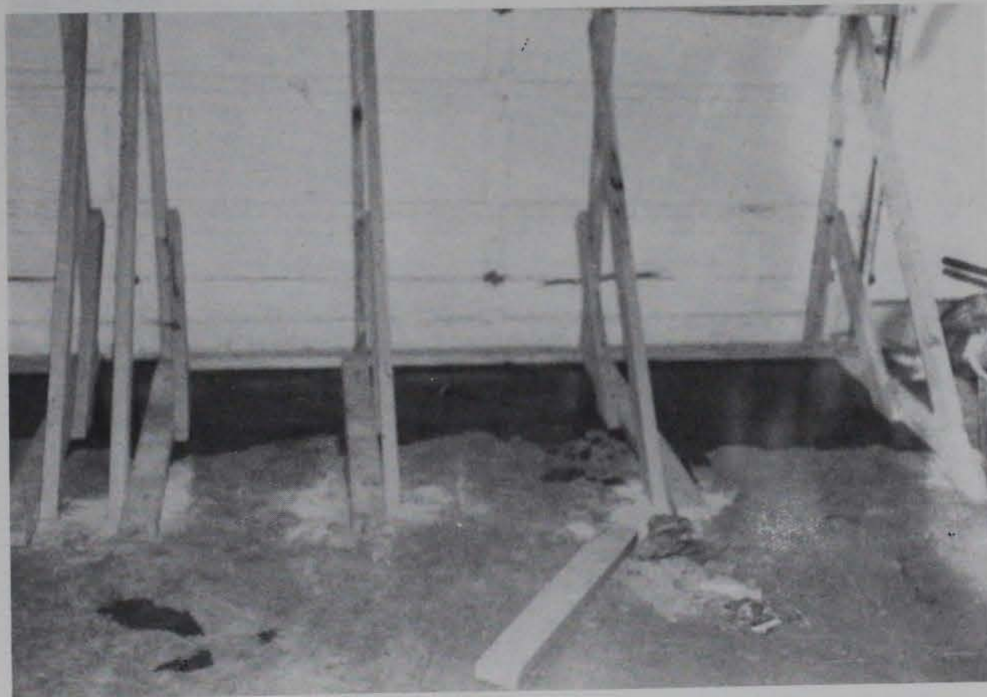
Figure 64. Water seeping under garage door due to allowing excessive water height in sump
