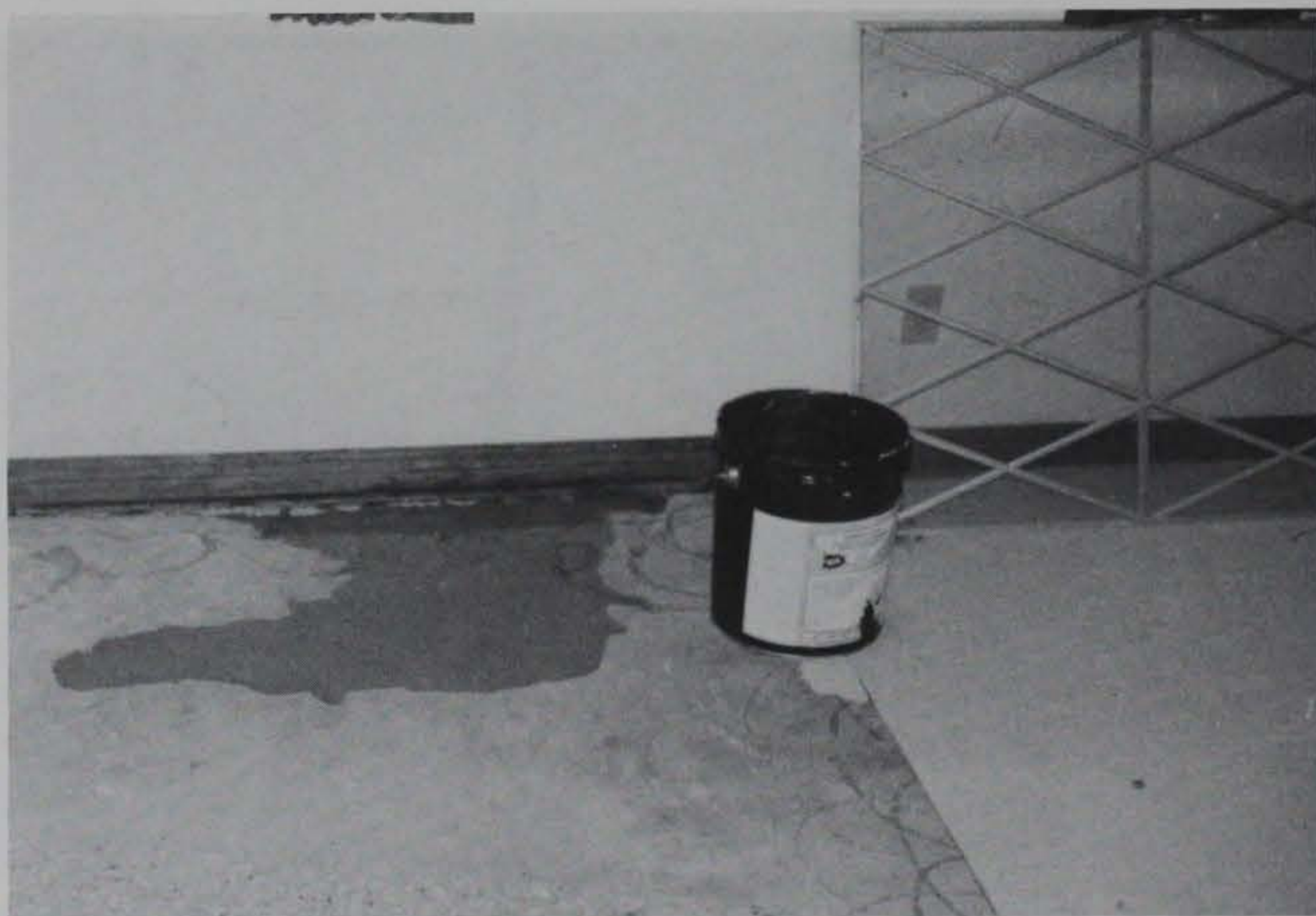
Figure 65. Seepage along baseboard due to leak in lap of fabric
