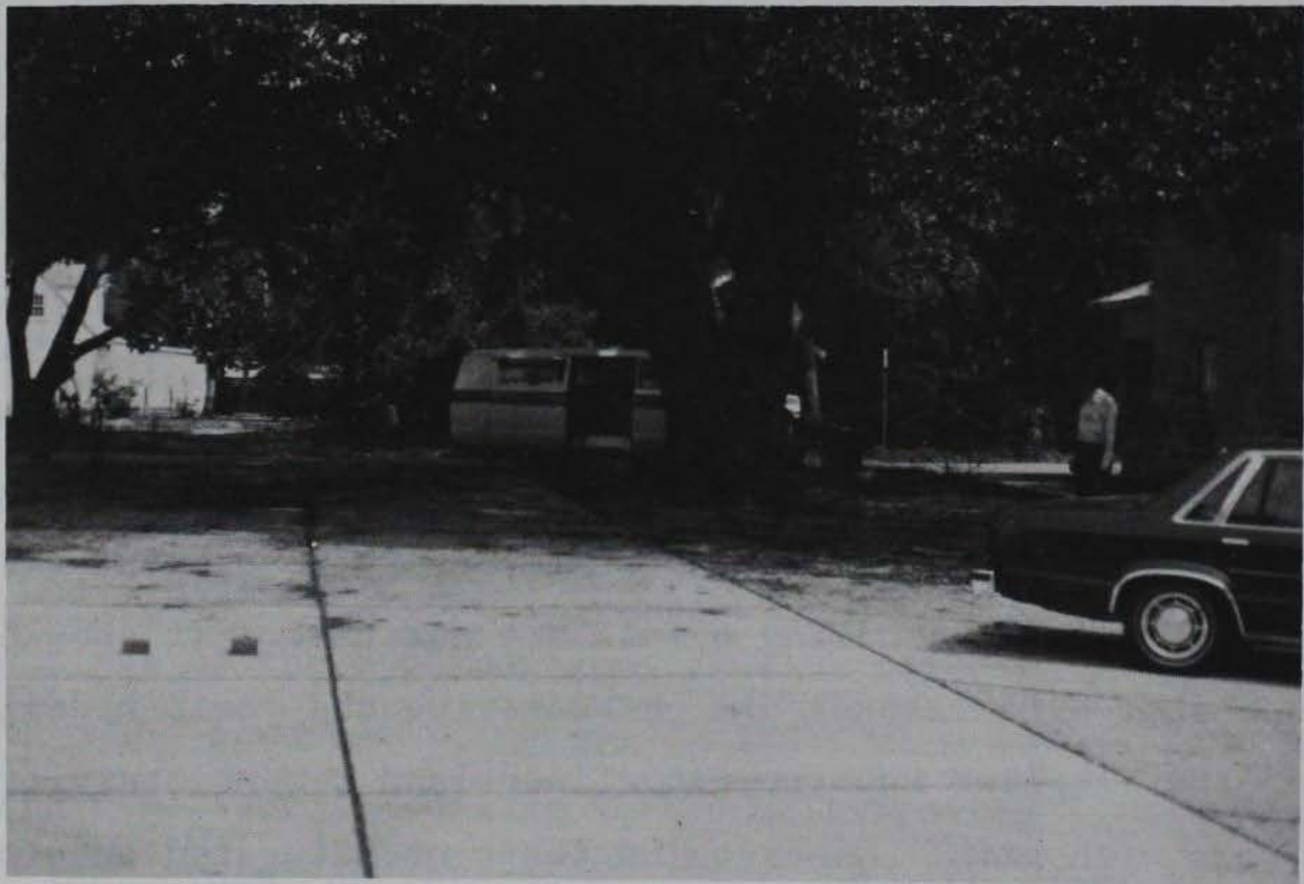
Figure 1. One-year condition of a porous concrete parking lot
