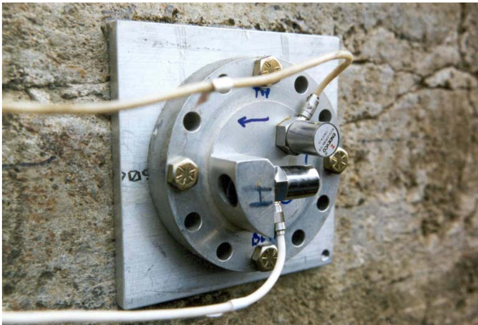
Figure 16. Biaxial accelerometers on lock wall
