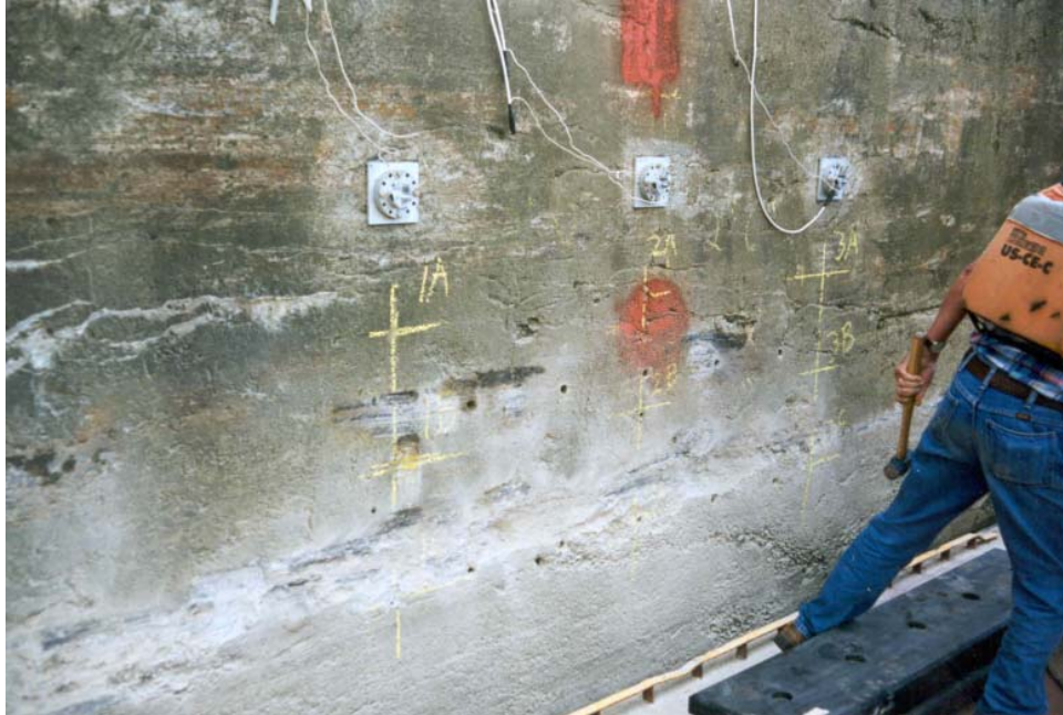
Figure 15. Lock wall accelerometers
