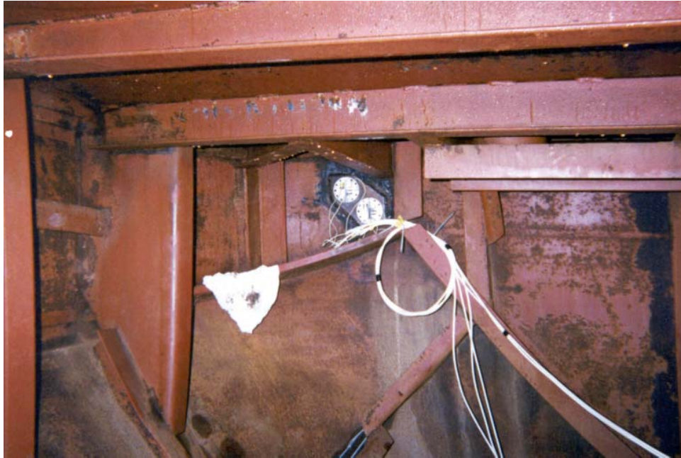
Figure 11. Accelerometers installed under deck
