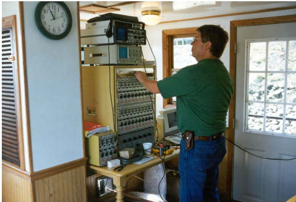
Figure 7. Data acquisition system located below the towboat's pilothouse
