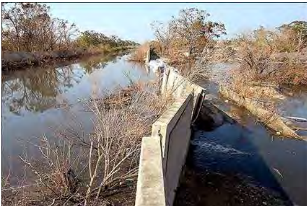
Figure 1.1. I-wall failures in London Canal during Hurricane Katrina.
