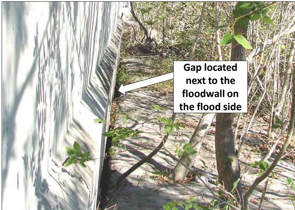
Figure 1.2. Development of a zone of separation between the I-wall and the soil interface on the flood side of the I-wall following Hurricane Katrina.
