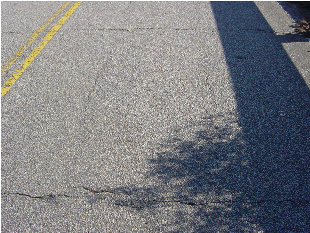
Figure 2. Longitudinal and transverse cracks in asphalt.
