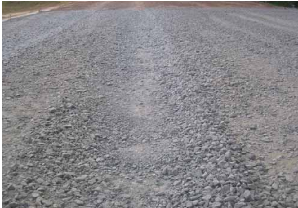
Photo C78. Item 9 (IGN), dry lane, new construction test section, 500 passes with pickup truck
