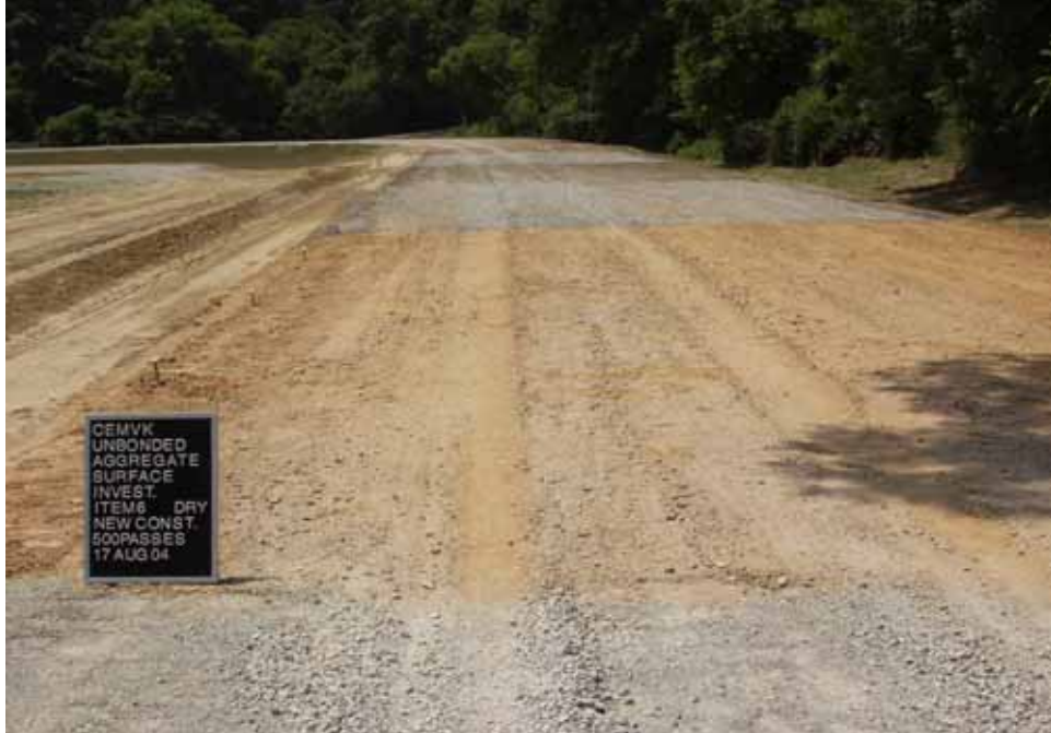
Photo C71. Item 6 (SCG), dry lane, new construction test section, 500 passes with pickup truck
