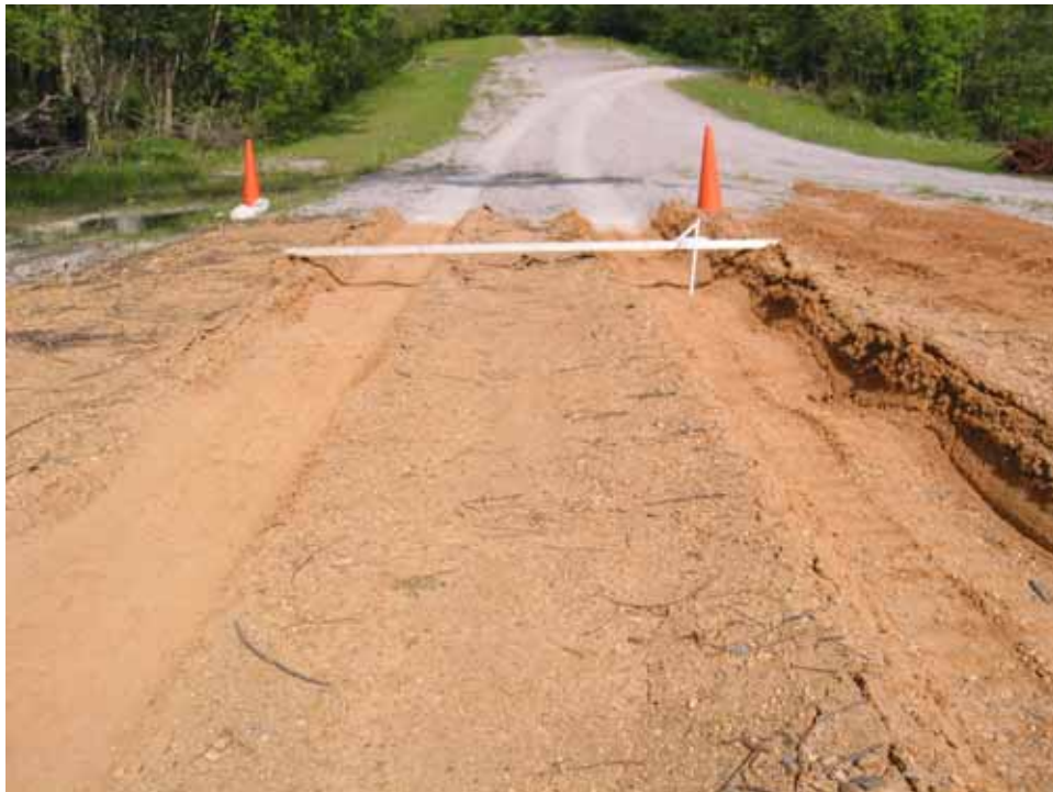
Photo C104. Item 6 (SCG), wet lane, new construction test section, 25 passes with CBR truck
