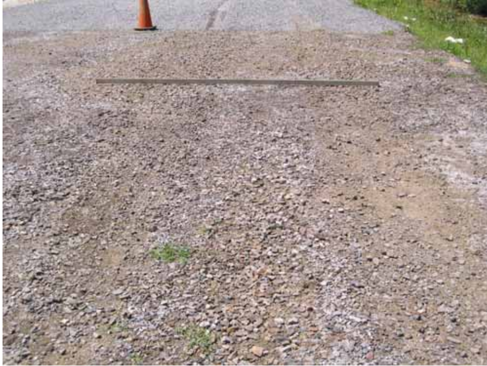
Photo C99. Item 8 (SST), wet lane, new construction test section, 25 passes with pickup truck
