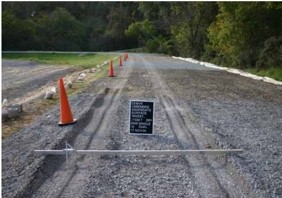
Photo C92. Item 7 (LST), dry lane, new construction test section, 10 passes with dump truck
