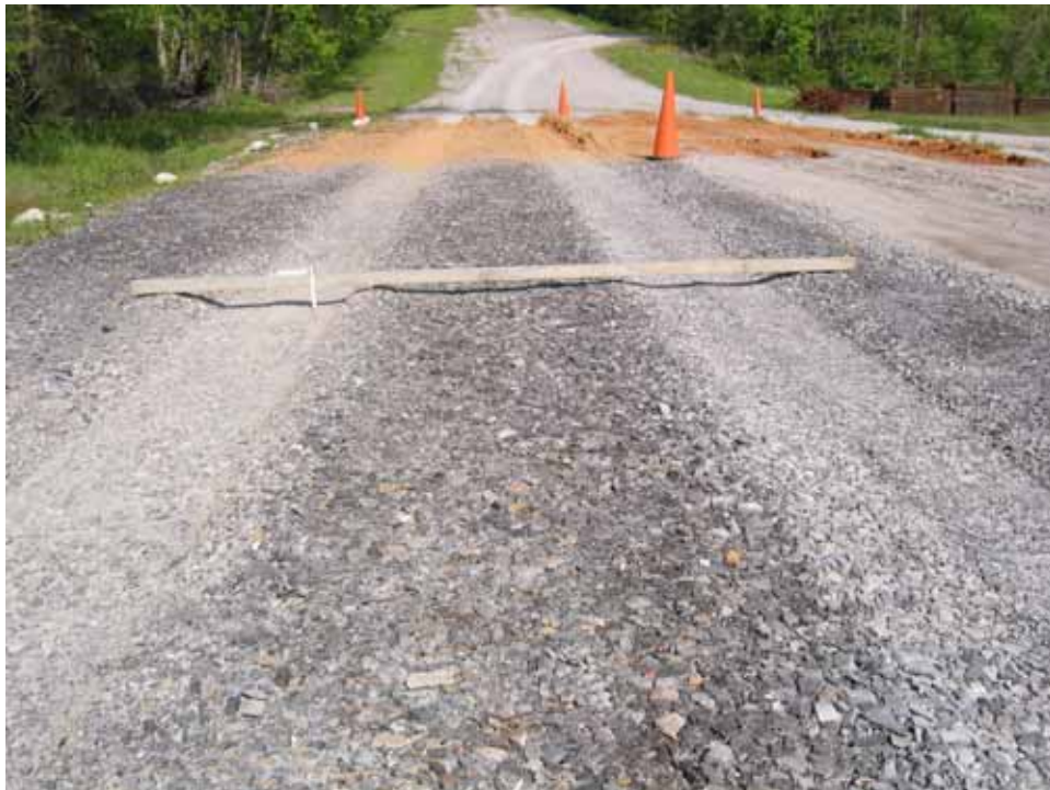
Photo C106. Item 7 (LST), wet lane, new construction test section, 25 passes with CBR truck
