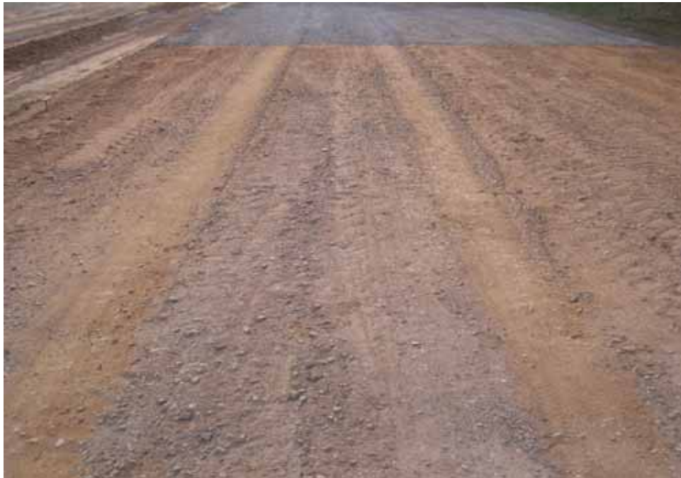
Photo C72. Item 6 (SCG), dry lane, new construction test section, 500 passes with pickup truck
