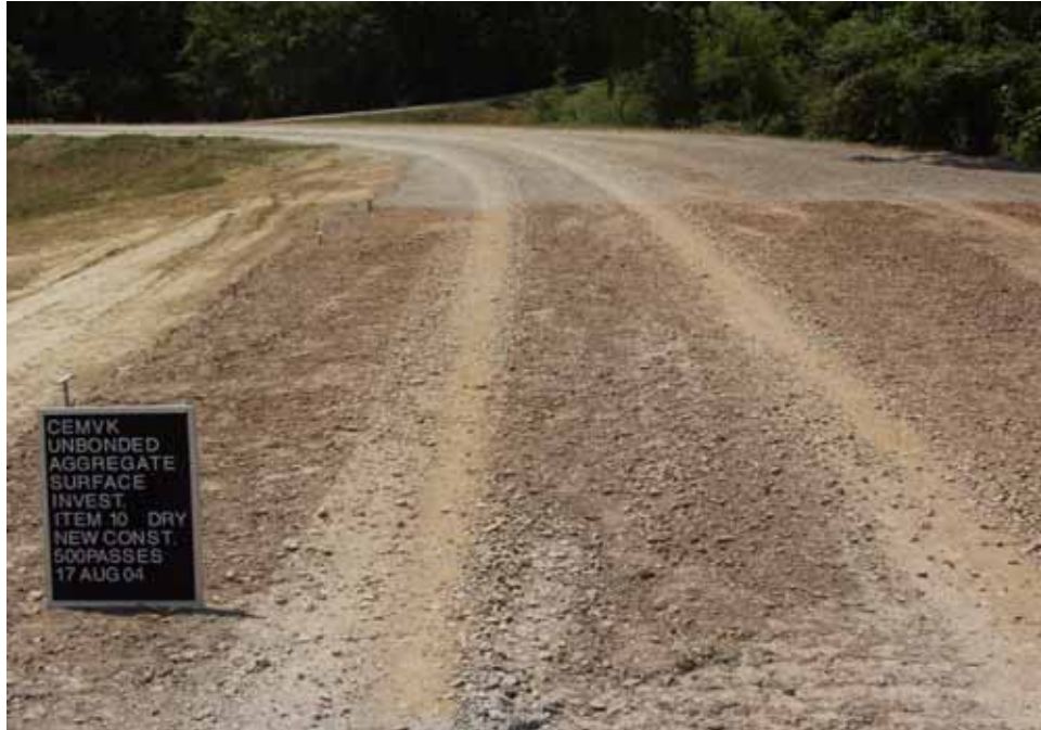
Photo C79. Item 10 (SSB), dry lane, new construction test section, 500 passes with pickup truck
