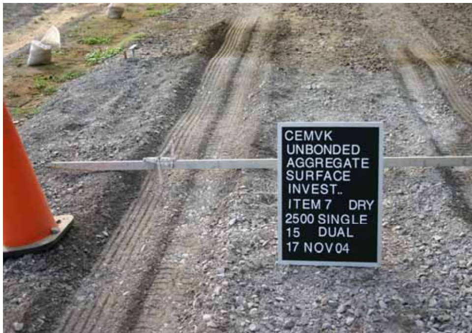
Photo C96. Item 7 (LST), dry lane, new construction test section, 15 passes with dump truck
