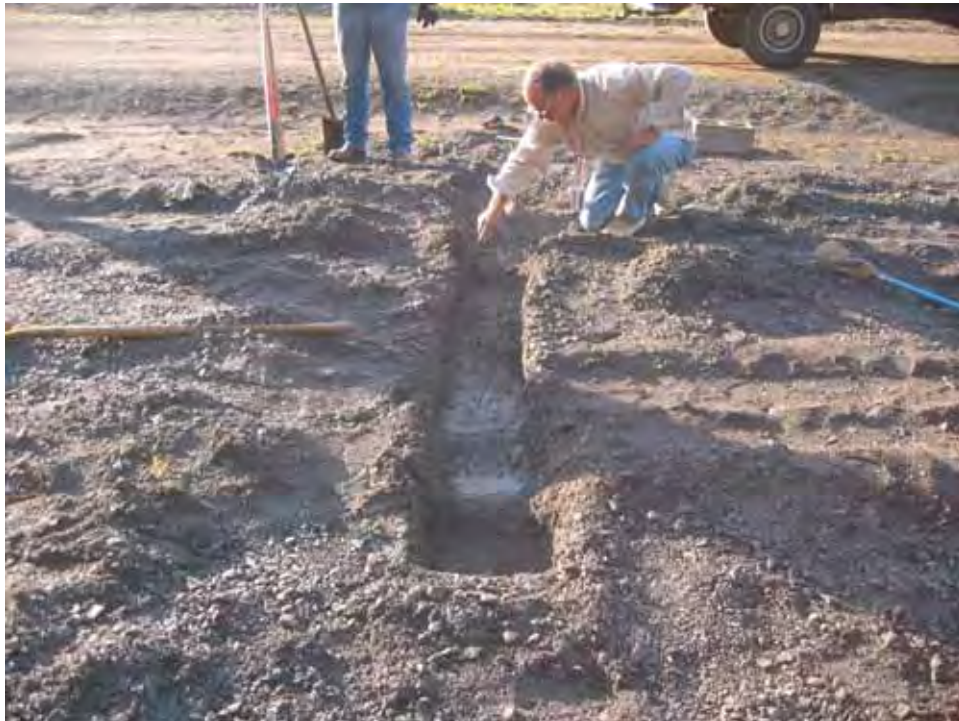
Photo 4. Wet subgrade under Item 7 (LST) surface aggregate
