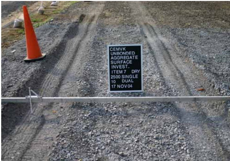
Photo C94. Item 7 (LST), dry lane, new construction test section, 10 passes with dump truck
