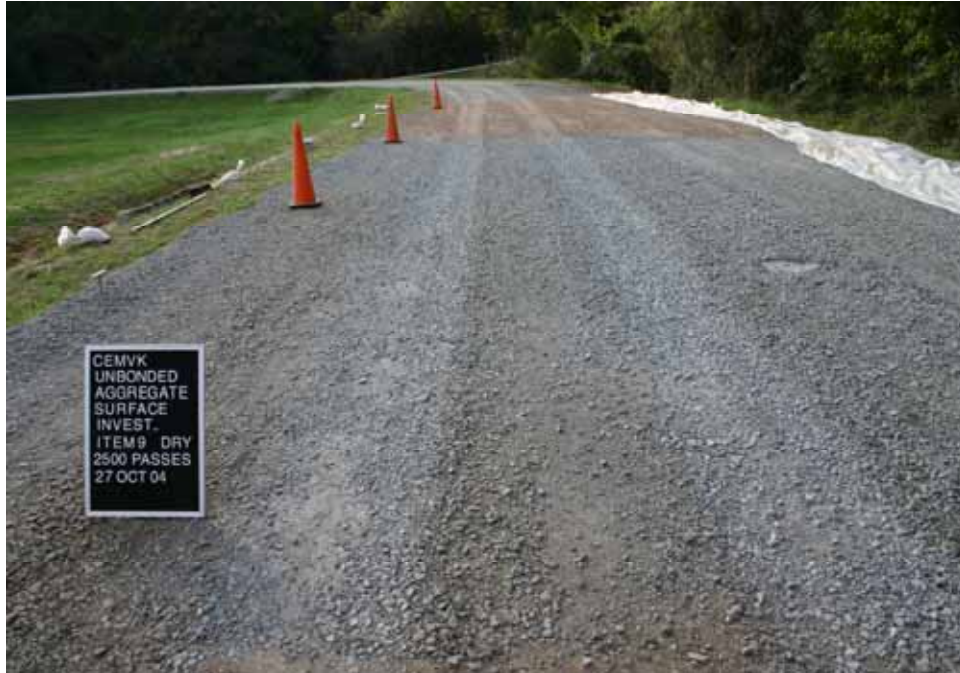
Photo C87. Item 9 (IGN), dry lane, new construction test section, 2500 passes with pickup truck
