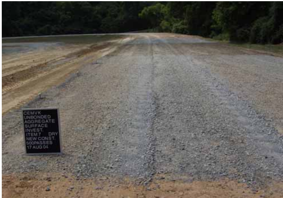
Photo C73. Item 7 (LST), dry lane, new construction test section, 500 passes with pickup truck
