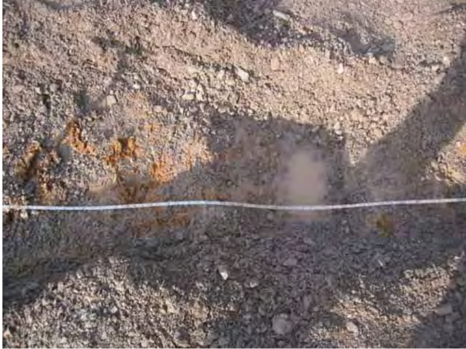
Photo 5. Subgrade pumping up into surface aggregate for Item 7 (LST)
