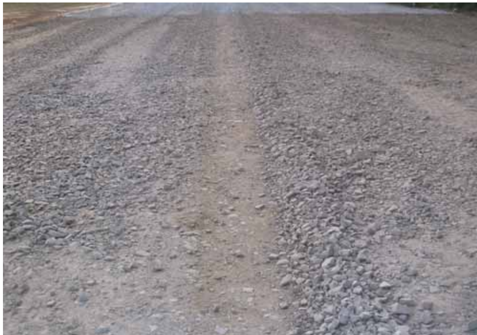
Photo C76. Item 8 (SST), dry lane, new construction test section, 500 passes with pickup truck
