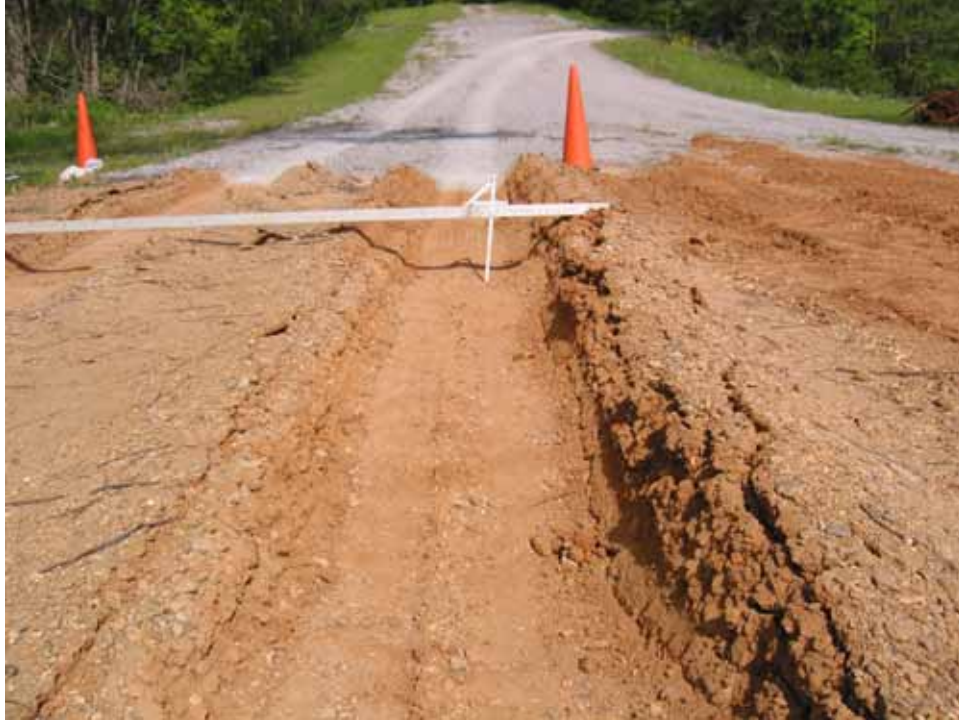
Photo C105. Item 6 (SCG), wet lane, new construction test section, 25 passes with CBR truck
