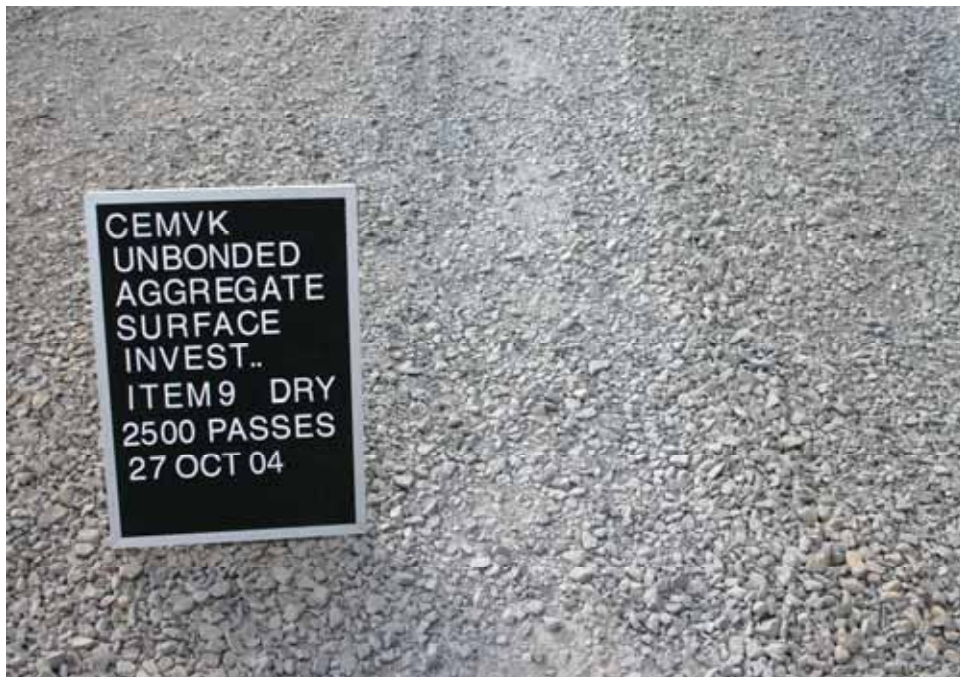
Photo C88. Item 9 (IGN), dry lane, new construction test section, 2500 passes with pickup truck
