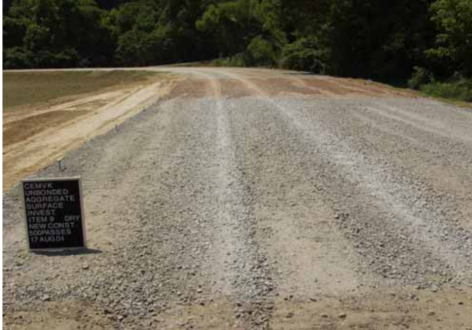
Photo C77. Item 9 (IGN), dry lane, new construction test section, 500 passes with pickup truck
