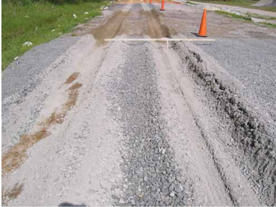
Photo C111. Item 9 (IGN), wet lane, new construction test section, 25 passes with CBR truck
