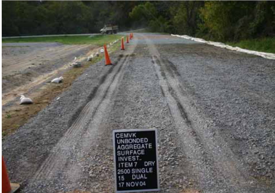
Photo C95. Item 7 (LST), dry lane, new construction test section, 15 passes with dump truck
