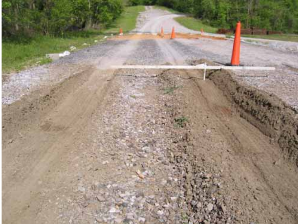
Photo C109. Item 8 (SST), wet lane, new construction test section, 25 passes with CBR truck
