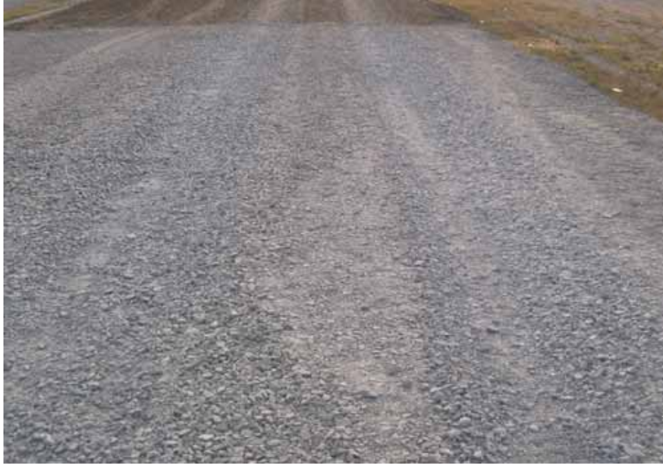
Photo C7. Item 4 (IGN), dry lane, maintenance test section, 500 passes with pickup truck
