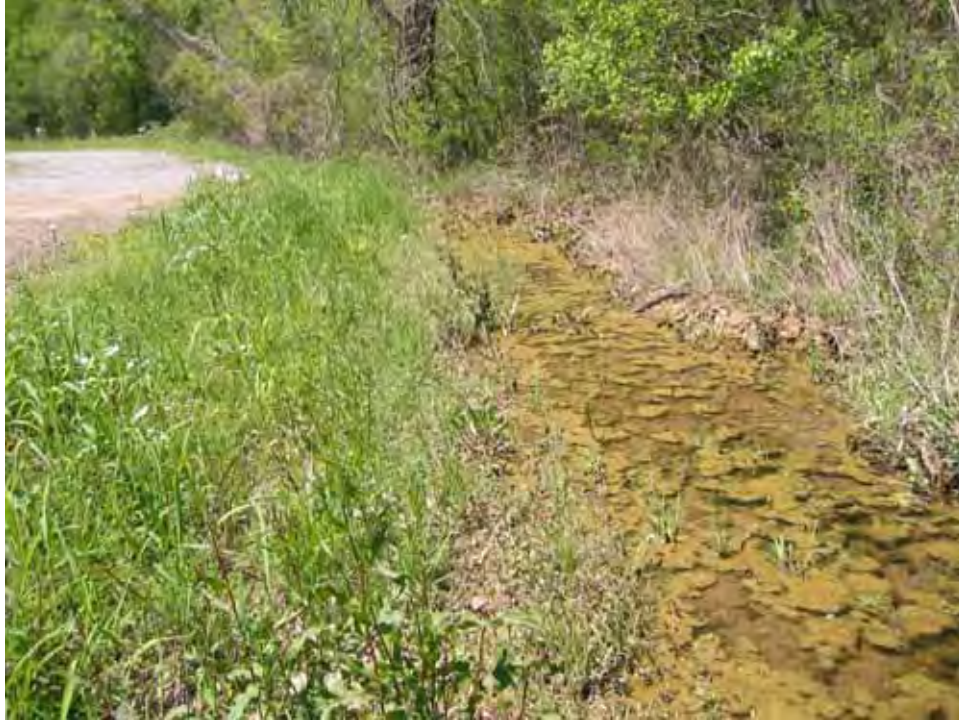
Photo 3. Ponding of water along outside shoulder
