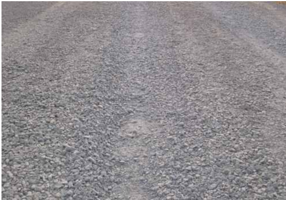
Photo C8. Item 4 (IGN), dry lane, maintenance test section, 500 passes with pickup truck
