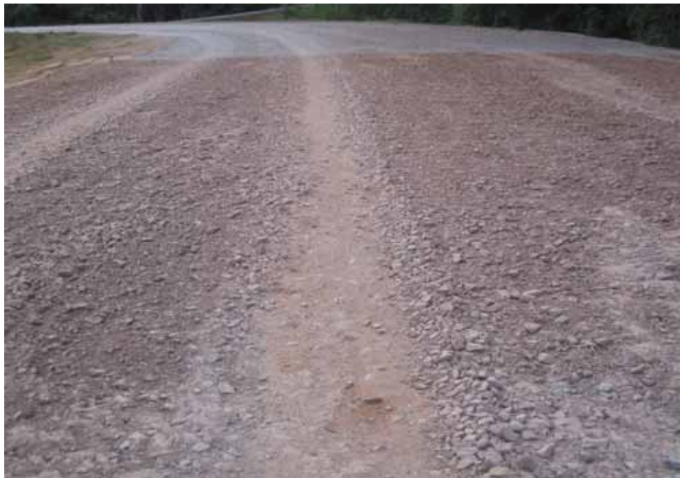
Photo C80. Item 10 (SSB), dry lane, new construction test section, 500 passes with pickup truck
