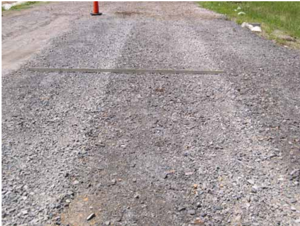
Photo C98. Item 7 (LST), wet lane, new construction test section, 25 passes with pickup truck
