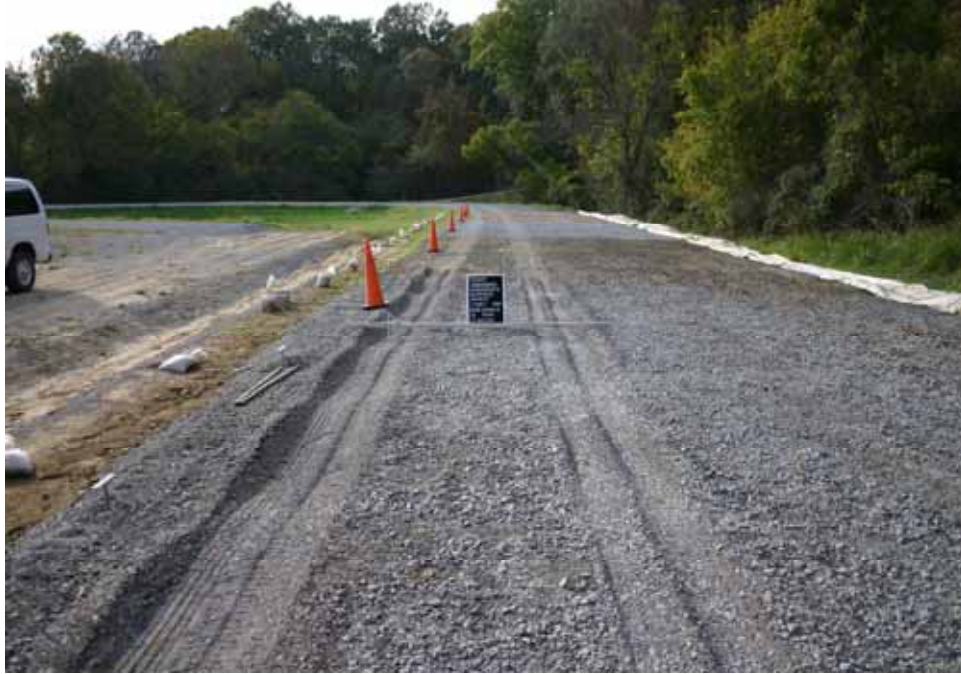
Photo C93. Item 7 (LST), dry lane, new construction test section, 10 passes with dump truck
