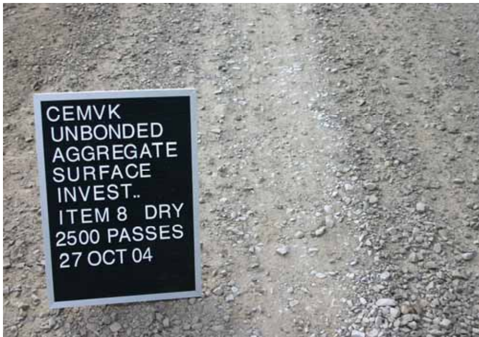
Photo C86. Item 8 (SST), dry lane, new construction test section, 2500 passes with pickup truck
