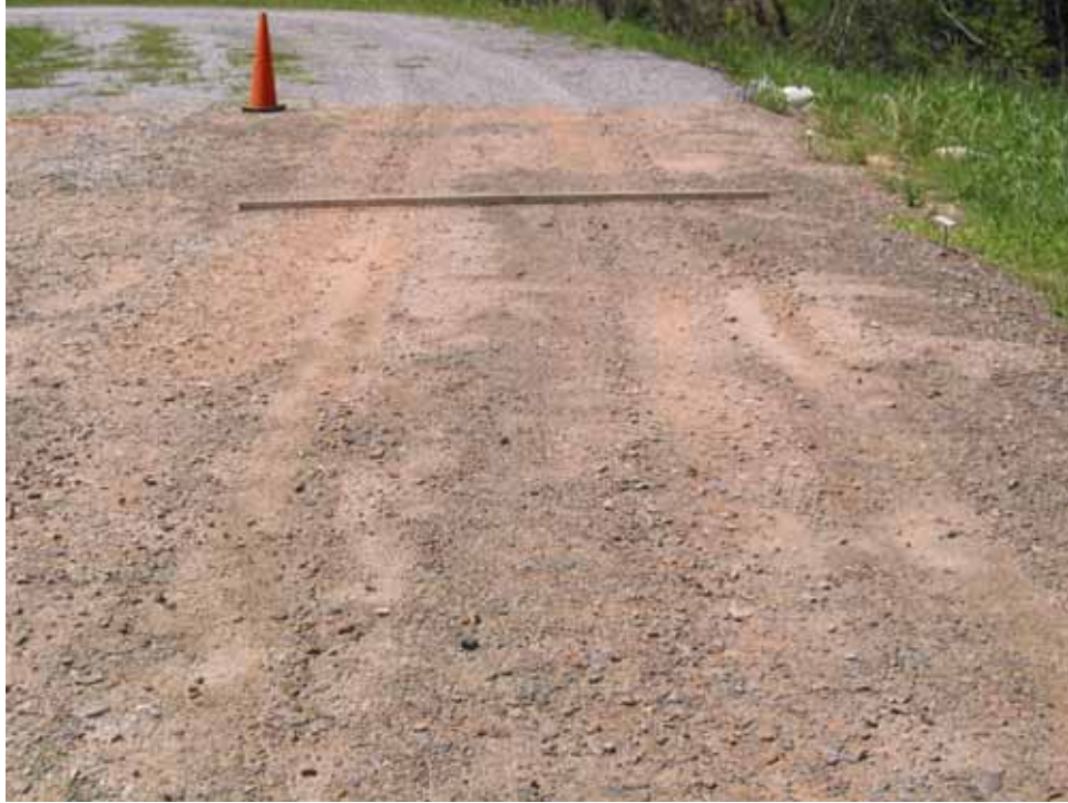
Photo C103. Item 10 (SSB), wet lane, new construction test section, 25 passes with pickup truck
