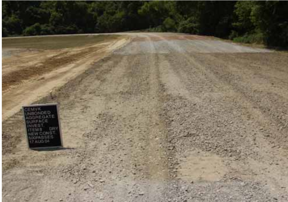
Photo C75. Item 8 (SST), dry lane, new construction test section, 500 passes with pickup truck
