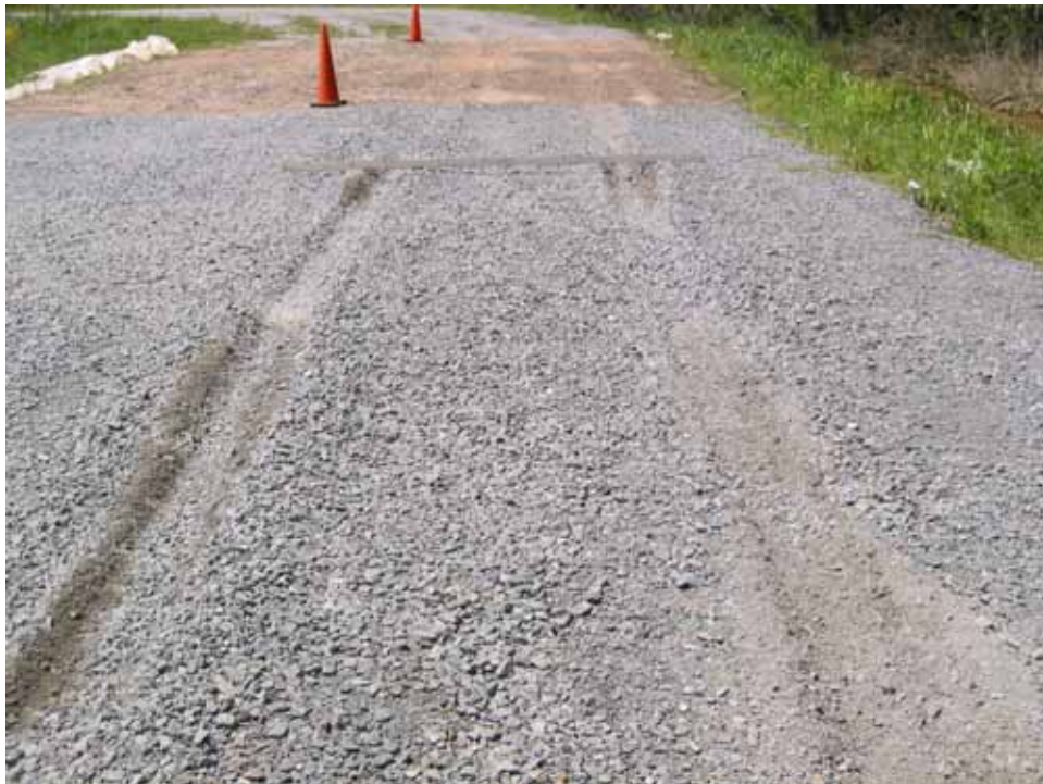
Photo C100. Item 9 (IGN), wet lane, new construction test section, 25 passes with pickup truck
