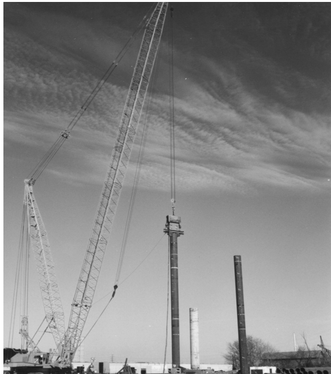
Figure 44. Pile driving with a submersible vibratory hammer, New Orleans IHNC pile test project
