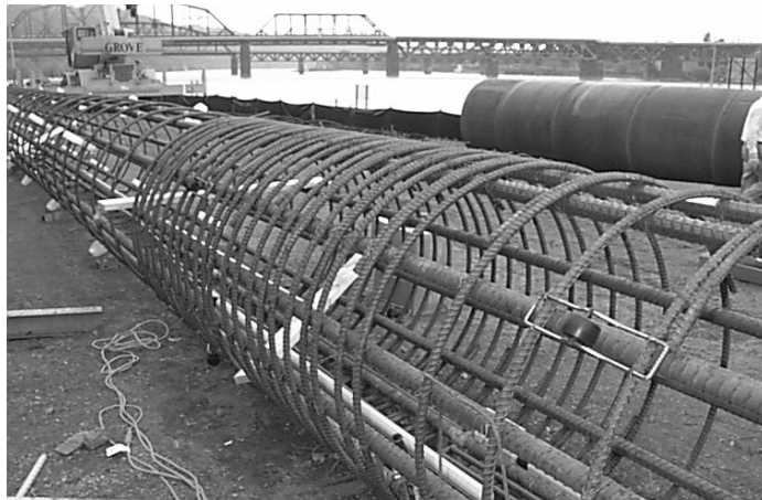
Figure 42. Reinforcing cage for the drilled shaft load test prior to project construction at Braddock Locks and Dam 2
